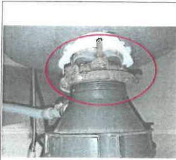
Connection bracket was significantly rusted
