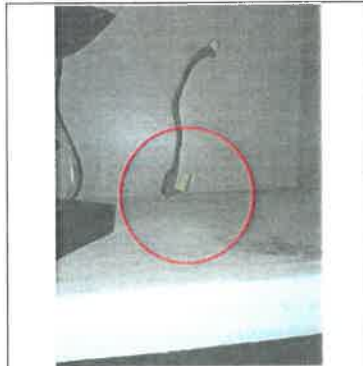
Loose "live" wiring above downstairs kitchen sink
