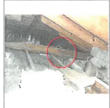
Spliced wiring on the northwest side of the attic
