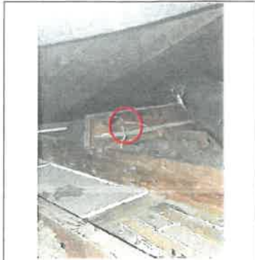
Wire on northeast side of attic was "nicked"
