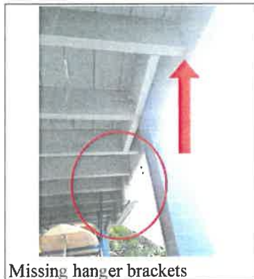
Missing hanger brackets
