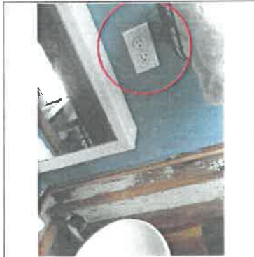
Downstairs bathroom outlet above sink not on GFCI
