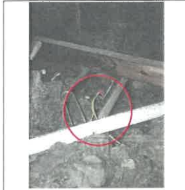
Spliced wiring on northwest side of attic
