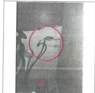
Wiring not in junction box, unit should have designated outlet
