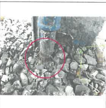
Hose bib supply line on front side of home is rusted at ground level
