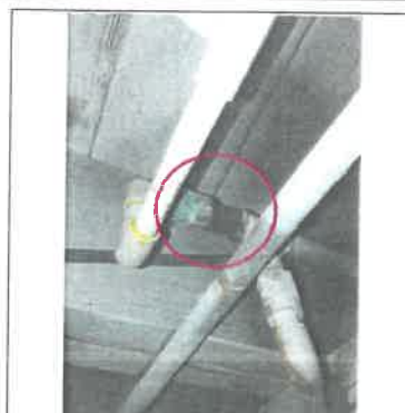
Water supply line above water heater is moderately rusted
