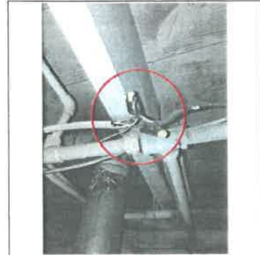
Wiring above water heater spliced and not in a box
