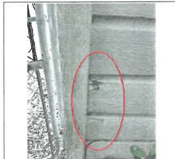
NW corner had deterioration
