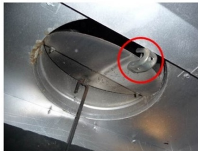
HEI file photo showing c-clamp in metal fireplace
