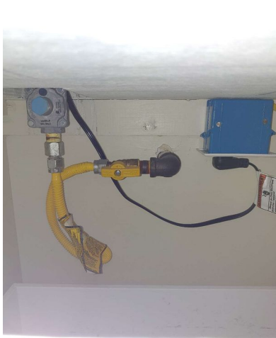
Gas shut off valve in cabinet below cooktop
