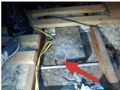
No vent pipe installed
