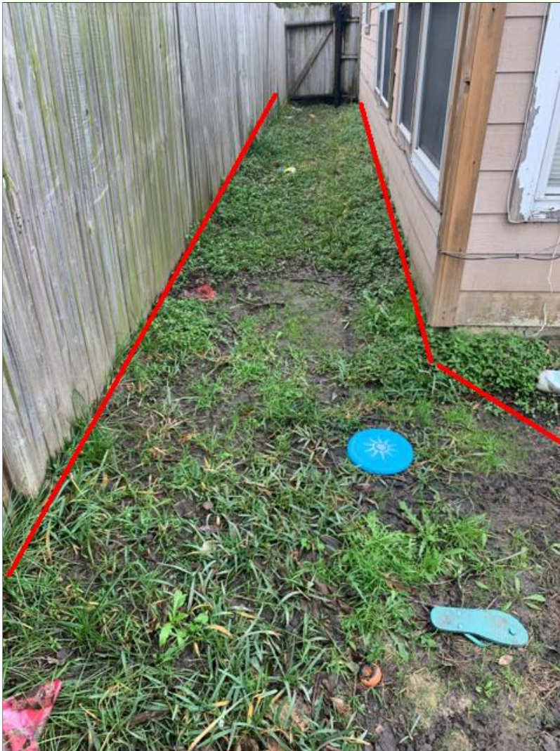
B. Photo 1(Picture) Drainage swales at rear and sides of home appears to have low spots. Water will most likely pool in the drainage swales and not drain normally towards the street. Possible remedies might include the installation of catch basins, or French Drains at low spots connected to underground drain pipe to the street.
