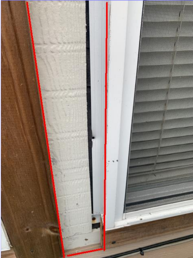
H. Photo 2(Picture) One of the windows is missing the trim board and is not sealed.
