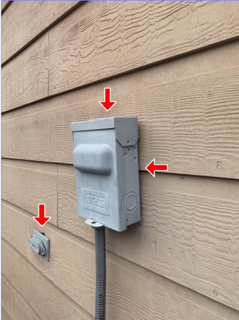
E. Photo 18(Picture) Exterior electrical wall panels, outlets and fixtures need to be sealed at the wall.
