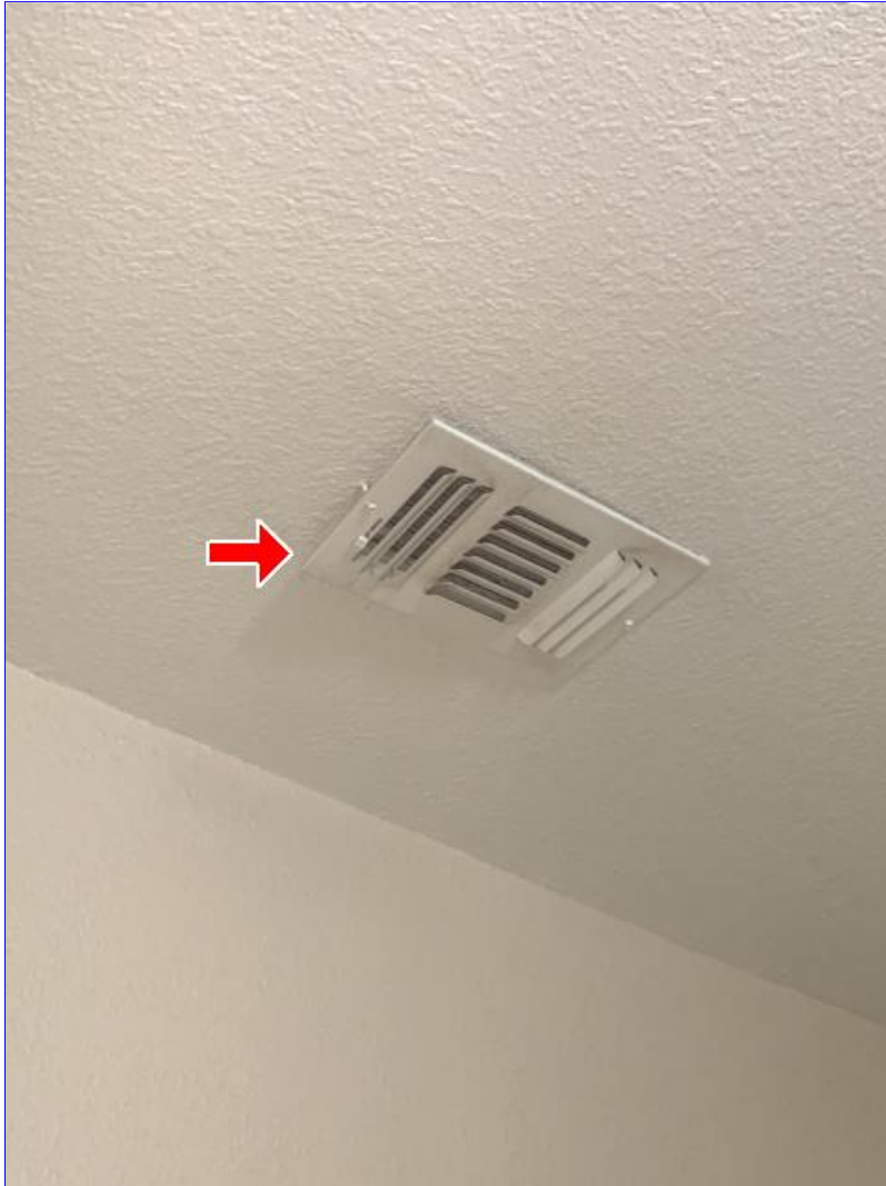
C. Photo 1(Picture) In the front right bedroom, the supply grill is loose at the ceiling.
