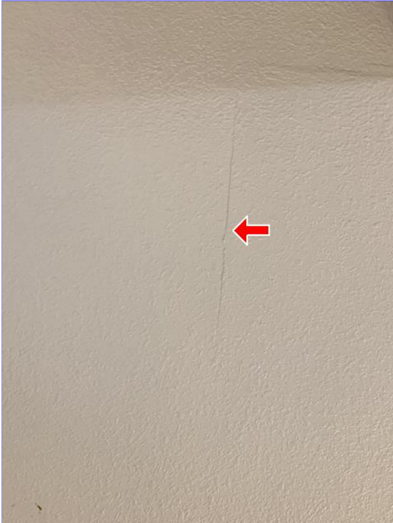
F. Photo 3(Picture) Drywall tape joint cracks and/or nail pops were observed around the home. These are cosmetic in nature, and can be repaired as needed.
