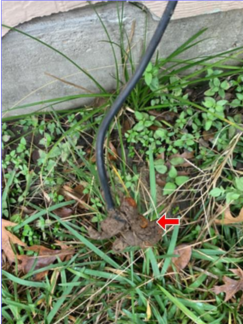
A. Photo 2(Picture) The system ground wire, is loose from the ground clamp or the ground clamp, is loose on the ground rod (electrode).
