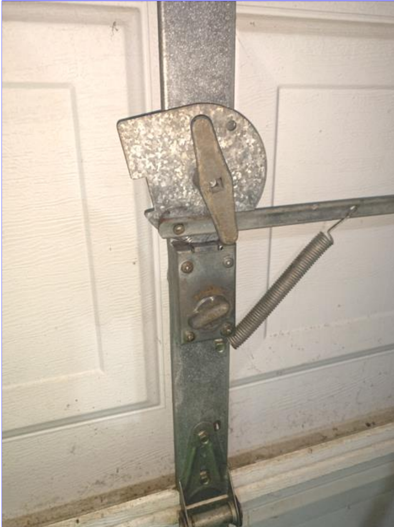
G. Photo 12(Picture) The garage door lock is inoperable.
