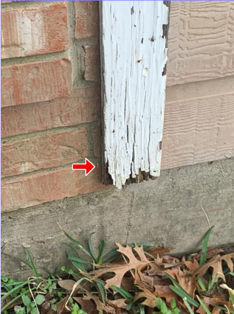
E. Photo 9(Picture) Areas of wood rot were observed on the trim boards.
