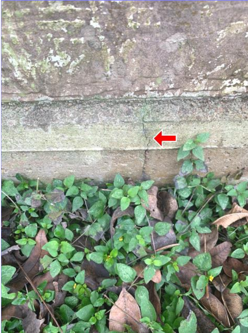
A. Photo 1(Picture) There is some slab edge cracking. There is little to no deflection across the crack. This type of flexural crack is generally the result of seasonal variations in soil moisture causing the soils to shrink and/or swell exerting pressure on the foundation.
