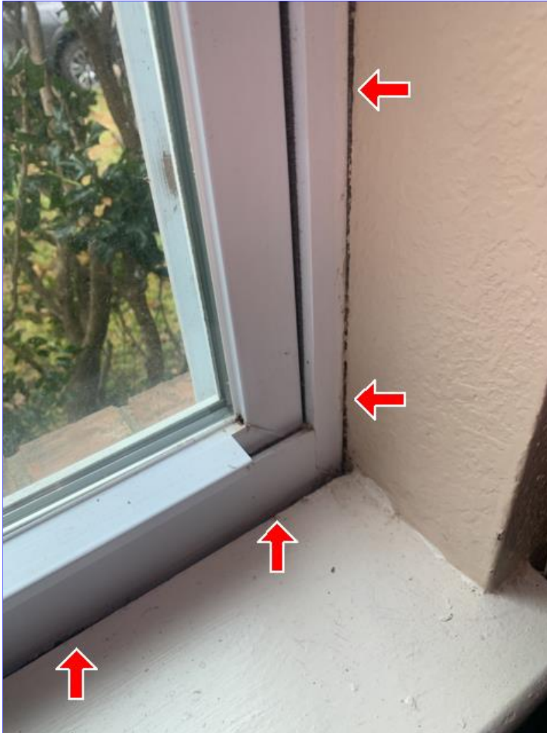
E. Photo 6(Picture) In the front right bedroom, the window needs to be sealed at the perimeter.
