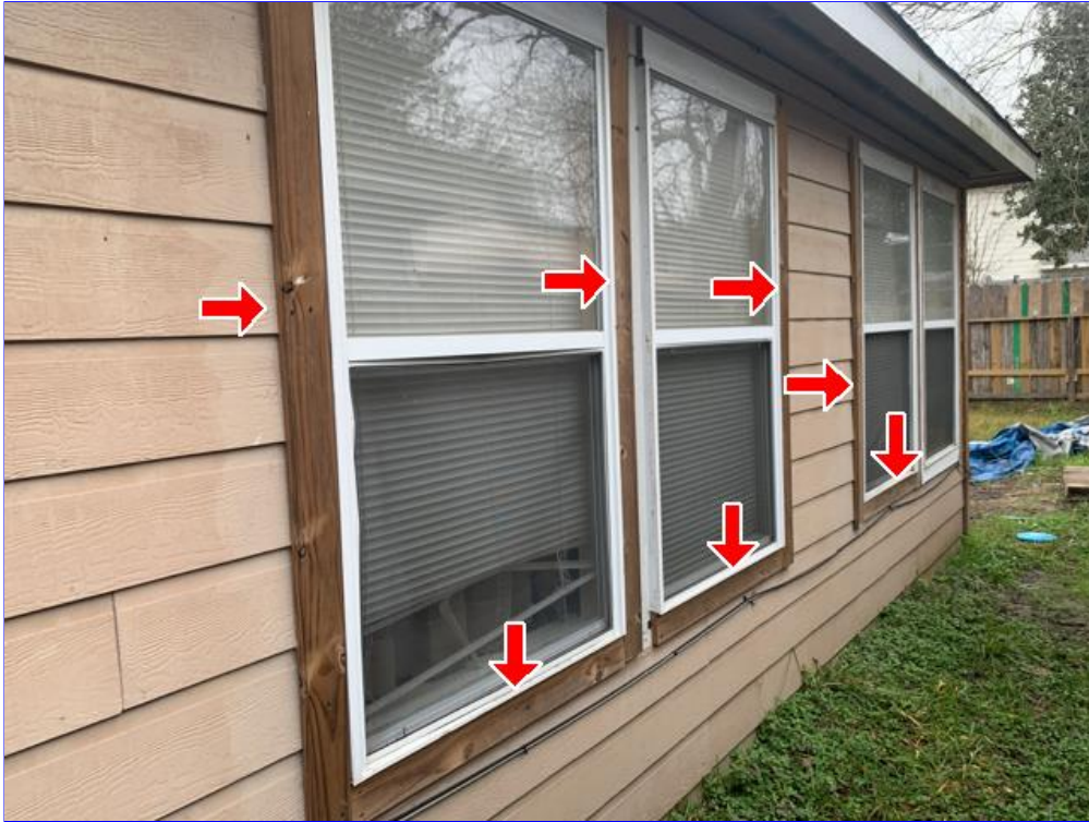
E. Photo 14(Picture) Areas of the home was observed to have bare wood. Recommend priming and painting.
