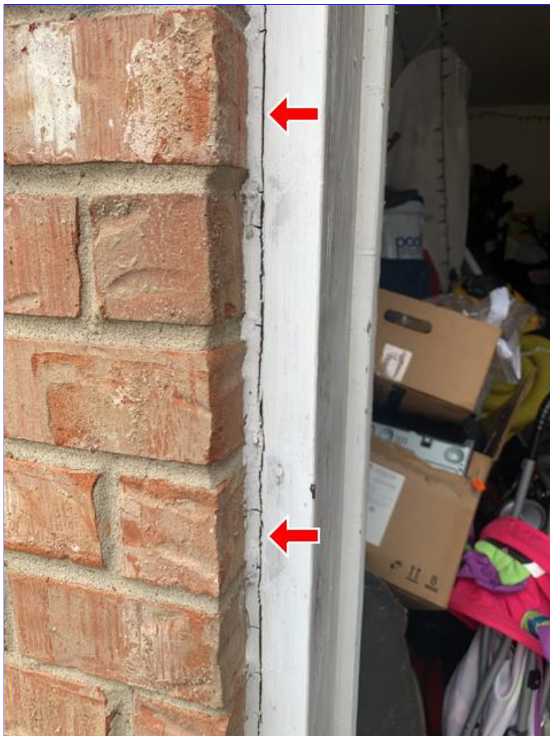
E. Photo 4(Picture) Areas were observed, where the brick, siding and/or trim needs to be resealed.
