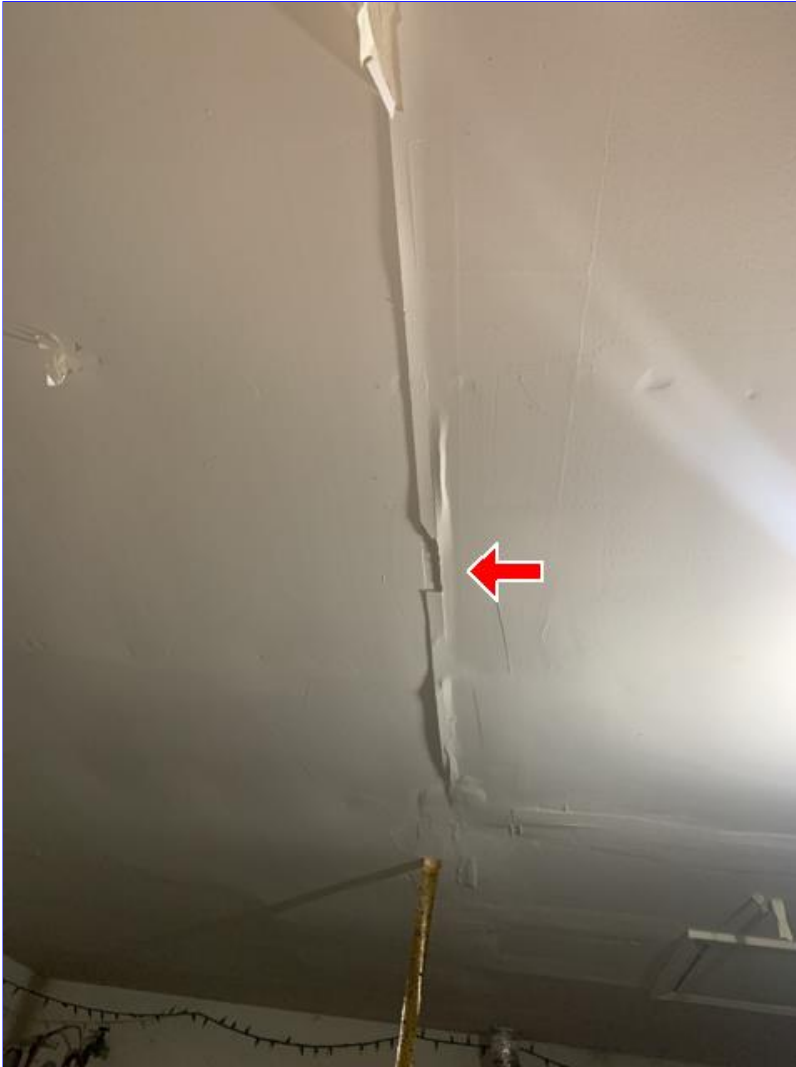
F. Photo 5(Picture) Drywall tape joint cracks and/or nail pops were observed around the home. These are cosmetic in nature, and can be repaired as needed.
