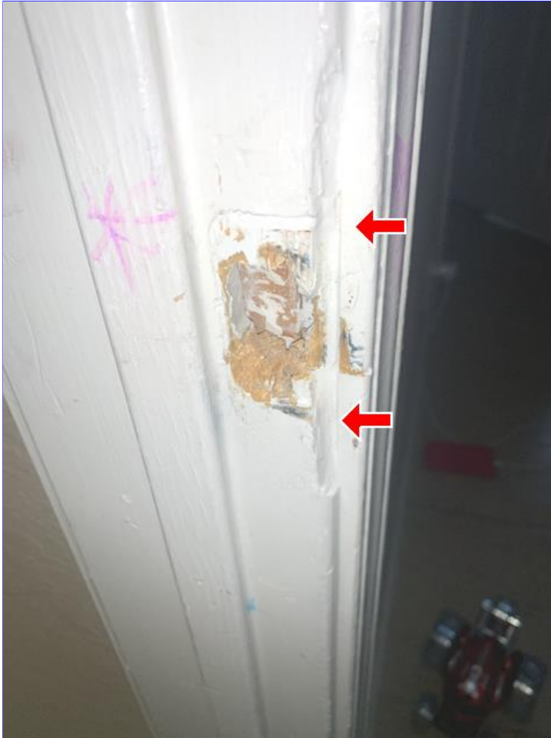
G. Photo 4(Picture) Damage was observed on the third right bedroom door frame.
