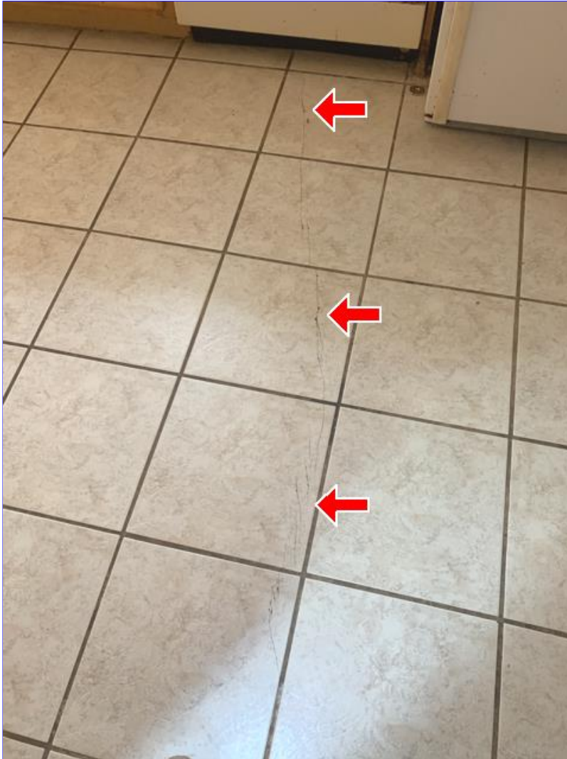
F. Photo 6(Picture) Floor tile cracks were observed throughout.
