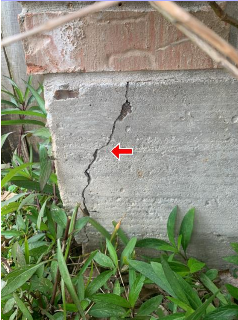
A. Photo 3(Picture) Typical corner "pops" observed at foundation corners. This condition is cosmetic in nature and not structurally significant.
