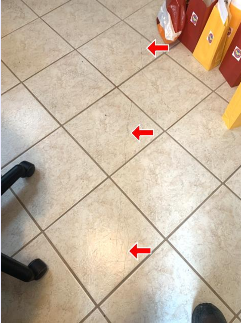
F. Photo 9(Picture) Floor tile cracks were observed throughout.
