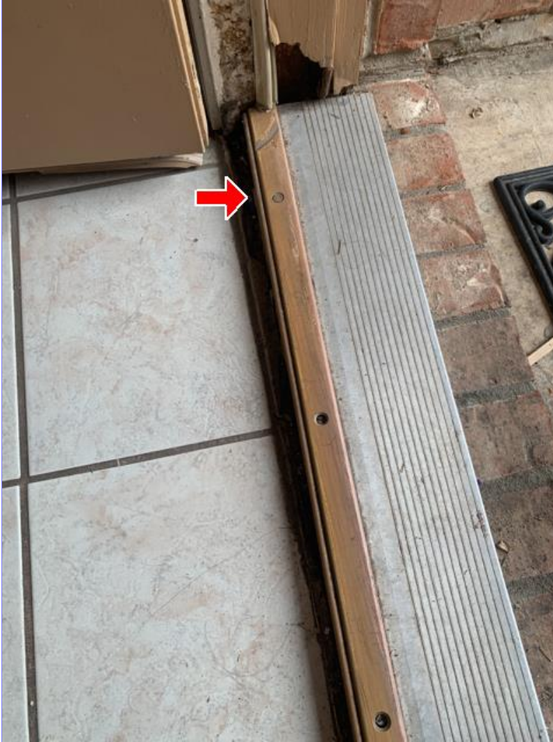
G. Photo 7(Picture) The front door frame is damaged, has wood rot, the threshold is loose and the bottom weatherstripping is loose.
