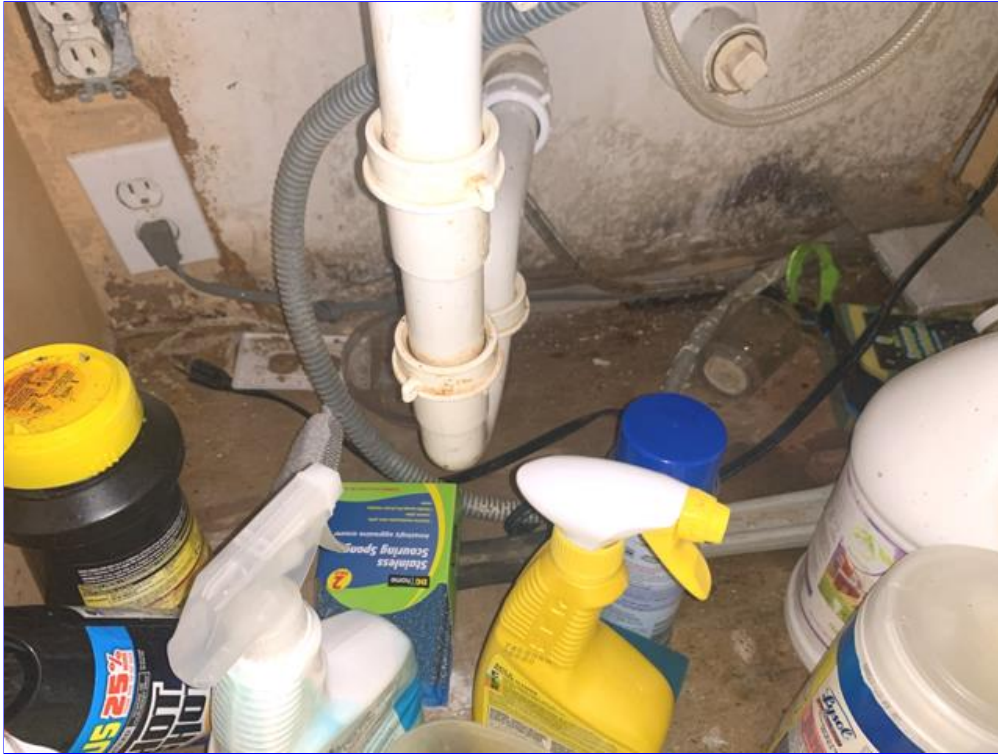
L. Photo 2(Picture) Areas of previous water damage were observed near the sink on the kitchen countertop and under the sink inside the cabinet.
