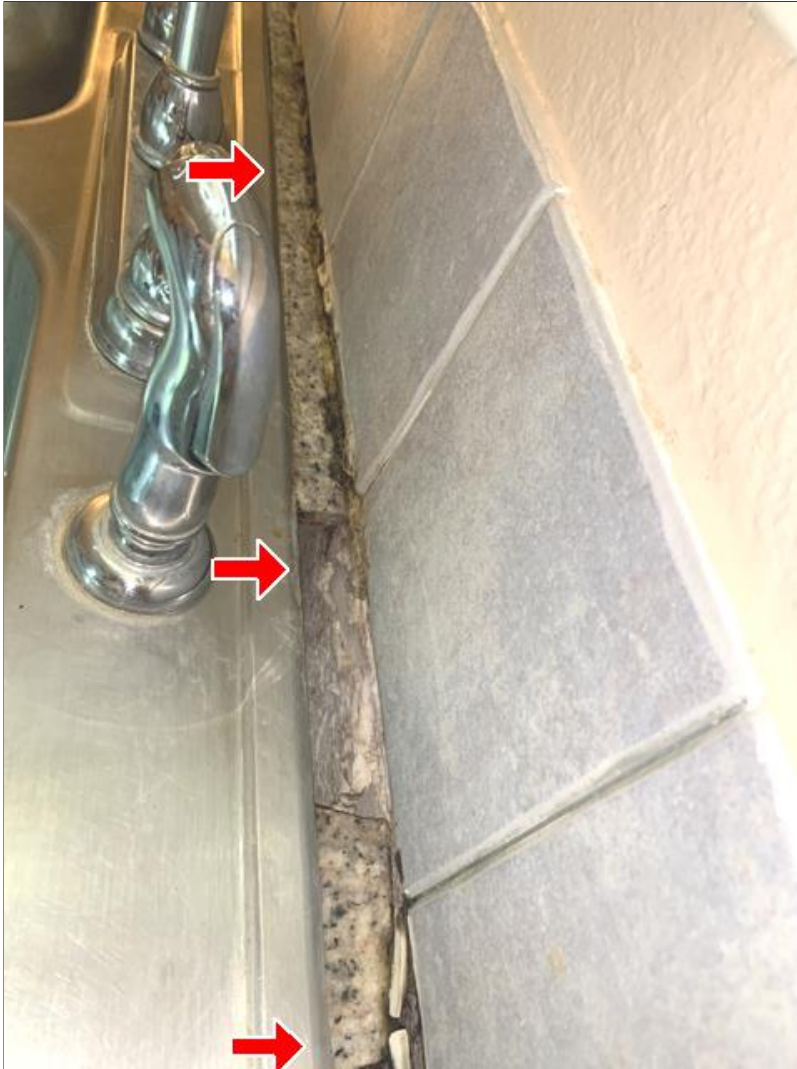
L. Photo 1(Picture) Areas of previous water damage were observed near the sink on the kitchen countertop and under the sink inside the cabinet.
