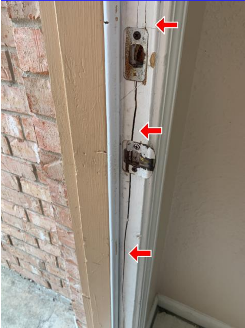
G. Photo 5(Picture) The front door frame is damaged, has wood rot, the threshold is loose and the bottom weatherstripping is loose.
