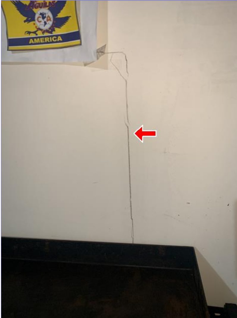
E. Photo 8(Picture) Drywall tape joint cracks and/or nail pops were observed around the home. These are cosmetic in nature, and can be repaired as needed.
