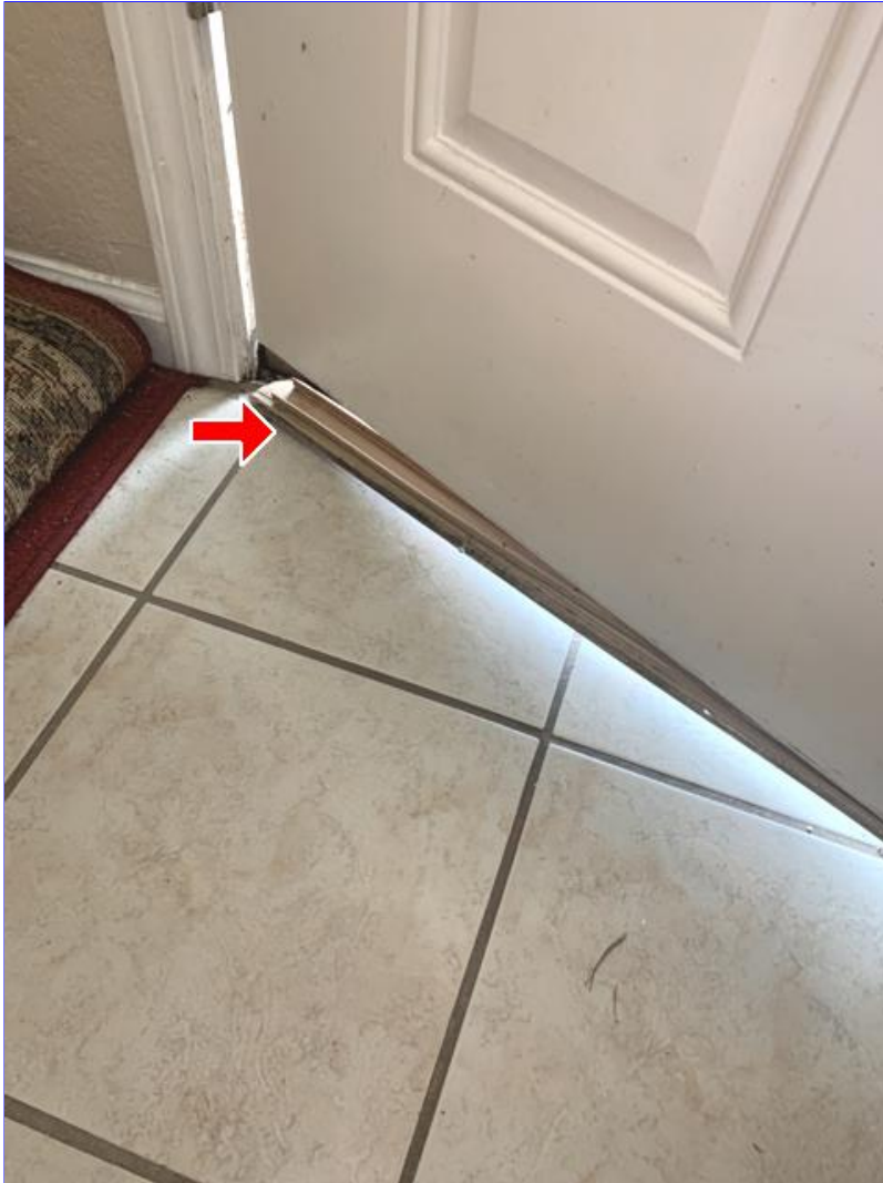
G. Photo 8(Picture) The front door frame is damaged, has wood rot, the threshold is loose and the bottom weatherstripping is loose.
