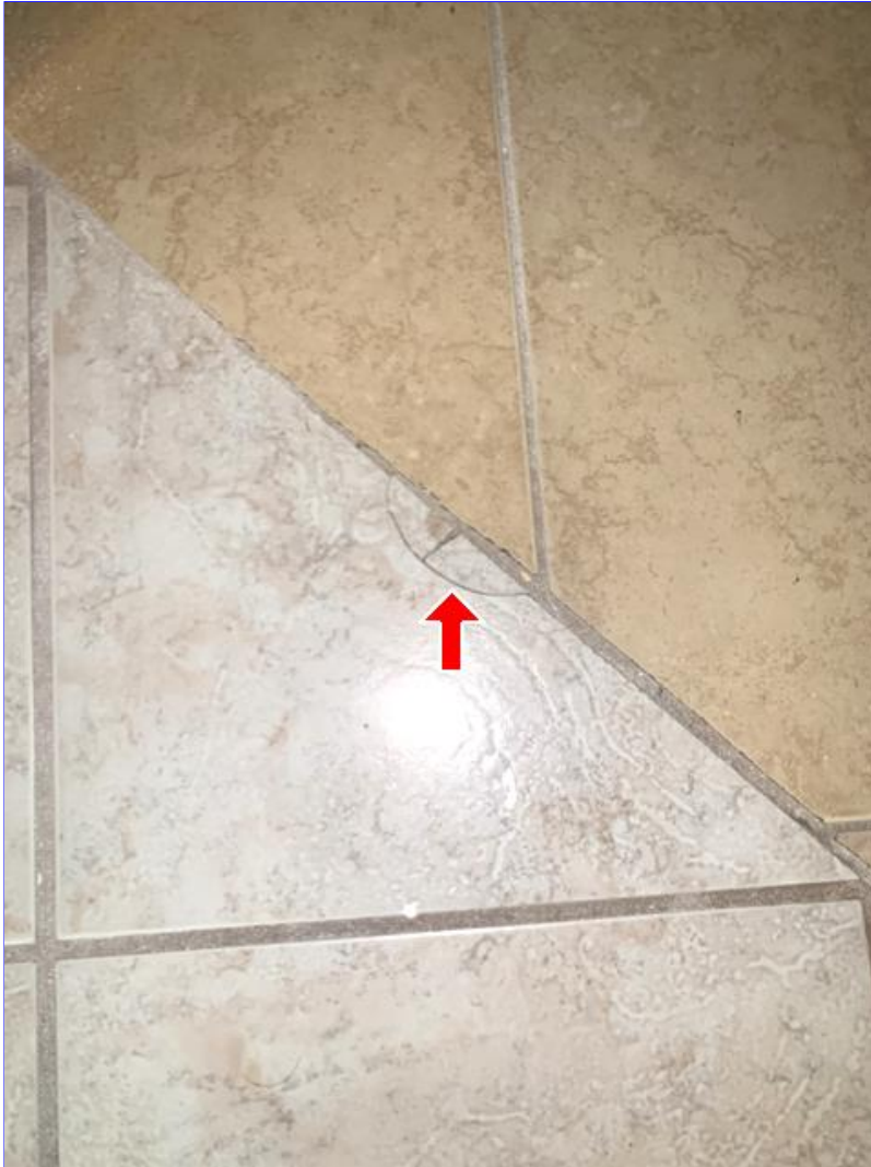
F. Photo 10(Picture) In the master bathroom, a cracked tile was observed near the left hand closet.
