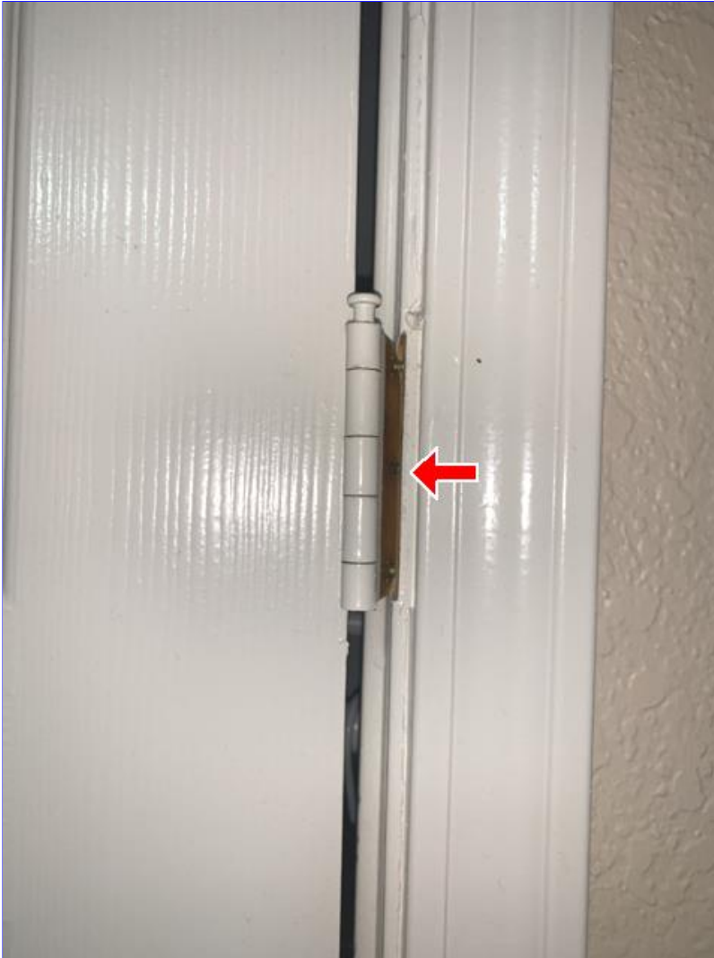
G. Photo 3(Picture) In the front right bedroom, the closet door hinge is loose at the frame.
