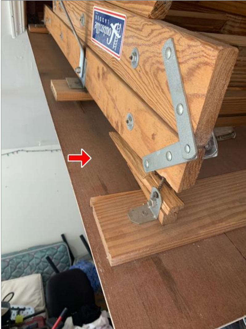
G. Photo 14(Picture) Damage was observed on the attic access ladder.
