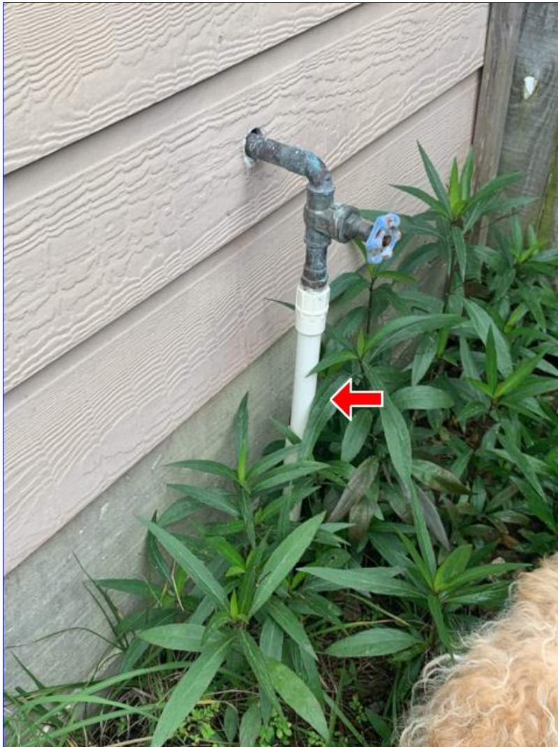
A. Photo 1(Picture) The main water supply line at the exterior, is not properly protected from freezing.
