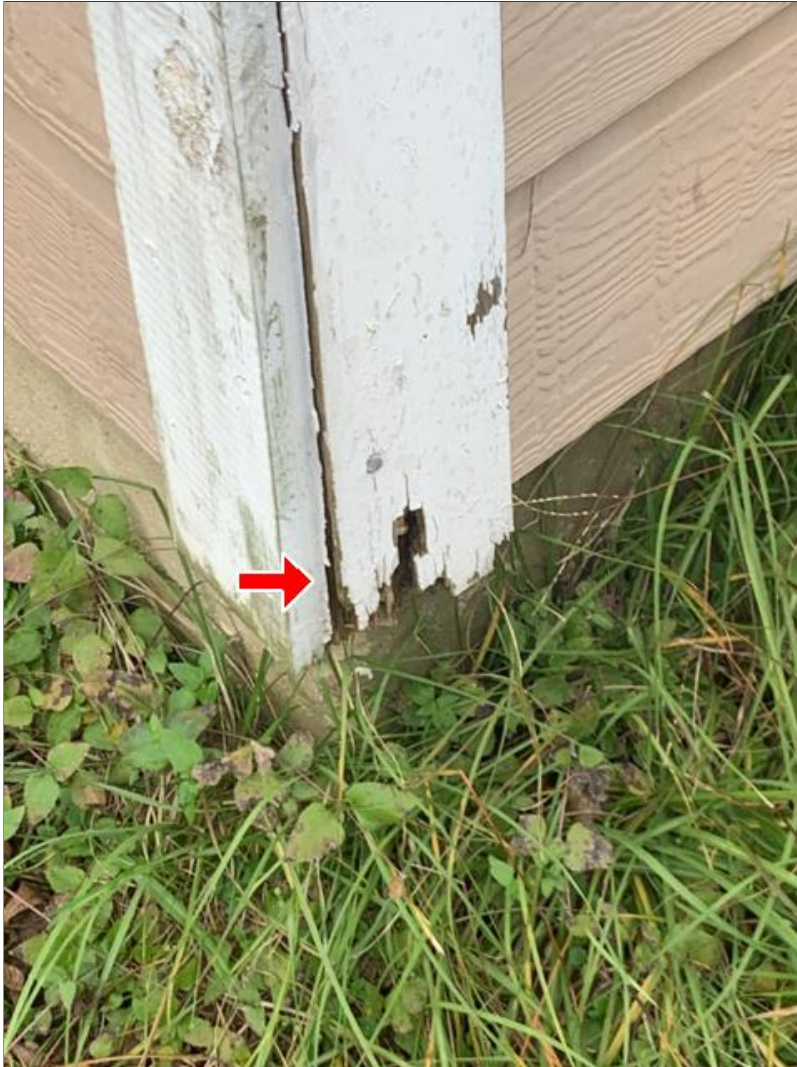
E. Photo 10(Picture) Areas of wood rot were observed on the trim boards.
