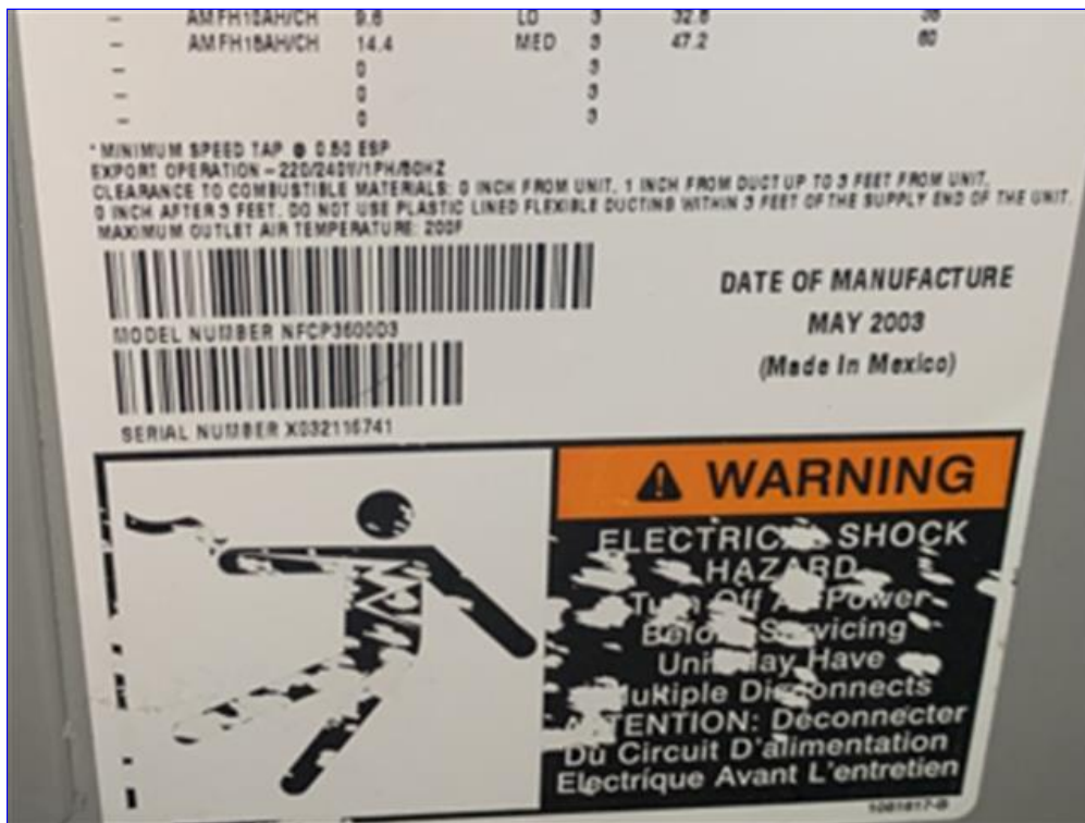
A. Photo 1(Picture) Furnace service tag(s).
