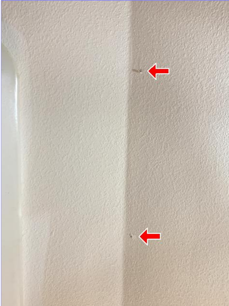
F. Photo 1(Picture) Drywall tape joint cracks and/or nail pops were observed around the home. These are cosmetic in nature, and can be repaired as needed.
