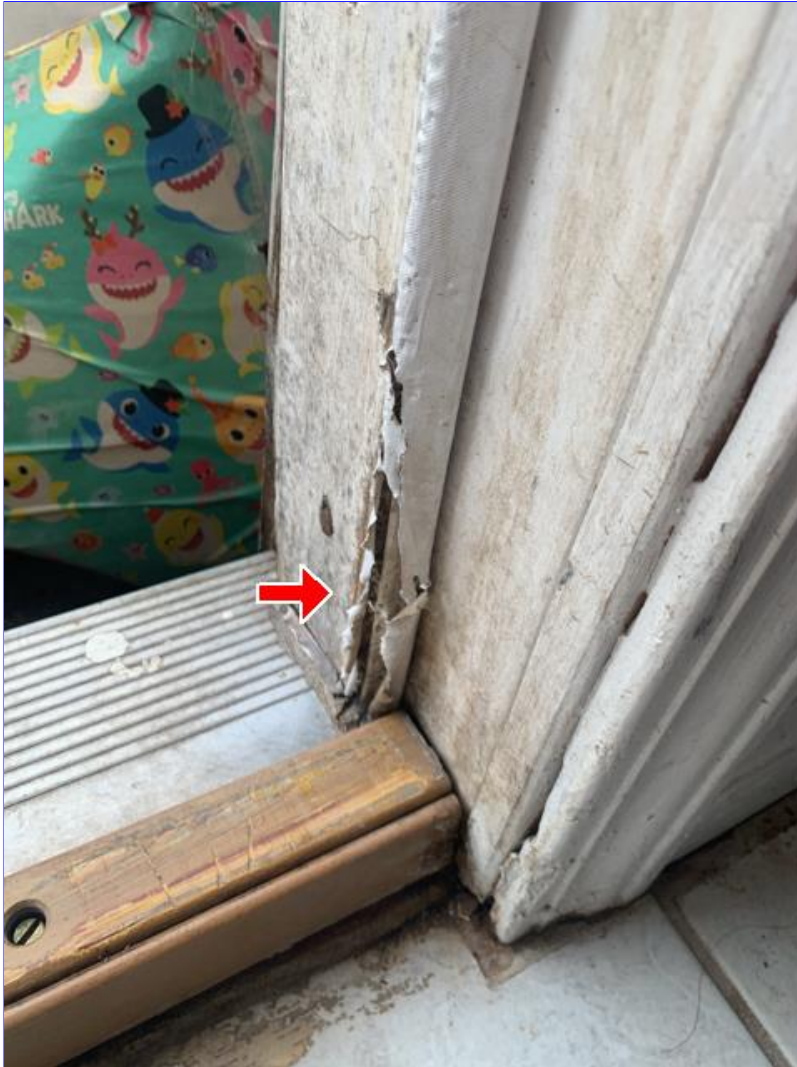
G. Photo 11(Picture) Damage was observed on the back door weatherstripping.
