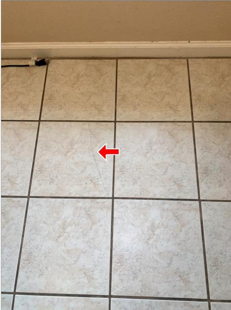
F. Photo 8(Picture) Floor tile cracks were observed throughout.
