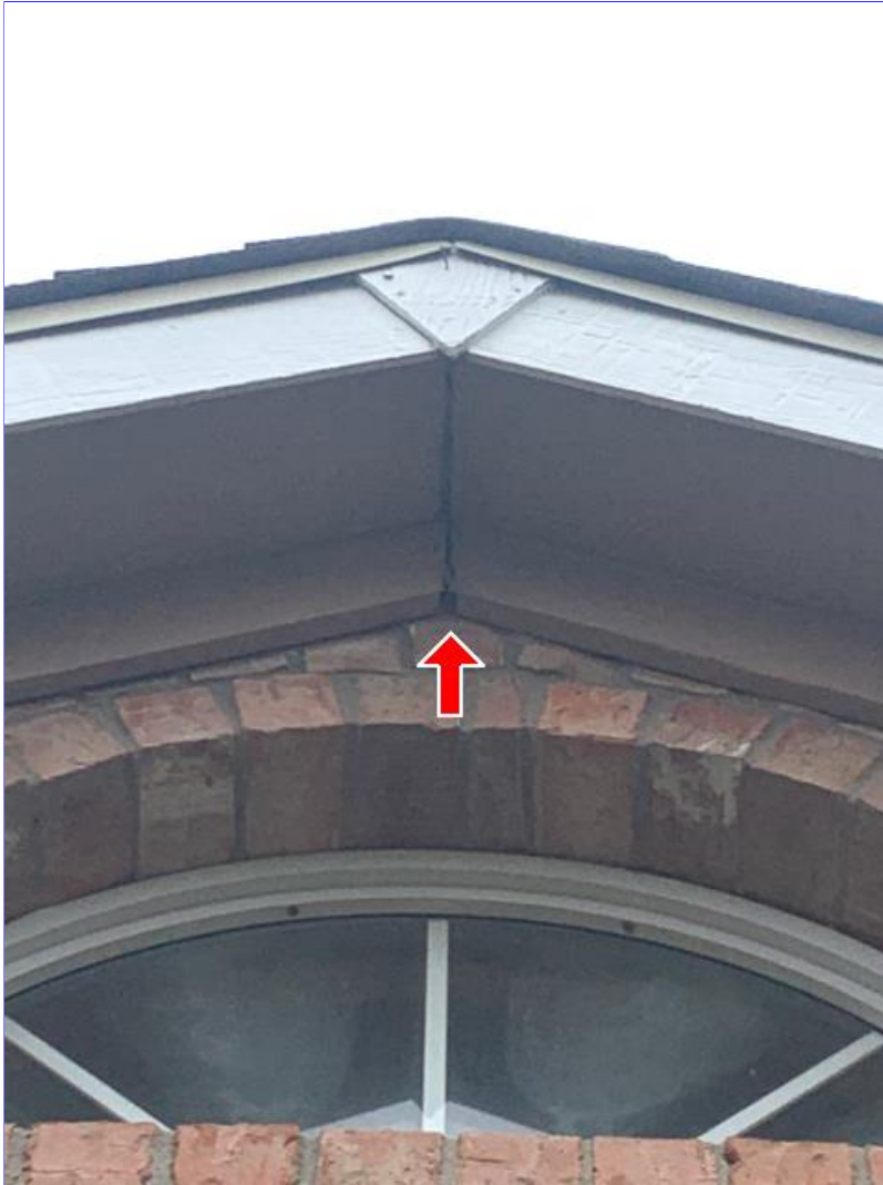
E. Photo 3(Picture) Areas were observed, where the brick, siding and/or trim needs to be resealed.
