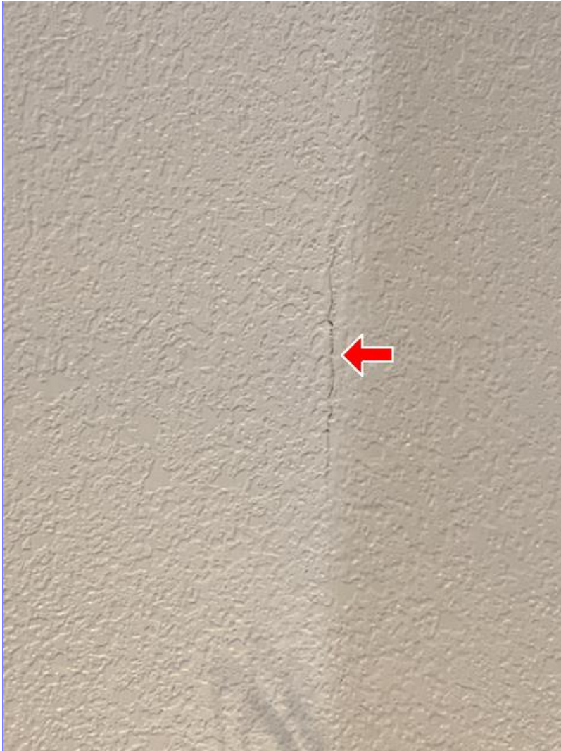
F. Photo 2(Picture) Drywall tape joint cracks and/or nail pops were observed around the home. These are cosmetic in nature, and can be repaired as needed.
