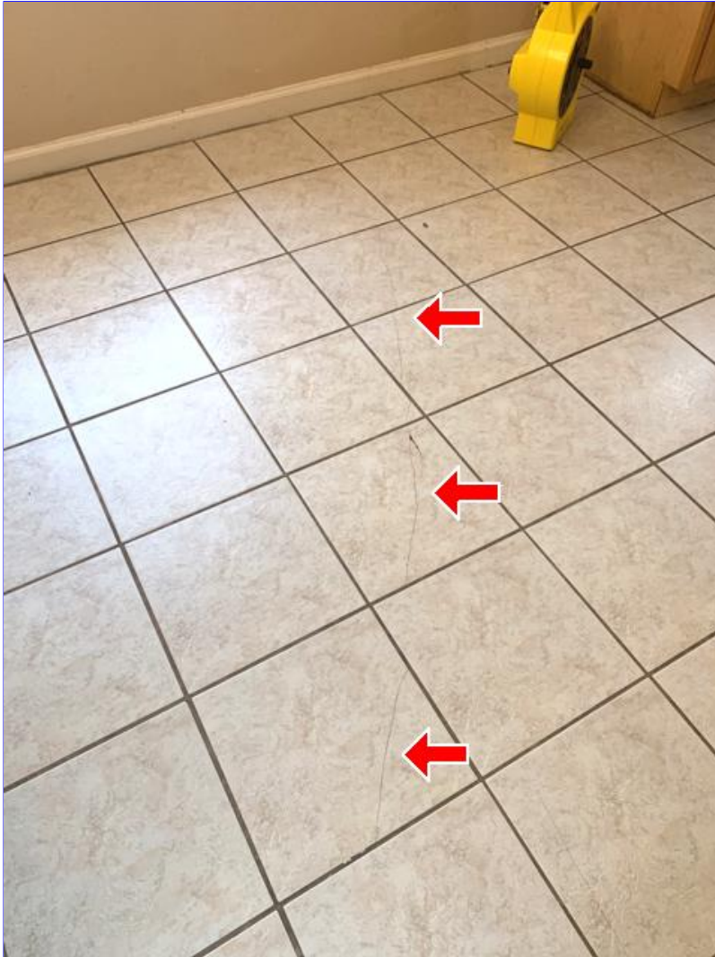
F. Photo 7(Picture) Floor tile cracks were observed throughout.
