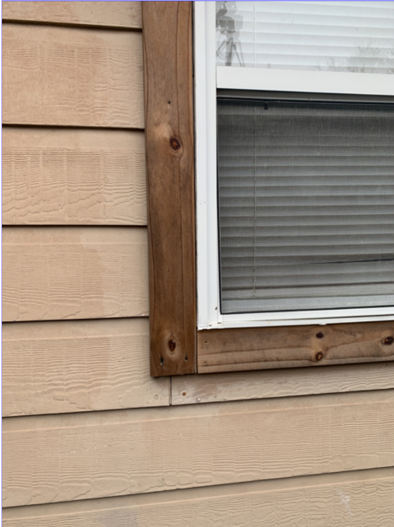
E. Photo 13(Picture) Areas of the home was observed to have bare wood. Recommend priming and painting.
