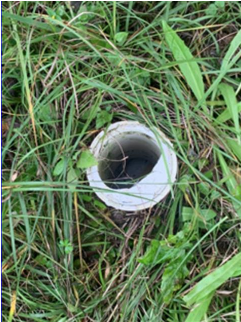
B. Photo 2(Picture) The plumbing clean out cap needs to be replaced.
