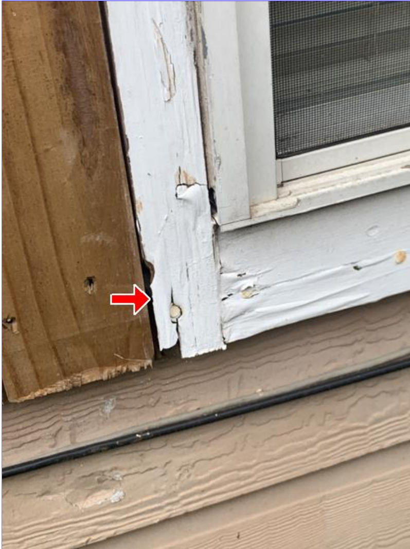
E. Photo 15(Picture) Areas of wood rot were observed on the window trim.
