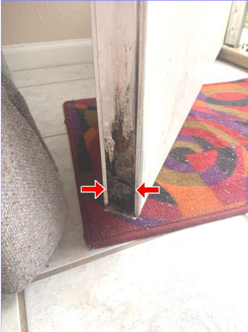
G. Photo 9(Picture) Wood rot was observed on the back door.
