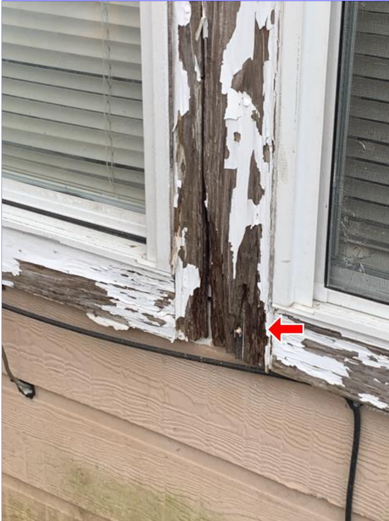
E. Photo 17(Picture) Areas of wood rot were observed on the window trim.
