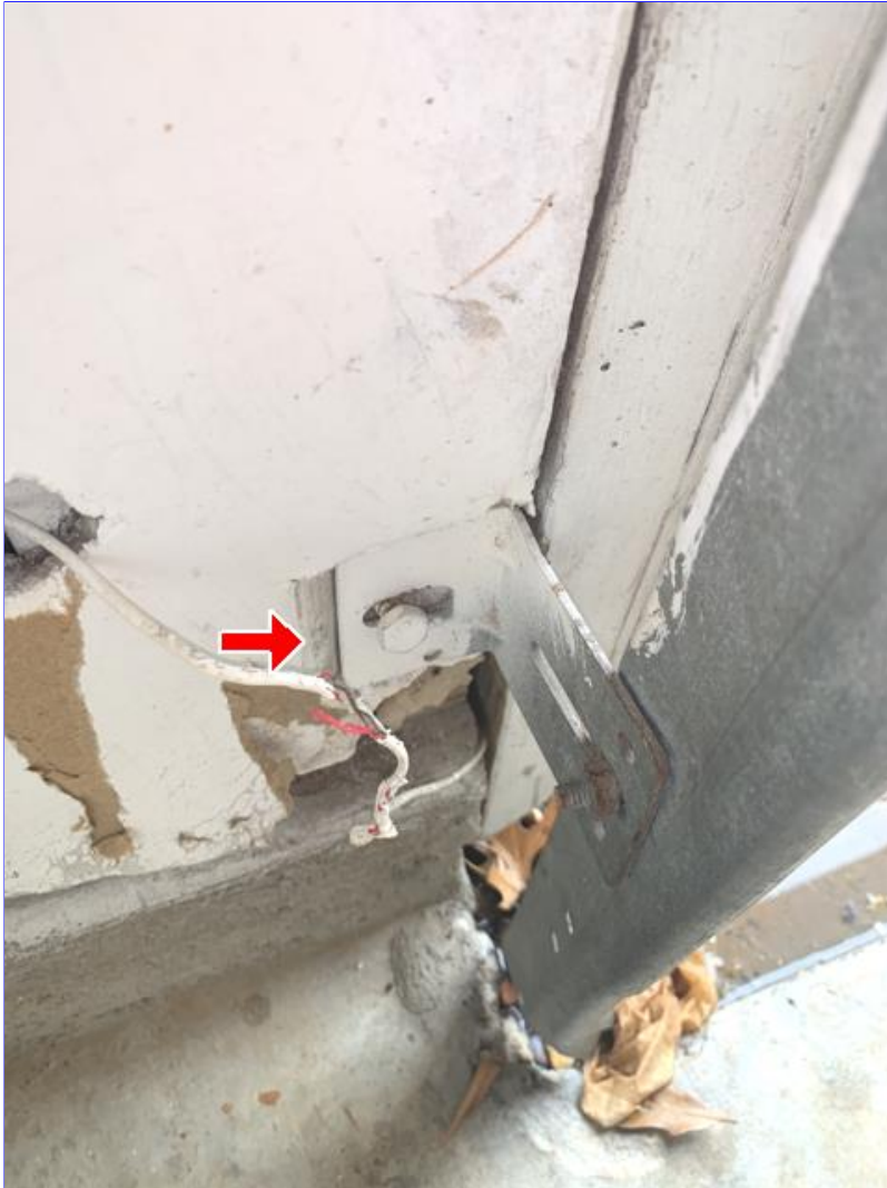
G. Photo 13(Picture) The garage door rail brackets are not properly secured.
