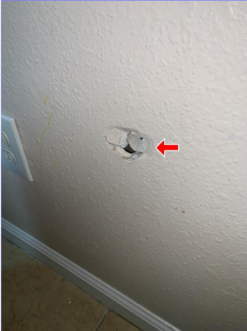
E. Photo 7(Picture) Drywall damage was observed in the second right bedroom
