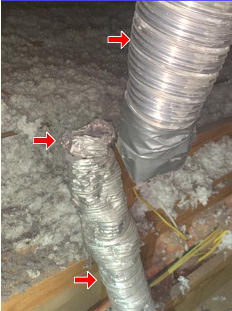
H. Photo 1(Picture) The dryer duct is not a smooth metal lined duct and it is separated in the garage.
