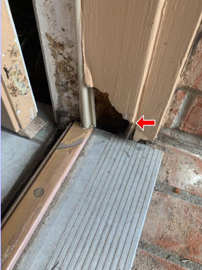
G. Photo 6(Picture) The front door frame is damaged, has wood rot, the threshold is loose and the bottom weatherstripping is loose.
