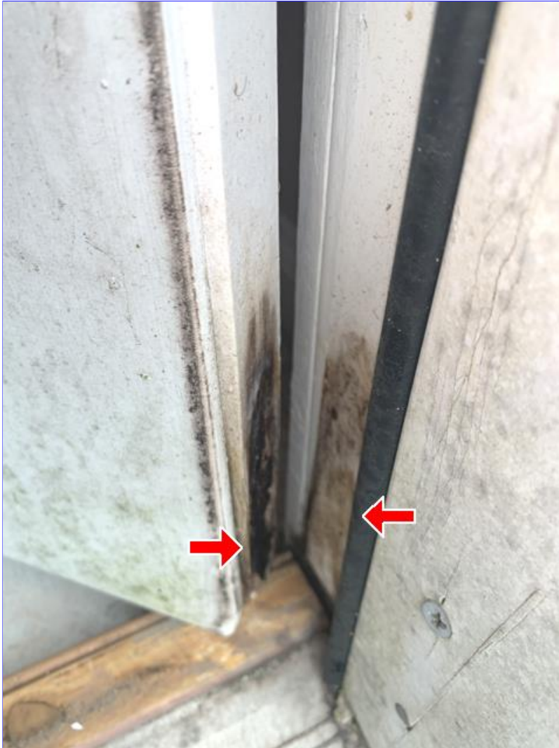
G. Photo 10(Picture) Wood rot was observed on the back door.
