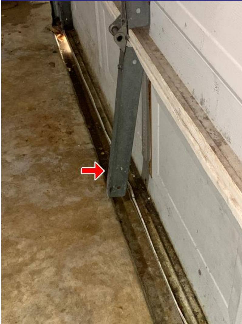
G. Photo 1(Picture) Areas of damage were observed on the garage door.
