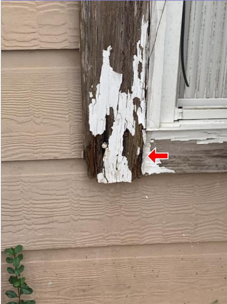
E. Photo 16(Picture) Areas of wood rot were observed on the window trim.
