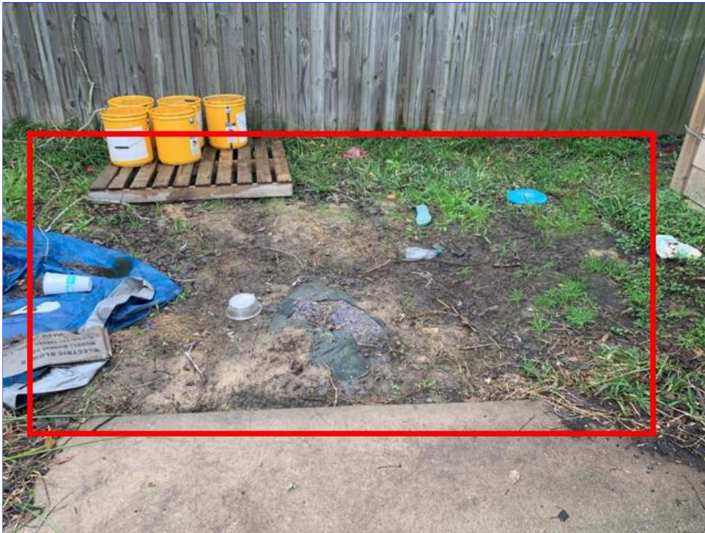
B. Photo 2(Picture) Drainage swales at rear and sides of home appears to have low spots. Water will most likely pool in the drainage swales and not drain normally towards the street. Possible remedies might include the installation of catch basins, or French Drains at low spots connected to underground drain pipe to the street.
