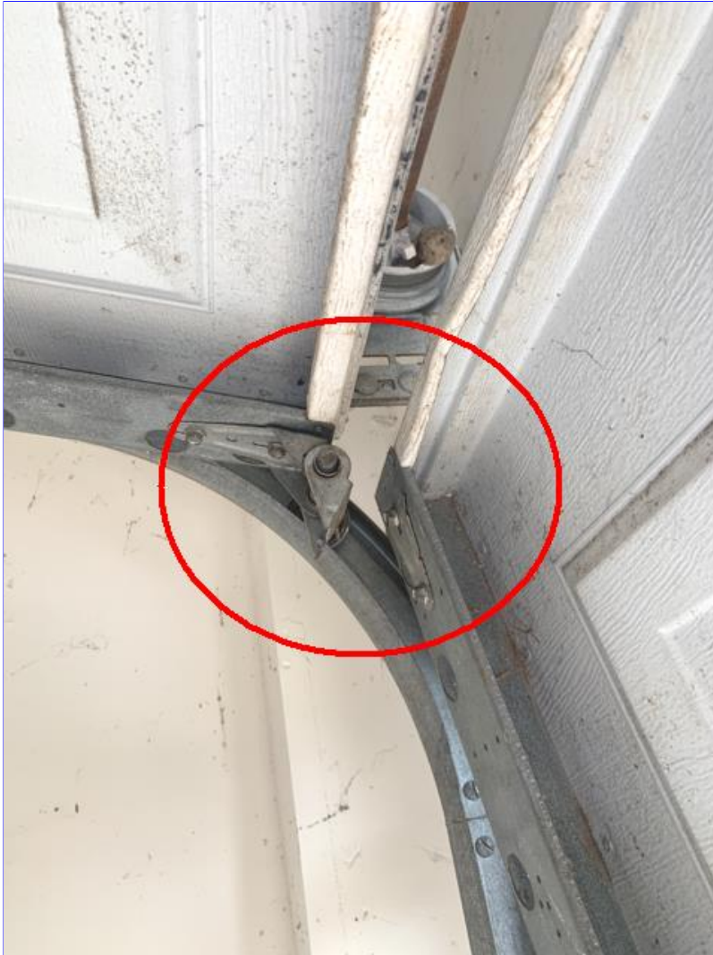
G. Photo 2(Picture) Areas of damage were observed on the garage door.
