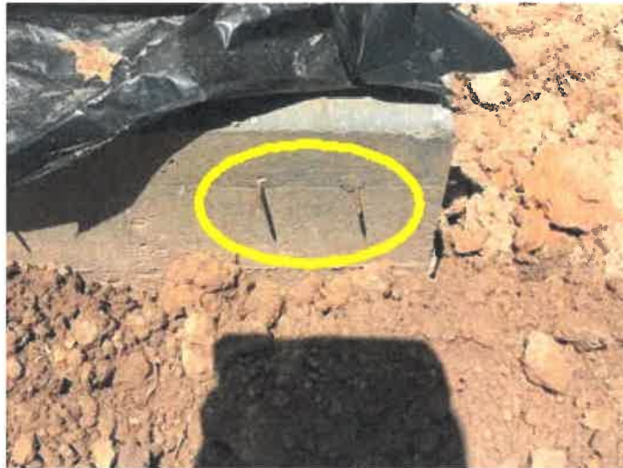
Nails sticking out of the foundation on the left front corner of this home.
