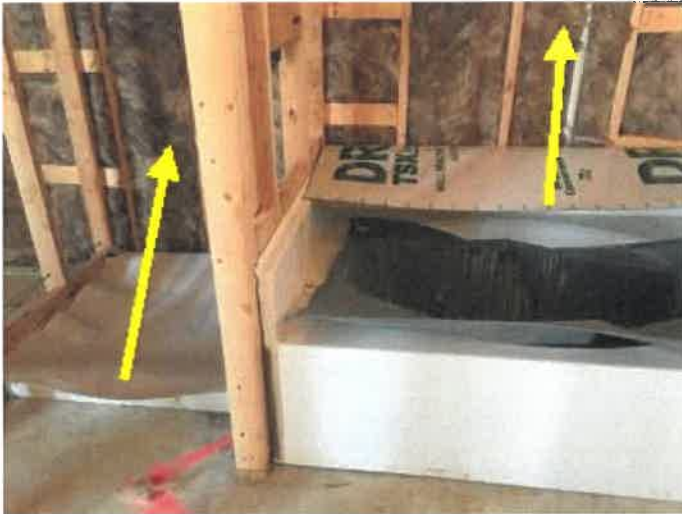
Loose sheathing at the master shower and bathtub.
