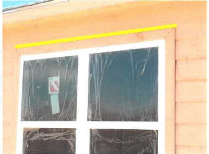
No visible through wall or "Z" flashing at the top of the master bedroom window.
