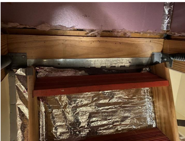
P10, 1: Gaps/Openings at Exteriors Walls Fix: Larger gaps were sealed with foam
