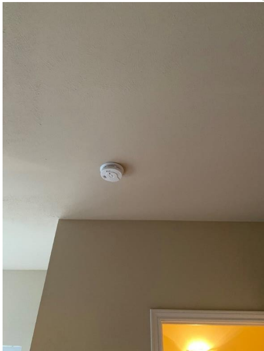
P23, 2: Damaged Vent Fix: secure vent
