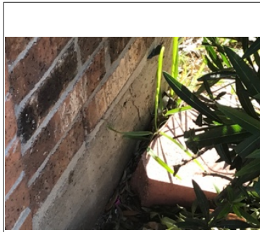
Broken right front corner
