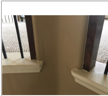
Seam failures at stairway
