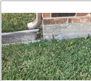
Broken right rear corner
