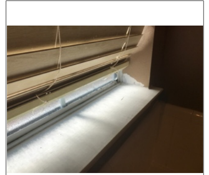
Moisture damage at primary window
