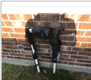
Damaged/ leaking valve assembly needs replacing
