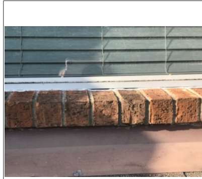
Exterior caulking improvements needed
