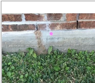
Crack on left side
