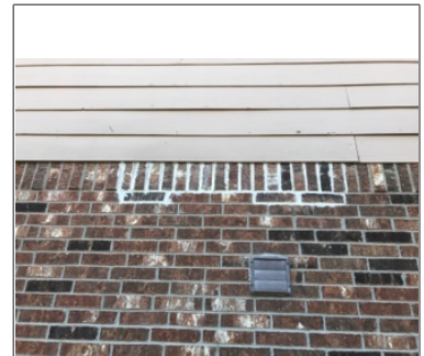
Patching on left side
