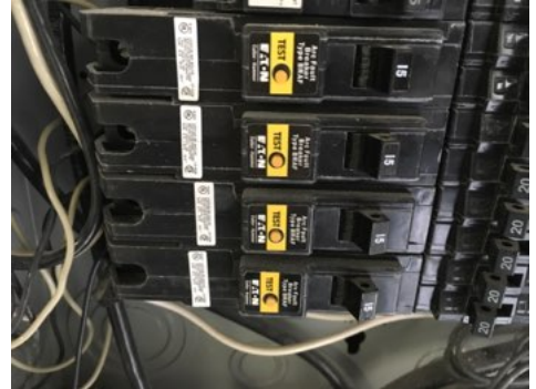
Branch feeder arc faults
