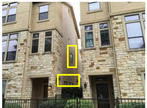
Flashing not over horizontal trim
