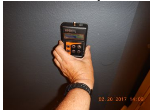
Elevated moisture reading
