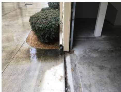
Should discharge away from foundation
