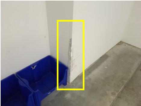
Garage wall damage
