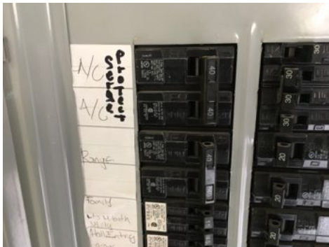
A/C compressor labeled as 40 amp
