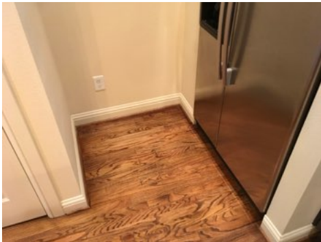
Not GFCI protected
