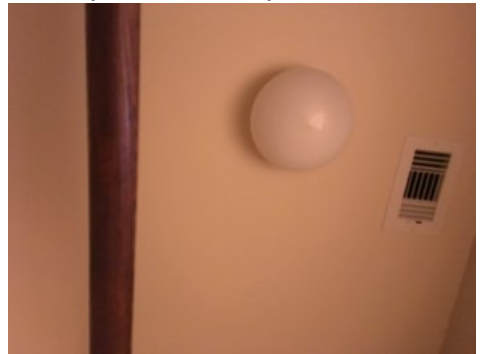
Example of improper location - closet light fixture
