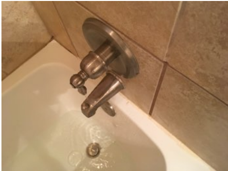
Fixture should be fully sealed to wall
