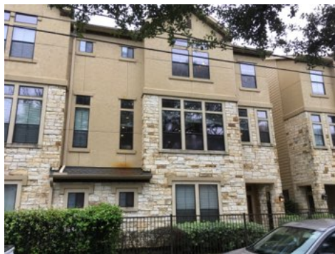
No visible drainage
