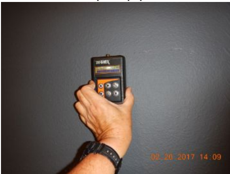
Elevated moisture reading
