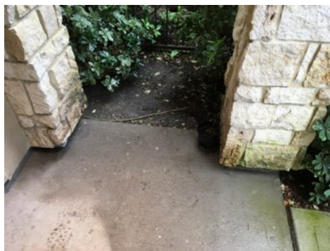
Too close to grade
