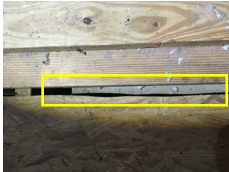
Missing insulation below platform
