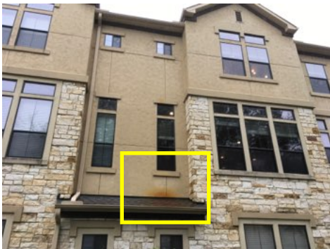
Evidence of AC condensation discharge issues
