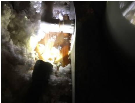
Leak at water heater safety pan
