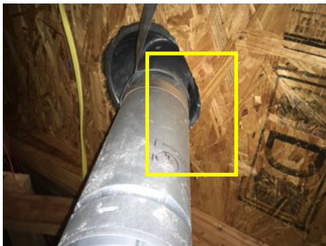
To close to roof sheathing
