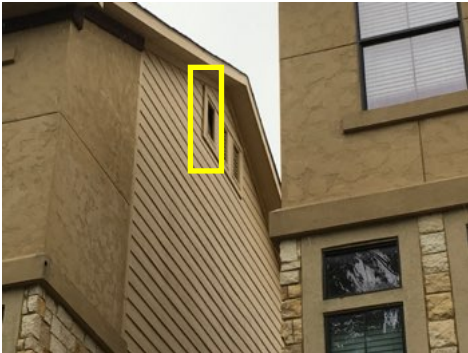
Vent not secured
