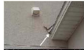
Fig 2: Improper installation (unsealed)
