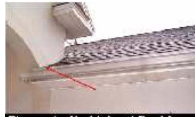
Figure 1: No kickout flashing
