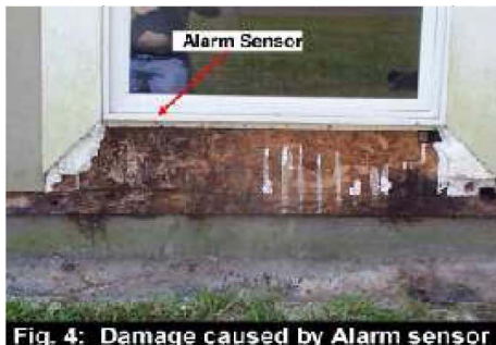
Fig. 4: Damage caused by Alarm sensor
