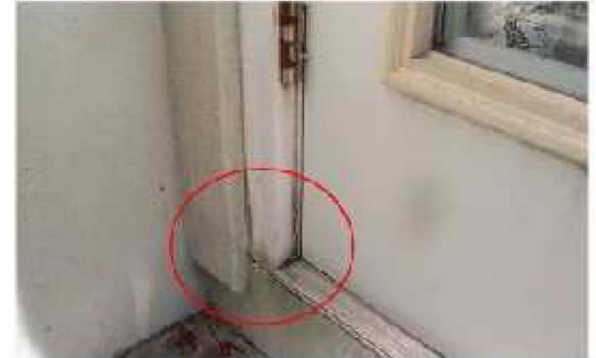
Fig. 1: Damage caused by No sealants
