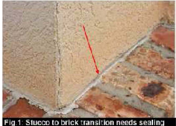
Fig.1: Stucco to brick transition needs sealing
