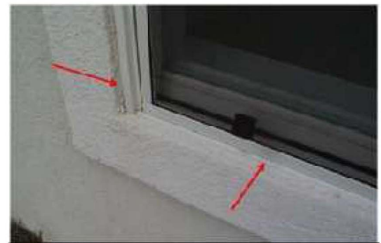
Fig. 2: Example of unsealed window perimeter
