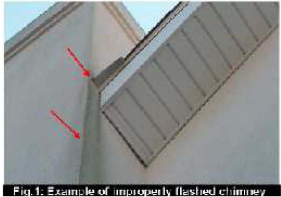
Fig.1: Example of improperly flashed chimney
