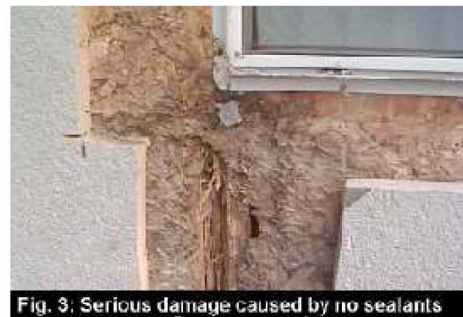
Fig. 3: Serious damage caused by no sealants
