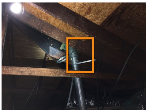
Furnace flue pipe
