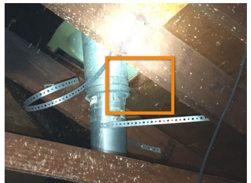
Furnace flue pipe
