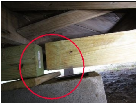
Not properly supported or installed
