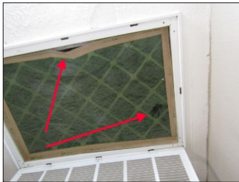
Filter is damaged and needs replacement.
