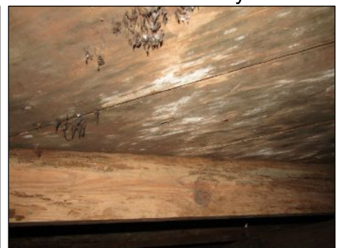
Appears to be mold and fungal activity on sub floor.
