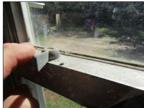
Several window hardware does not latch because of window frame twist.
