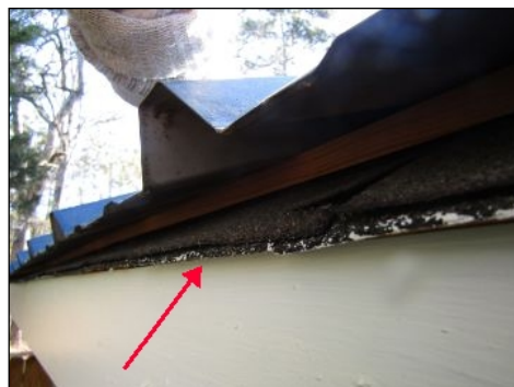
Medal ends close to fascia board without any drip flashing on left side. In need of improvement.
