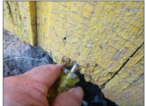
Exterior siding has wood decay at several rain splash areas.
