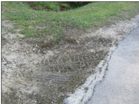
Pot hole forming at street.
