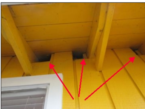
Missing bird blocking will allow animal and insect entry to attic.
