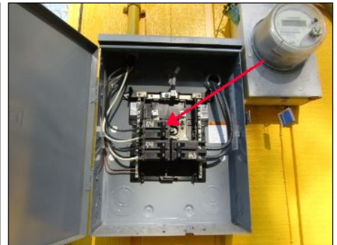
Over sized breaker for A/C condenser.
