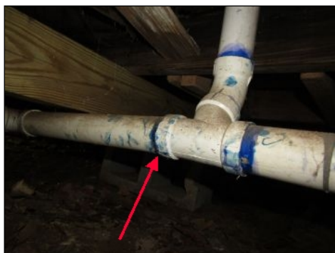
Observed slow leak/drip at "T" fitting in crawlspace. Bathroom Lavatory is missing gasket at drain connection.
