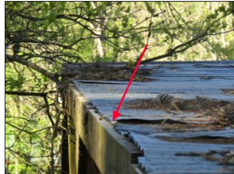
Metal roof for carport has damage and undersized over hang at framing. Water runs into framing.
