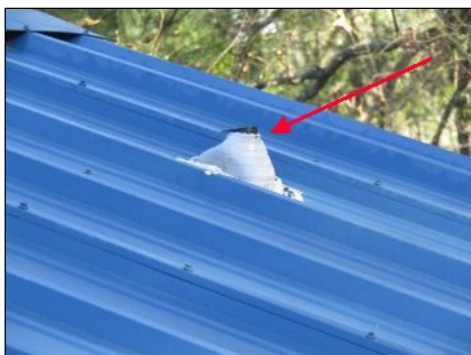
Plumbing vent pipe shall be minimum of 6 inches above roof covering at penetration.
