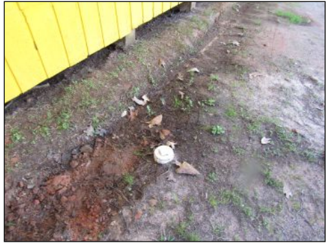
Drip edge erosion because of lack of gutter system.
