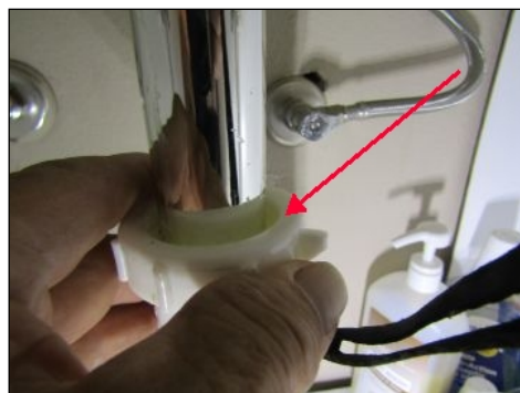
Bathroom Lavatory is missing gasket at drain connection.
