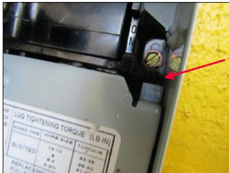
Damage to cover clip at A/C disconnect.
