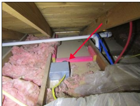
Bathroom fan vents in attic.
