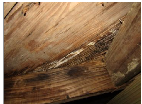
Sub floor decay.
