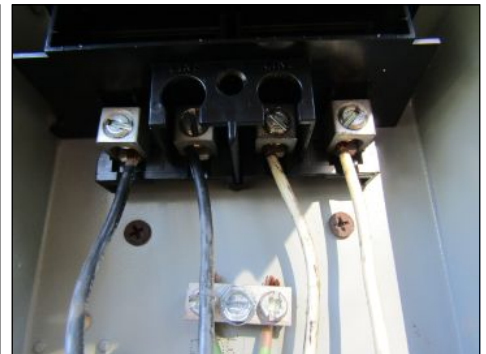
Appear functional and properly installed.
