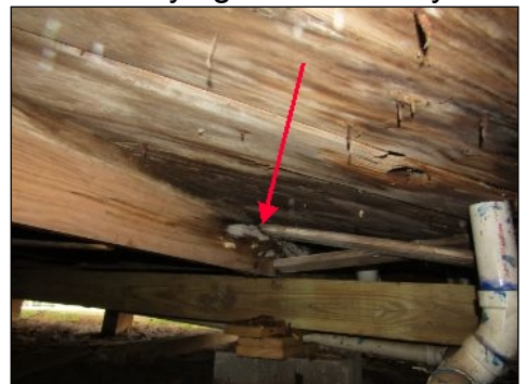
Decaying and damaged floor joist in crawlspace.
