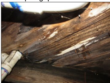
Sub floor under bathroom has decay.
