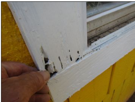
Wood frames have damage.
