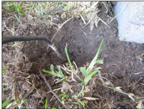
Ground rod not visible.
