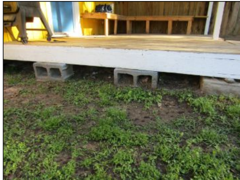
Side deck board has improper placed sideways concrete block supports.
