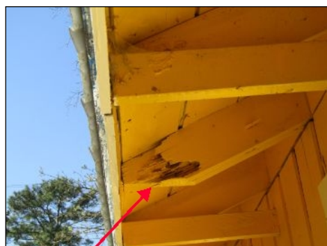
Rafter tail decay.
