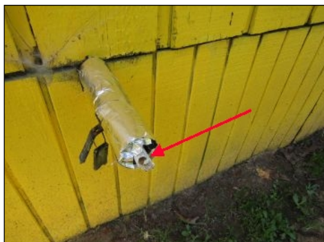
Abandon pipe with broken area at backyard.
