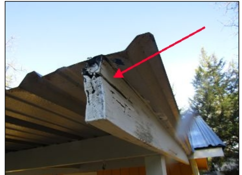
Exposed wood is rotting at tail end.
