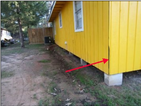
Missing corner trim with open gaps.
