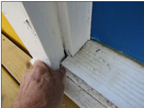
Caulk needed at several areas around framing.
