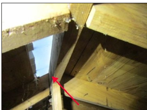
No insect screen at ridge vent area.
