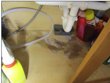
Damaged cabinet floor under sink.
