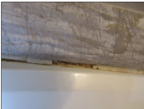
Grout damage in bathroom shower.
