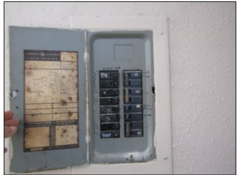
No main disconnect.
