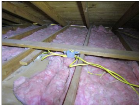
Electric box needs cover plate.
