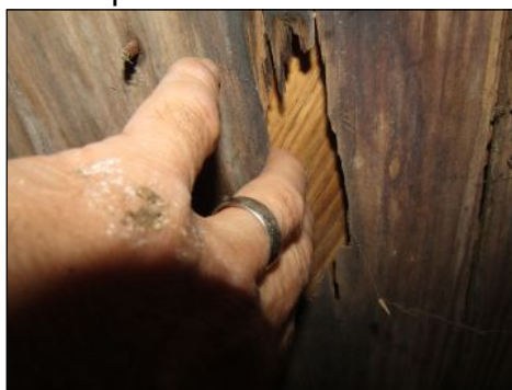
Sub floor decay
