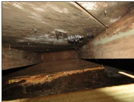
Evidence of floor joist and sub floor decay, fungal activity.
