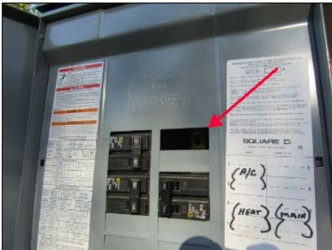
There are open breaker slots in the panel. This is a safety hazard.
