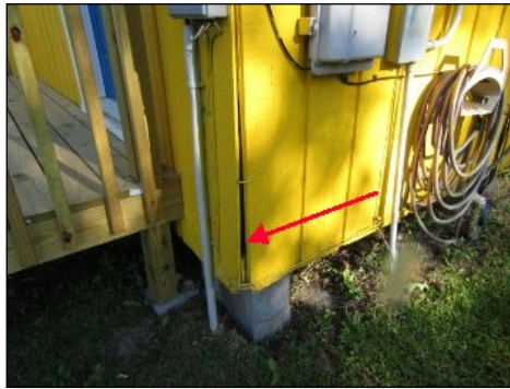
Open gap at missing corner trim.
