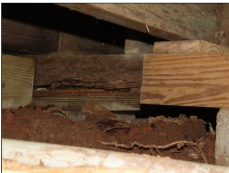
Sill beams and floor joist are too close to soil.
