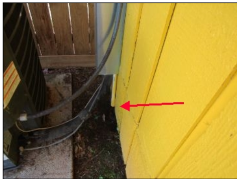
Condensation drain line terminates at exterior onto ground.
