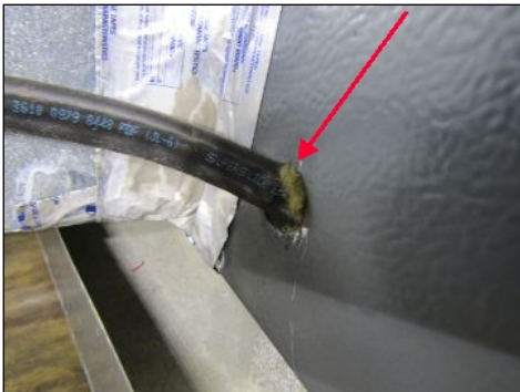
Missing protective bushing at air handler electrical entry.
