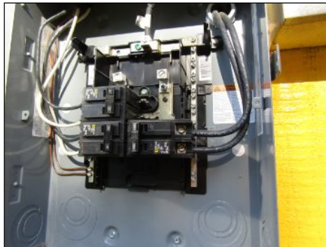
No separate ground present to main panel.
