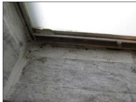
Poor quality tile installation.
