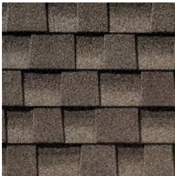
Roof. Weathered Wood 1.4.2020
