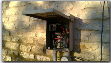
Sub Panel Box General Electric - GE Sub Panel Box Location: AC Unit Sub Panel Service Entrance: Within Structure
