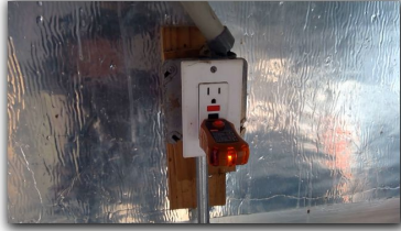
( Inside the pump house )
