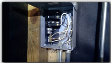
Sub Panel Box General Electric - GE Sub Panel Box Location: Out Building Sub Panel Service Entrance: Within Structure
