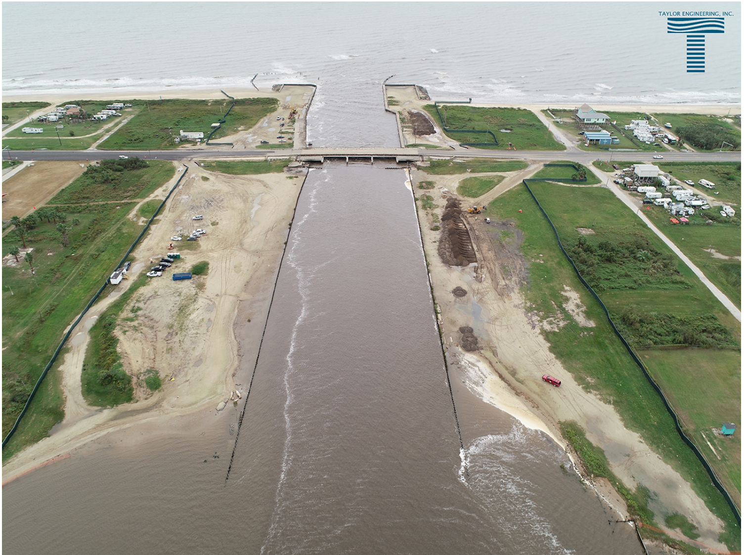
Drone footage capturing the erosion occurring at Rollover Pass before the construction began
