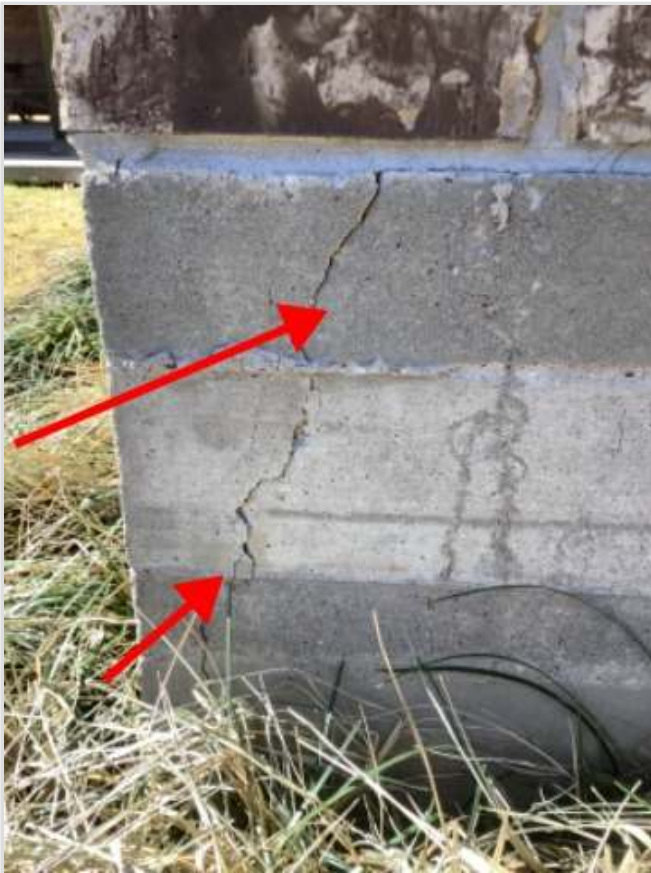
Corner pop on foundation left front of house
