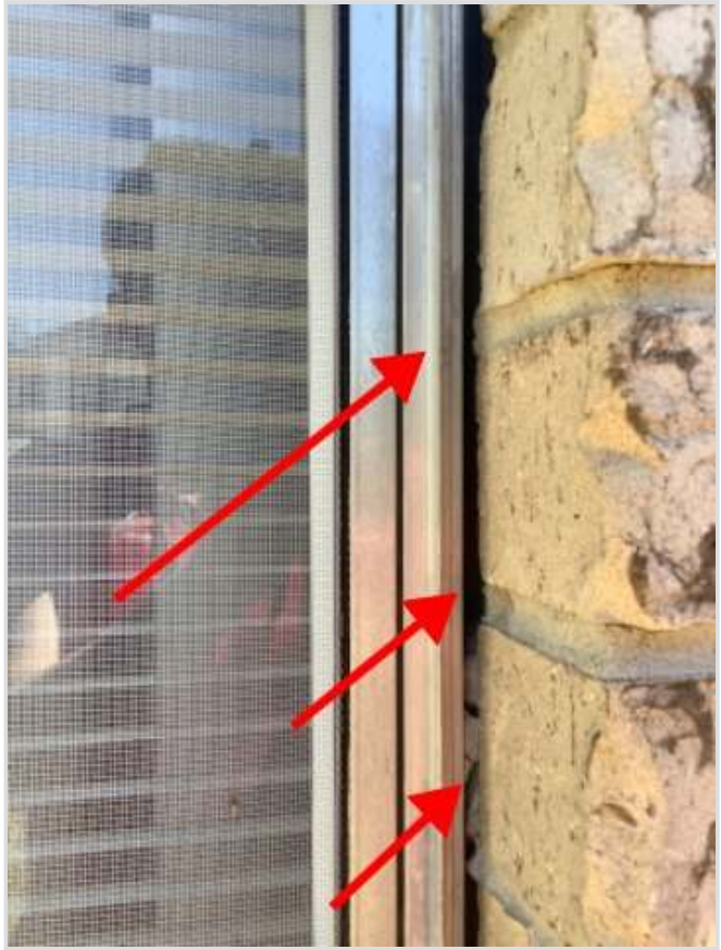
Gaps round window needs to be caulked
