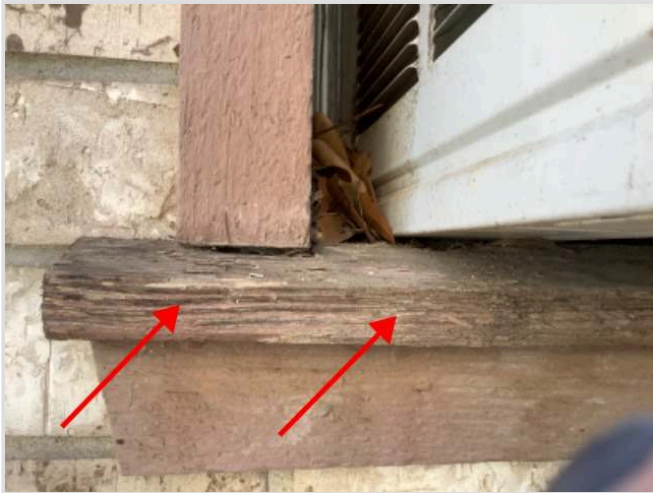
Around window AC unit
