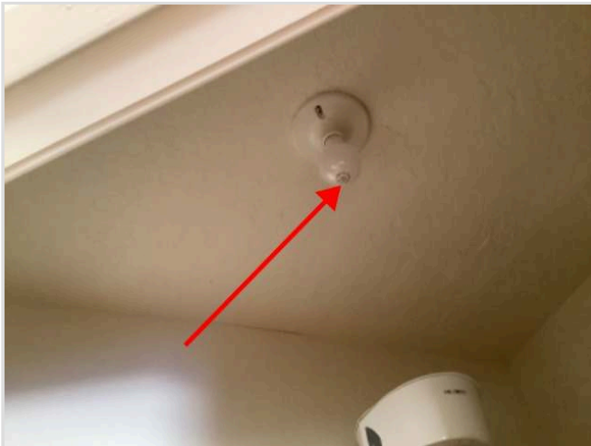
Unprotected lightbulb in kitchen pantry
