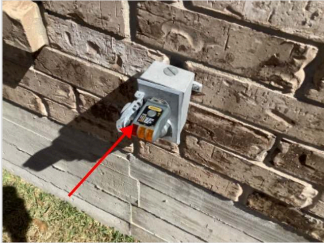
No GFCI protection on exterior walls
