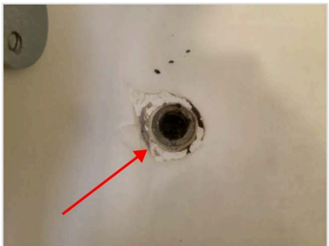
Corroded tub drain
