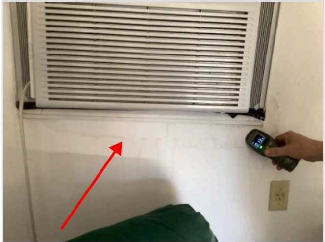
Evidence of past water damage around window air unit and converted garage room
