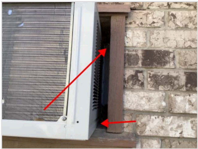
AC window unit is not sealed around the perimeter.
