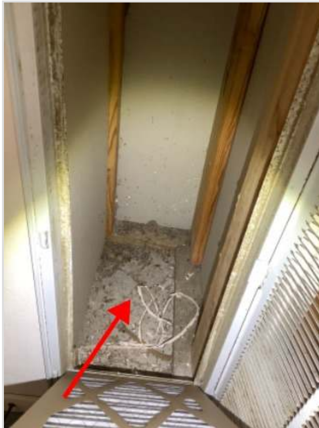
Dirty supply air intake vent in hallway
