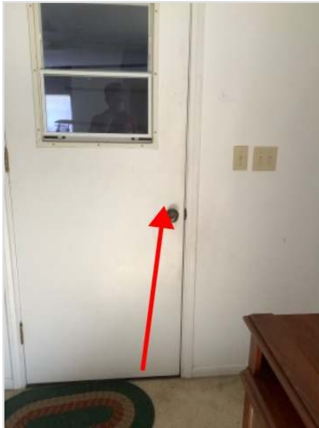
Door lock does not work
