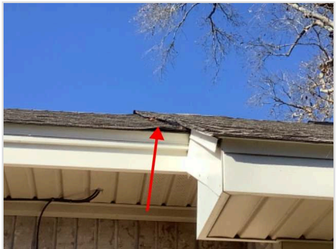
Shingles lifted to the left of garage
