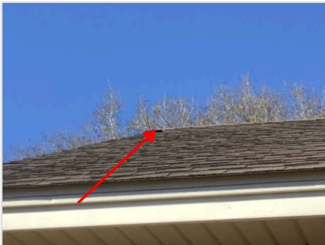
Shingle lifting left side of house
