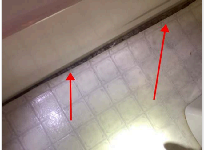
Linoleum is peeling up around the master tub
