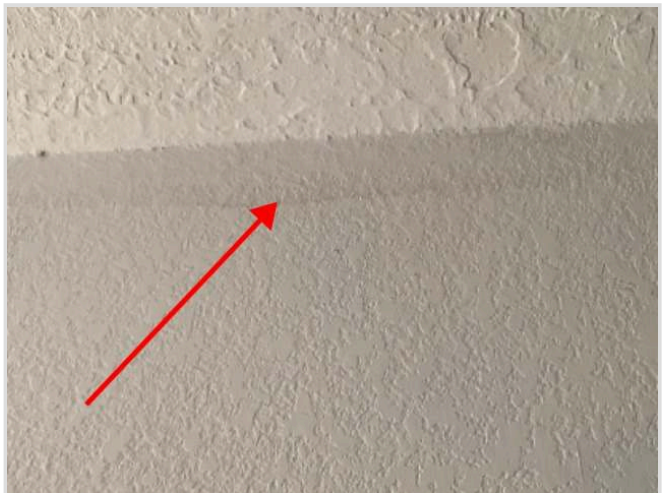
Evidence of past moisture in wall in converted garage room
