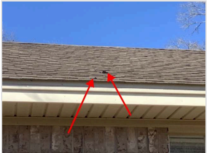
Shingles are lifting left side of house
