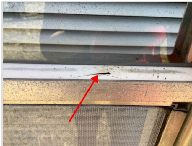
Window pane plastic trim is cracked on right rear of home
