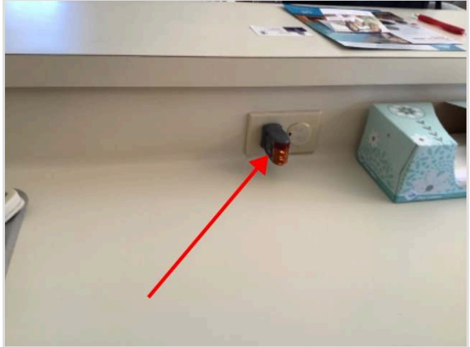
Outlets in kitchen are not GFCI protected.
