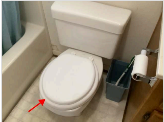
Toilet in master is loose
