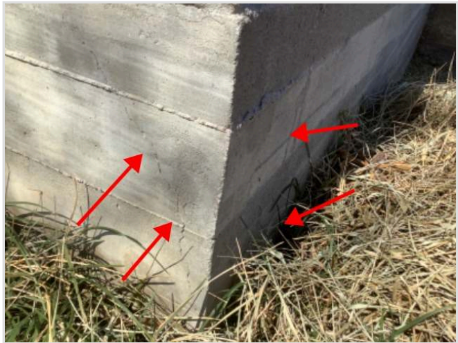
Corner pop on foundation left front of house on both sides.
