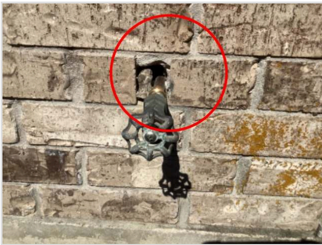
Area around faucet needs to be sealed to prevent intrusion of insects left side of house
