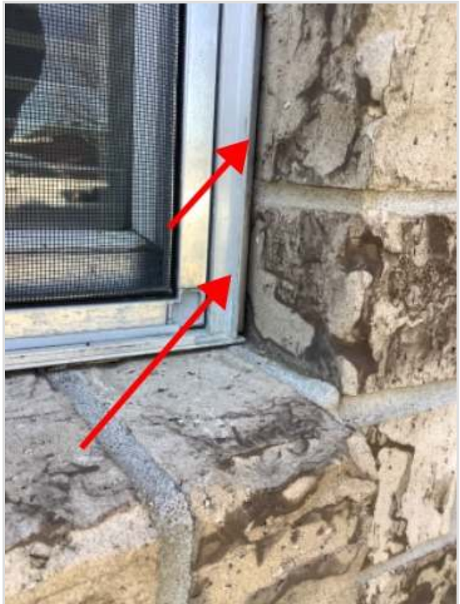
Gaps around windows that need to be caulked
