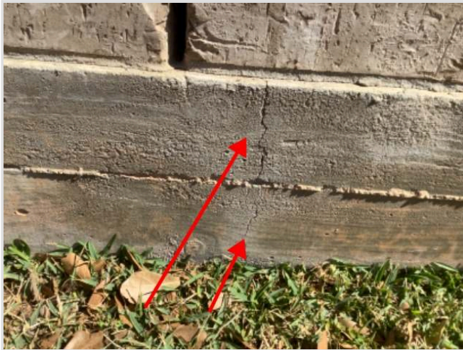
Minor cracking at rear of house
