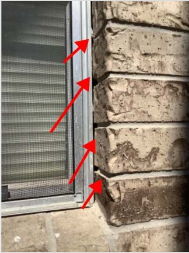
Gaps surround windows that need to be caulked
