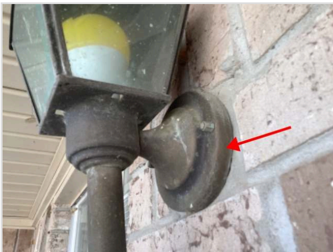
Area around base of all light fixtures on the exterior need to be sealed to prevent water intrusion
