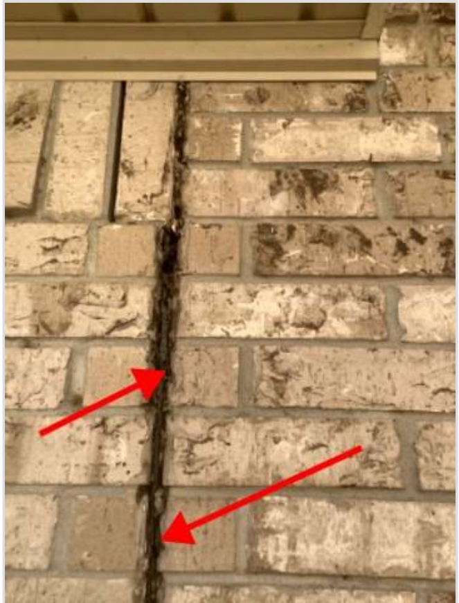
Expansion joint sealant is deteriorated and needs to be replaced
