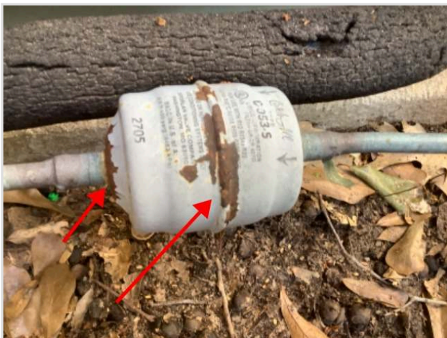
Rusted dryer filter at condenser
