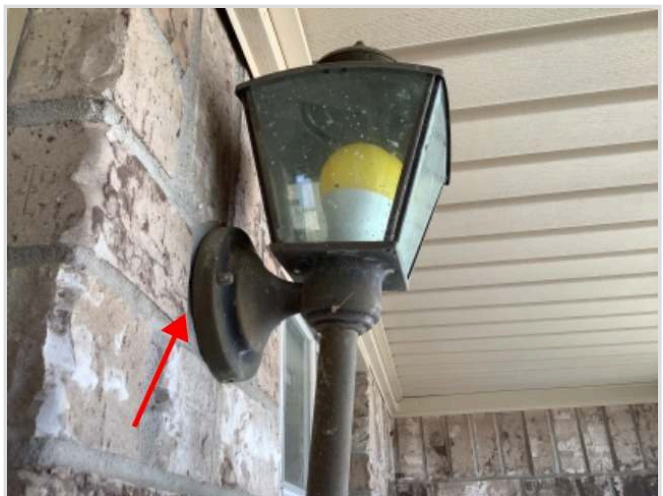
Seal around base of light fixture
