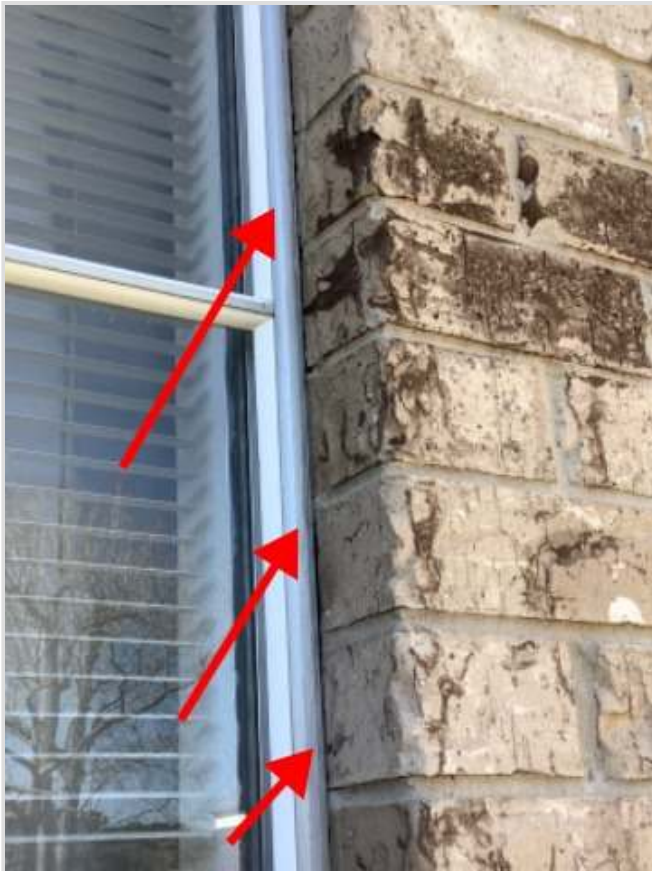
Gaps around windows that need to be caulked
