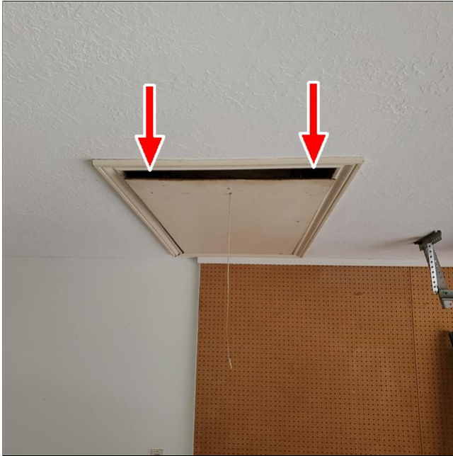
D. Item 1(Picture) Pull down does not close properly.
