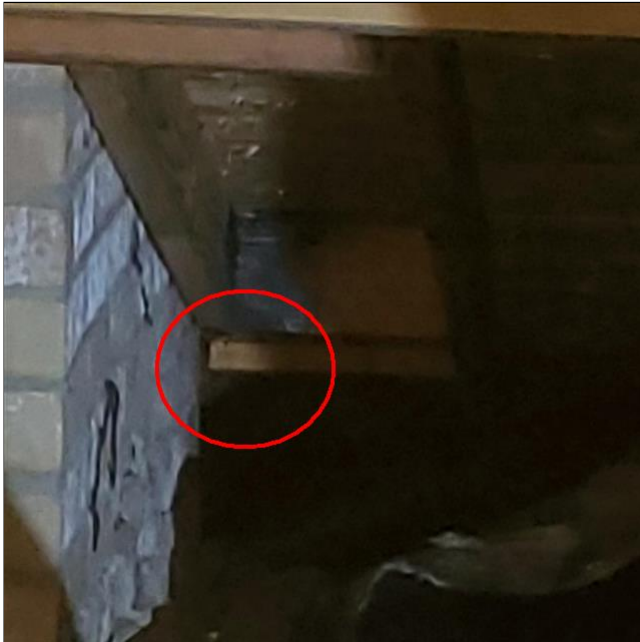
D. Item 2(Picture) Light was shining during picture and the burned framing is not visible in photo.
