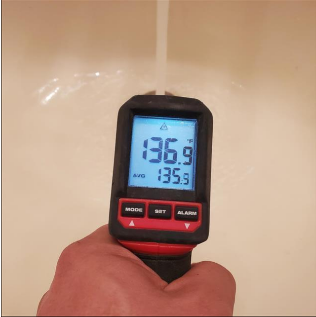
C. Item 8(Picture) Water was too hot.
