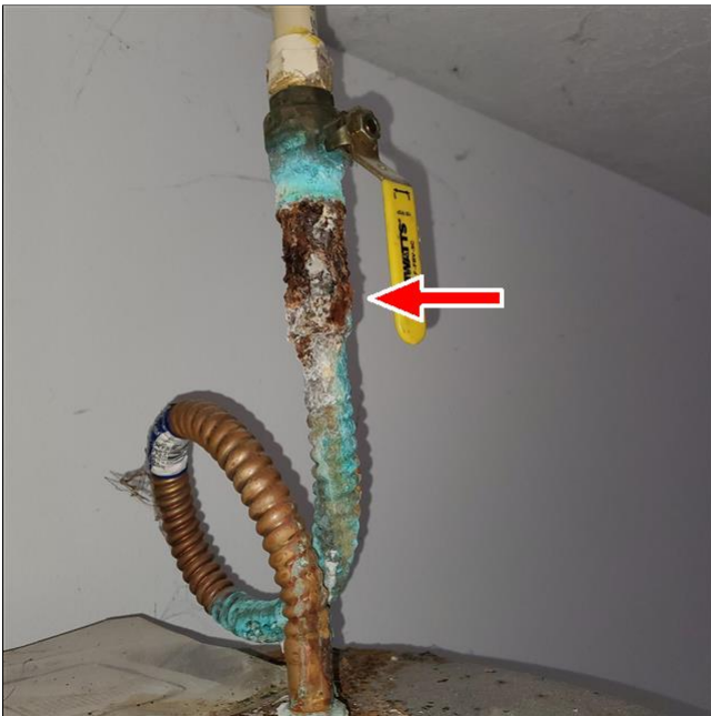
C. Item 3(Picture) Photo of corrosion at connections.
