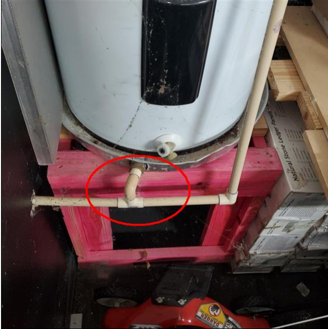
C. Item 4(Picture) Pipes should not be tied together.
