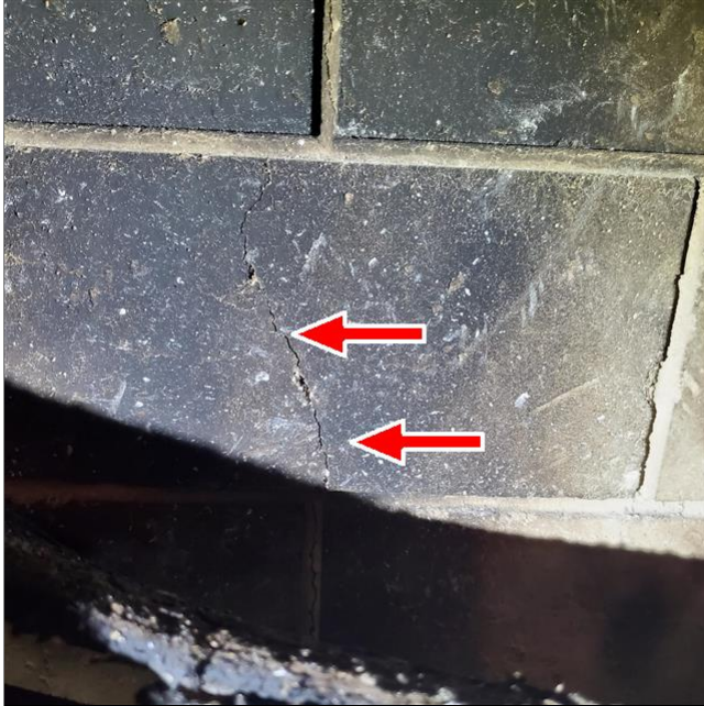
J. Item 1(Picture) Photo of hairline crack at back wall.
