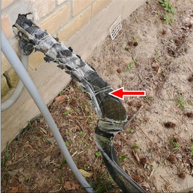
B. Item 5(Picture) Suction line for older unit needs to be re-insulated.
