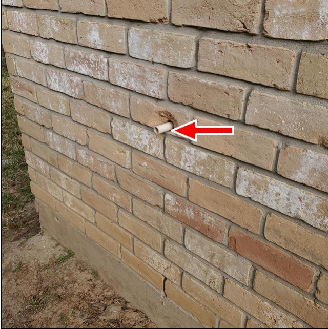
C. Item 2(Picture) Pipe does not have a turndown elbow and is too high from the ground.
