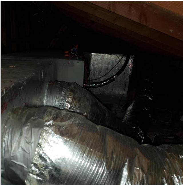
A. Item 2(Picture) Overview of second heating system.
