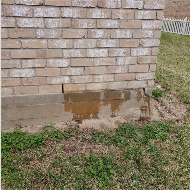
A. Item 5(Picture) Photo of water running down foundation after master shower was tested.
