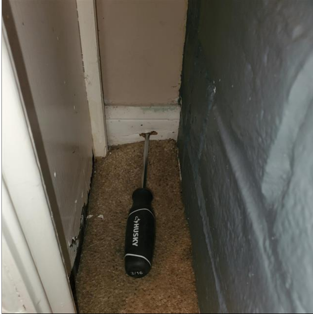
F. Item 2(Picture) Baseboard was soft and was damaged.
