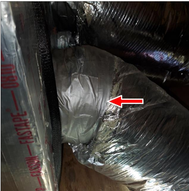
C. Item 4(Picture) Duct tape should not be used to seal ducts to plenums.
