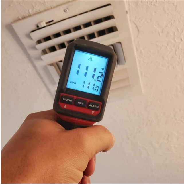
A. Item 3(Picture) Heating system #1 warming the home.
