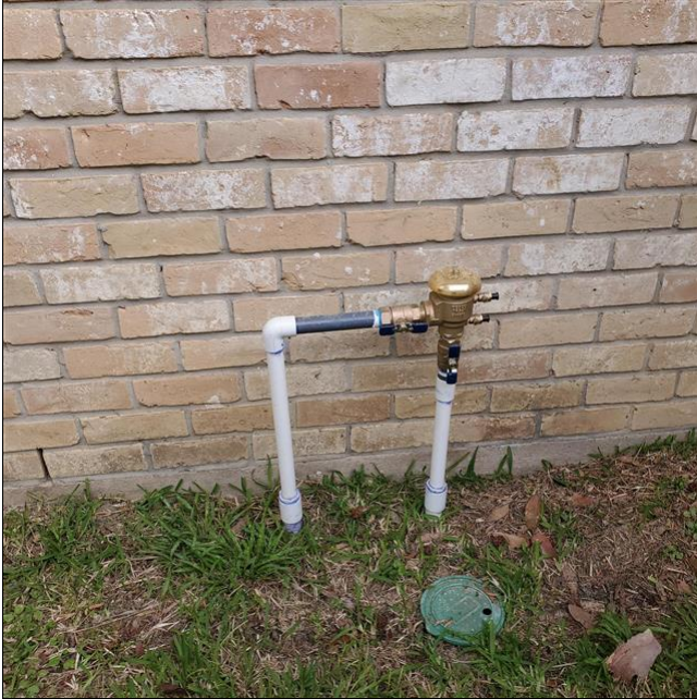
A. Item 2(Picture) Pipes should be strapped to the wall for security.
