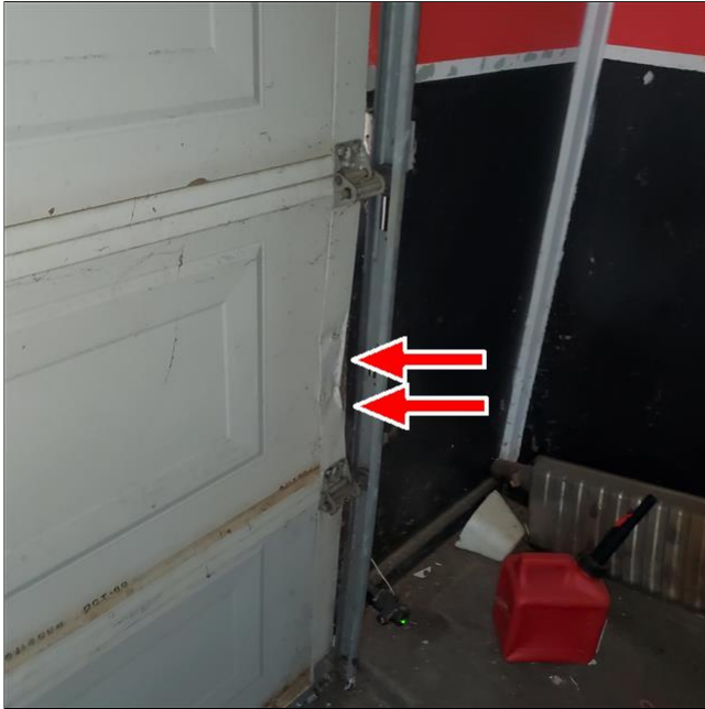
G. Item 1(Picture) Door is damaged.
