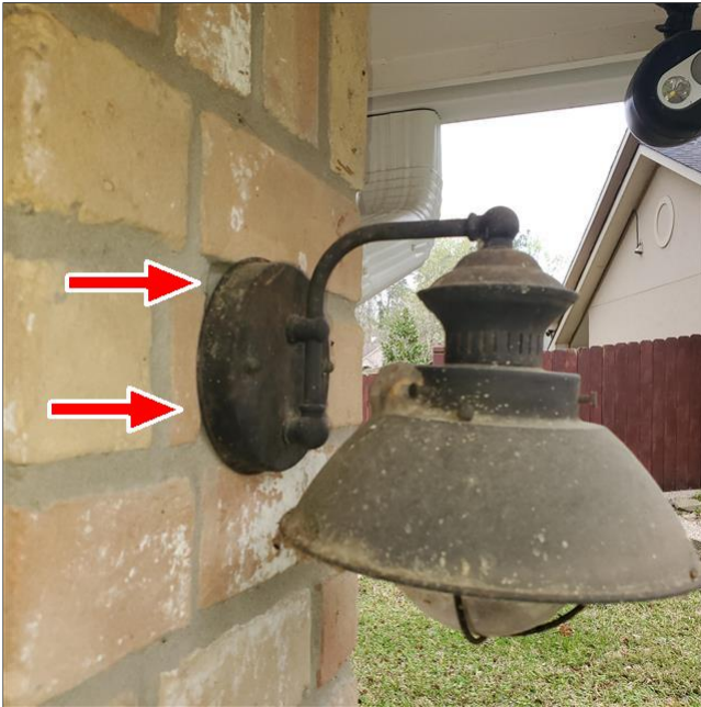
E. Item 3(Picture) Need to seal all wall penetrations to brick.
