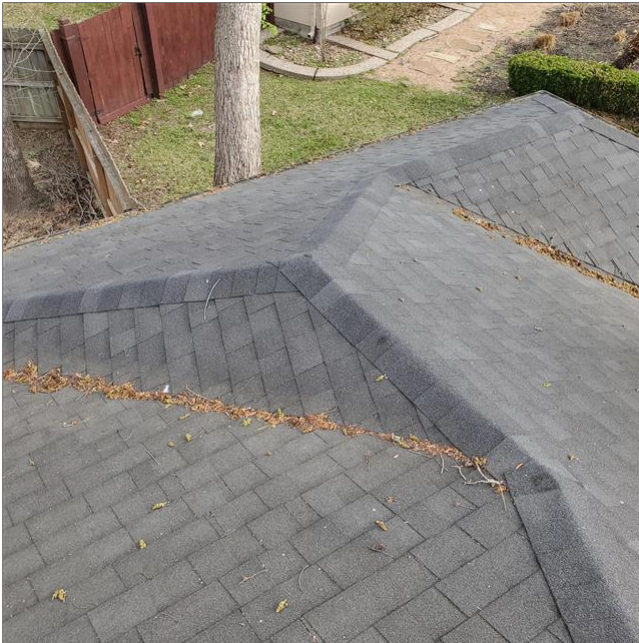
C. Item 4(Picture) Debris should be cleaned off of the roof.
