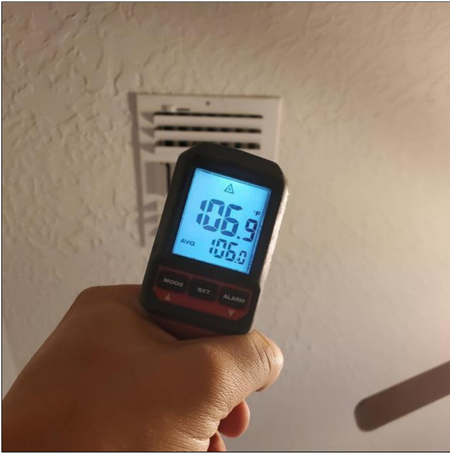
A. Item 4(Picture) Heating system #2 warming the home.
