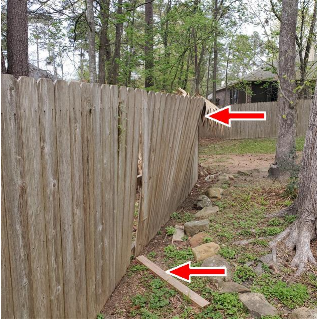
L. Item 1(Picture) Photo of damaged and leaning fence.
