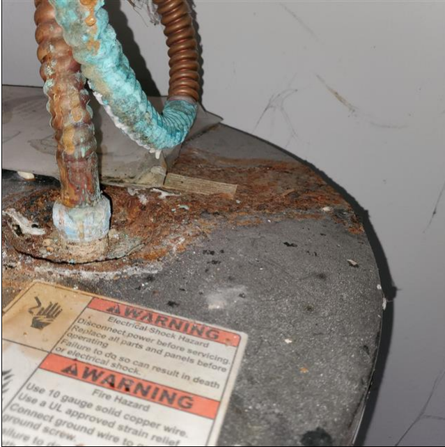
C. Item 6(Picture) Rust at top.
