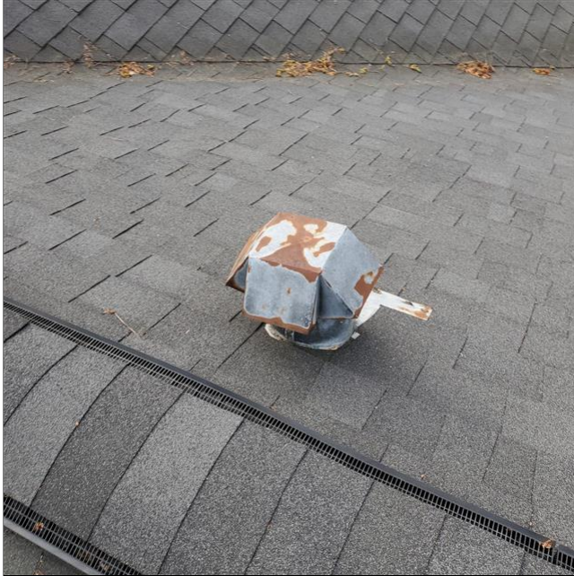
C. Item 7(Picture) Exhaust cap should be replaced.
