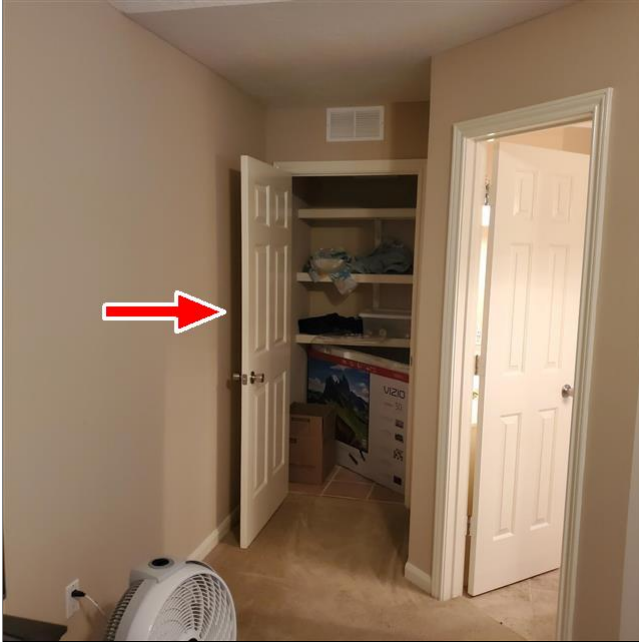
G. Item 3(Picture) This door needs repair.
