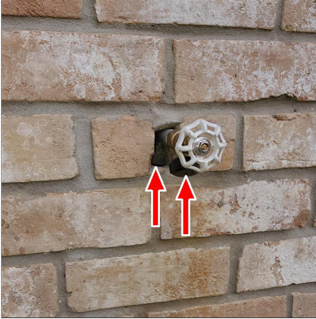
E. Item 4(Picture) Large gap around hose bib at the back.
