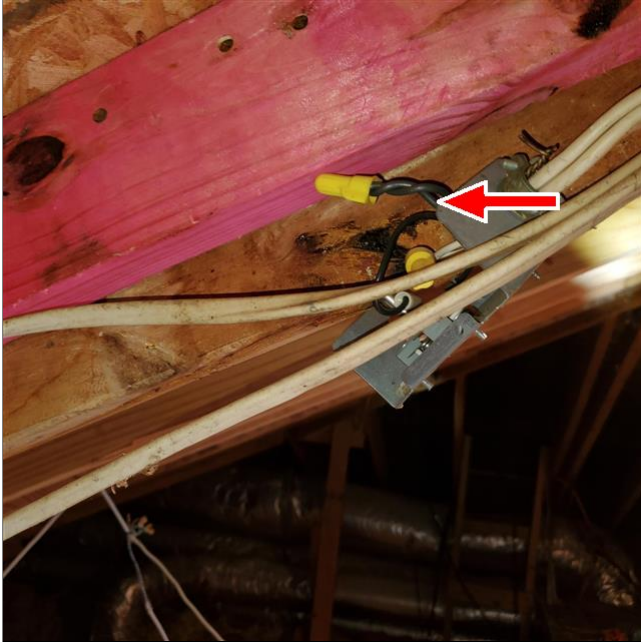
D. Item 6(Picture) Splices not contained in junction box.
