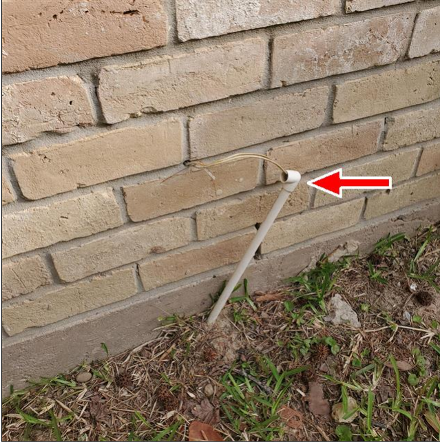
B. Item 1(Picture) Conduit not secured to wall.
