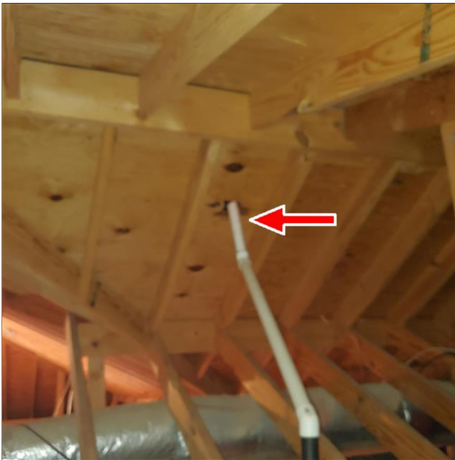
D. Item 5(Picture) Stain around plumbing vent pipe at the left side.
