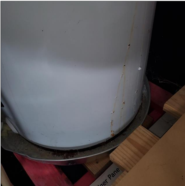
C. Item 7(Picture) Rust near bottom.
