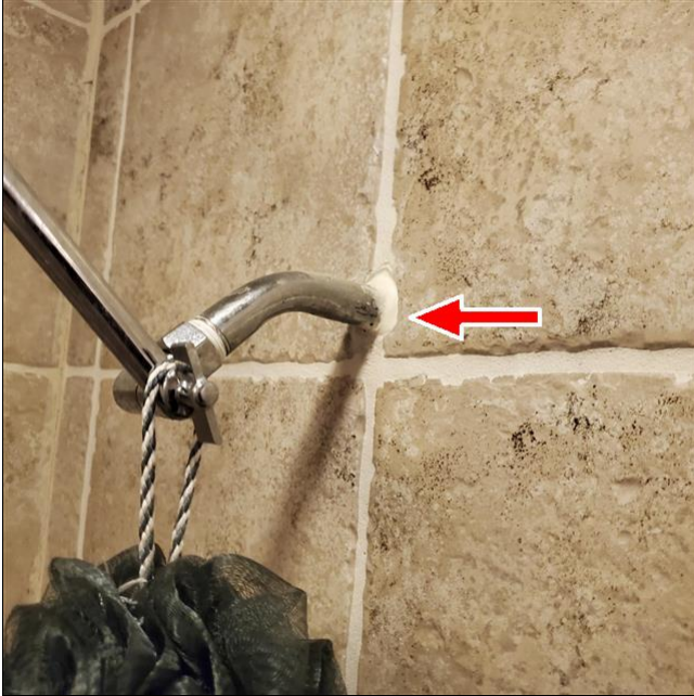
A. Item 3(Picture) Missing an escutcheon.
