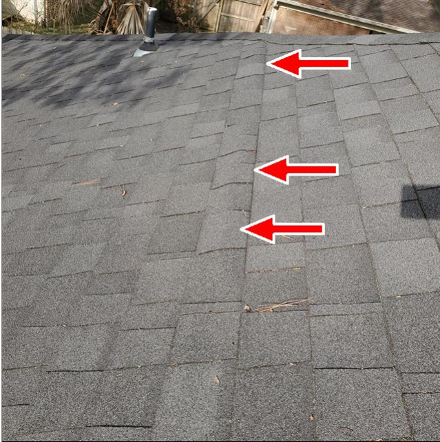
C. Item 5(Picture) Photo of buckled shingles.
