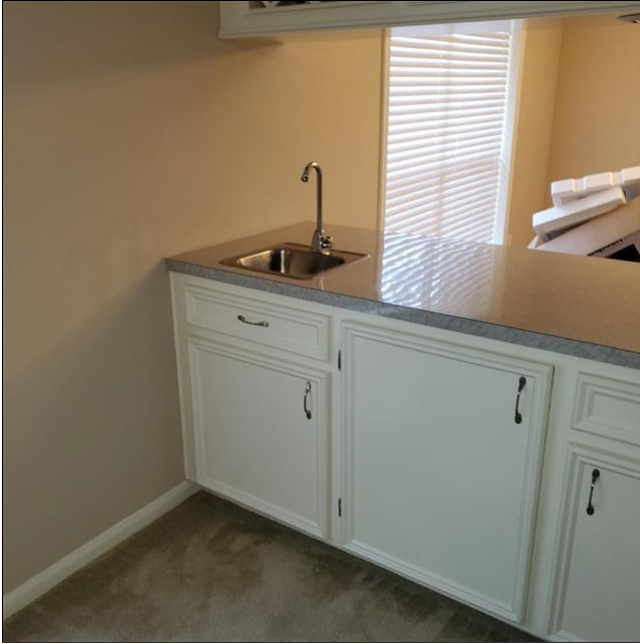
B. Item 2(Picture) There is no outlet close to this sink.
