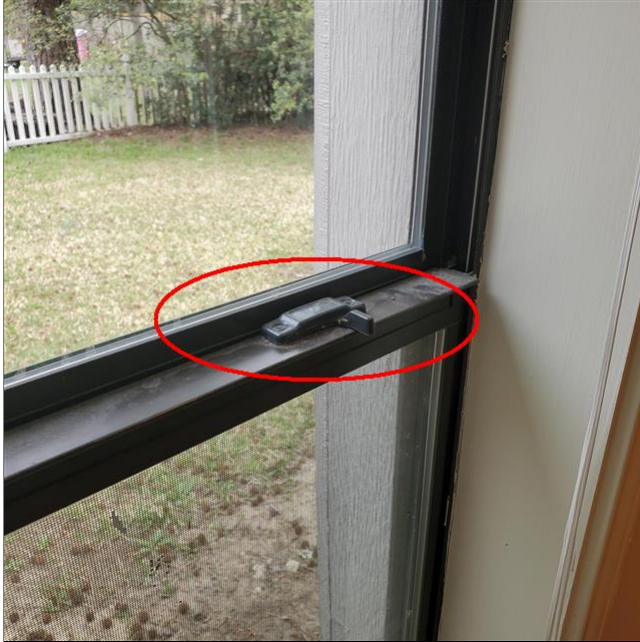
H. Item 1(Picture) Right side of window was unable to lock.
