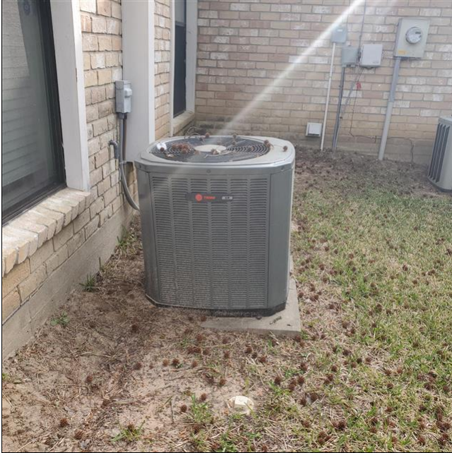
B. Item 3(Picture) Pad does not elevate unit 3" above the ground.
