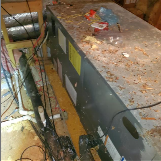
A. Item 1(Picture) Overview of heating system.
