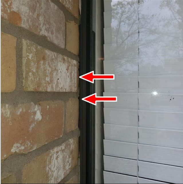
E. Item 2(Picture) Windows need to be caulked and sealed.
