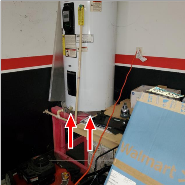
C. Item 5(Picture) Pan should slope toward drain line.
