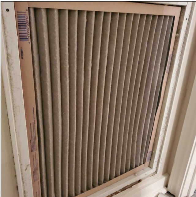
C. Item 1(Picture) Filters were dirty.
