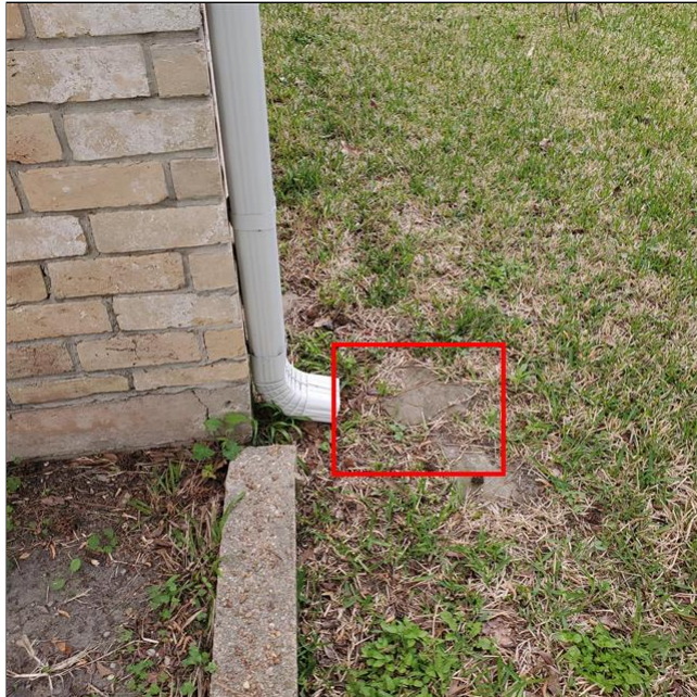
B. Item 1(Picture) Need splash blocks under all downspouts.
