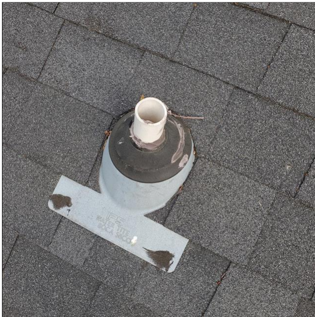
B. Item 2(Picture) PVC should be painted.
