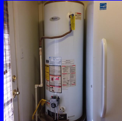
50 gallon gas water heater located in washer/dryer room
