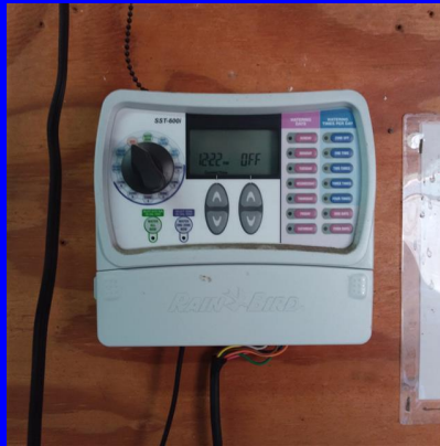
Sprinkler system control panel located at right side of garage
