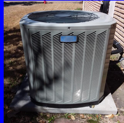
HVAC outside condenser
