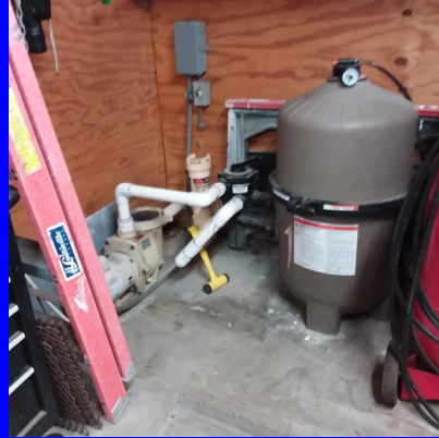
Pool equipment located in garage
