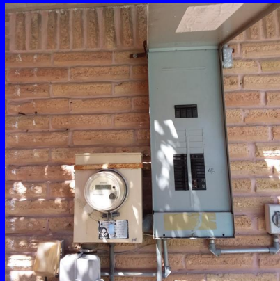
Below ground service located at rear of home
