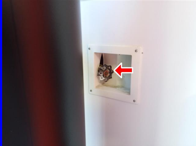
main water supply in garage
