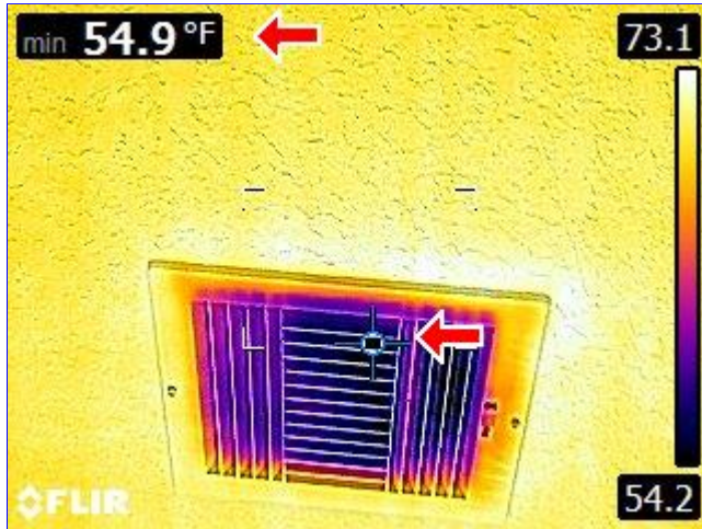
B. Item 1(Picture) 1st floor vent
