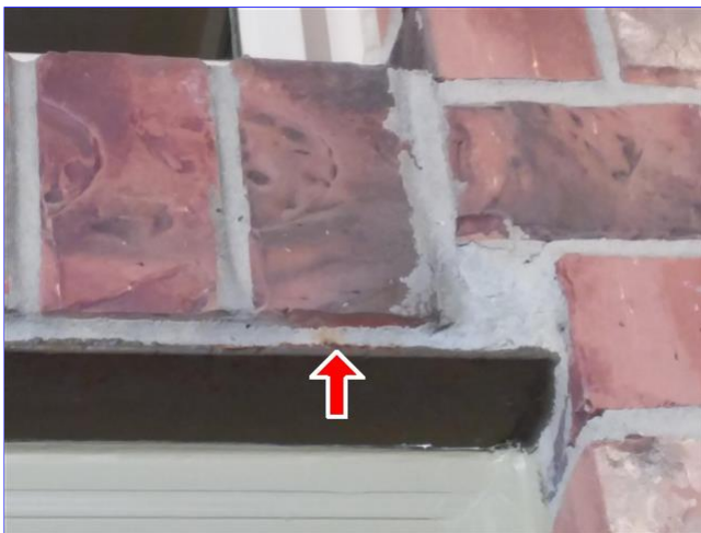
E. Item 2(Picture) door lintel rust
