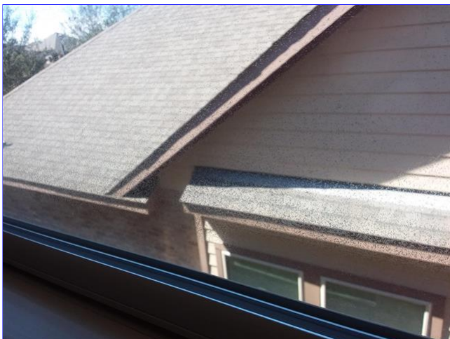
H. Item 3(Picture) cloudy glass second floor living room
