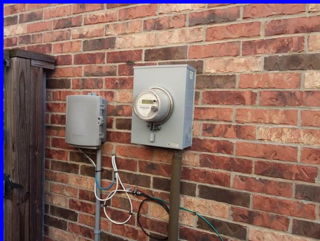
electrical meter right side underground service
