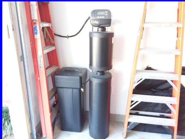
water filter in garage
