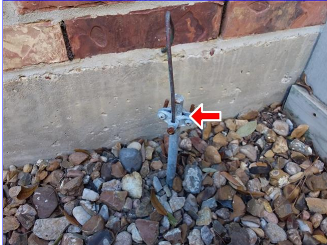
A. Item 2(Picture) improper grounding clamp
