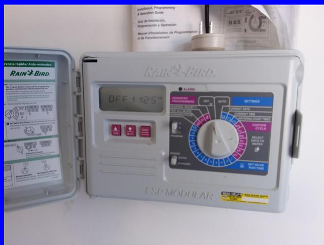
irrigation control and garage
