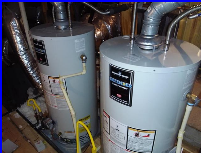
water heaters in attic
