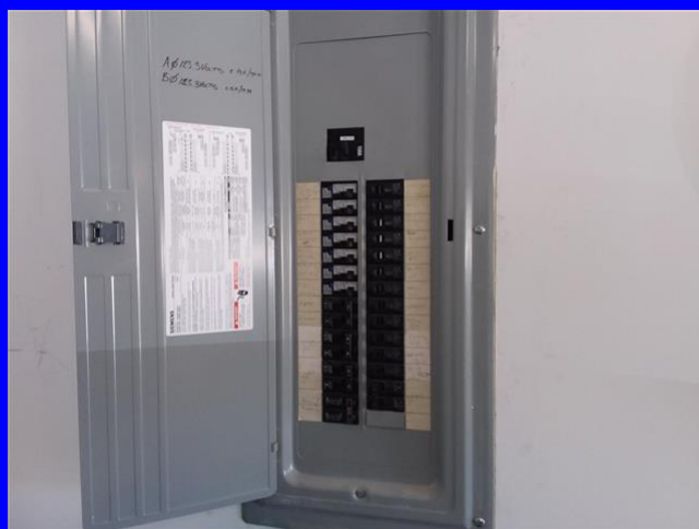
150 amp panel in garage
