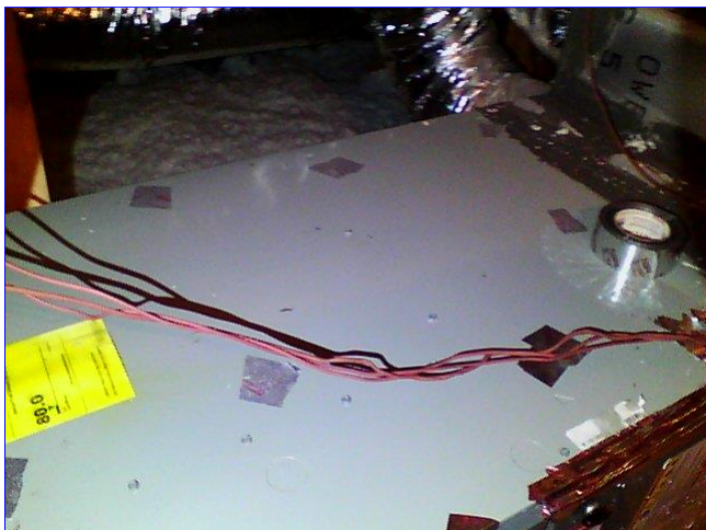
B. Item 7(Picture) fungal growth removed on furnace
