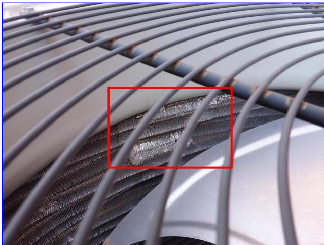
B. Item 5(Picture) minor coil damage observed
