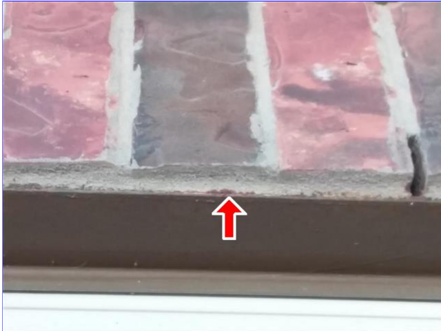
E. Item 1(Picture) window lintel rust
