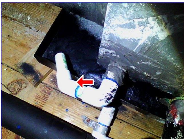
B. Item 8(Picture) fungal growth removed on furnace piping
