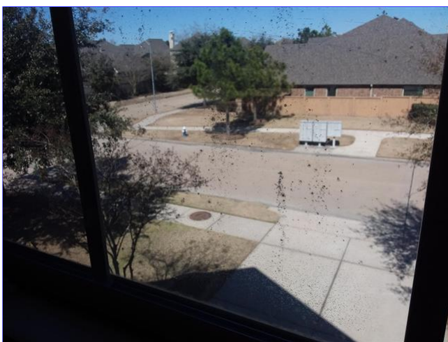
H. Item 4(Picture) cloudy glass second floor front bedroom
