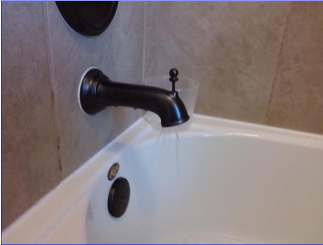
A. Item 1(Picture) leaking second floor faucet diverter
