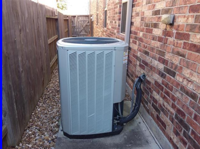
condenser unit right side
