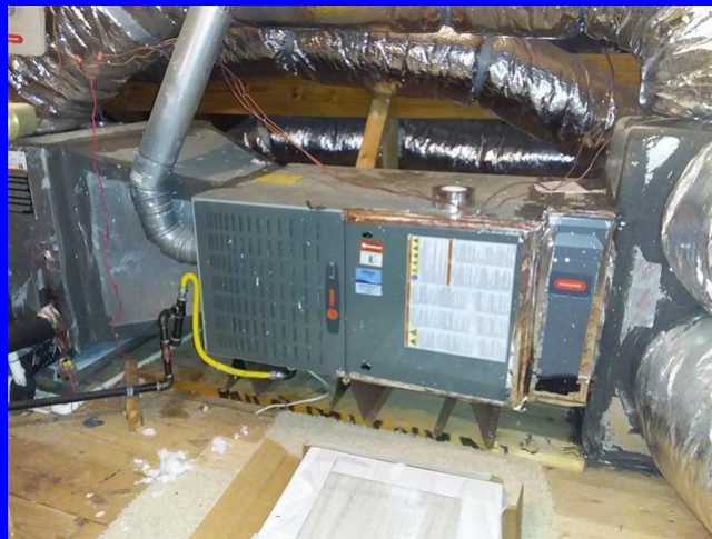
gas furnace in attic
