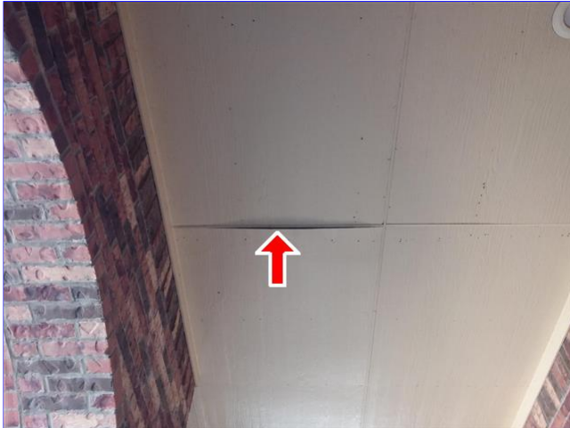
K. Item 1(Picture) loose cover at entryway
