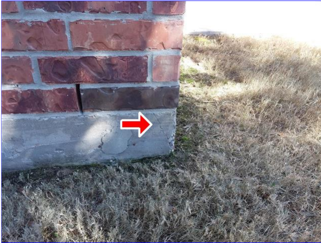
A. Item 1(Picture) minor corner pop back of home
