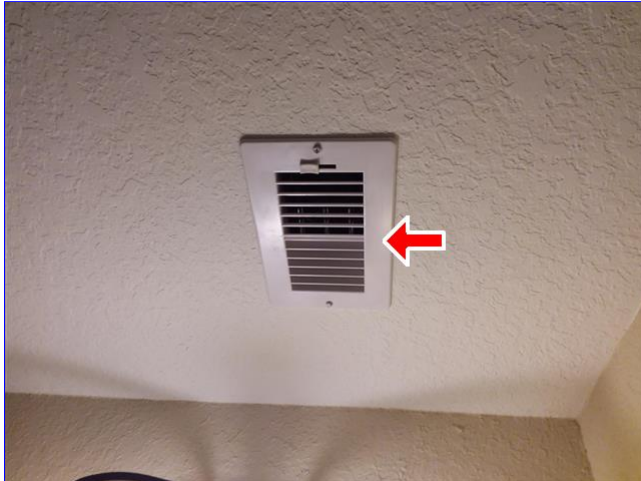
C. Item 1(Picture) low air flow 2nd floor middle bathroom
