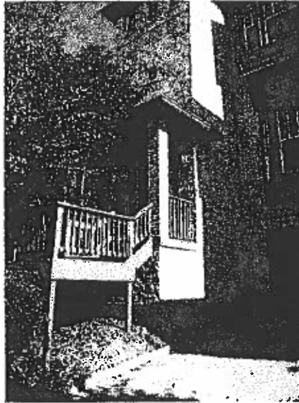
FRONT VIEW WITH VENT UNDER STAIRS, 12-10-2013
