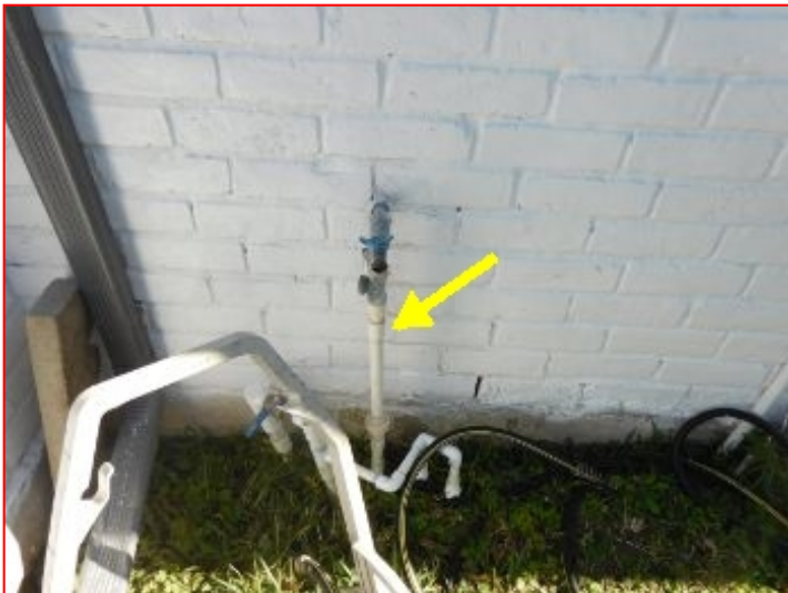
Supply pipe at the shut off valve is located such that it is susceptible to damage / freezing. Insulation is recommended.
