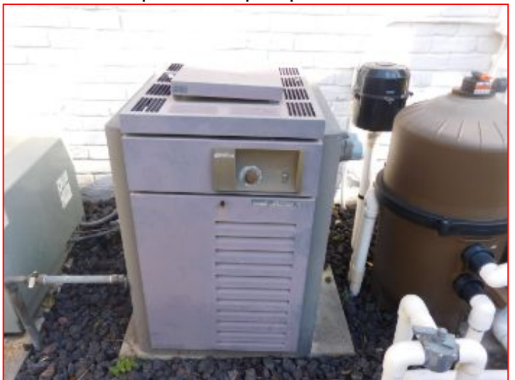
Pool / Spa Heater: Gas operated pool / spa heater is in poor condition and not connected. Needs to be replaced. Consult a qualified provider.
