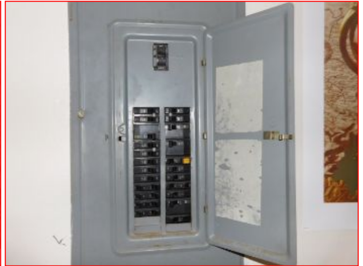
Panel is not labeled properly.
