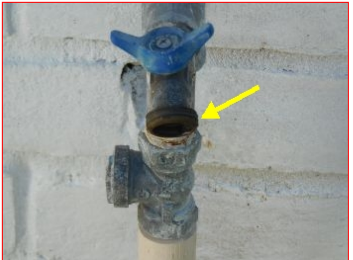
Back flow check valves are not installed on the outside hose bibs.
