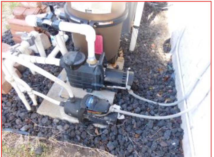
Motors are not grounded as required. Corrective action required for safety reasons. Consult a qualified repair provider.
