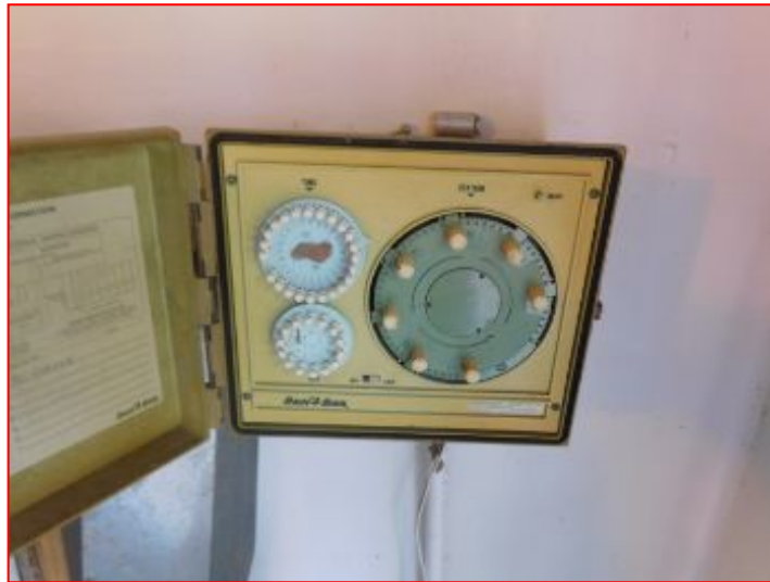
System is not operating. Needs evaluation.
