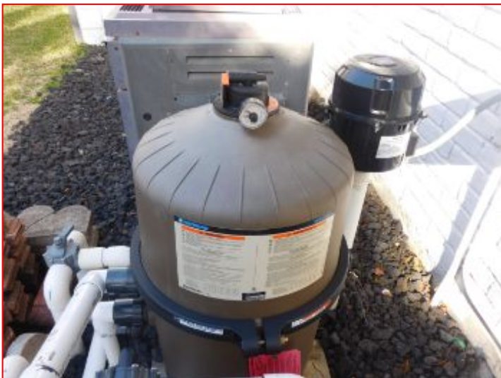
Filter type: Diatomaceous Earth: The filter is in good condition and appears to be operating as designed.
