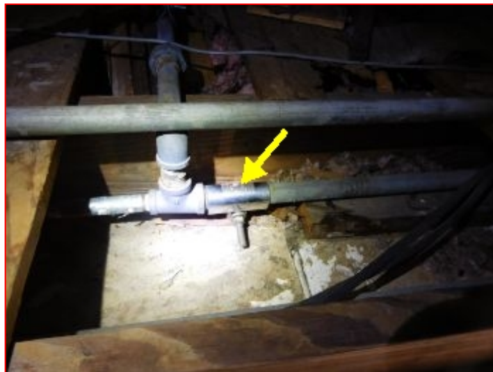
Sign of past patching of galvanized pipe
