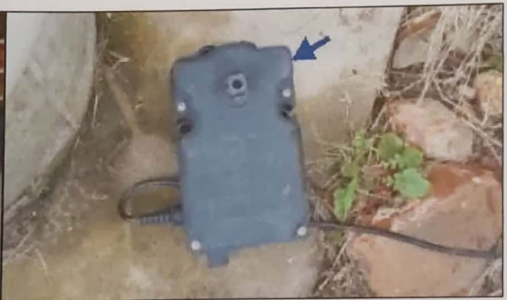
Control valve has been removed and was not operating at the time of inspection. Recommend pool specialist be consulted for further evaluation and/or repairs.
