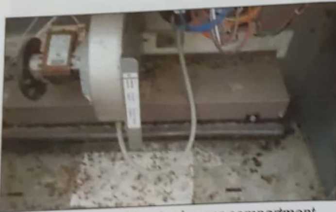
overview of pool heater burner compartment
