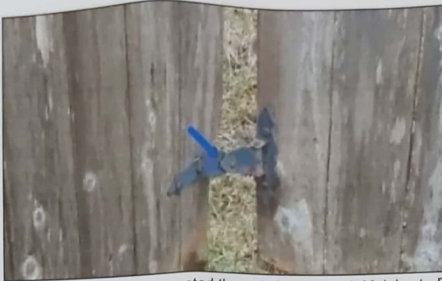
Although fences are not inspected it was noted the gate is damaged. Mainly at - Right side gates
