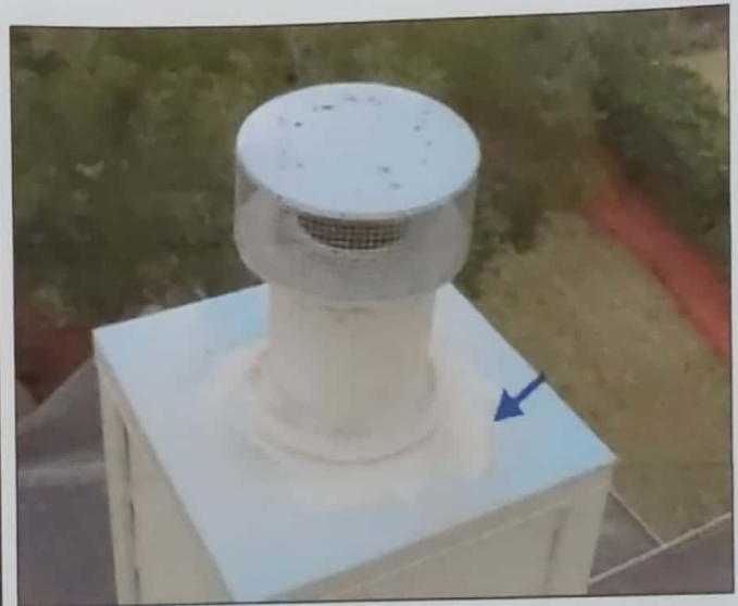
Fireplace cap was rusting paint cap to chimney to help prevent further deterioration.
