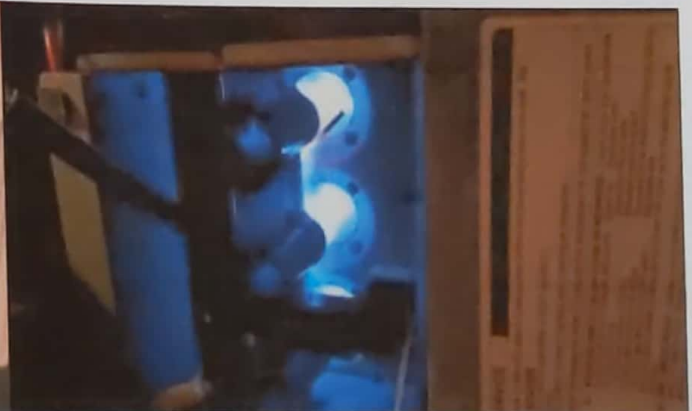
Overview of furnace burner compartment.
