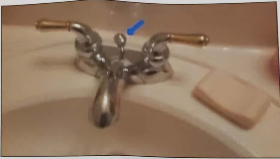
The sink drain stopper is not sealing/functioning. Mainly at - Upstairs bathroom
