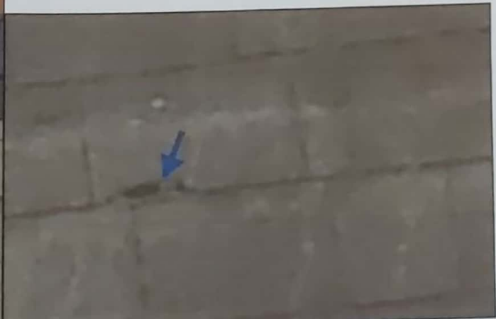
There are damaged shingles on the roof, recommend repairs or replacement of damaged shingles. Mainly at - Rear side above porch
