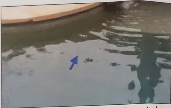
The pool light did not respond to the control.
