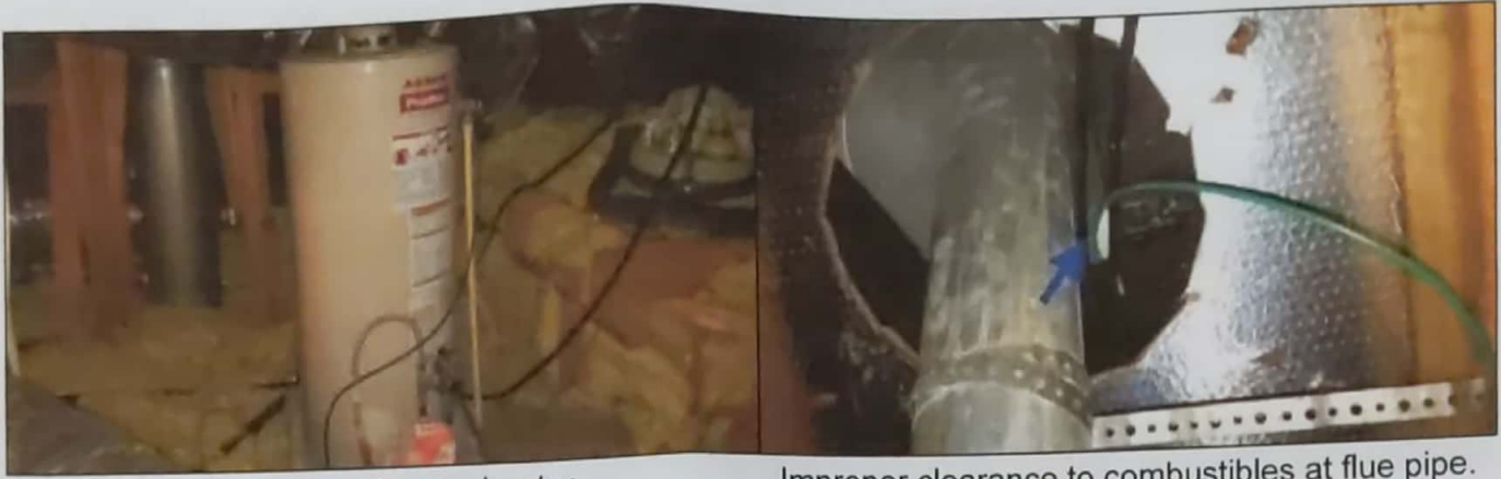
Overview of water heater
