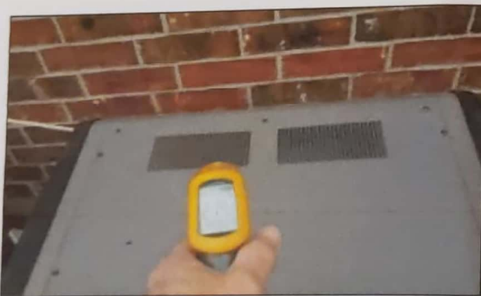
Overview of pool heater temperature
