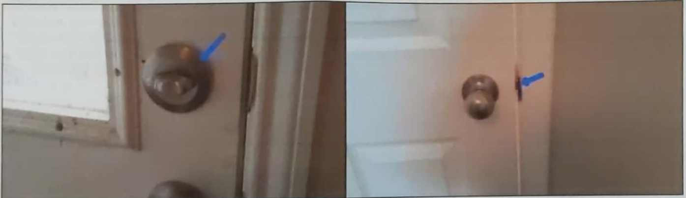
The door lock is not locking. Mainly at - Rear garage door dead bolt
