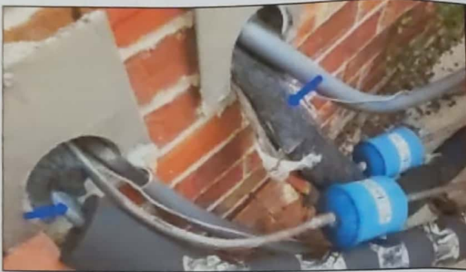
The insulation is missing or damaged on the A/C suction line at the condensing unit. Recommend repair or replacement to prevent cooling loss from exterior temperatures.
