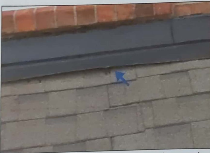
The roof flashing is lifted. Recommend resealing flashing and sealing nails to help prevent water penetration. Mainly at - Front side above garage
