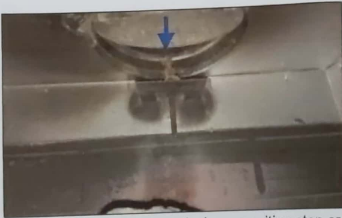
The fireplace damper is missing a positive stop or damper clamp to ensure proper ventilation for the gas logs, recommend adding damper clamp.
