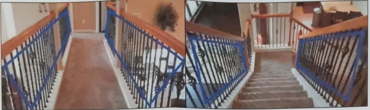
Loose balusters is noted. Mainly at - Balcony
