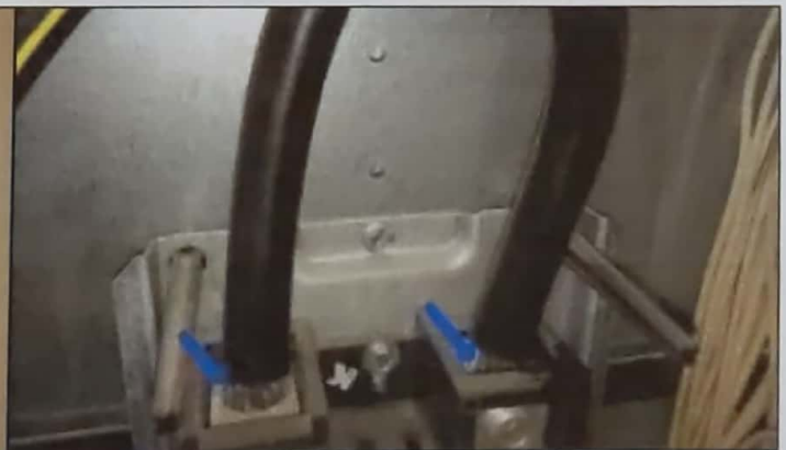
There is no antioxidant on main aluminum feeds to the panel box. This should be used to help prevent overheating.
