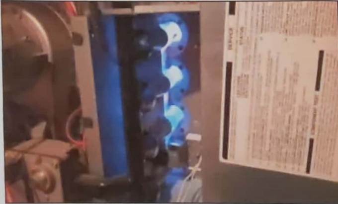
Overview of furnace burner compartment.
