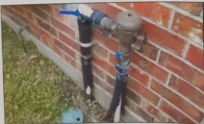
Sprinkler vacuum breaker lines insulation is damaged or missing.
