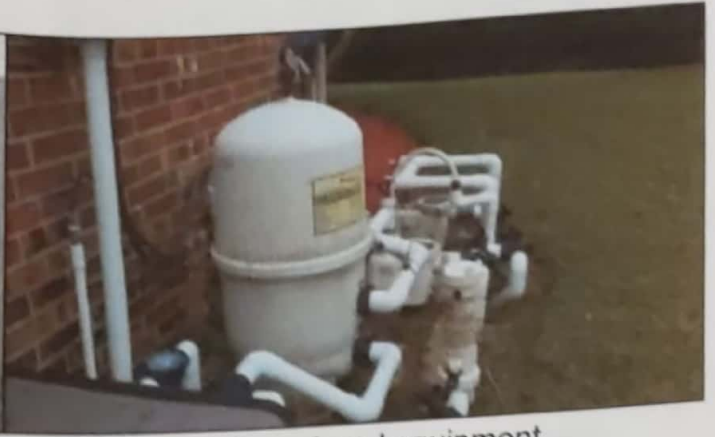
Overview of pool equipment
