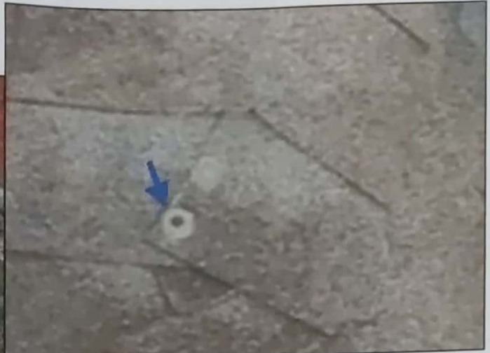
All exposed nails and fasteners on roof should be sealed at all penetrations, ridges and roof to wall connections.
