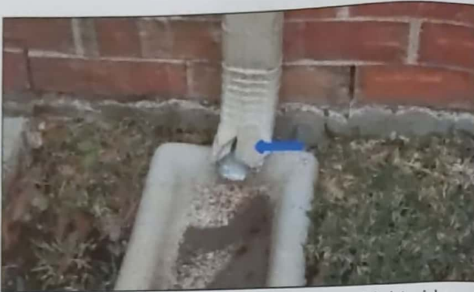
The gutter is damaged. Mainly at - Right side
