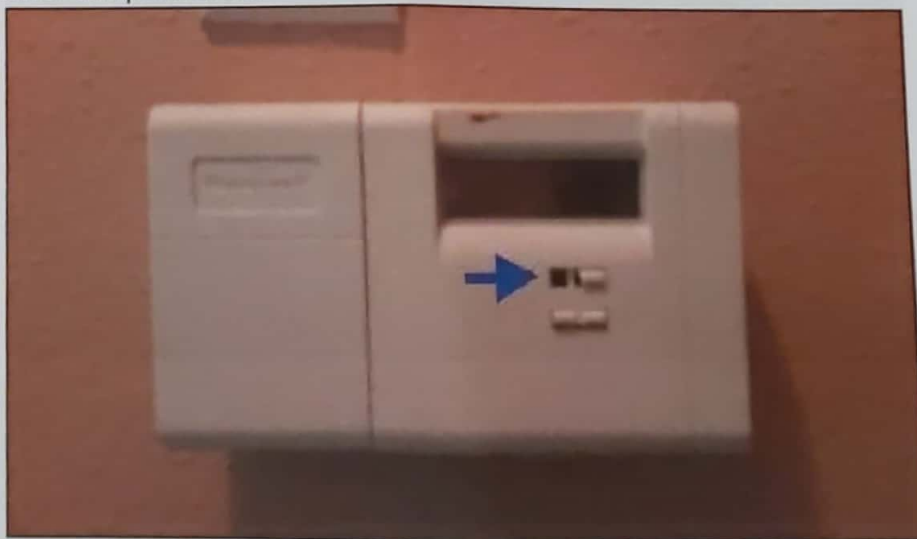
The thermostat cover is damaged. Recommend repairs or replacement as needed for proper operation
