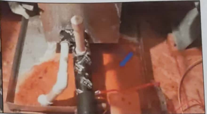
There is rust noted in the drain pan. Indications are that the pan is operating as intended at time of inspection. Upstairs unit
