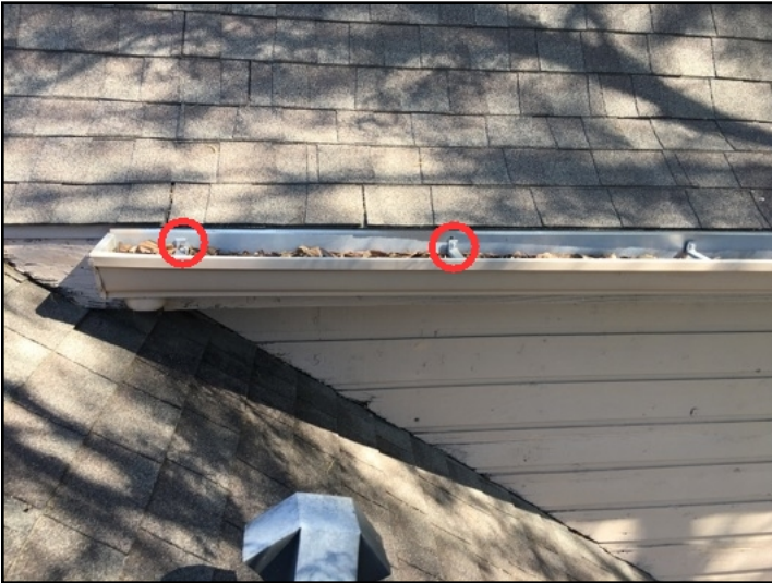
The nails/screws were coming loose and pulling out on a gutter section on the back right side of the roof
