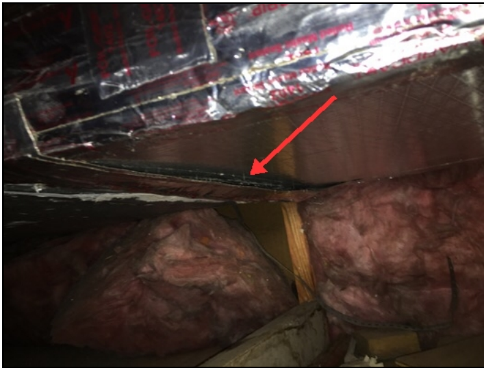
A joint in the supply plenum for the right HVAC unit was not secured properly, which was allowing conditioned air to escape
