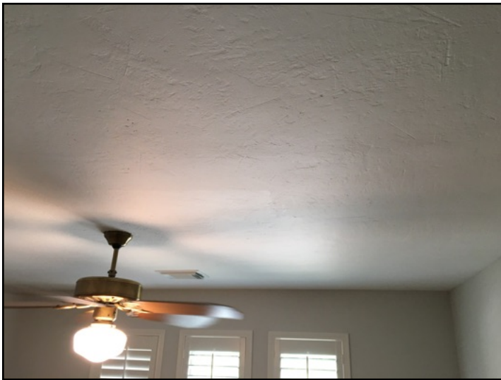
Indications of repairs (different type of texture) observed on the upstairs front bedroom ceiling
