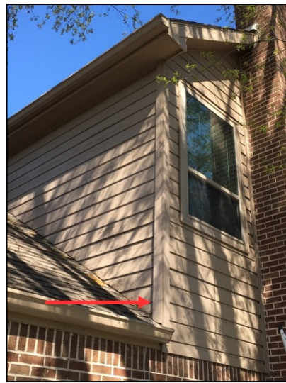
Observed loosely attached corner trim on the back side of the home
