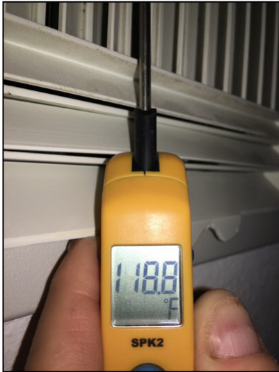
Downstairs supply temperature
