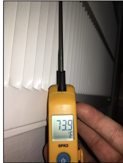
Downstairs return temperature
