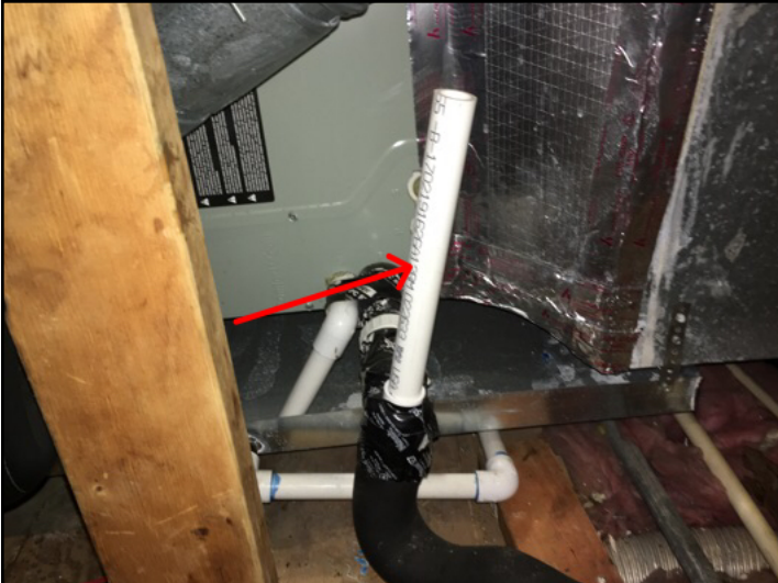
Clean-outs were installed for both AC unit primary condensate drain lines in the attic
