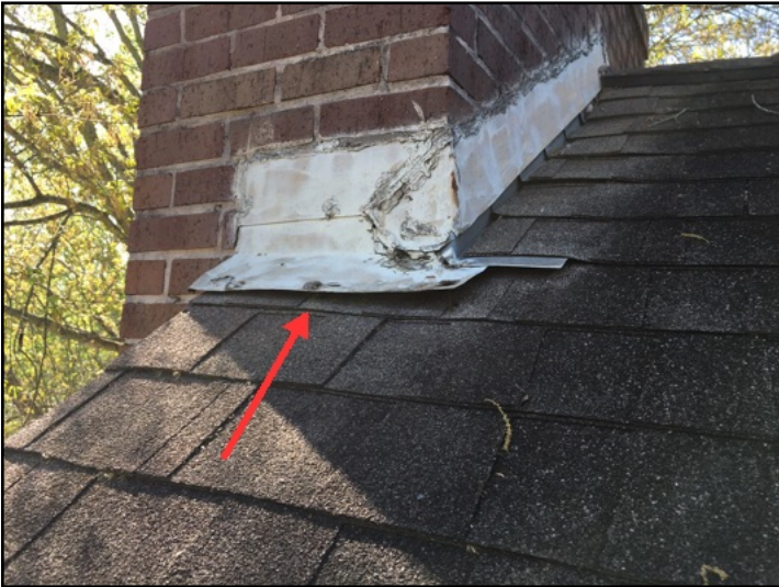
The base flashings on both sides of the chimney were lifted and should be resealed/re-secured to ensure leak free conditions
