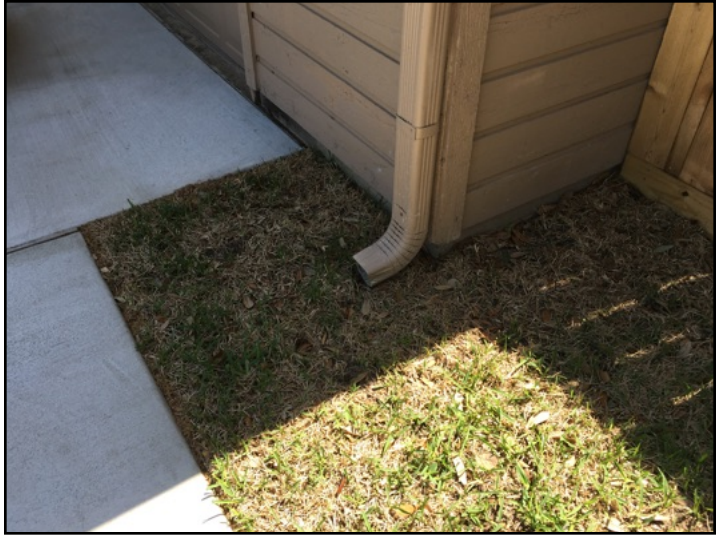
The garage slab crack may be caused by a gutter downspout (to the right of the garage door) not properly extended away from the foundation
