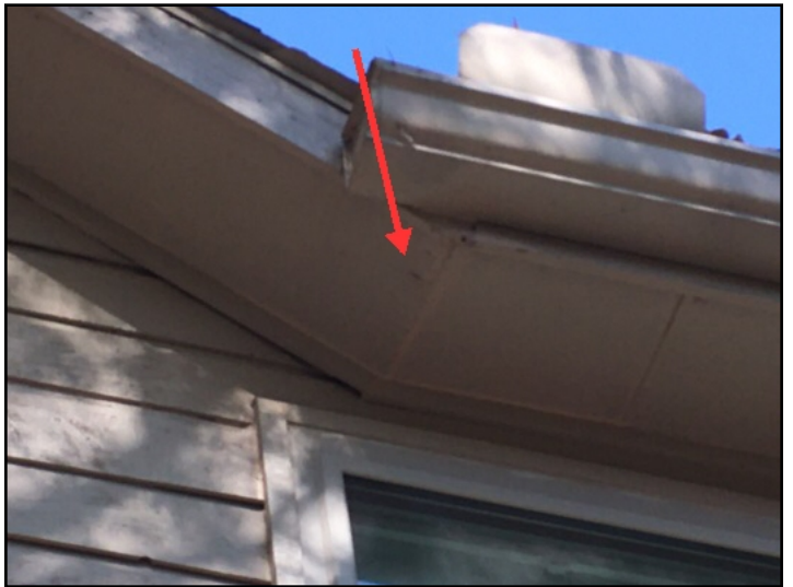
Observed a moisture deteriorated section of soffit trim on the backside of home
