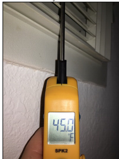
Downstairs supply temperature
