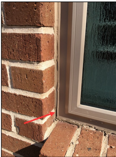
Observed areas where sealant should be applied around the windows and/or voids in the brick ledge, which penetrate the exterior veneer
