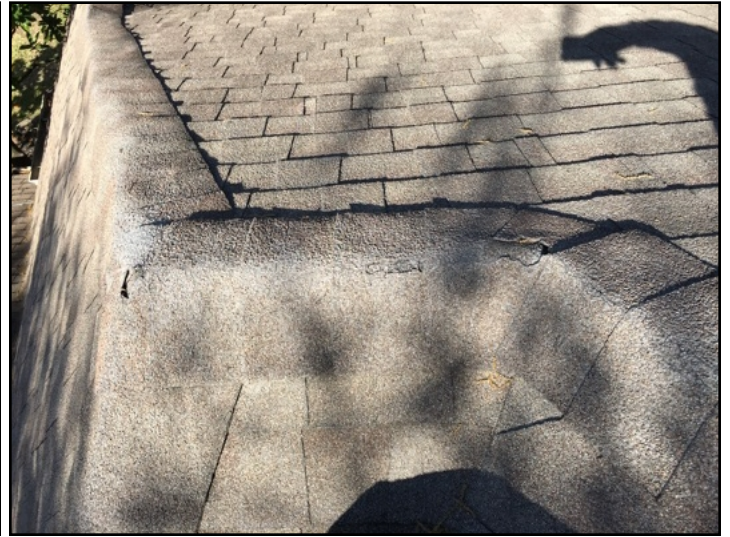
Granular loss, exposed felt and damage observed to the ridge shingles
