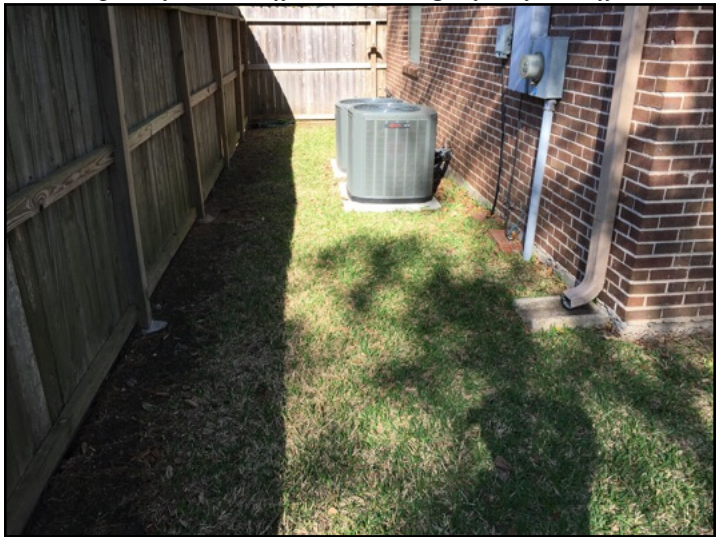
Grading appeared to be inadequate and does not slope away from the foundation on the right side of the home
