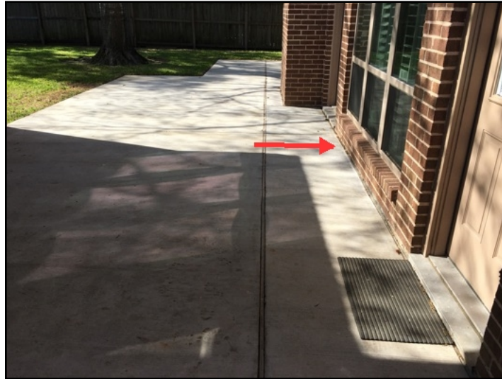
The back patio was sloping toward the home, which can cause water to settle next to the home foundation
