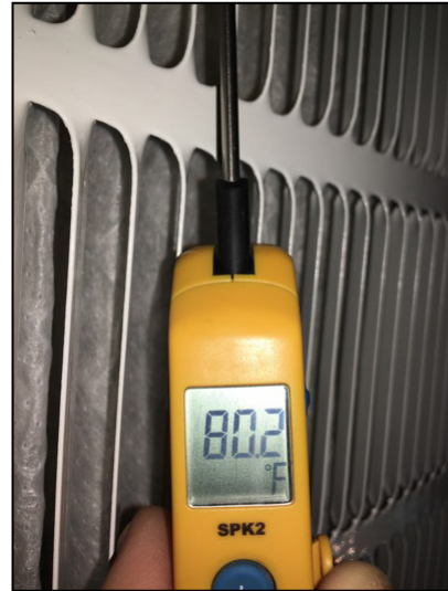
Upstairs return temperature
