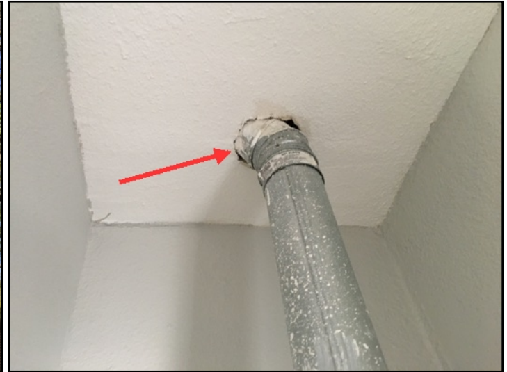
A fire-stop plate was not installed for the water heater flue vent at the ceiling penetration in the laundry room
