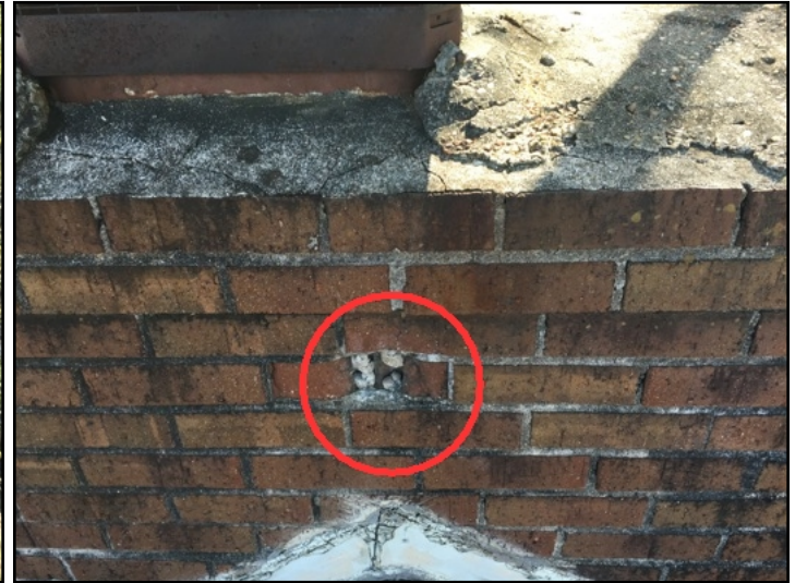
A chimney brick was deteriorated/damaged on the left side of the chimney
