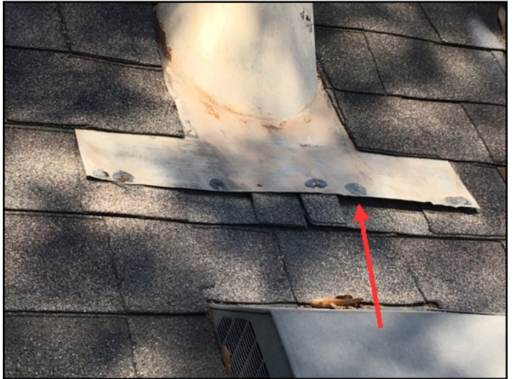
The furnace flue vent flashing on the back side of the roof was lifted and should be resealed/re-secured to ensure leak free conditions
