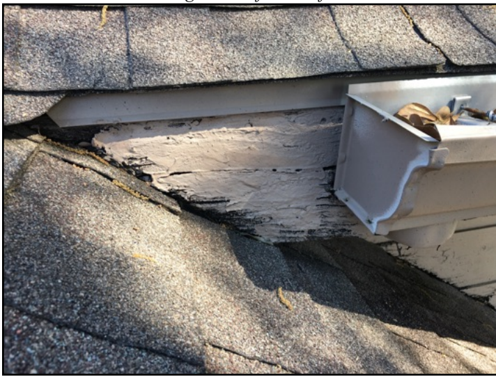
6. Observed a moisture deteriorated section of fascia trim on the back right side of the roof
