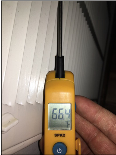
Downstairs return temperature
