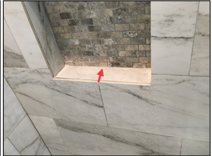
The master bathroom shower soap shelf was sloped towards the wall which can cause standing water and possible moisture penetration behind the wall
