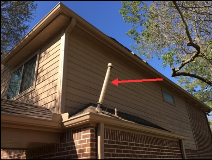
The water heater flue vent termination at the back left corner of the home was improper
