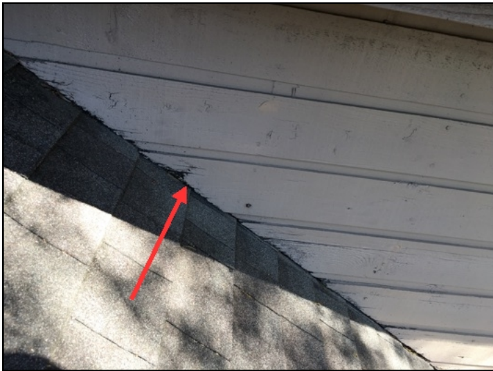
The siding had inadequate clearance between the lower edges of the siding and roof, where it intersects the roof plane on the back right side of the roof
