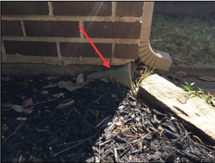
Foundation corner pops (common hairline cracks at the corner of the slab) were noted
