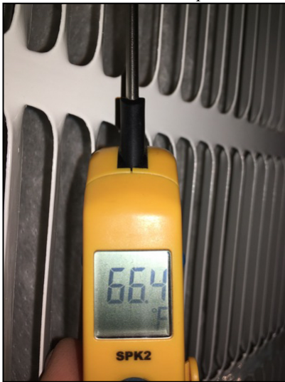
Upstairs return temperature
