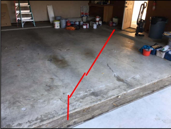
Stress crack observed on the garage slab extending from the garage door to the garage side door and penetrating the foundation beams at both locations
