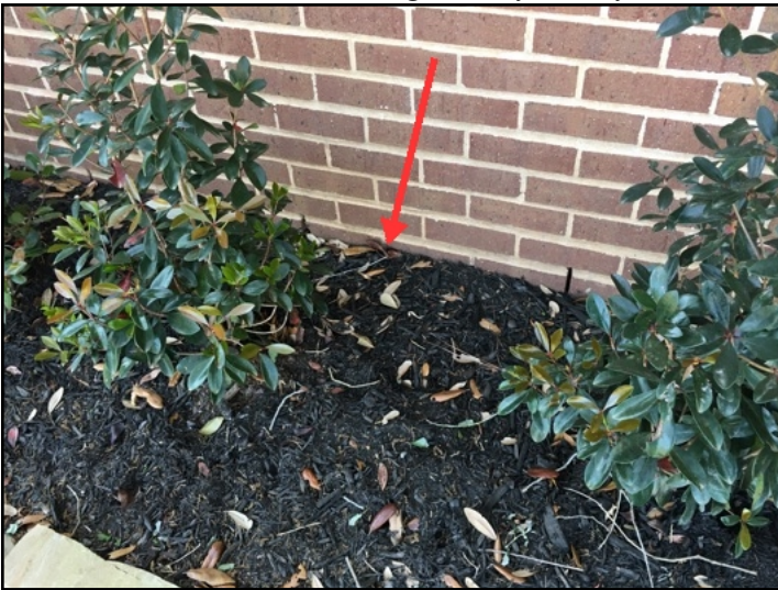
Areas next to the foundation on the left side of the home had high soil that may allow water/insects in
