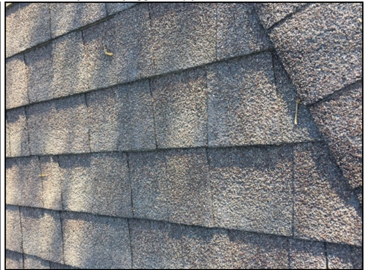
Granular loss (and loose granules) observed on the roof shingles
