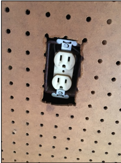
Observed missing receptacle cover plates in the garage
