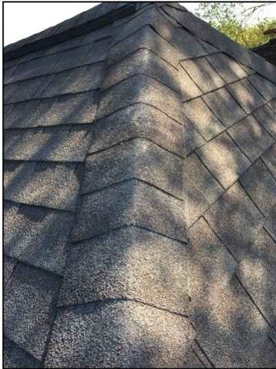
Granular loss, exposed felt and damage observed to the ridge shingles
