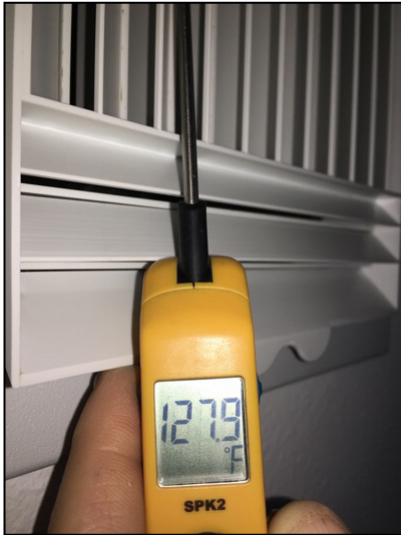
Upstairs supply temperature
