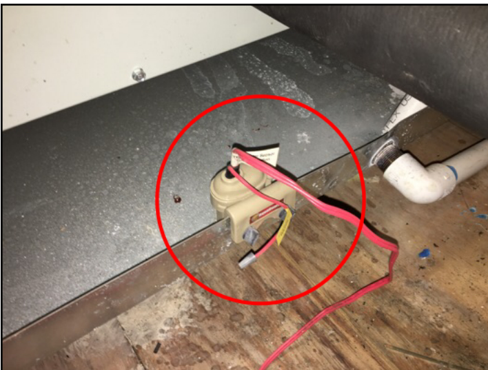
Float switches were installed for both AC unit overflow pans in the attic, which will turn the units off if the overflow pans fill with water
