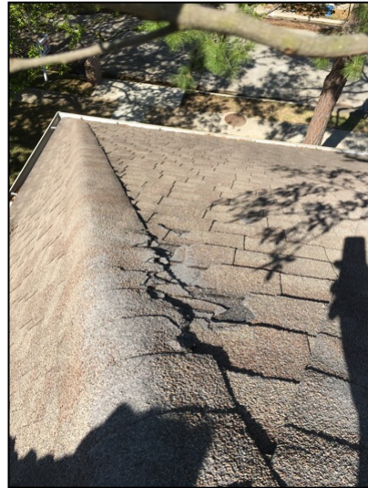
Damaged hip shingles and roof shingles observed on the front side of the roof apparently from tree abrasion
