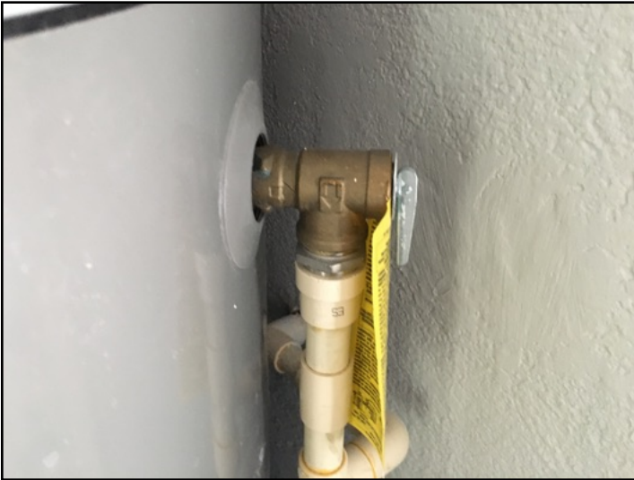
Water heater TPR safety valve
