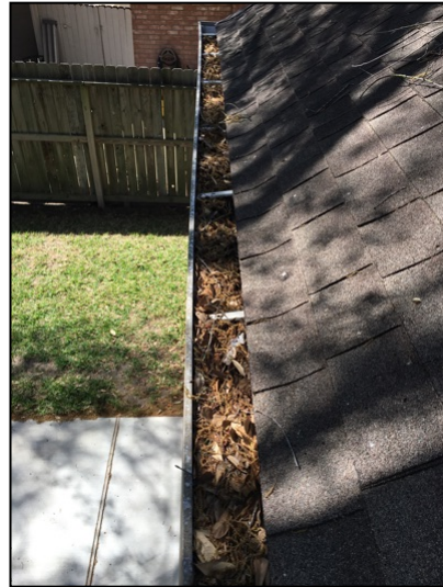
Recommend leaves and debris be cleaned from gutters and downspouts for more effective drainage of roof run-off water
