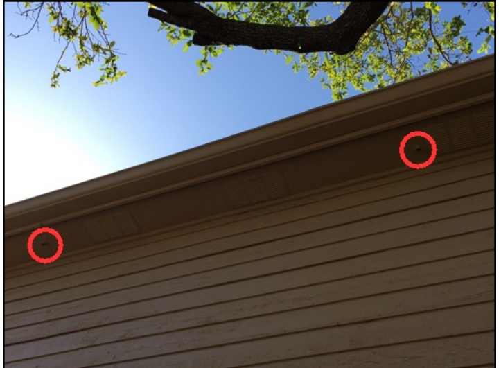
Overflow pans and drain lines were installed for both A/C units in the attic and the drain lines exited at a high location on the left side of the home
