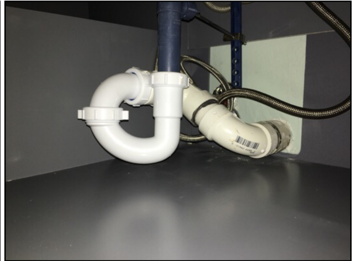
An improper S-trap was installed for the half bathroom lavatory
