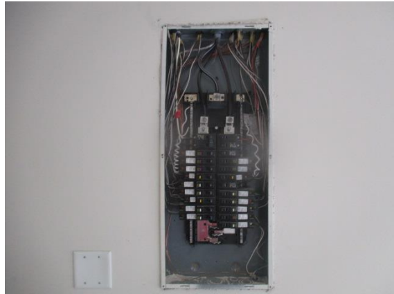
4. Electric Panel Interior
