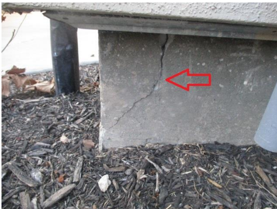
17. Crack at right front corner
