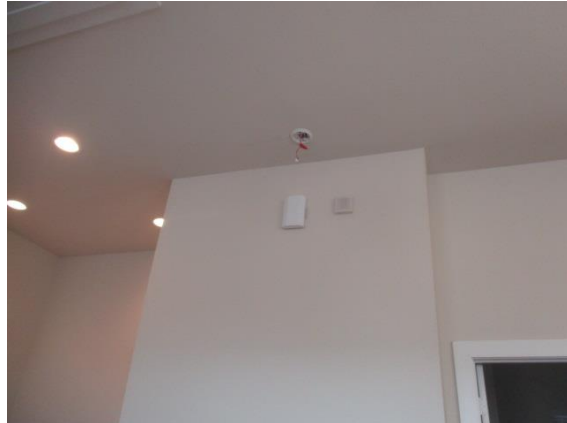
20. Missing smoke detector
