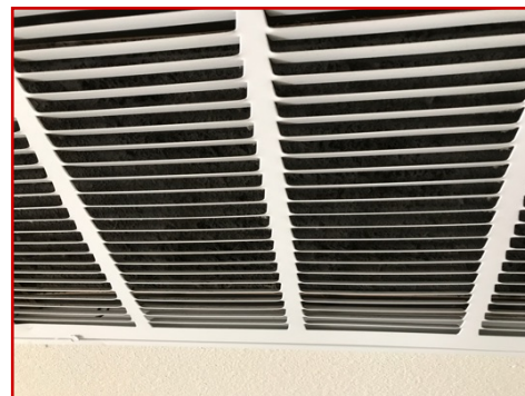
Downstairs return, very dirty filter
