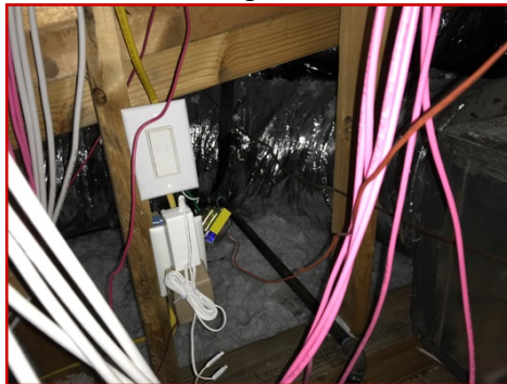
Attic outlet and furnace shutoff
