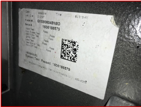
Amana natural gas furnace, mfg 2016
