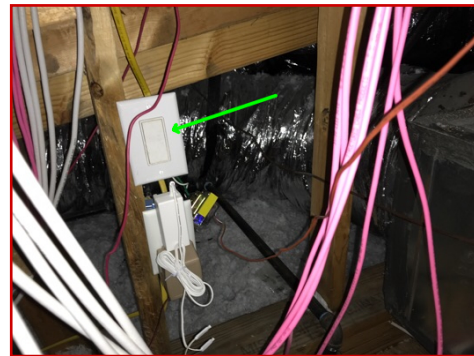
Furnace electrical shutoff
