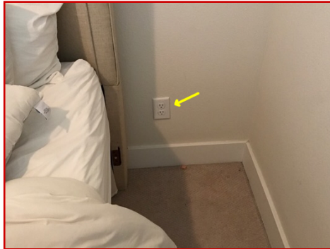
Loose outlet in downstairs bedroom
