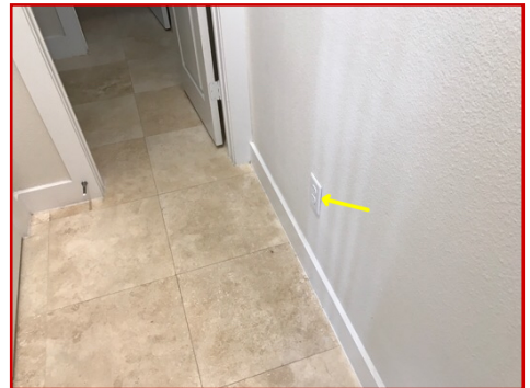
Loose outlet by downstairs bathroom
