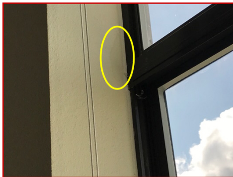
Signs of past moisture intrusion in down stairs bedroom window
