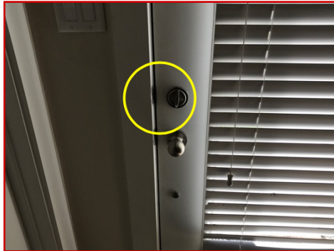
Main entry door rattles when closed
