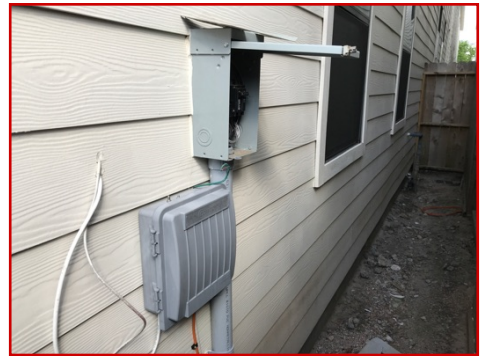
Additional 125 amp shutoff on rear of structure
