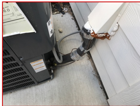
Lines are properly insulated
