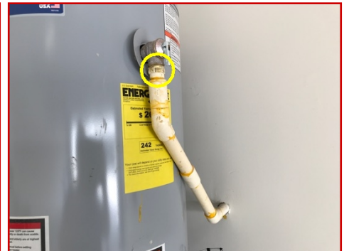
TPR valve coupler is wrong material
