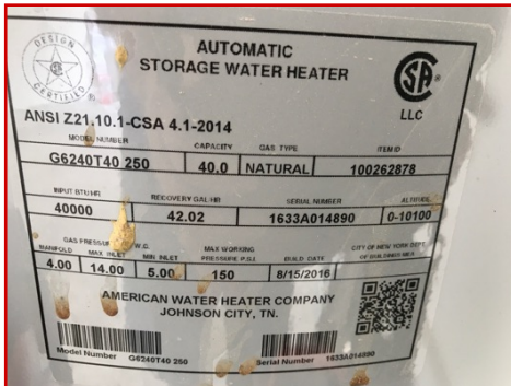
American, 40 gal natural gas water heater, mfg 2016
