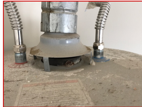
No visible corrosion at water connections
