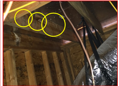
Signs of moisture intrusion
