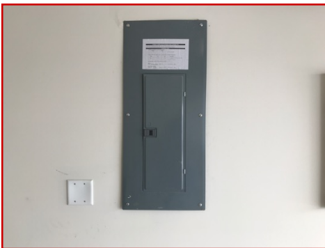
Main service panel in garage
