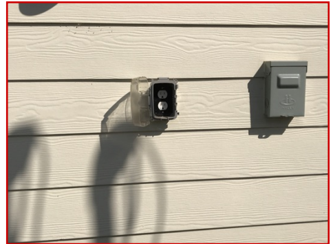
AC outlet, weather protected, no GFCI
