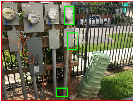
Service shutoff, meter and driven rod ground
