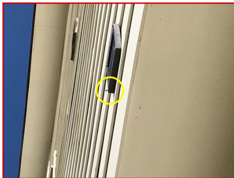
Loose fastener on bath fan cover
