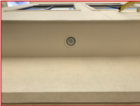
Exterior garage light did not respond
