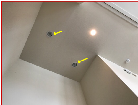
Unresponsive light fixtures
