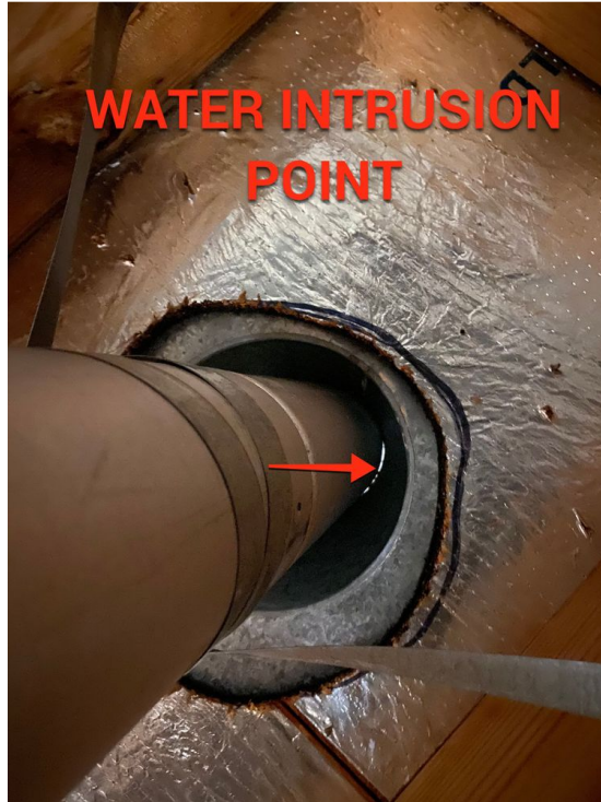
Water intrusion point through an HVAC pipe.
