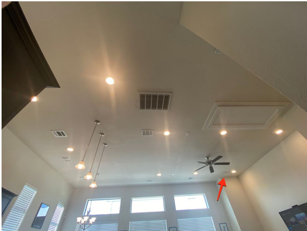
Water marks due to leak on ceiling.
