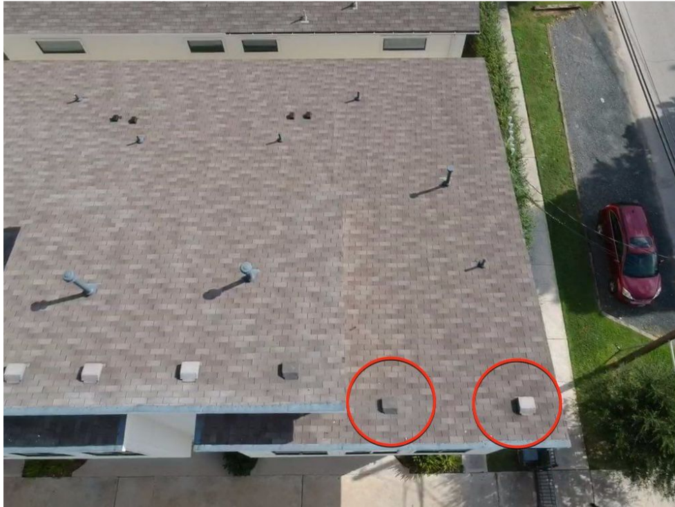
Leaking square vents
