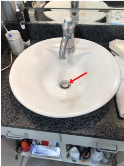
The drain stop did not properly hold water in the primary bathroom left sink.
