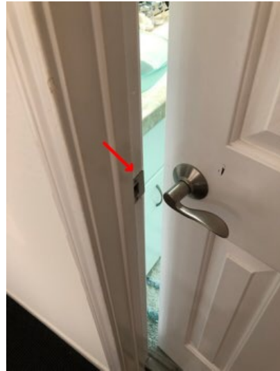
The door does not latch at the kitchen, second-floor bathroom, second-floor front left bedroom closet.
