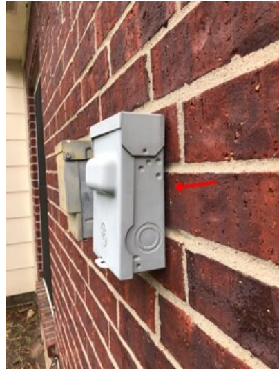
Recommend caulking around all exterior wall penetrations.
