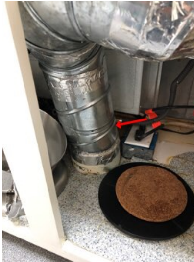
There was an air leak from the range hood vent.
