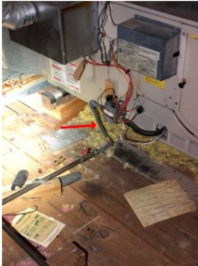
Missing drip legs on the gas lines for both units. These help prevent sediment in the gas line from entering the units.
