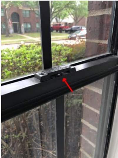
Multiple locations where the window hardware was damaged.
