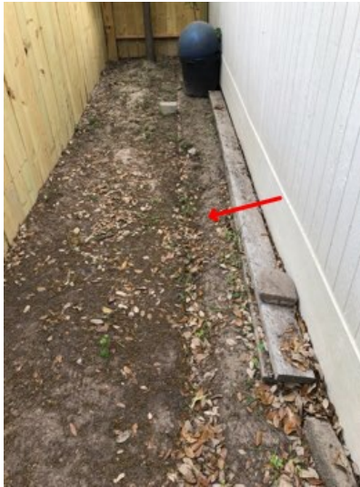
Soil erosion was observed during the inspection. Location: rear, garage
