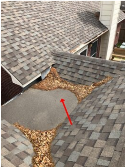
Recommend removing debris from the roof covering. Unable to determine the condition of the roof covering underneath.
