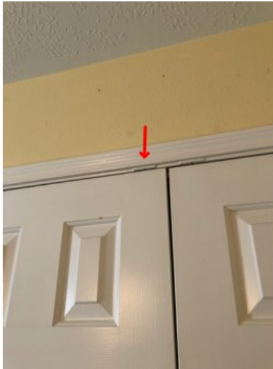
The door does not latch at the kitchen, second-floor bathroom, second-floor front left bedroom closet.
