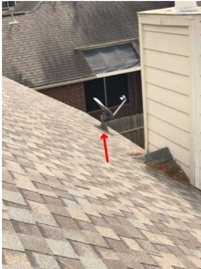
The condition of the roofing materials under the satellite dish could not be determined.
