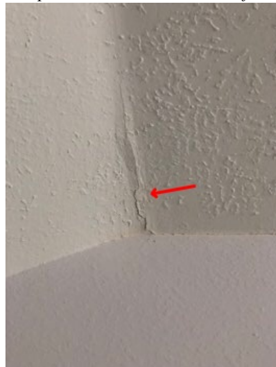
Cosmetic cracks were noted at the first floor living room and second floor left rear bedroom.
