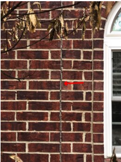
Multiple locations where the expansion joint sealant was deteriorated.
