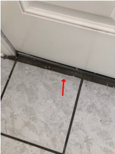
Cracked tiles were noted at the front entry and laundry area.
