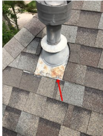
Attic vent is rusted.
