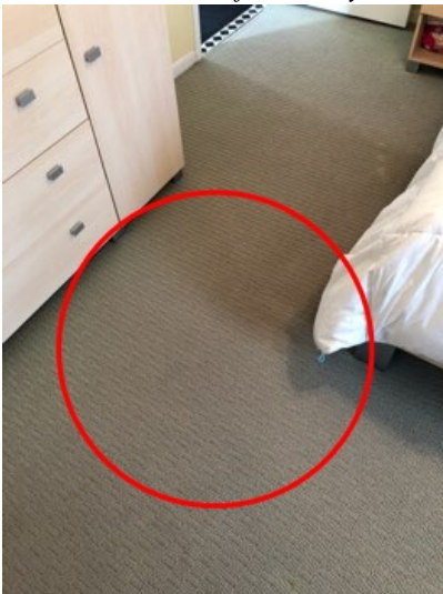
Areas on the second floor where the subfloor was squeaky when stepped on. This is due to the subflooring Not properly fastened to the joist.
