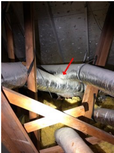
There were ducts in contact with one another.
