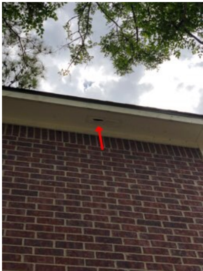
There were damaged soffit vent screen(s).
