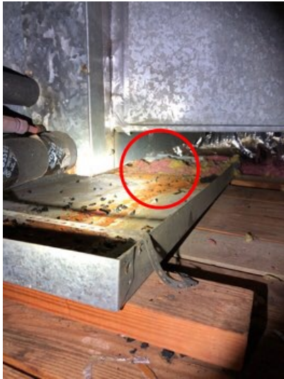
There was rust and insulation inside one of the drain pans.
