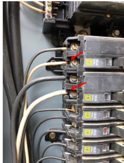
There are white wires in the panel that should be labeled as hot wires.
