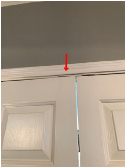
The door does not latch at the kitchen, second-floor bathroom, second-floor front left bedroom closet.
