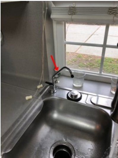
The pot filler in the kitchen did not work.
