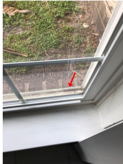
Cracked window panes were observed at the first floor living room.
