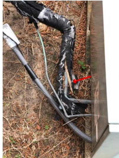
The insulation on the refrigerant lines was deteriorated.
