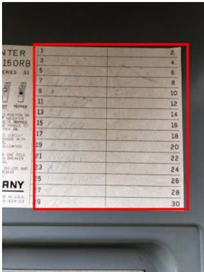
The circuit labels are worn and difficult to read.
