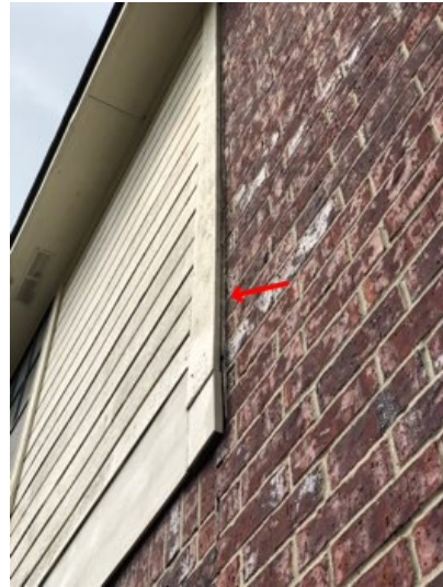
Recommend caulking around all exterior wall penetrations.
