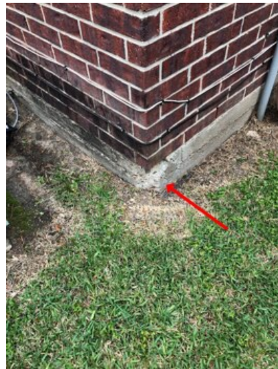
There was a shear crack in the foundation. These are cosmetic and are not associated with structural movement. Location: front, rear
