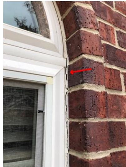
The sealant around the window on the right side was deteriorated.
