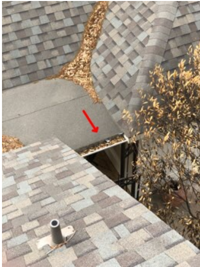
The gutters have debris in them.
