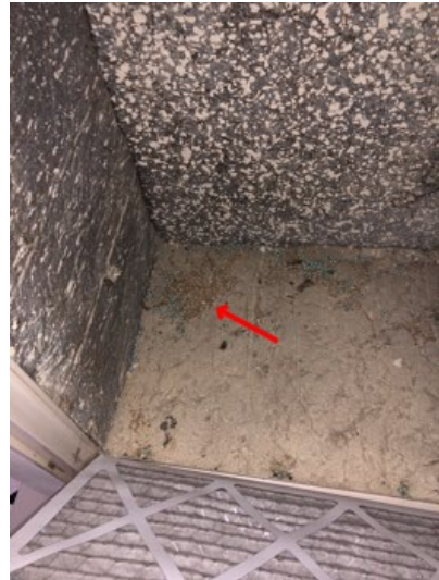
There was dust inside the return chase on the first floor.
