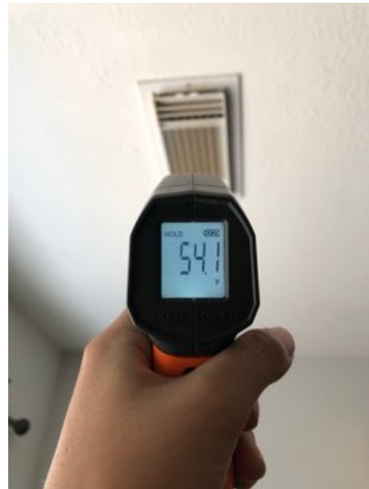
Cooling system was functioning.
