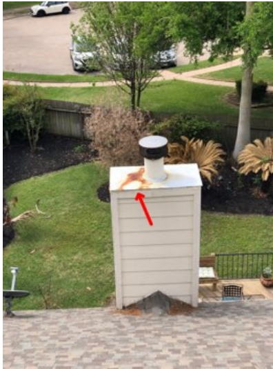
The chimney cap was rusted.
