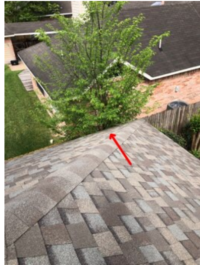
Trees in contact with/hanging near the roof.
