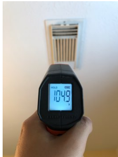
Heater was functioning.
