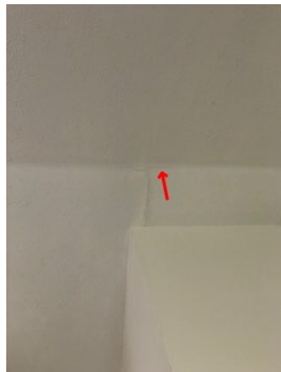
Cosmetic cracks were noted at the first floor living room and second floor left rear bedroom.
