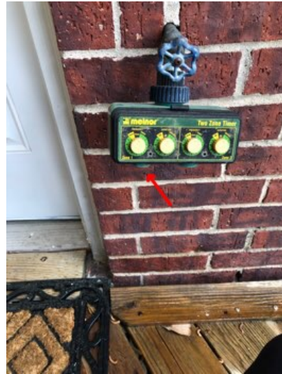
An exterior water faucet was dripping at the rear of the house.
