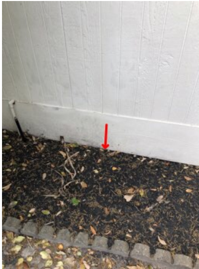
High soil was observed at the front and the garage. There should be 4 inches of slab showing for brick and 6 inches for siding.
