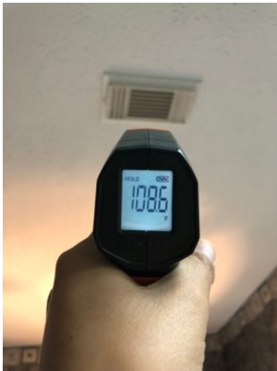
Heater was functioning.
