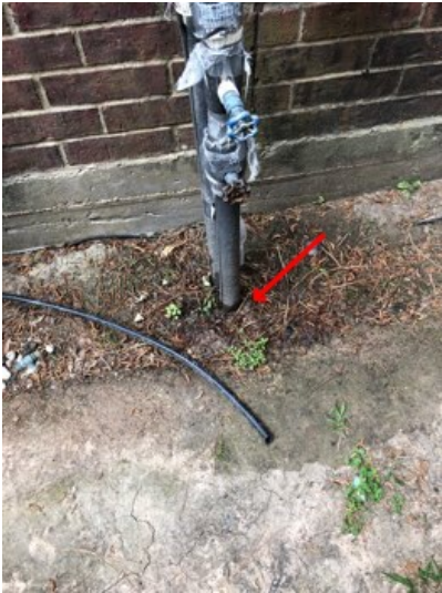
There was a leak from the piping on the left side of the house.
