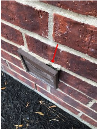
Recommend caulking around all exterior wall penetrations.
