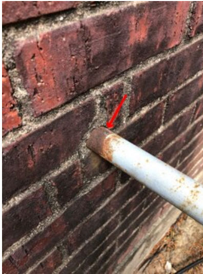
The gas service line entering the house was rusted.
