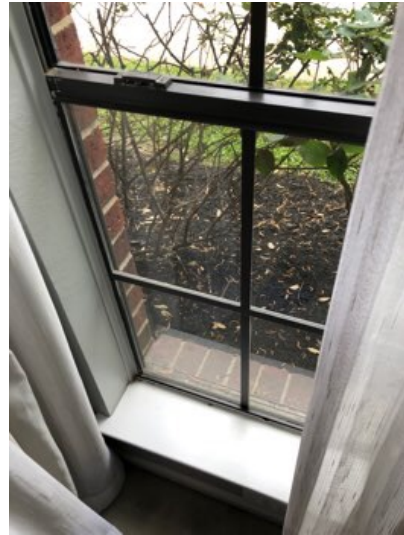
Missing window screens for the windows at the front and right of the house.
