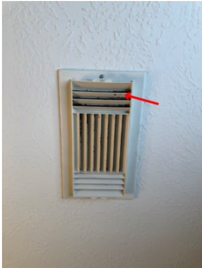
There was a dark substance on the registers on the second floor. This can be due to an excessive amount of humidity in the system at times.
