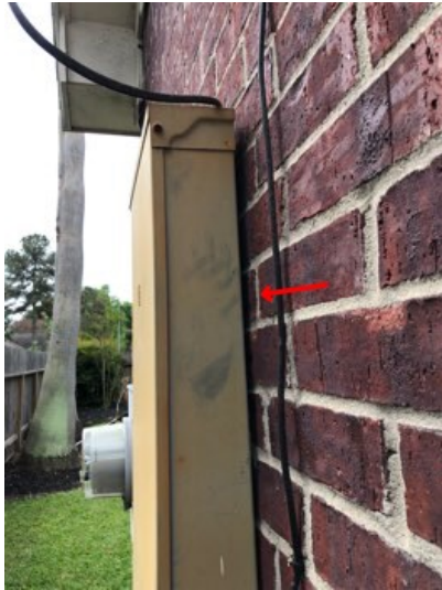
Recommend caulking around all exterior wall penetrations.
