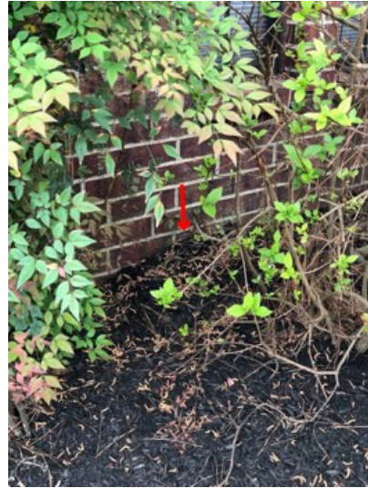
High soil was observed at the front and the garage. There should be 4 inches of slab showing for brick and 6 inches for siding.
