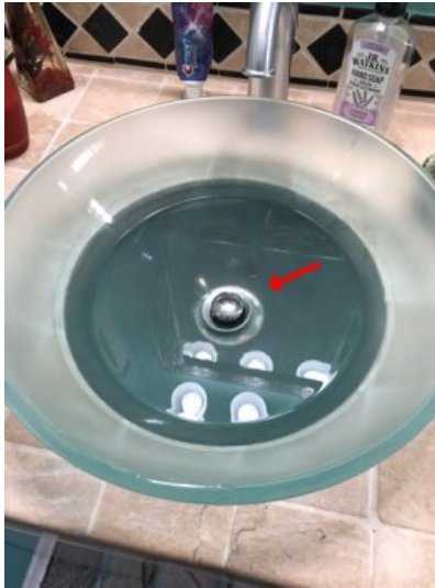
The second-floor bathroom left sink drained slowly.
