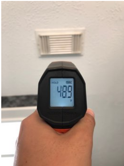
Cooling system was functioning.
