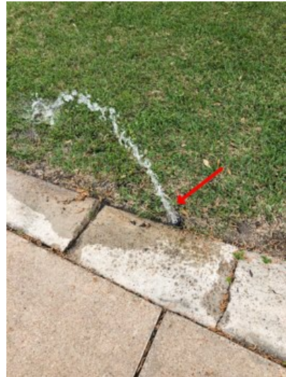
Multiple locations where the sprinkler heads were broken.
