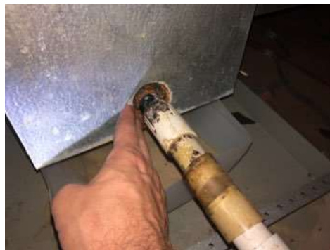
Unit 1: air leak at cabinet
