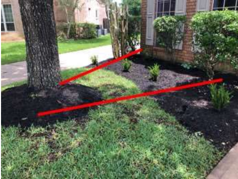
Front: tree roots near foundation
