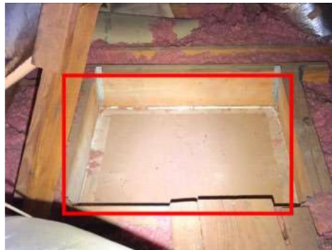
Scuttle panel lacked insulation
