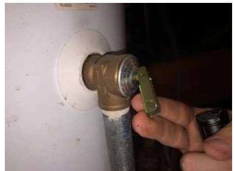
FYI: Test TPR Valve yearly
