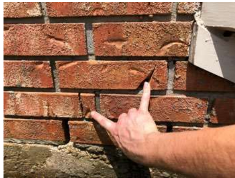
Right: step crack
