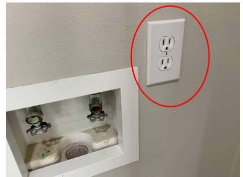
Laundry Room: outlet not GFCI
