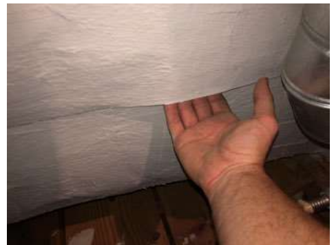
Unit 2: air leak at cabinet
