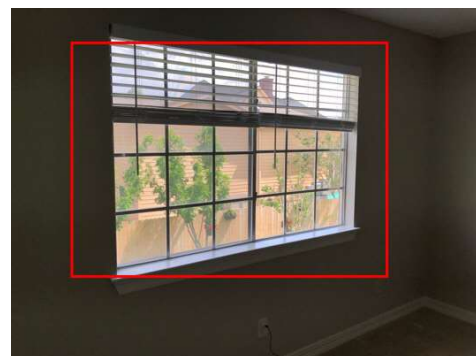
Bedroom 3 and Bedroom 4: windows inoperative
