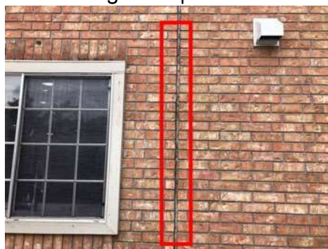
Left: missing caulk at expansion joint
