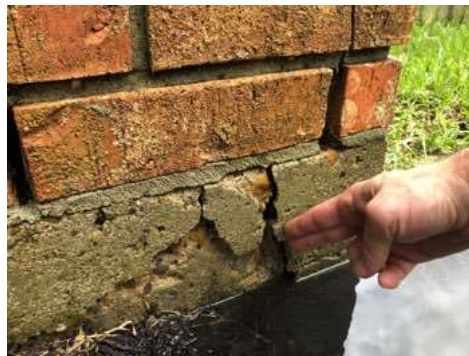
Right front: corner crack
