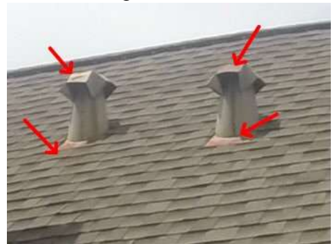
Rust on flashings
