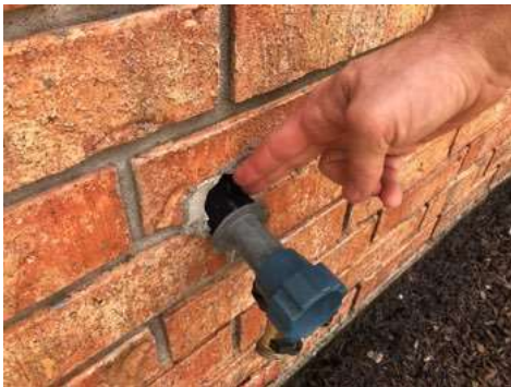
Around house: caulk needed at wall protrusions
