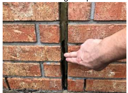
Left: wood decay at expansion joint spacer
