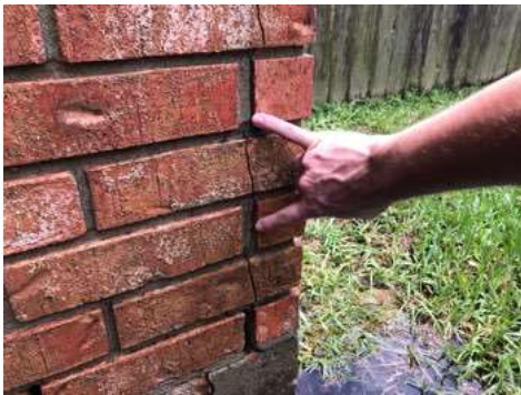
Right front: step crack
