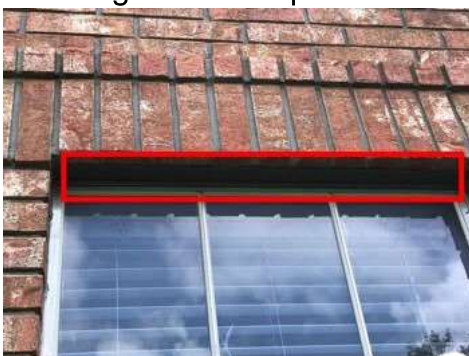
Front: rust on lintels
