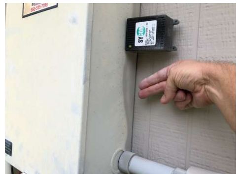
Service panel : Caulk missing at wall connection
