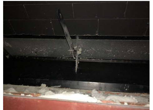
Flue closed: Clamp missing on damper
