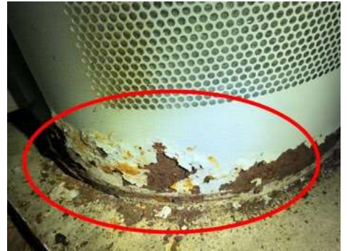
Unit 1: corroded tank
