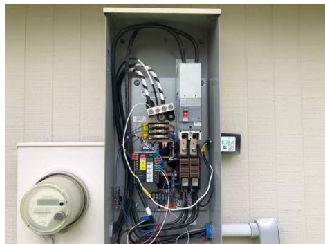
Garage rear: service panel with dead front removed
