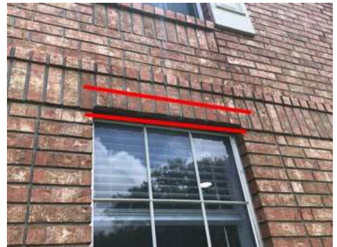
Front: missing weep holes
