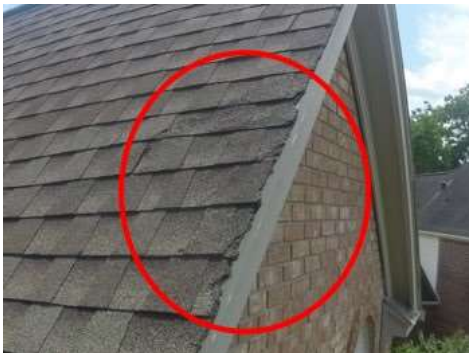
Front: damaged shingles
