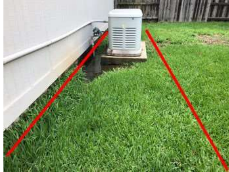
Garage rear: insufficient grading
