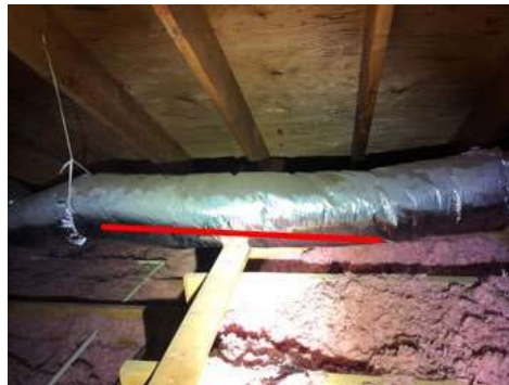
Duct on attic floor
