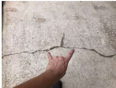
Back porch: hairline crack
