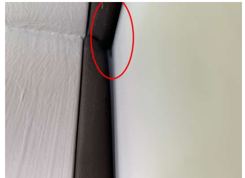
Back door: did not close flush.
