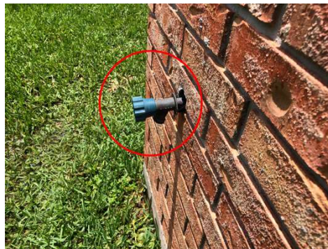
Around house: Missing back flow preventer
