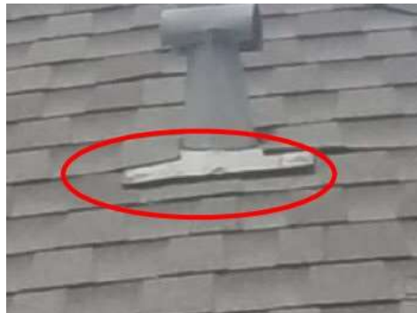
Right: uplifted flashing
