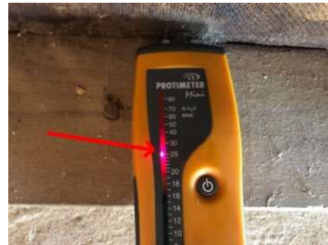
Garage: moisture stains confirmed wet
