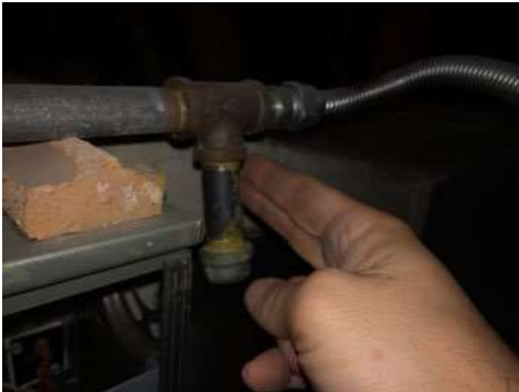
Improper drip leg installation
