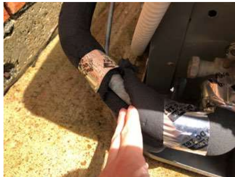
Both units: Old and deteriorated refrigerant line insulation
