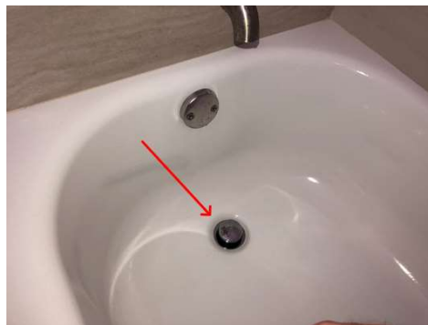
Bathroom 2 : inoperable stopper
