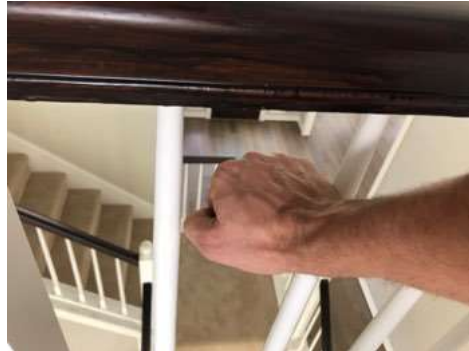
Guardrail: Spindles more than 4" apart
