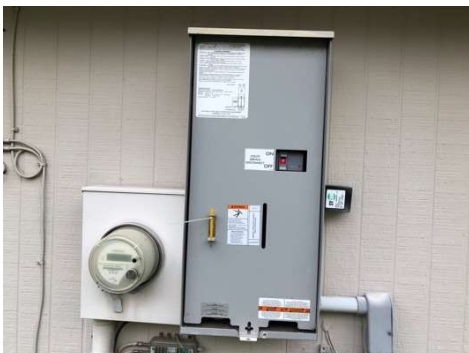
Garage rear: generator service panel
