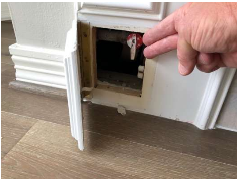
No locking mechanism on valve hatch
