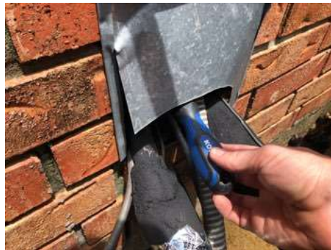
Right: hole in wall at AC lines
