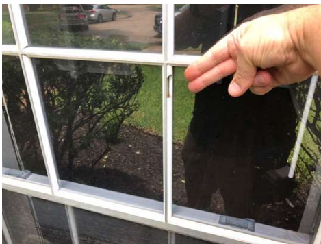
Around house: Damaged weather stripping
