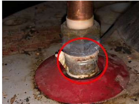
Both units: corroded fittings
