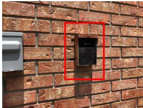
Unit 2: missing deadfront at disconnect
