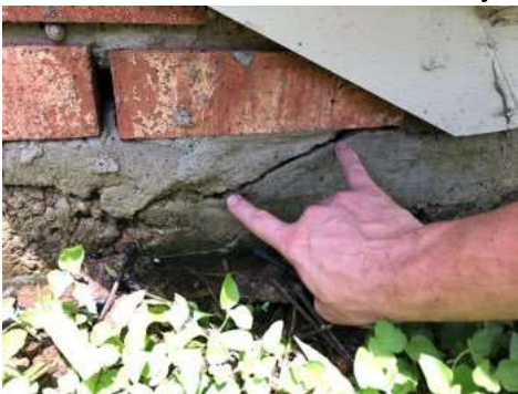
Right: crack with displacement
