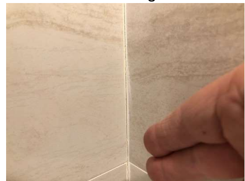
Bathrooms: cracked grout
