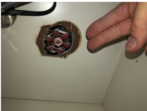
Kitchen cabinet Left: Main Water Shutoff Valve
