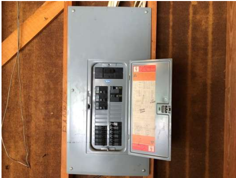
Garage: sub panel
