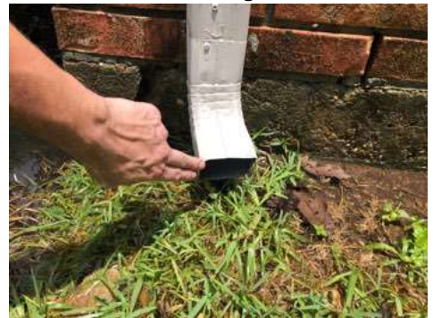
Downspout extension missing, discharge near structure
