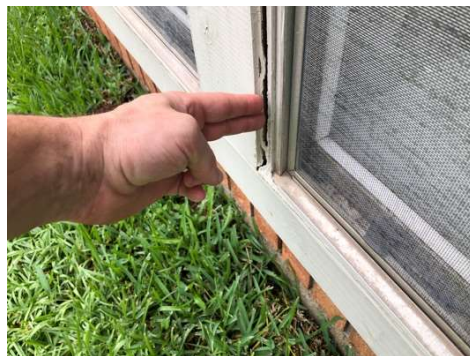
Around house: deteriorated caulk
