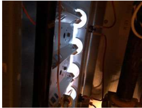
Furnace 1 fired up
