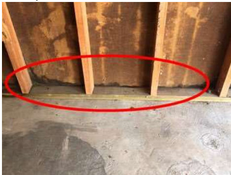
Garage: moisture stains
