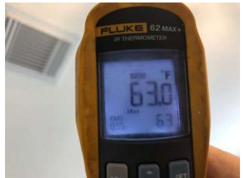
1st floor: vent temperature
