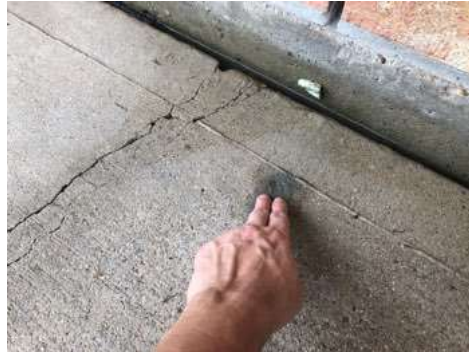
Rear: evidence of prior wood destroying insect treatment
