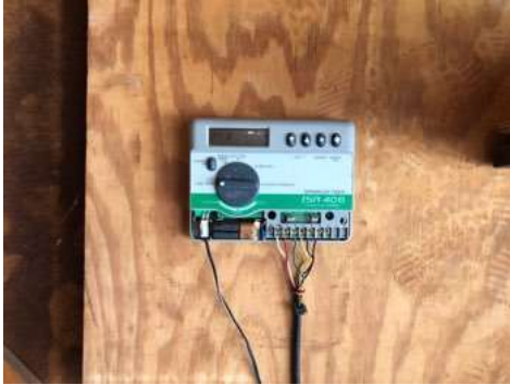
Garage: controls to sprinkler system
