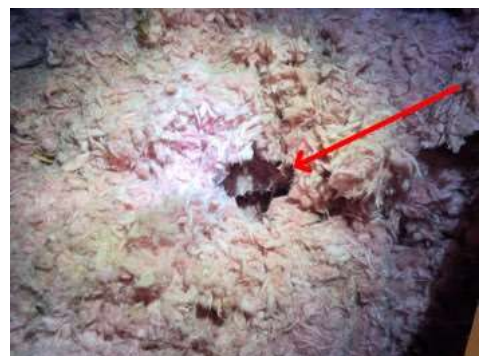
Tunneling: evidence of vermin activity
