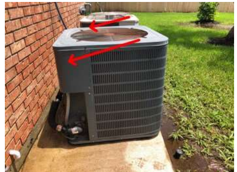
Both units: out of level
