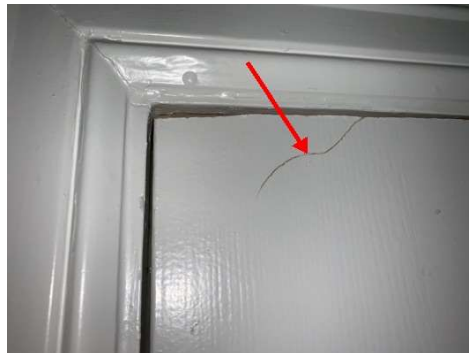
Bathroom 2: Damaged door
