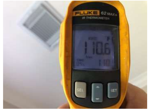
1st floor hot air temperature
