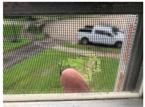
Throughout house: Damaged screen
