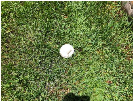
FYI: Main Cleanout located on the rear
