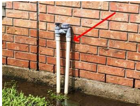
Right: Backflow preventer
