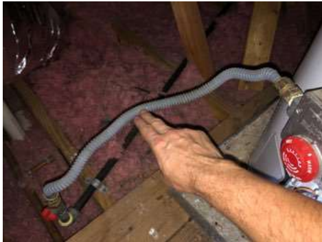
Both units: missing drip leg
