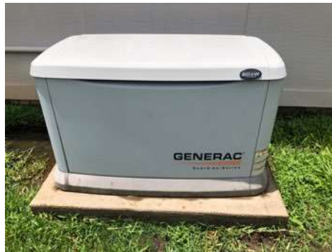
Garage rear: whole house generator
