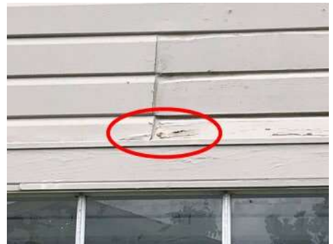
Rear: wood decay at siding
