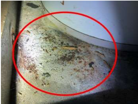
Both units: debris in safety pan
