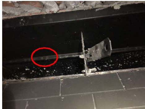
Flue open, missing clamp
