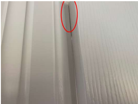
Bedroom 1: rubbed on frame
