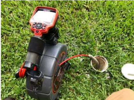
Point of entry: main cleanout
