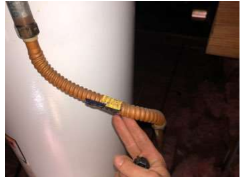
Both units: Improper material for TPR extension pipe
