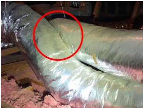
Ducts in contact
