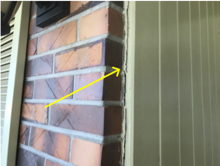
Deteriorated sealant at siding transition
