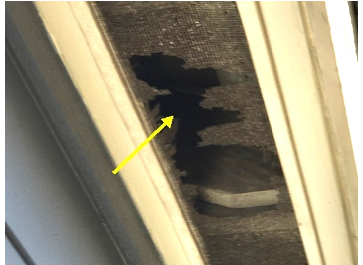
Damaged soffit vent at rear of garage
