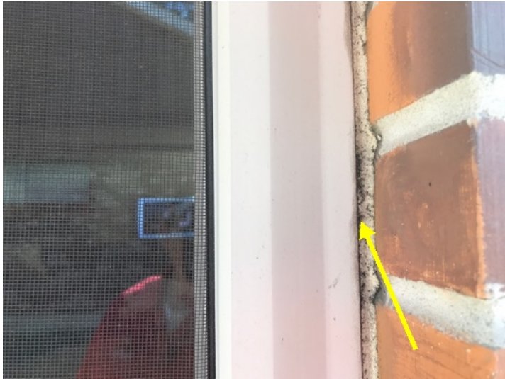
Deteriorating window sealant
