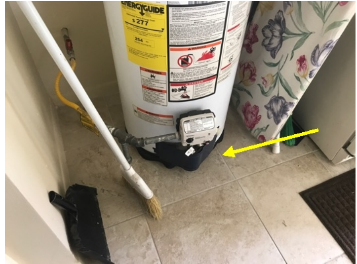
Missing Emergency drain pan
