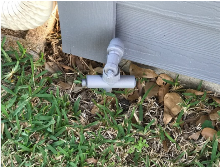
Damaged exterior faucet (left rear corner of garage)
