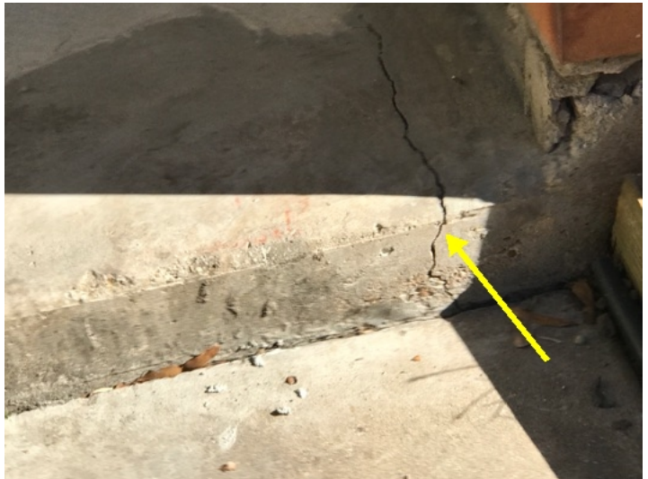
Cracks found at various places at front porch
