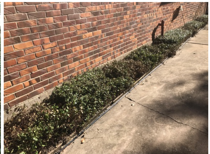
Heavy vegetation against slab
