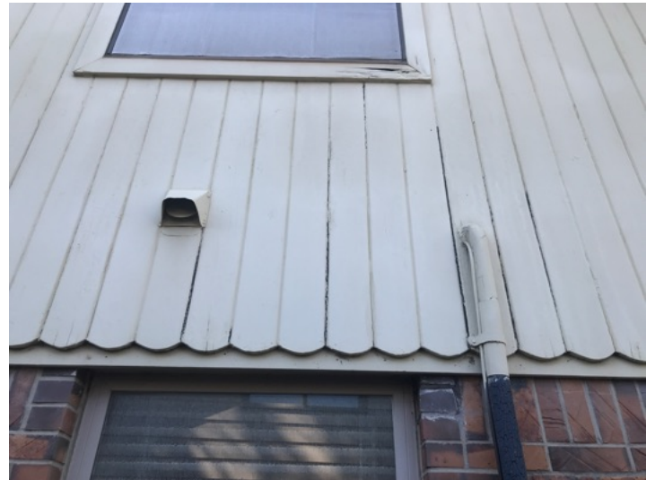
Siding butt joints need sealant
