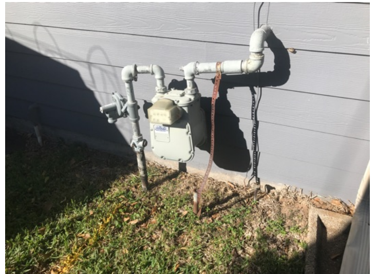
Gas meter at rear side of garage
