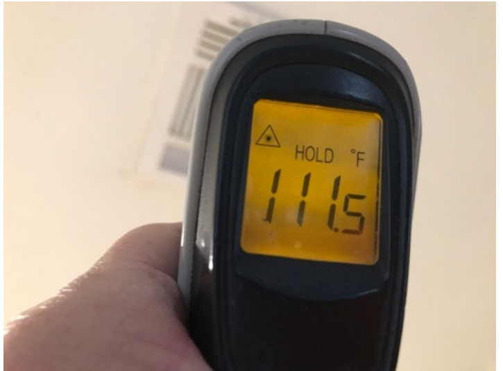
Furnace air temperature at supply air register
