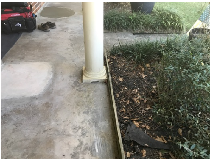
Signs of previous foundation work on house
