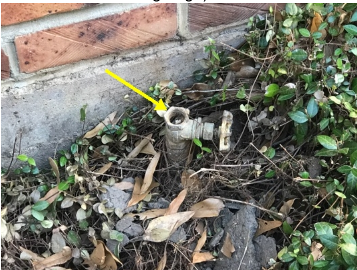
Faucet at right side of house inoperative
