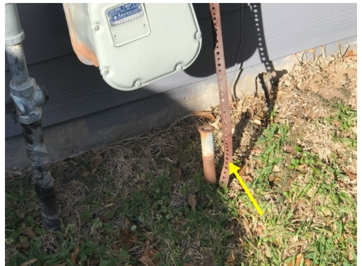
Gas meter not grounded
