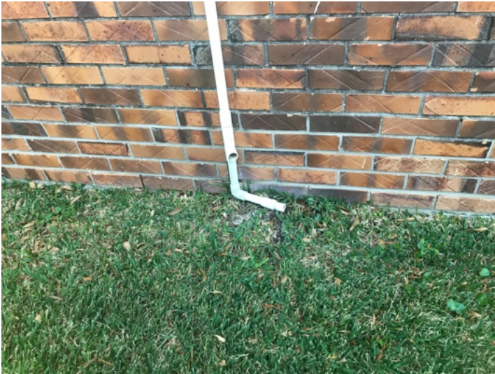
A/C discharge line terminates at slab
