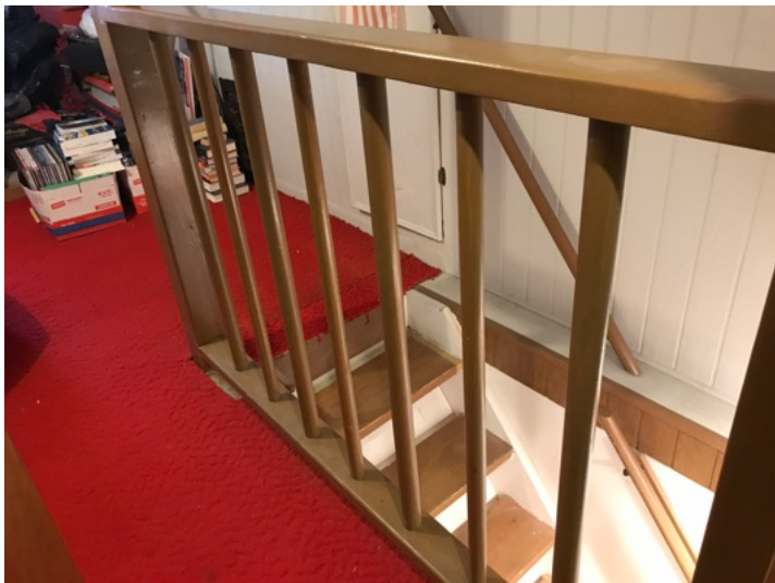
Hand railing balusters spaced too far apart
