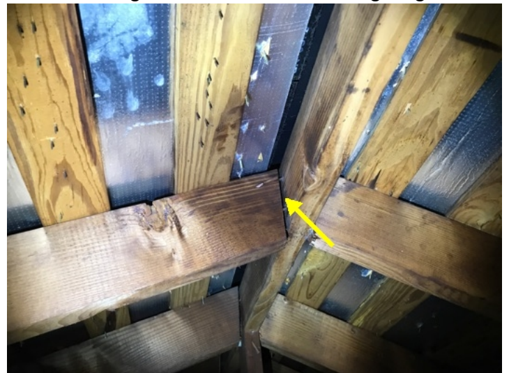
Rafters not adequately secured to ridge board
