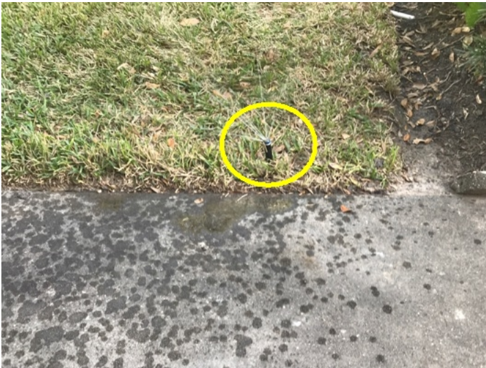
Sprinkler head would not oscillate
