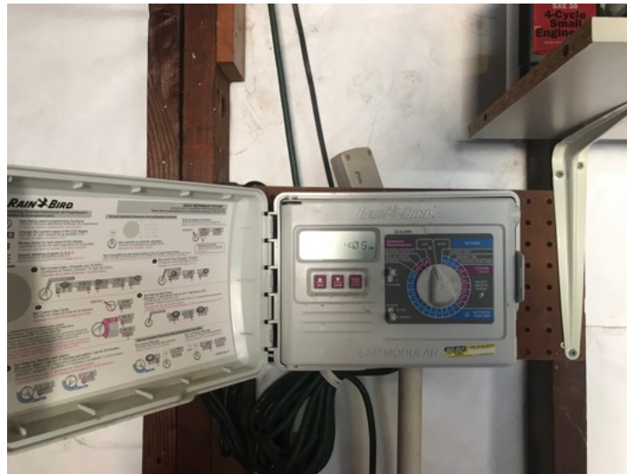
Sprinkler control panel located in garage
