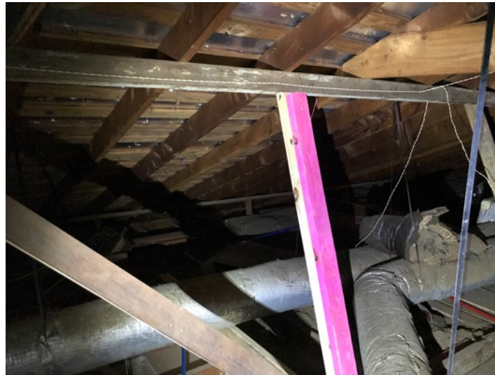
Observed previous repairs to structural members
