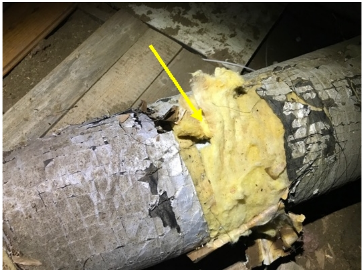
Damaged/missing insulation on air ducts
