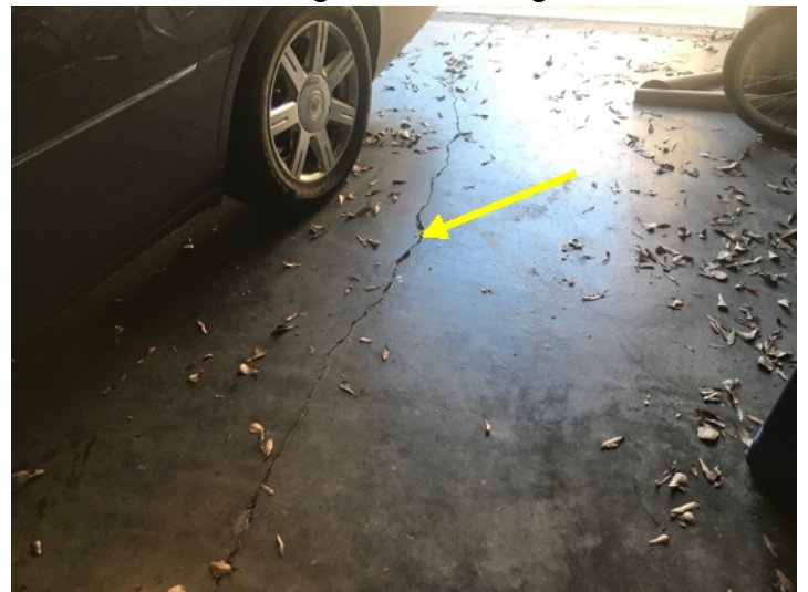
Cracks in the garage floor
