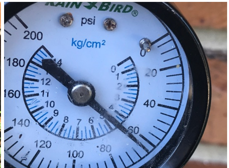
Static water pressure: 64 psi
