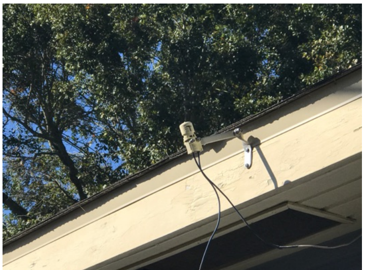
Sprinkler's rain sensor
