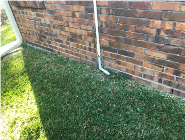
High soil at slab
