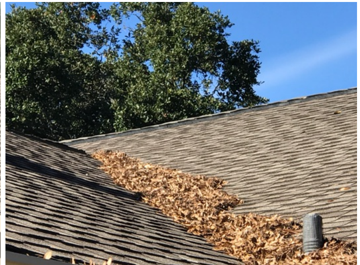
Debris on the roof
