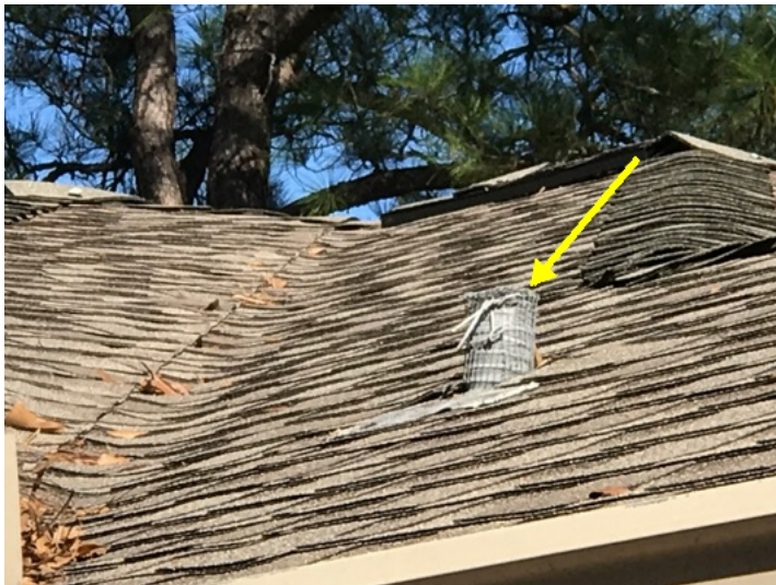
Inadequate height for vent stack at right rear corner of roof
