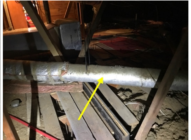
View of air ducts
