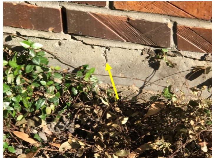
Cracks in grade beam right side
