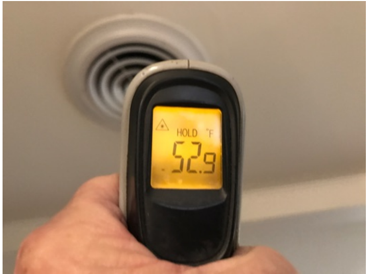
A/C air temperature at supply air register
