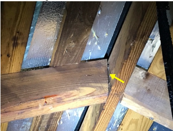
Rafters not adequately secured to ridge board
