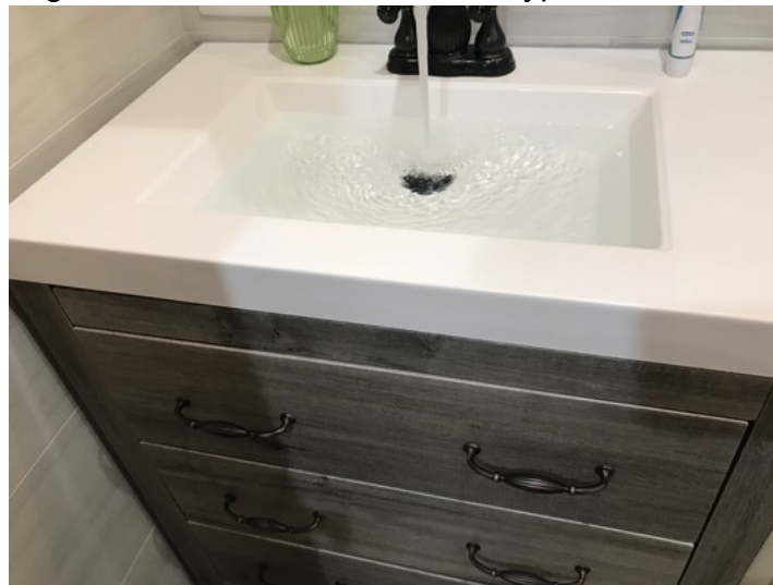
Typical view of testing drains at sinks
