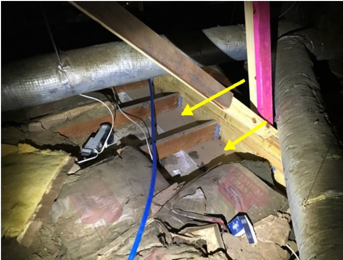
Missing insulation in attic
