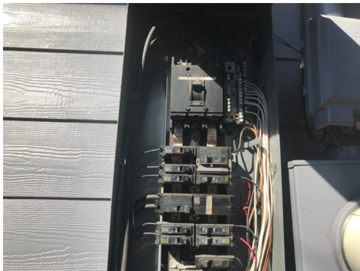
Main service panel at rear of garage
