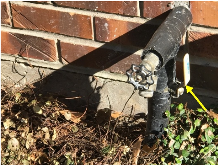
Main water cut-off valve
