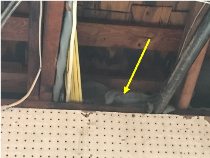
Inadequate firewall for conductors at the breezeway
