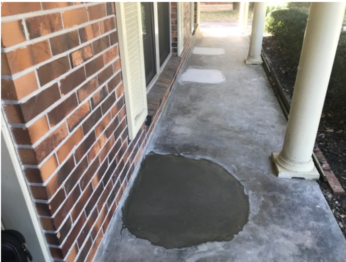
Signs of previous foundation work on house
