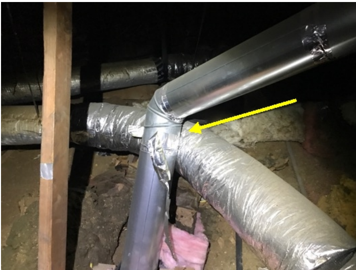
Air ducts in contact with vent pipe
