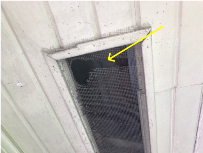
Damaged soffit vent at rear of house
