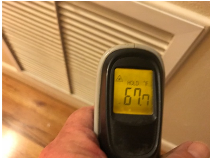
A/C air temperature at return air register
