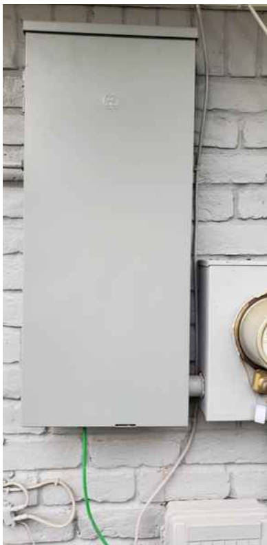
Meter Location: Left Side
