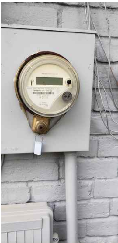
Main Distribution Panel: Breakers Electric Panel Manufacturer: GE Ground Connector: Ground Rod Service Entrance Wires: Copper Service Ground: Copper
