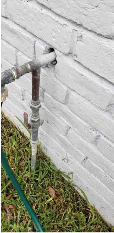
Location of Water Meter: At Street, Front yard Left
