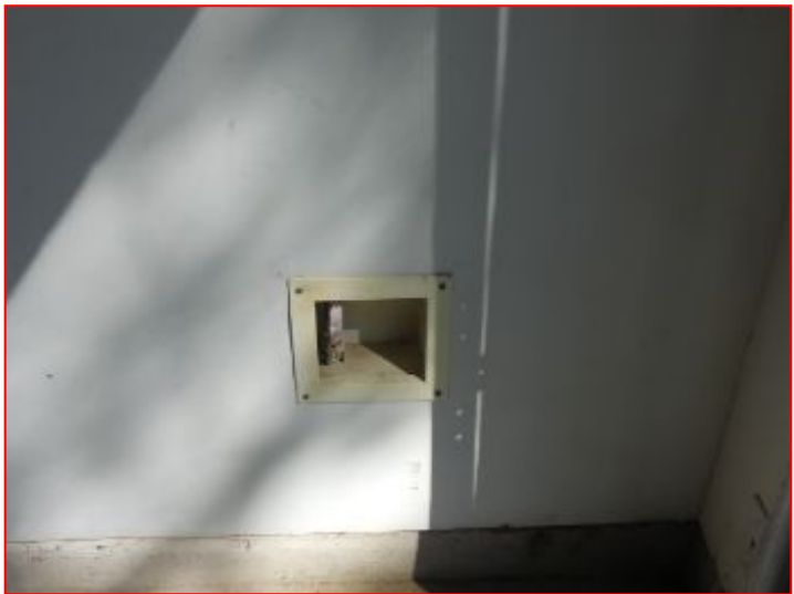
MAin shut off valve
