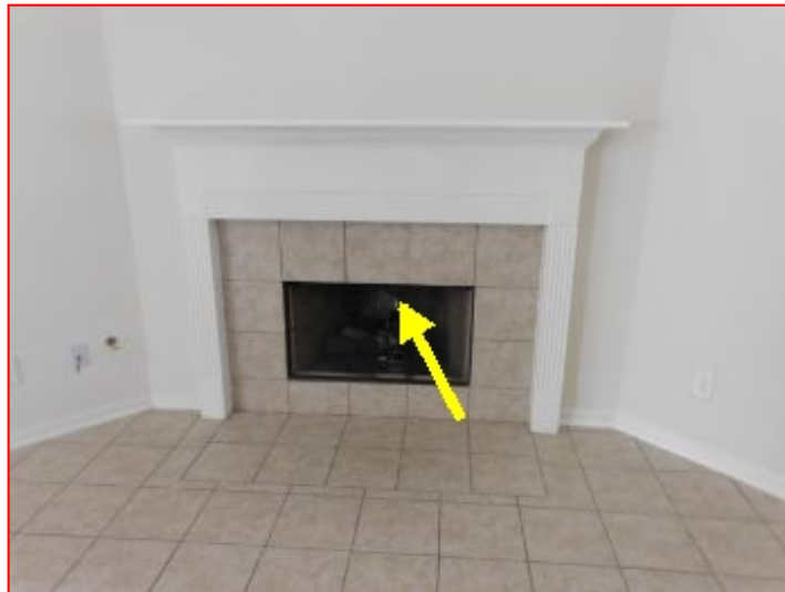
This fireplace is not equipped with a damper stop.
