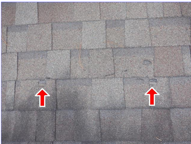
C. Damaged shingles, back of home
