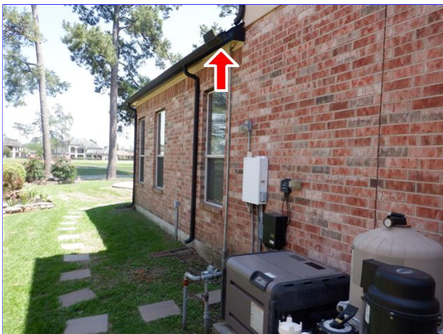
B. Back left side of home, loose gutter
