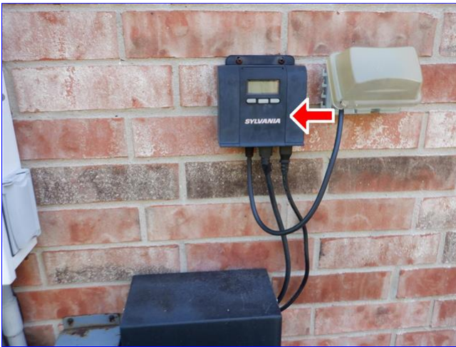
B. Exterior yard lights controller
