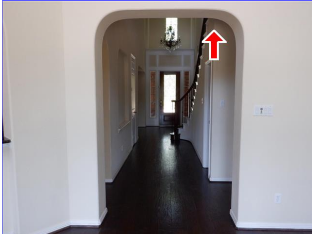
B. Downstairs hallway, missing smoke detector
