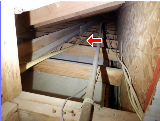
E. Upstairs back attic, CSST gas supply line
