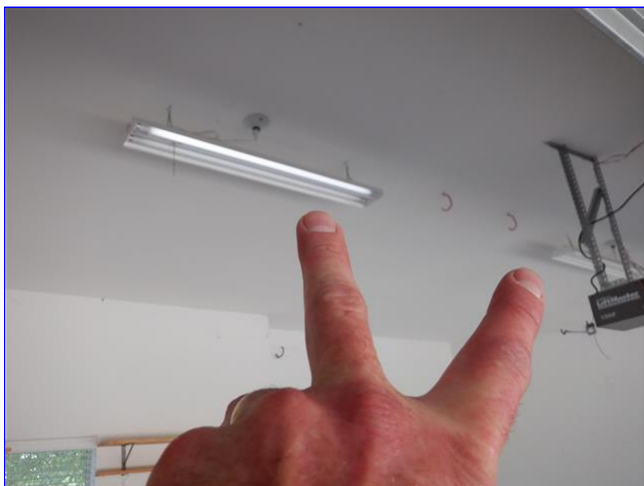
B. Front garage lights
