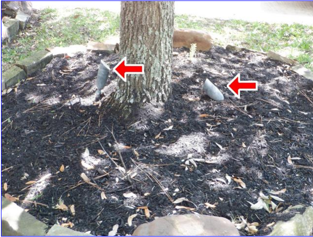
B. Exterior yard lights
