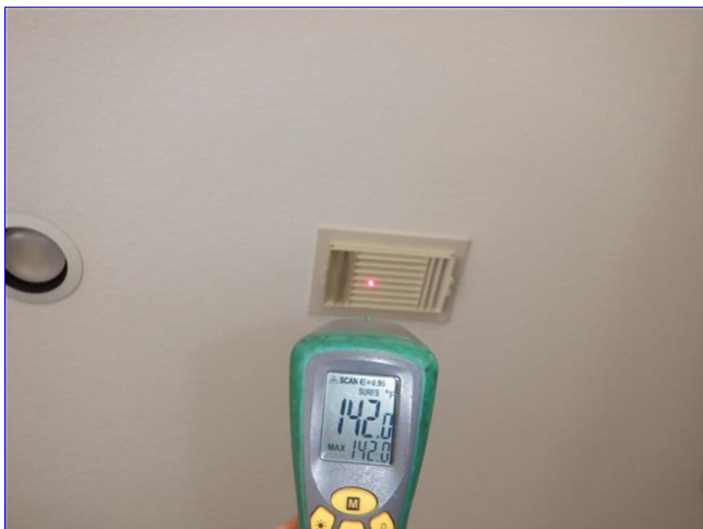
A. Downstairs furnace temperature reading
