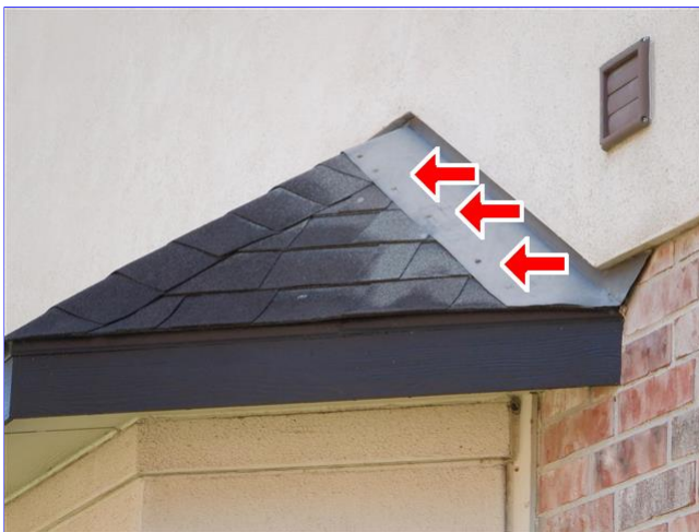
C. Exposed nail heads on flashing, left side of home
