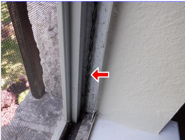
H. Upstairs front left bedroom window, broken hardware
