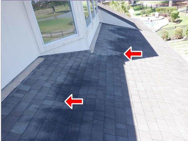
C. Damaged shingles, back of home
