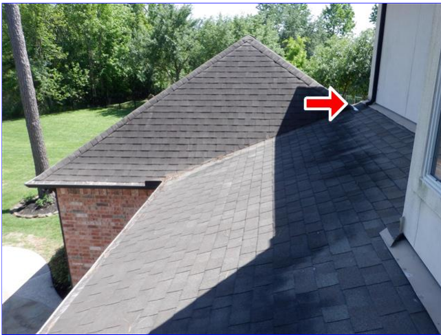
C. Exposed nail heads on flashing, back of home
