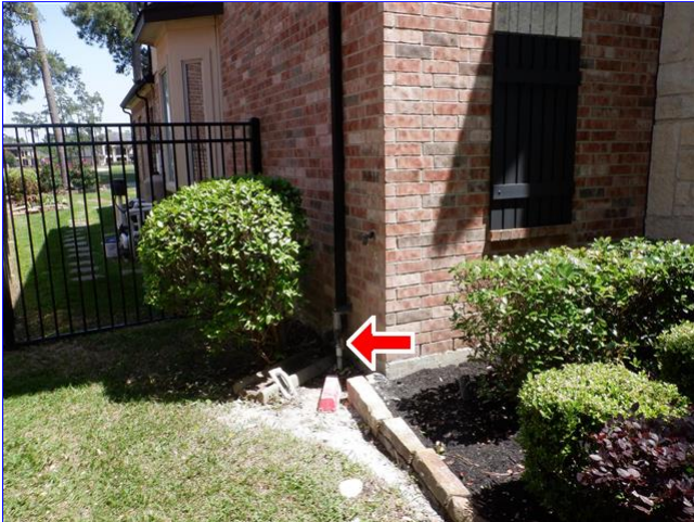
A. Front left corner of home, main water supply line, insulation needed
