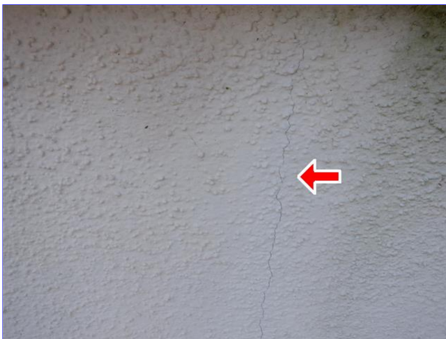
E. Back of home, cracks on exterior siding
