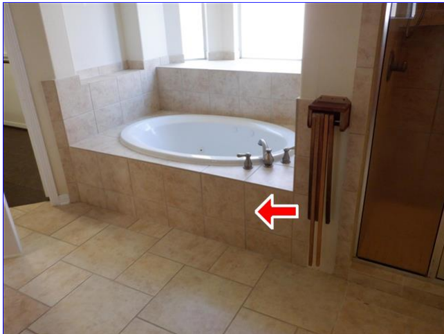
A. Master bathroom hydro-massage tub, no mechanical access panel
