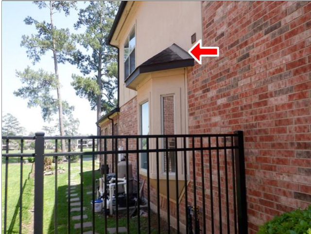
C. Exposed nail heads on flashing, left side of home
