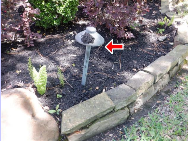
B. Exterior yard lights
