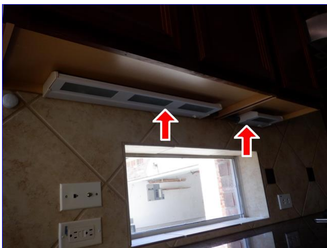
B. Kitchen cabinet lights
