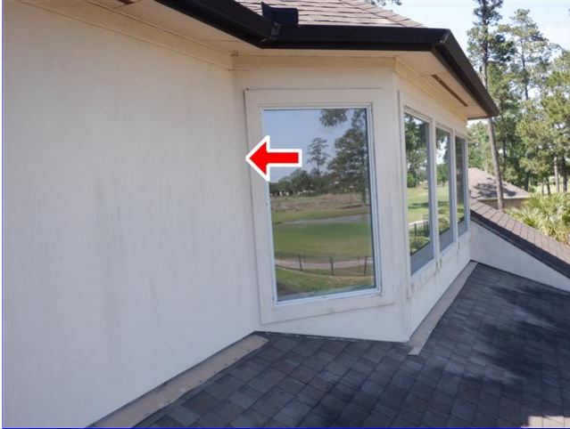
E. Back of home, cracks on exterior siding
