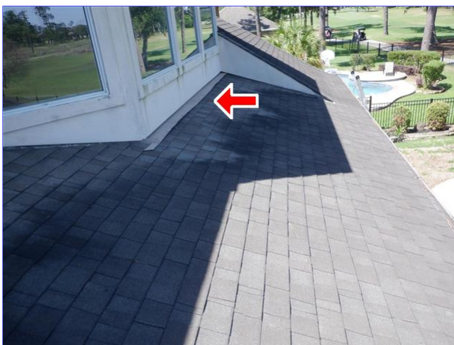
C. Loose flashing, back of home
