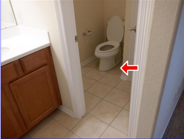
A. Jack and Jill bathroom toilet, loose to floor
