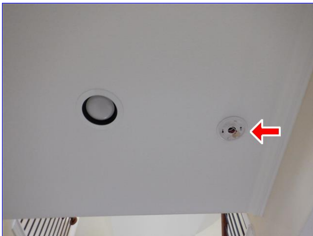
B. Downstairs hallway, missing smoke detector
