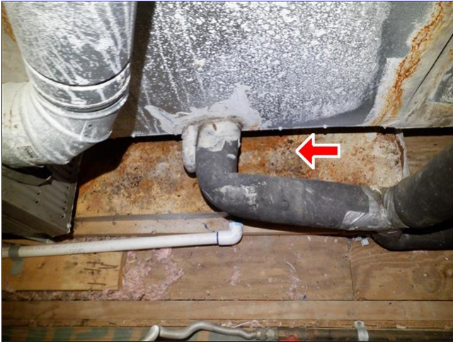
B. Downstairs AC auxiliary drain pan
