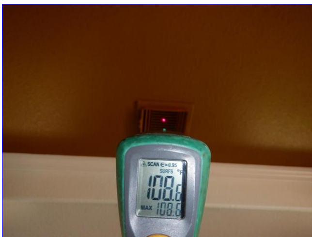
A. Master bedroom furnace temperature reading
