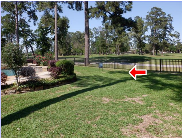
A. Zone 6, broken sprinkler head
