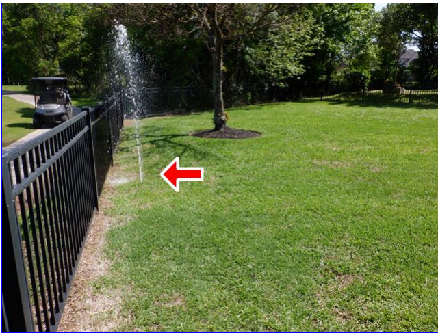
A. Zone 7, broken sprinkler head
