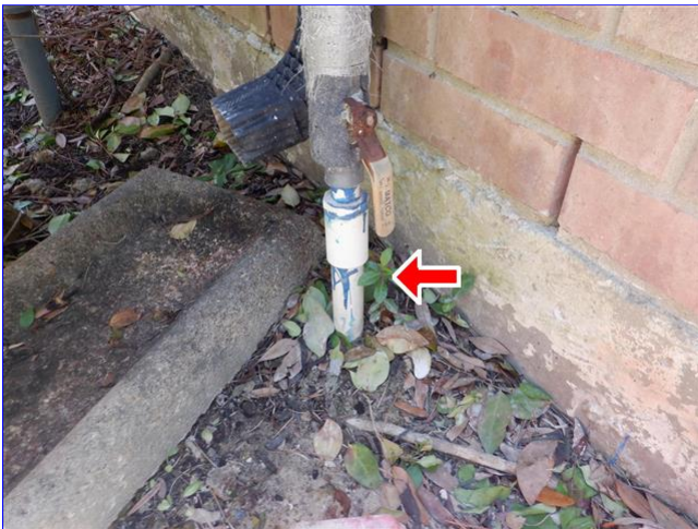
A. Front left corner of home, main water supply line, insulation needed
