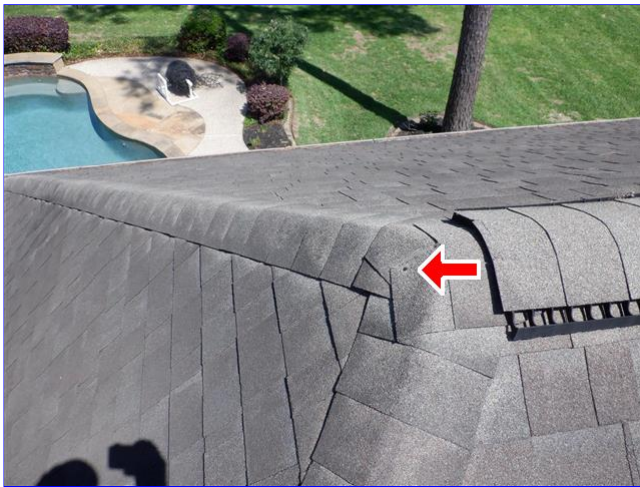
C. Exposed nail head, cap shingle
