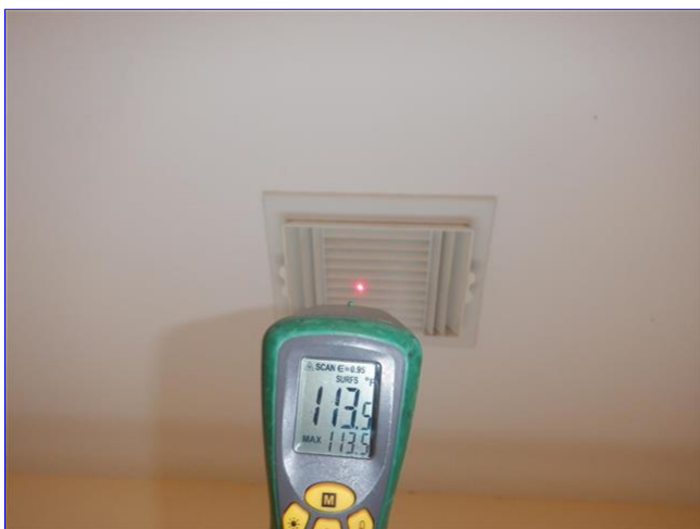
A. Upstairs furnace temperature reading
