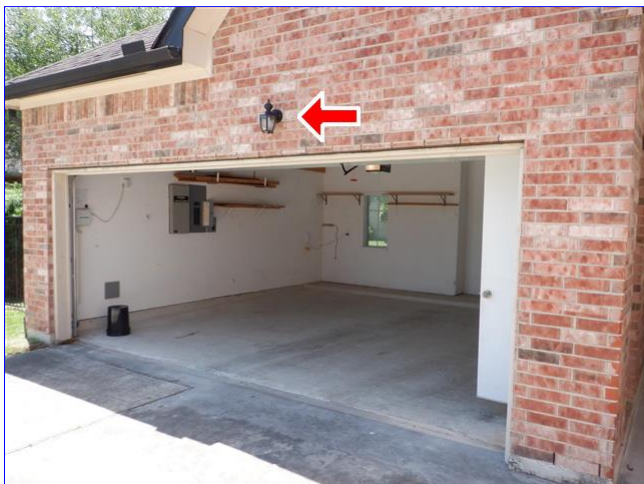
B. Driveway light not working
