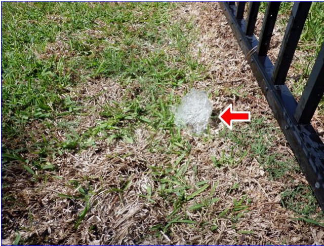
A. Zone 6, broken sprinkler head
