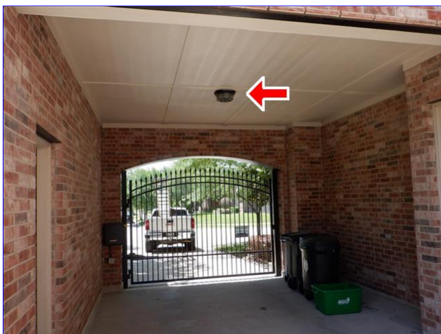
B. Driveway light not working
