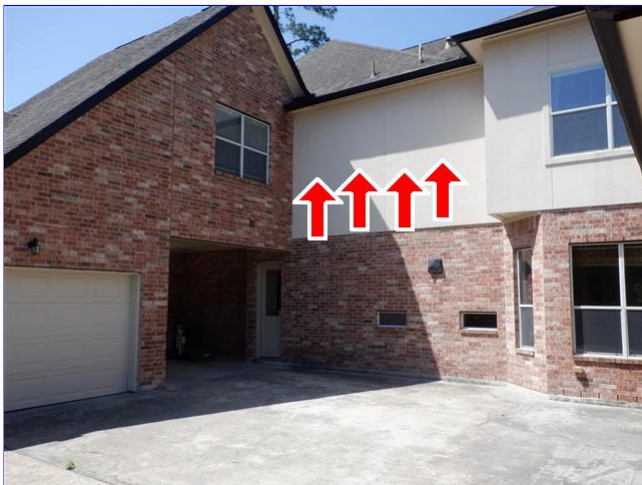
E. Cracks on exterior wall, near driveway
