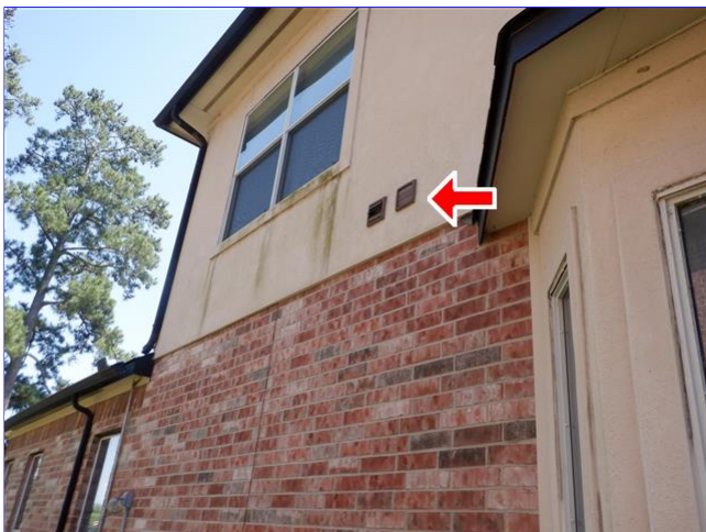
F. 1/2 bathroom exhaust vent
