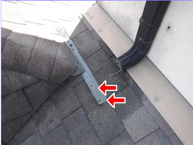
C. Exposed nail heads on flashing, back of home
