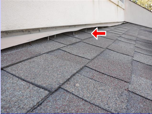
C. Loose flashing, back of home
