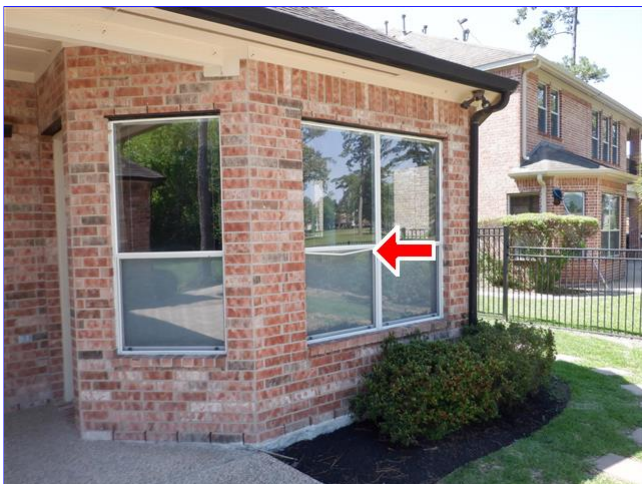
H. Master bedroom window, damaged window screen
