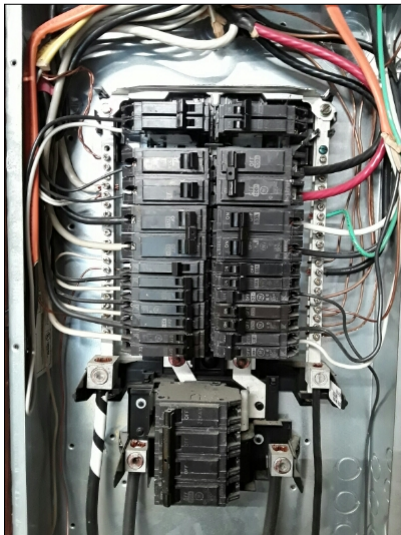
Overview of main electrical panel
