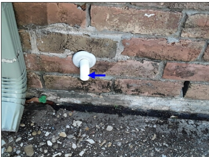
-Recommend painting all exposed plastic pipe to prevent premature deterioration from UV rays.
