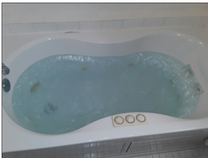
The hydro therapy tub is operating as intended.
