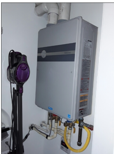
Overview of water heater(s)
