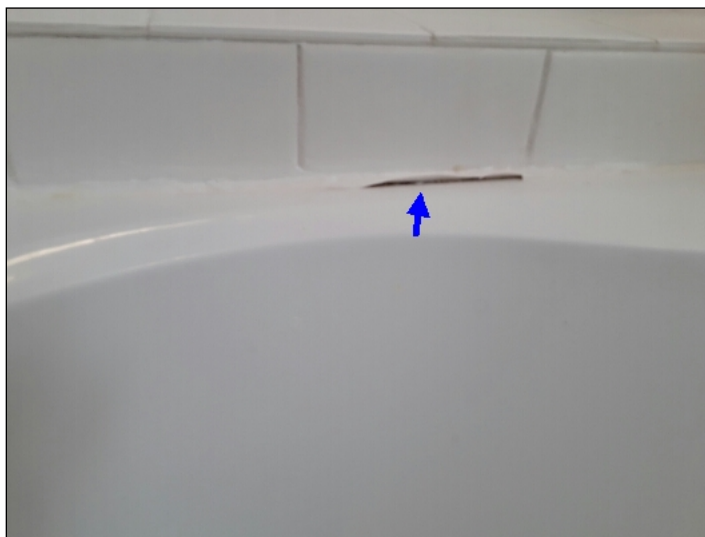
-Recommend re-sealing the tub to help prevent water penetration to underlying materials. Mainly at - upstairs right rear bathroom
