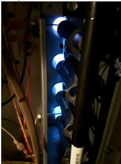
Overview of furnace burner compartment.
