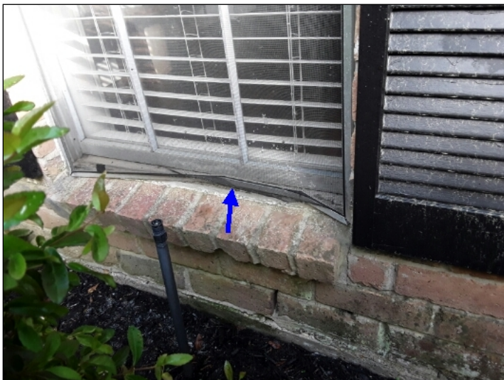
-Window screens are bent or damaged on the home. Mainly at - front right
