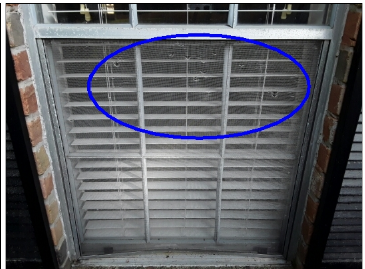
-Window screens were damaged or had holes in them and should be repaired to help prevent insects from entering. Mainly at - front right
