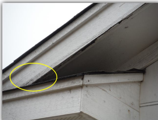
Small spot of fascia rot beginning over left rear lower roof joint to siding.
