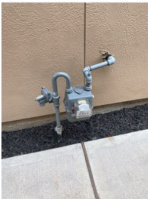
Gas meter located inside gate
