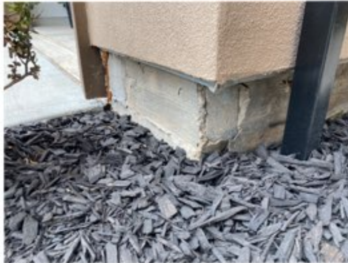
Front right corner of foundation has a galvanized metal plate. (Appears to be hurricane strapping - Recommend further evaluation)
