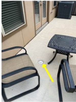
Main drain clean out located at rear of structure
