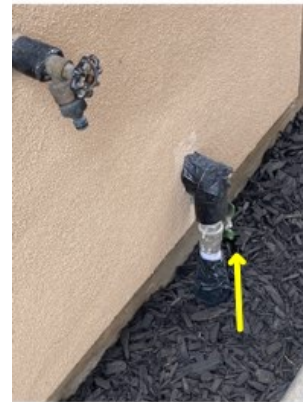
Main water shutoff located inside gate on side of garage
