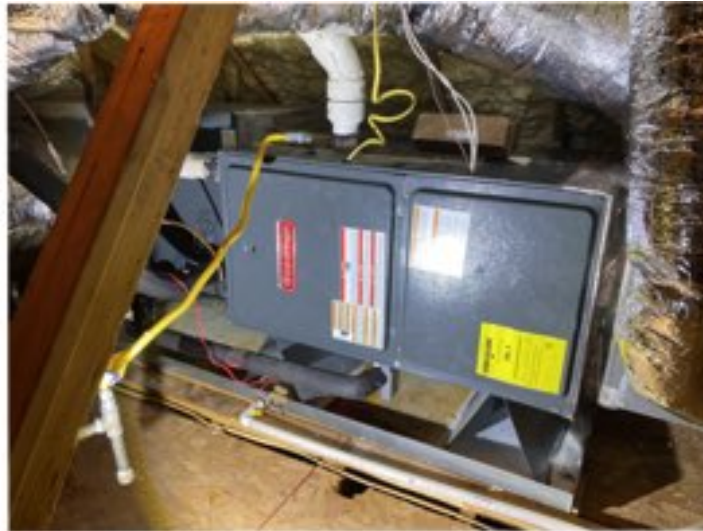
90 Percent Furnace Located in attic
