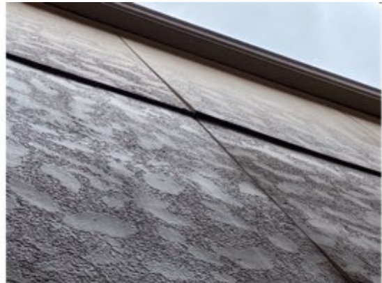
Siding appears to be loos or bowing out. (This may not be a real problem and could be the Z flashing creating an uneven look.)
