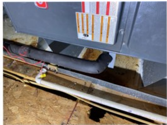
Rust in drip pan
