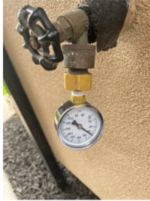
Static water pressure is 60 psi
