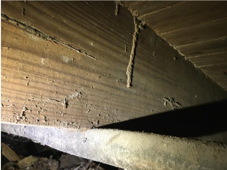
Previous Subterranean termites.
