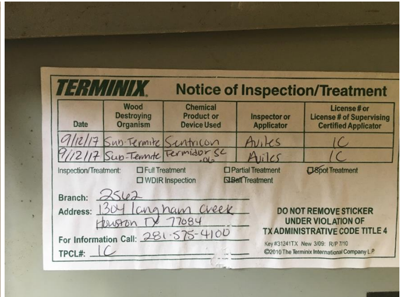
Evidence of Subterranean termites treatment
