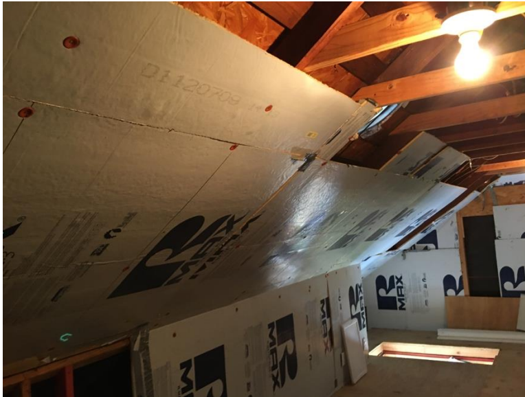
Obstructed view in attic
