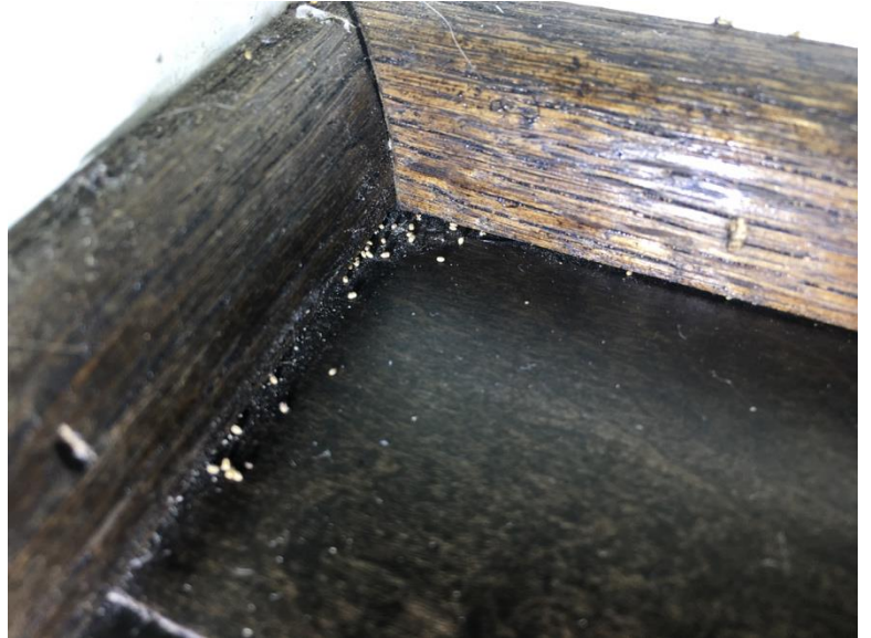
Evidence of Drywood termites observed in Closet.
