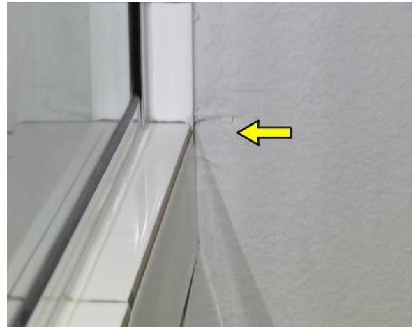
Drywall damage noted - master shower area.
