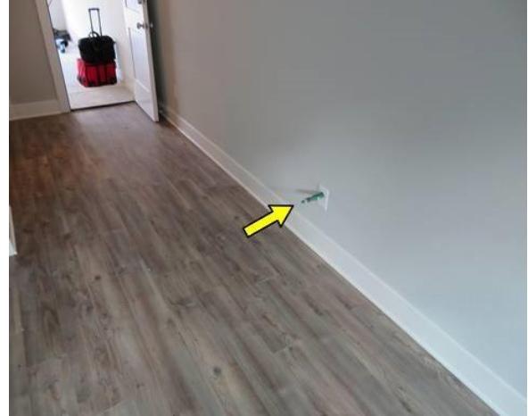
Loose outlet box - family room.
