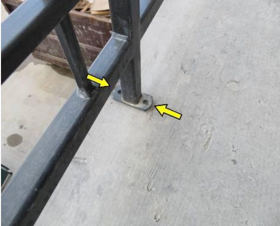
Missing securing screws - upstairs balcony.
