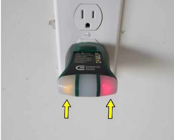
Hot and neutral reversed - garage wall.
