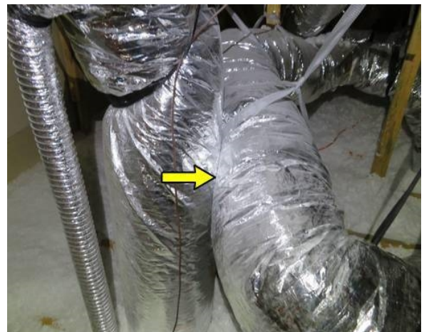
Example ducts in contact - attic.
