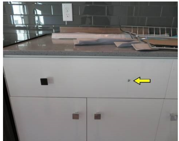
Cabinet pull missing - kitchen draw.
