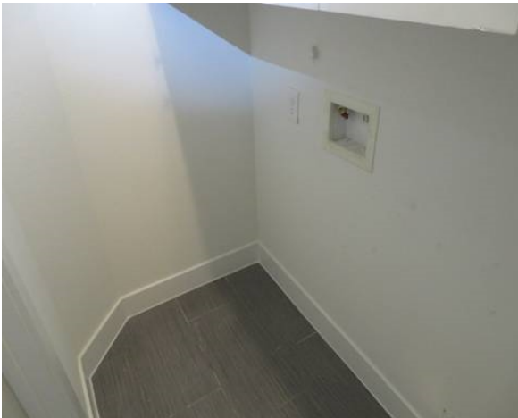
Missing washing machine pan - upstairs utility room.
