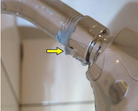
leak noted - upstairs Jack & Jill bath tub.
