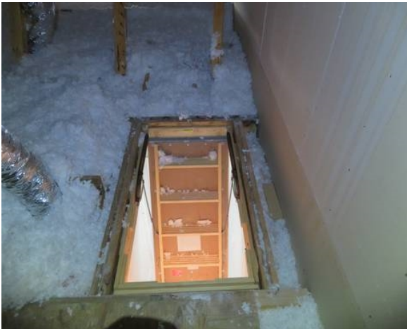
Attic stairs missing the required landing and walkway.
