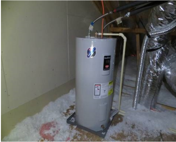
Water heater located in the attic.
