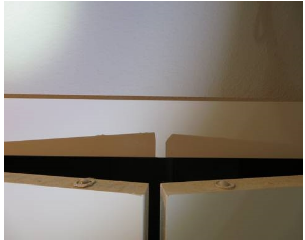
Utility room latching balls will not engage.
