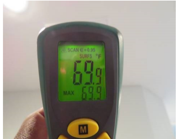
Return air reading is outside supply and return differentials - unit should be serviced.
