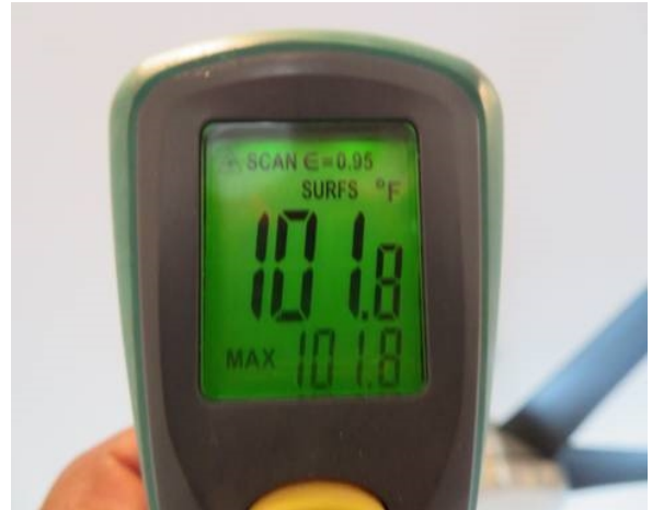
Average temperature reading from heat supply registers - no deficiencies noted.
