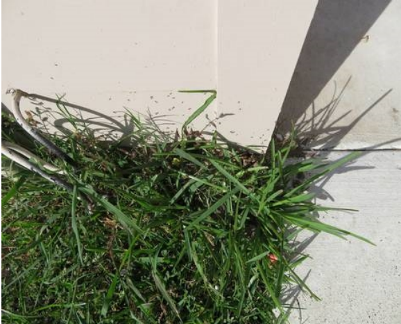
Active ant bed noted - front elevation.
