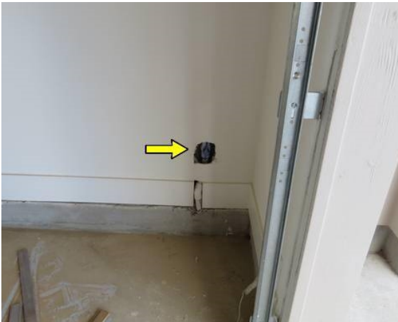
Location of the main water shut-off - Garage wall.
