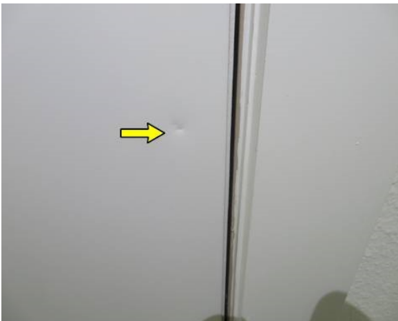
Example dent noted - master bedroom door to the balcony.
