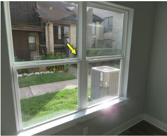
Broken window sash - breakfast area.
