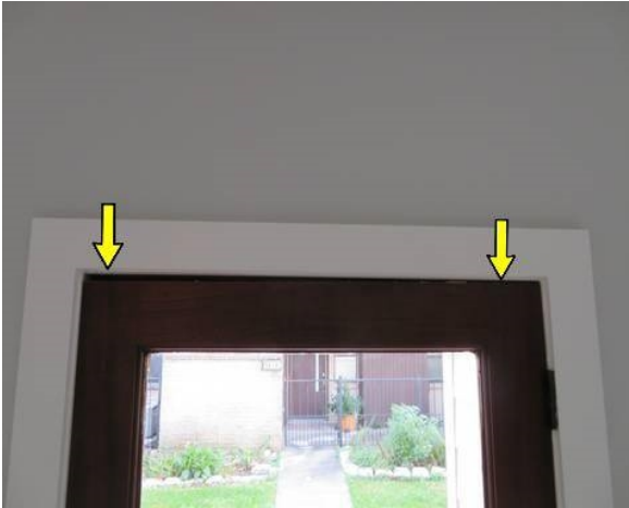
Front door out of level.
