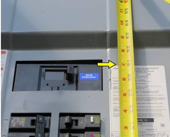
Main electrical shut off switch above 6'7" height - service panel.
