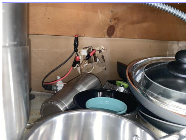
B. Item 1(Picture) Below stove
