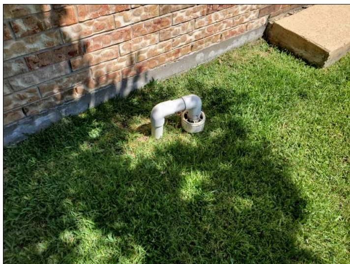
Pool drain needs to have a 1" air gap.
