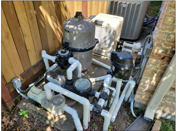
All PVC piping should be painted with UV protectant paint to prevent sun damage and cracking. Along with proper labeling.
