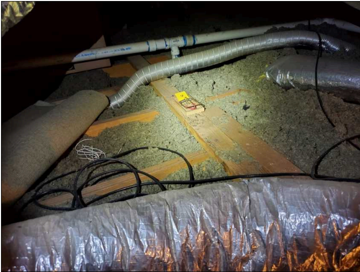
Rat and pest traps noted in attic.
