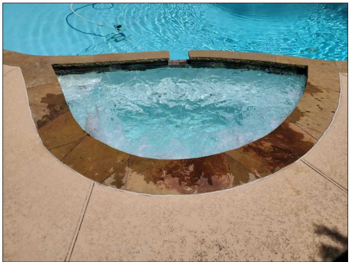
Air blowers operated.
