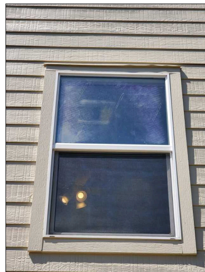
Windows have film that is damaged with age. Sign of leaking gas.
