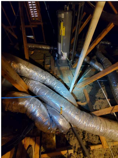
Missing clear stable walk path to equipment in attic.
