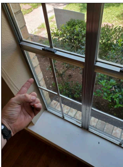
Older aluminum windows are difficult to operate.
