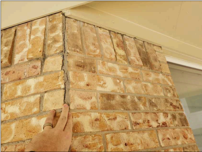
Exterior cracks in brick mortar noted.
