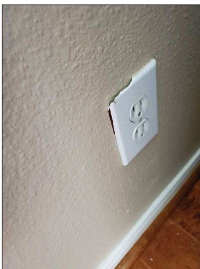
Broken receptacle cover.
