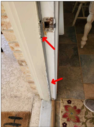
Damaged door seal
