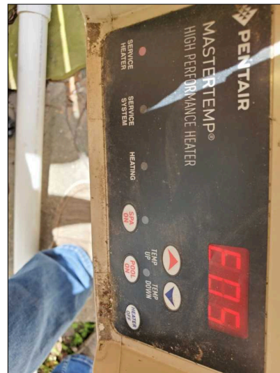
Heater error code E05. Ignition failure. Repairs suggested for operation.
