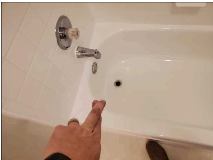
Missing stopper in sink / tub.
