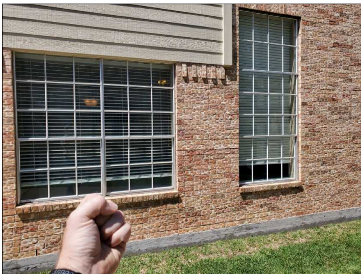
Missing / damaged screens noted.
