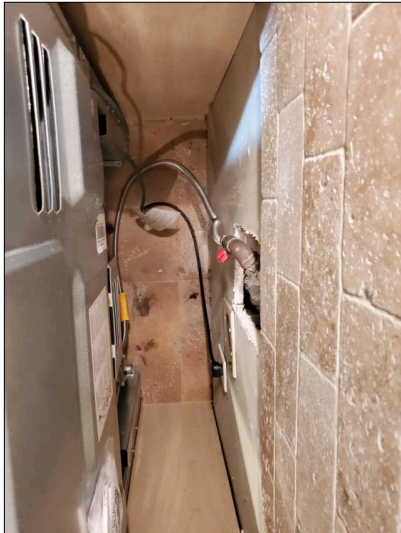
SAFETY CONCERN: Free standing range missing anti-tip bracket/device. Should be installed.
