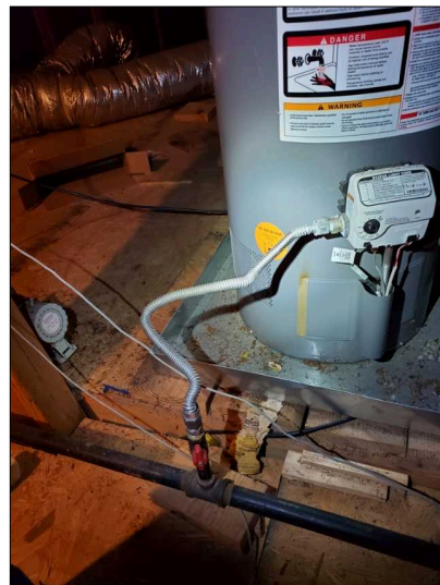
Sediment trap missing / not correct at fuel fired appliance.
