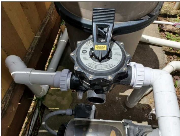
Backwash selector not tested to all functions.
