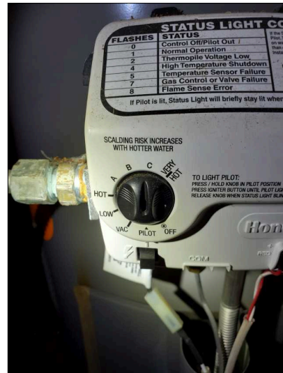
Water heater is set to [B]. This is high, and my scold as well as be less energy efficient as the normal 120F setting.
