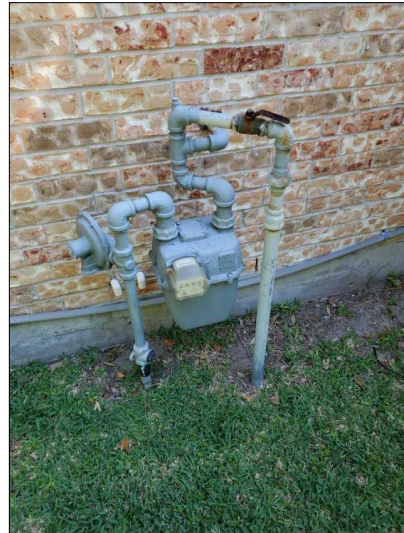
Gas meter and shutoff location.
