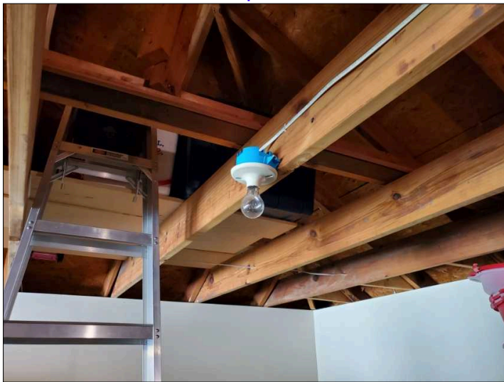
Some lights did not function at time of inspection.
