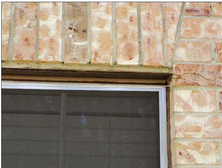
Rusted steel lintel above windows. This supports brick, and should be painted. Cracked brick noted.
