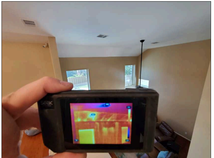
Missing insulation in several places. Noted Via thermal camera.
