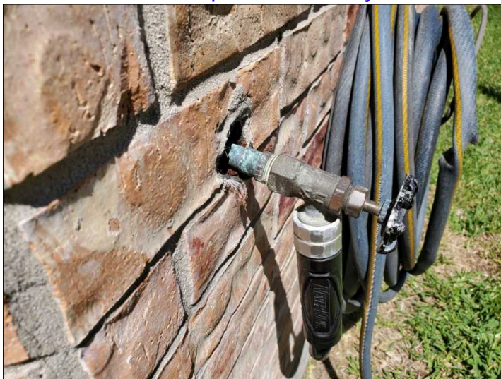
Exterior piping not insulated.
