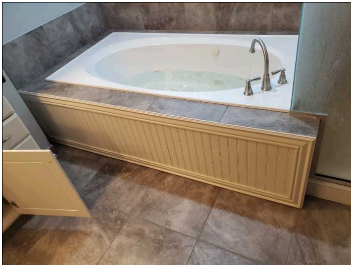
No access panel to pumps or receptacle.
