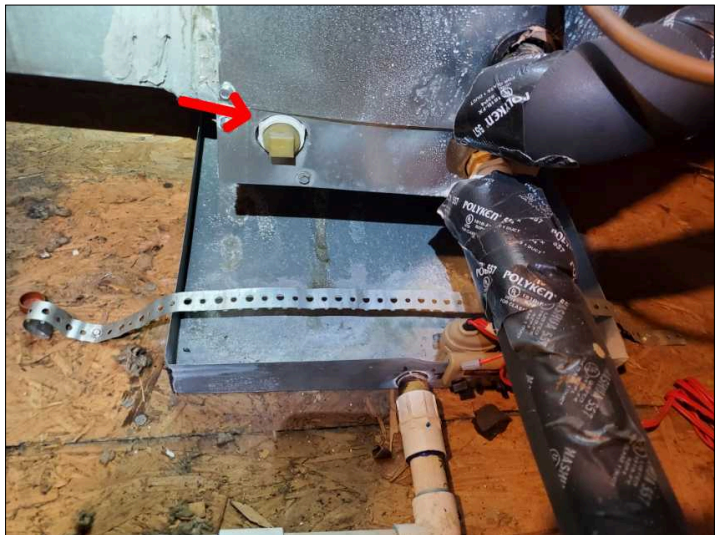
No secondary drain installed. This should drain into a new pan if the primary is clogged.
