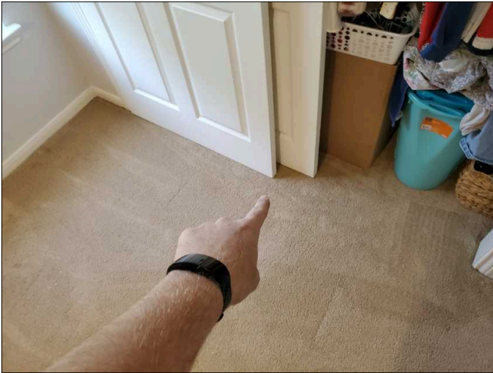
Sliding door missing lower guide. Doors may easily come off track.
