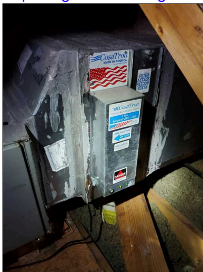
Electronic filters present and appear functional.
