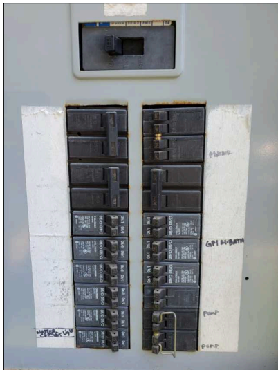
The electrical panel is not properly labeled.
