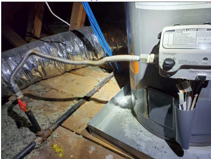
Sediment trap missing / not correct at fuel fired appliance.
