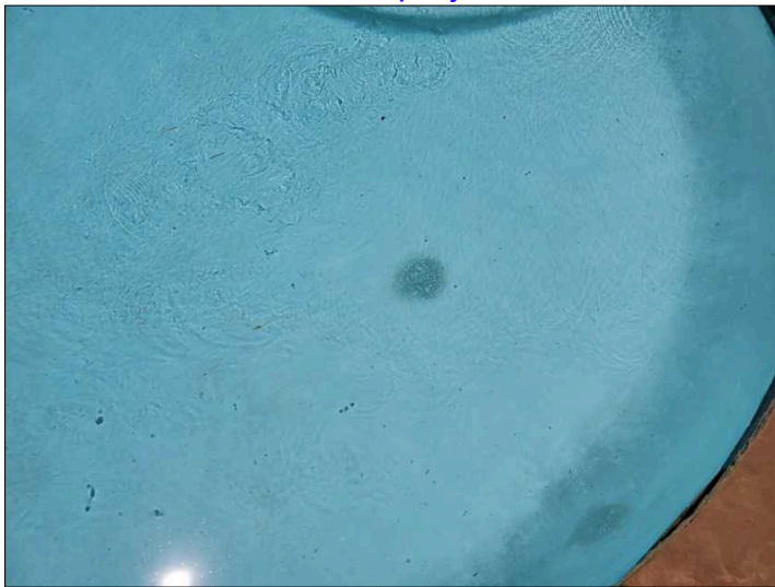
Stains noted in pool surface. Cleaning suggested, no cracks noted.
