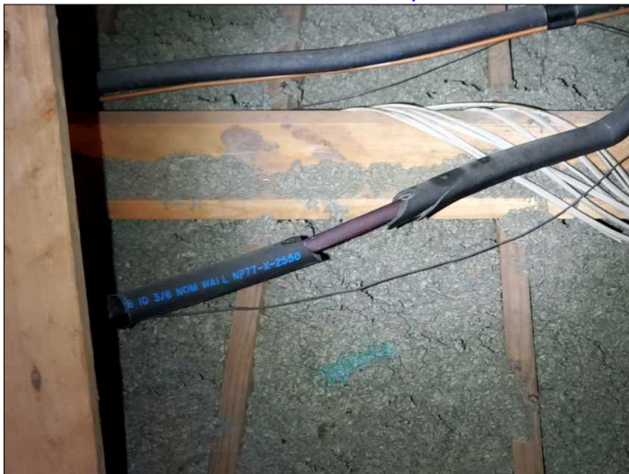
Coolant lines missing insulation in attic space. This will condensate and drip onto attic floor / ceiling.
