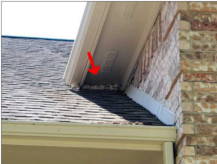
Pest foam noted.
