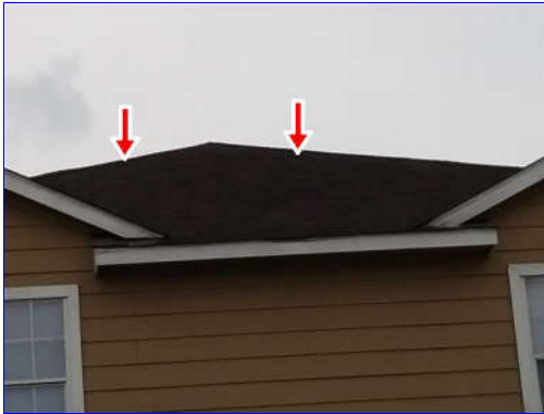
C. Item 6(Picture) Examples of damaged shingles
