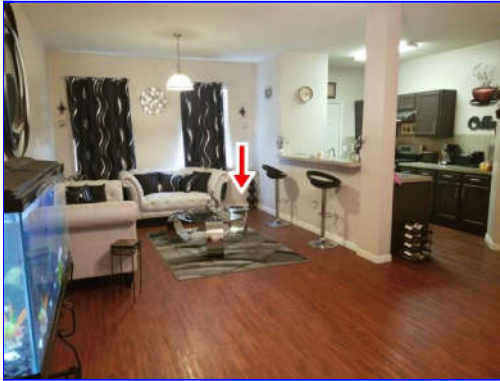
A. Item 1(Picture) Floor is slopes toward the rear right corner of the house
