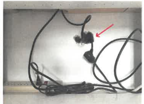
Electrical wiring from the TV is routed through the wall
