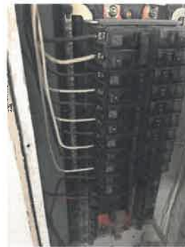
Neutral wiring as hot
