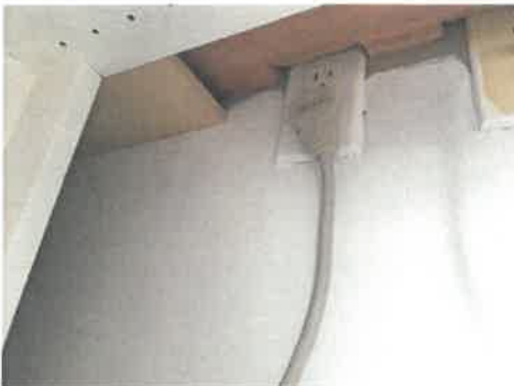
Blocked receptacle behind bench
