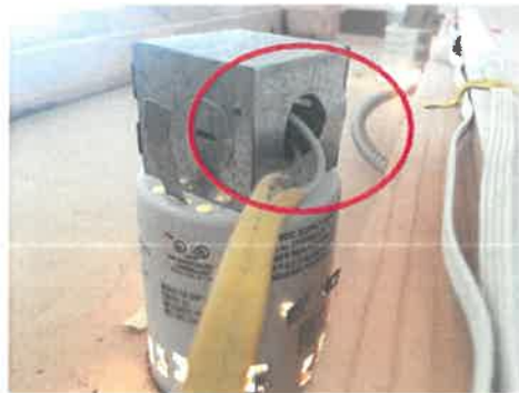
Missing wiring protection
