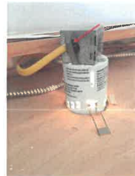
Missing wiring protection
