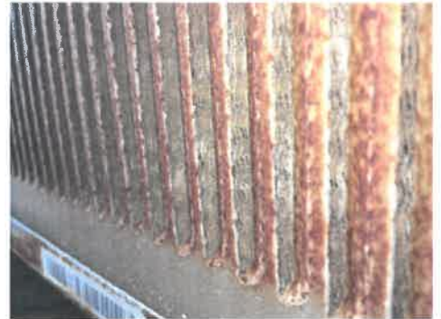
Dirty condensing coils
