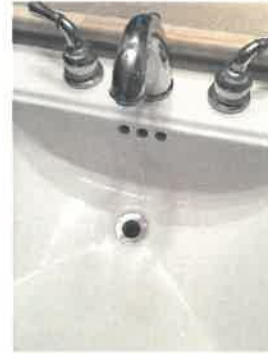
Missing pop up drain stopper
