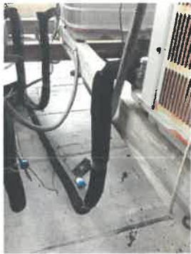
Refrigerant piping hanging with no support
