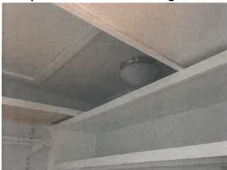
Bedroom closet lights inoperative
