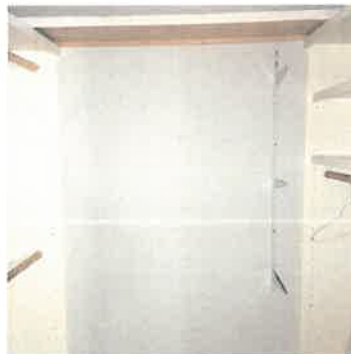
Improperly installed metal shelving unit in closet
