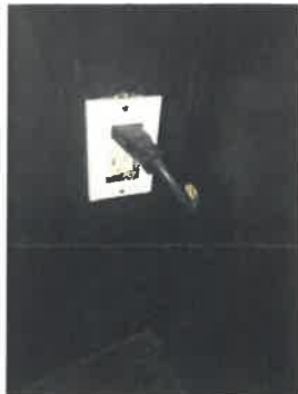
Washing machine power cord is routed through the cabinet
