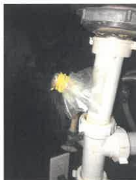
Unprofessional repair at kitchen sink drain
