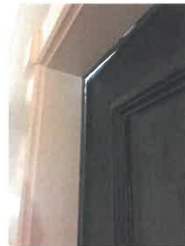
Front door weatherstripping issue
