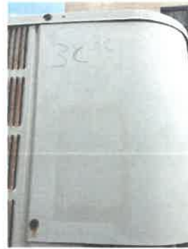
Poor labeling and missing data plate
