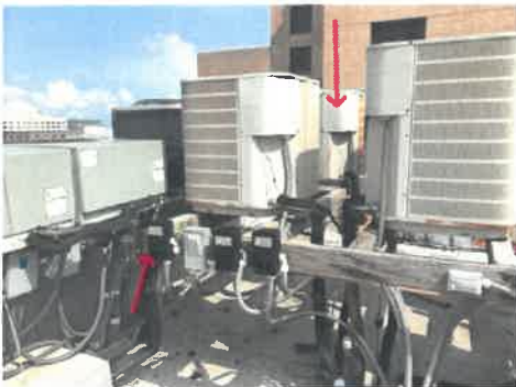
AC disconnect and condensing unit location
