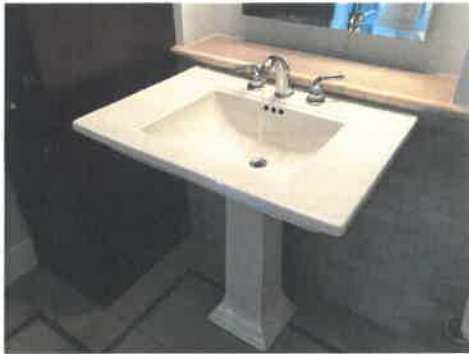
Loose pedestal sink (slightly)
