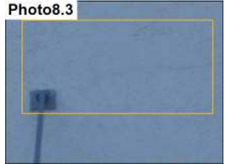
Cracks/ Seal And Paint
