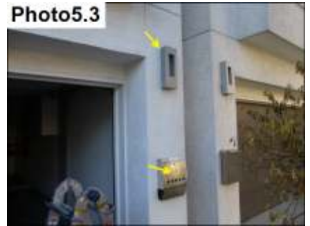
Penetration Sealants/ Seal
