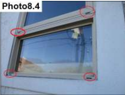
Missing Window Weep Louvered Door/ Install Door
