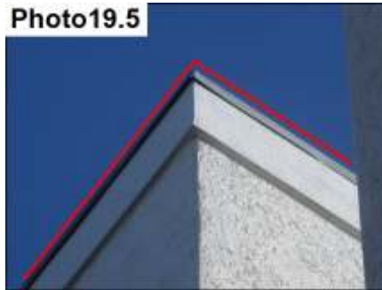
Under-Sized Metal Cap And Parapet Cap/ Replace Cap
