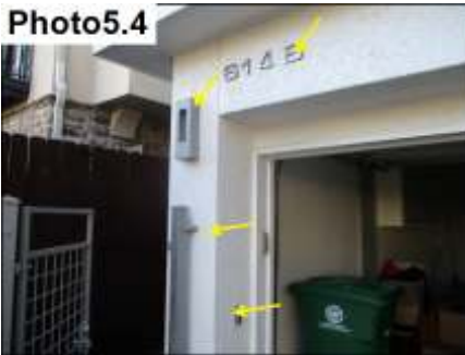
Penetration Sealants/ Seal
