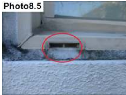
Missing Window Weep Louvered Door/ Install Door
