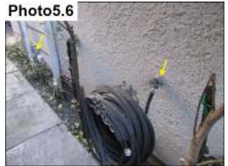
Penetration Sealants/ Seal
