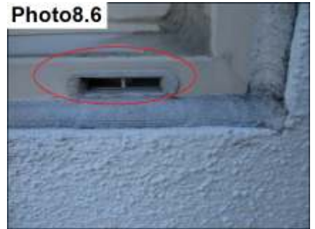
Missing Window Weep Louvered Door/ Install Door
