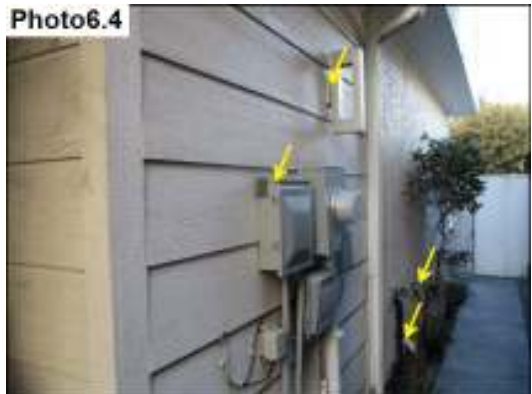
Penetration Sealants/ Seal
