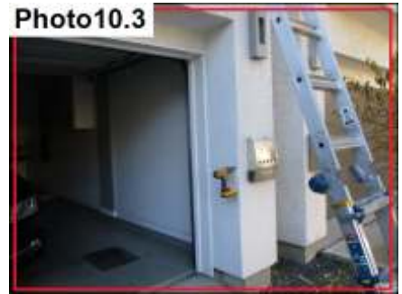
Confirmed Substrate Damage/ Repair And Add Relief
