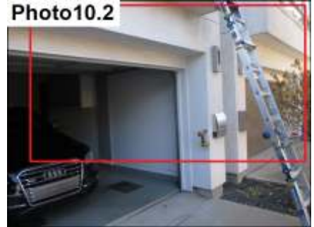
Confirmed Substrate Damage/ Repair And Add Relief
