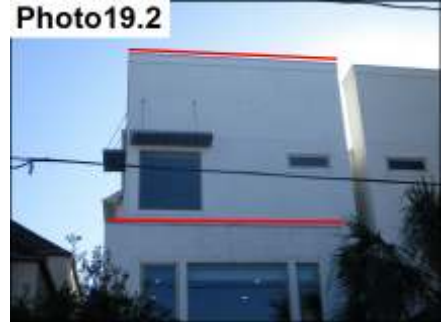
Under-Sized Metal Cap And Parapet Cap/ Replace Cap
