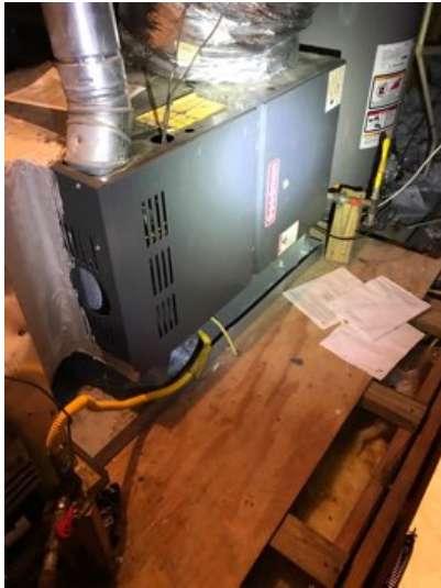
Heating, Ventilation and Air Conditioning Systems Heating Equipment
