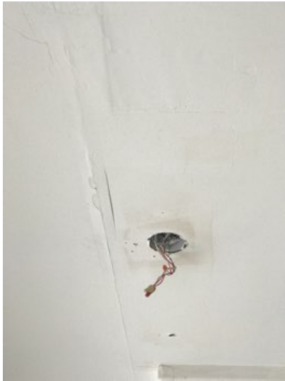
The garage ceiling has sustained damage and has repairs.
