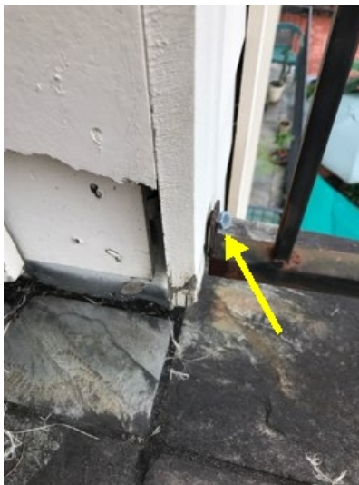
Damaged siding was noted at the upper level balcony.
