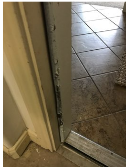
The garage pedestrian door has a damaged weather strip.
