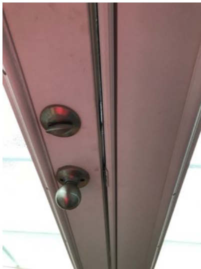
Balcony door weatherstrip do not seal properly and need adjustment or replacement.
