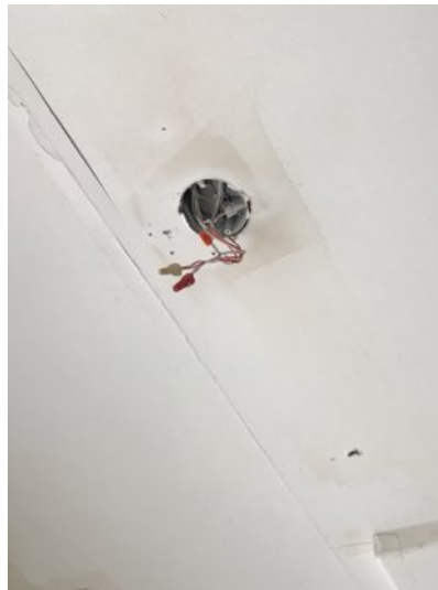
Exposed wiring was noted in the garage ceiling.
