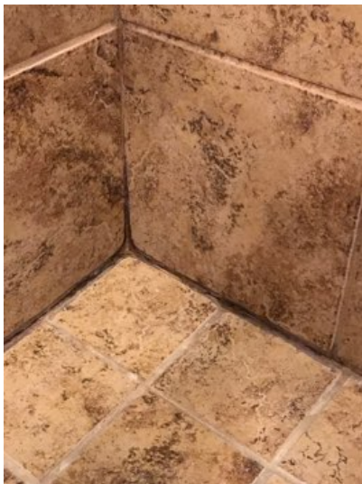
Caulking joints in the master shower should be improved.
