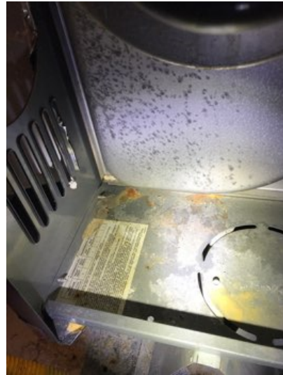
Furnace contained minor rust and is likely from rain water leaking through the furnace flue.
