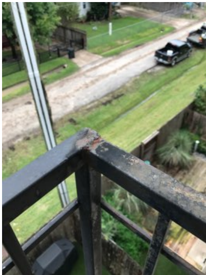
Balcony hand rails were showing signs of rust were noted and indicate rails should be refinished to arrest oxidation.
