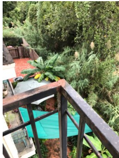
Balcony hand rails were showing signs of rust were noted and indicate rails should be refinished to arrest oxidation.
