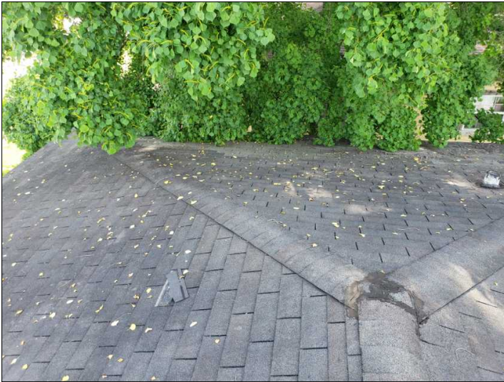
-Tree limbs should be kept trimmed at least 5' from roof to help prevent damage to the roof during windy conditions.
