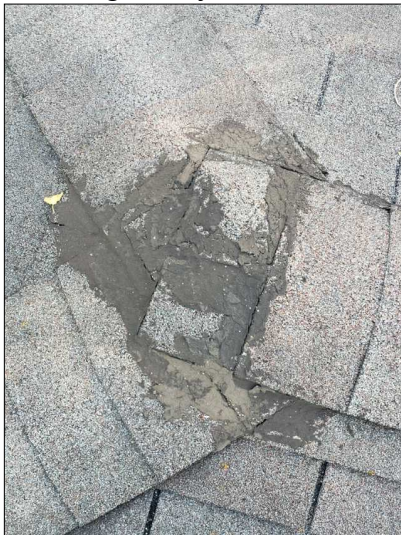
-Signs of improper previous repairs were noted on the roof. Recommend a roofing professional verify the integrity of the repair.
