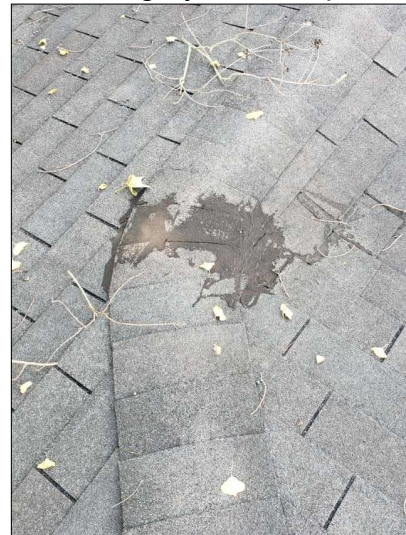
-Signs of improper previous repairs were noted on the roof. Recommend a roofing professional verify the integrity of the repair.
