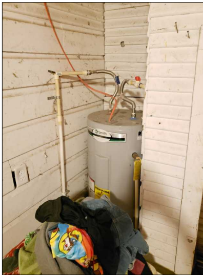
Overview of water heater(s)
