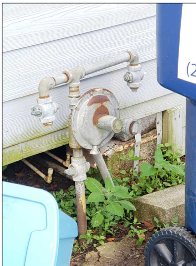
Gas meter is installed however it is not plumbed to the house.
