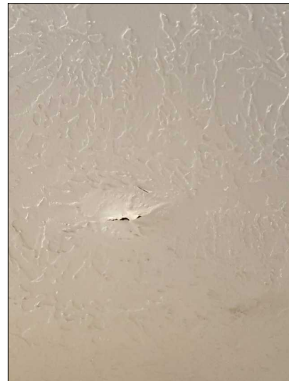
Damaged ceiling. Mainly at- kitchen
