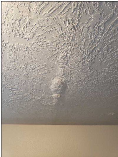
Damaged ceiling. Mainly at- kitchen
