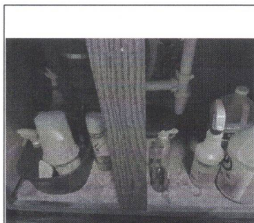
Kitchen vanity has been repaired likely from a leak
