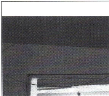
Possibly lead based paint in older doors and window frames
