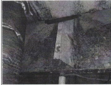
Pan needs replaced
