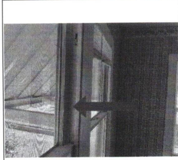
Missing rope and counterweight
