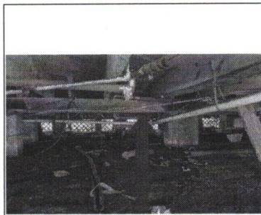
There is a visible slope in the beam near the middle of the home however there did not appear to be a foundation concern
