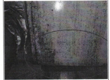
Interior is very old and heavily rusted
