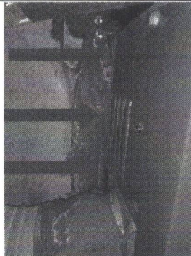
Leaking lots of air near furnace
