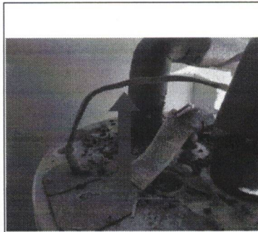
Wiring needs to be in conduit and there needs to be a safety disconnect to kill the power
