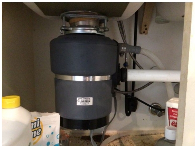
General Photos of Range Hood/Exhaust Systems:
