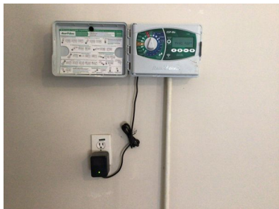
Rain sensor: Installed
