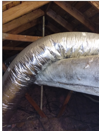
-The ducts do not have the proper separation. It is recommended that an air gap or insulation be used to separate ducts that are in contact with each other to help prevent condensation.
