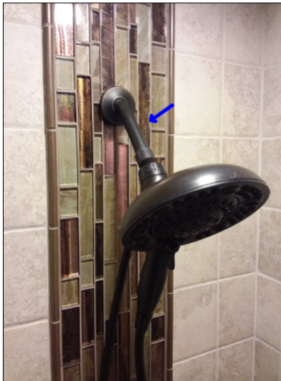
-The shower head loose. Mainly at -master bath
