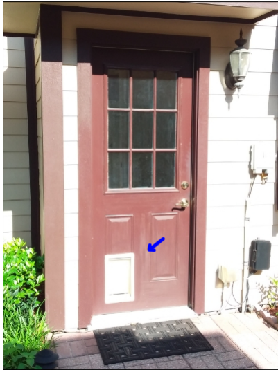
-Doggie door is a security hazard If it can't be locked.
