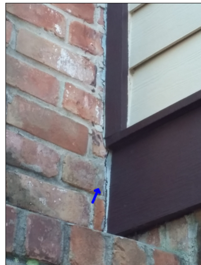
-Recommend sealing between the trim and brickwork to help prevent water penetration. Mainly at -right
