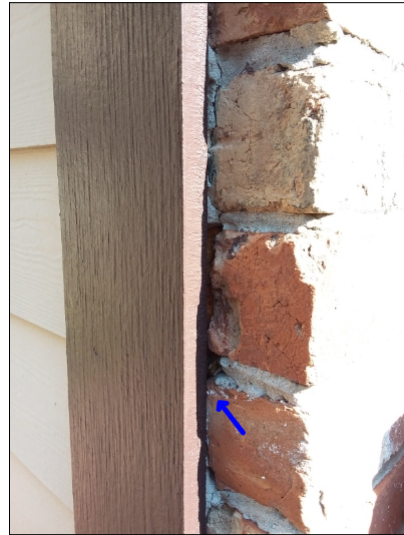
-Recommend sealing between the trim and brickwork to help prevent water penetration. Mainly at -rear/left
