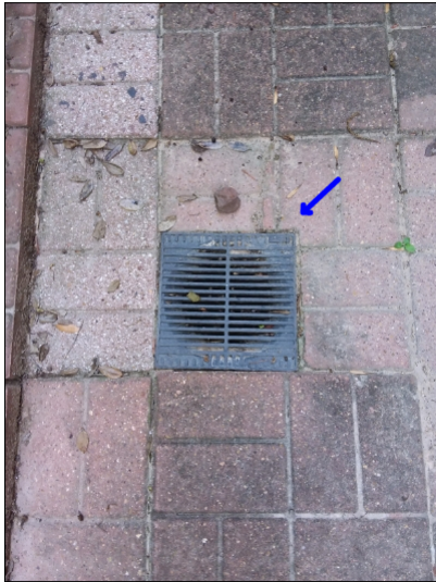
-Surface drains have been noted on the property. We can not determine the condition of drains that are below grade level. Mainly at -right
