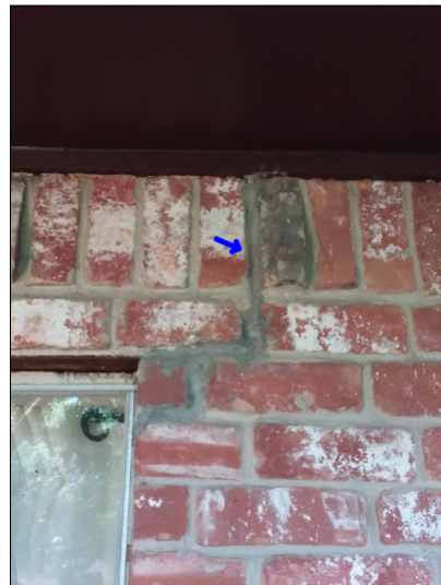
-There are signs of previous repairs in the brickwork. Mainly at -front
