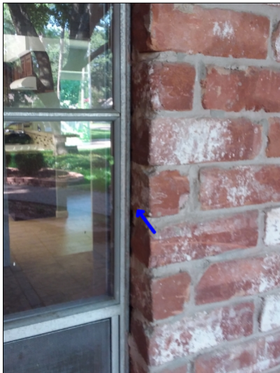
-Sealant is needed around various windows between the window framing and exterior brickwork to help prevent water penetration, recommend checking all windows for proper sealant.
