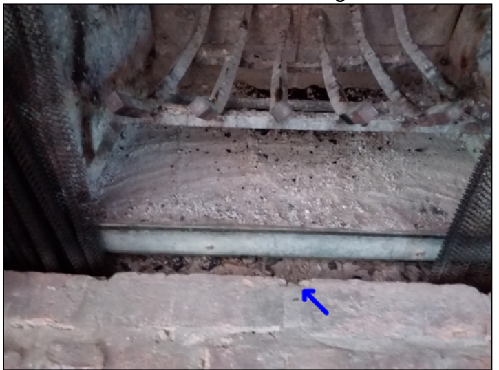
-There is a gap between the fireplace and the firebox. Recommend sealing the gap for safety.
