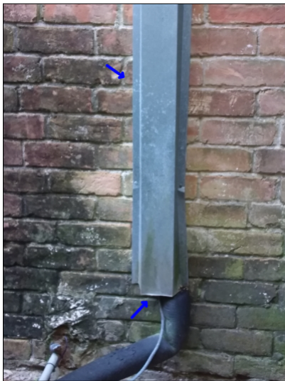
-Seal A/C line entry cover at wall connection to help prevent water penetration.
