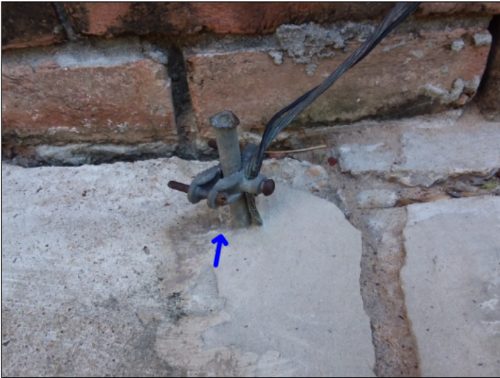
-The ground connection is loose at the ground rod, this could be hazardous, it is recommended that ground wires be secured with the proper acorn style clamp for proper protection.
