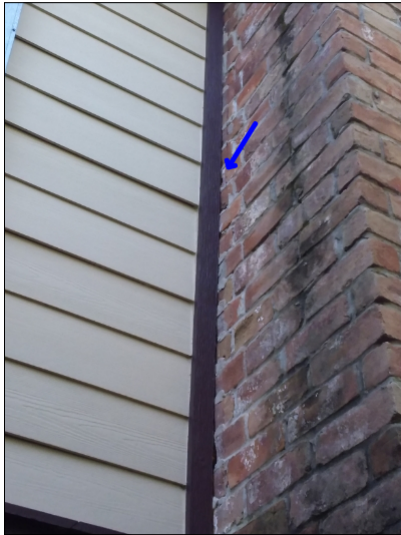
-Recommend sealing between the trim and brickwork to help prevent water penetration. Mainly at -chimney
