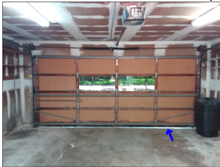
-Garage door is deteriorating.
