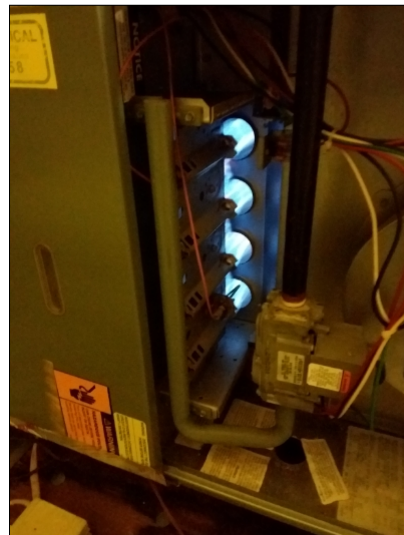
Overview of furnace burner compartment.
