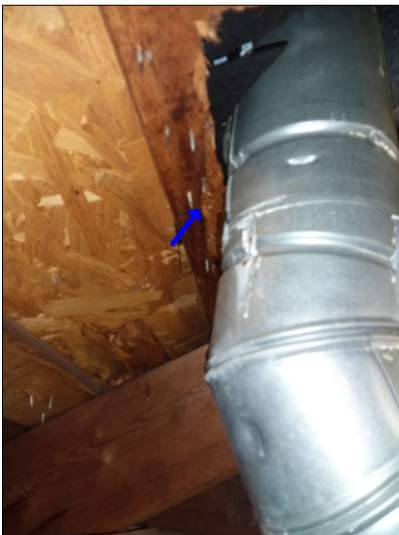
-There is improper clearance around the flue pipe, the furnace vent should have at least 1" clearance to combustibles.
