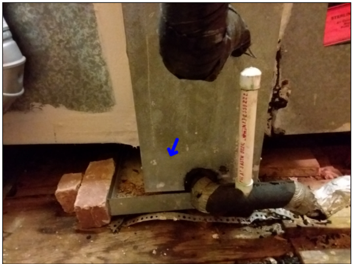
-The evaporator unit was not manufactured with a secondary drain to release condensation to pan or exterior incase the primary drain line is clogged, recommend adding a high water shutoff to primary condensation line if not present for additional protection.
