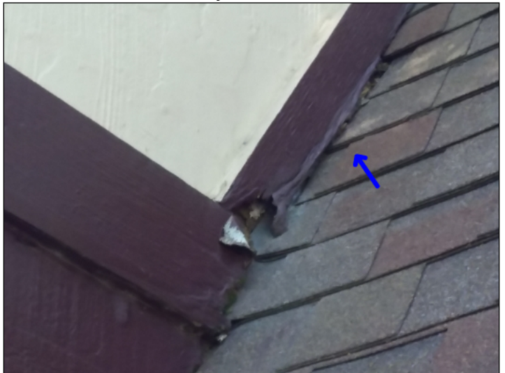
-Deterioration was noted at the trim, recommend replacing all deteriorated trim. Unable to determine the condition of the underlying materials. Mainly at -front
