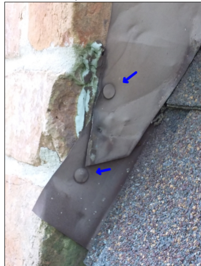
-All exposed nails and fasteners on roof should be sealed at all penetrations, ridges and roof to wall connections.
