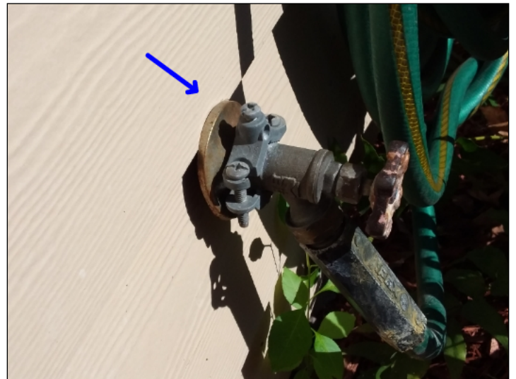
Bonding was noted on the water line.
