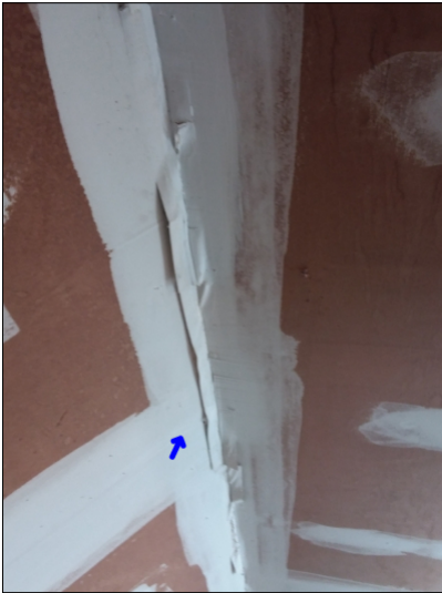
-The drywall tape is loose. This is often due to higher humidity or improper installation. Mainly at -garage
