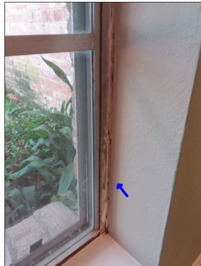
-Sealant is needed around the interior of the windows between the window framing and the drywall to help prevent water penetration. Mainly at -dining room
