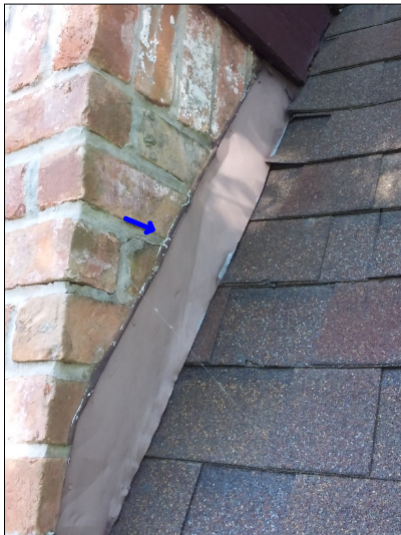
-The flashing needs to be sealed. Recommend repairs to help prevent water penetration. Mainly at -front
