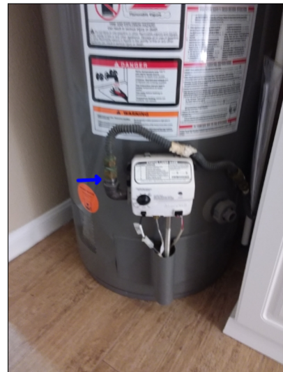
-No drip leg or sediment trap for gas line on water heater. This helps prevent trash from clogging jets.
