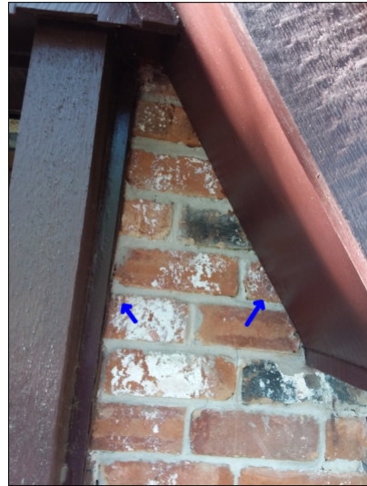
-Recommend sealing between the trim and brickwork to help prevent water penetration. Mainly at -front
