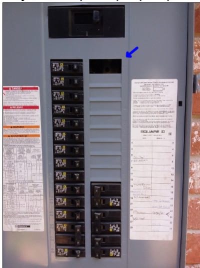
-There is at least one filler plate missing on the main electrical panel cover. Recommend adding missing filler plates to help prevent electrical shock.
