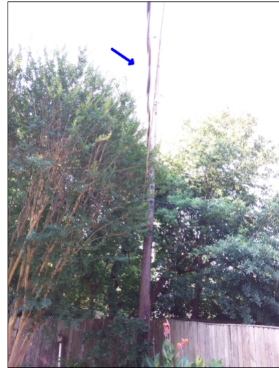
-Electrical feeds were running through the trees, recommend trimming limbs from wires.
