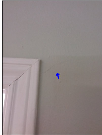
-Settlement cracks were noted in the drywall. Mainly at -game room
