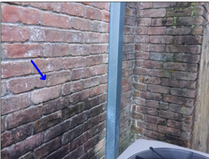
-There are signs of growth on exterior siding, recommend cleaning.
