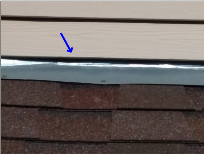
-Recommend painting all unpainted vents and flashings to help prevent damage due to UV rays or rust.
