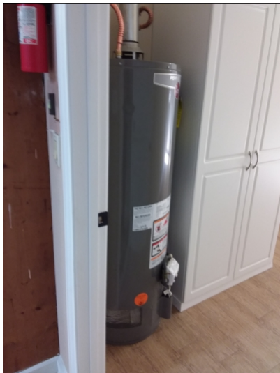
Overview of water heater(s)
