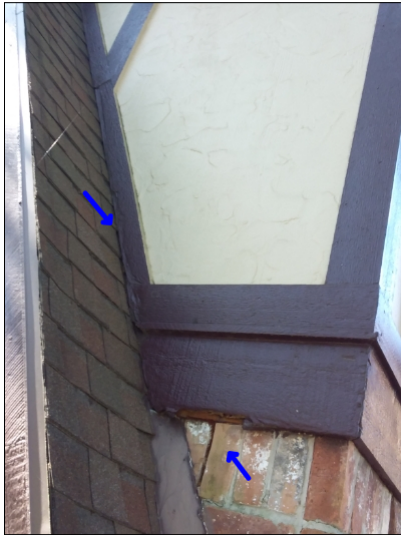
-Deterioration was noted at the trim, recommend replacing all deteriorated trim. Unable to determine the condition of the underlying materials. Mainly at -front
