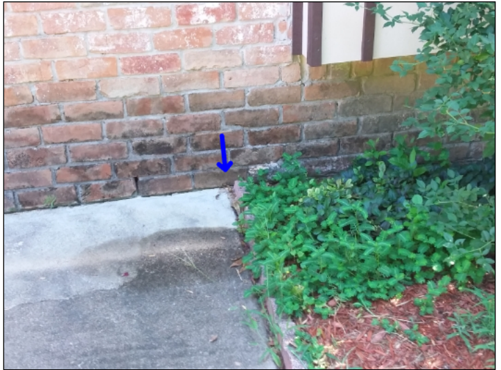
-The soil or rock level around the home is higher than recommended or in contact with the siding materials. Recommend lowering the soil line to help prevent water penetration and/or damage to the structure. Mainly at -rear
