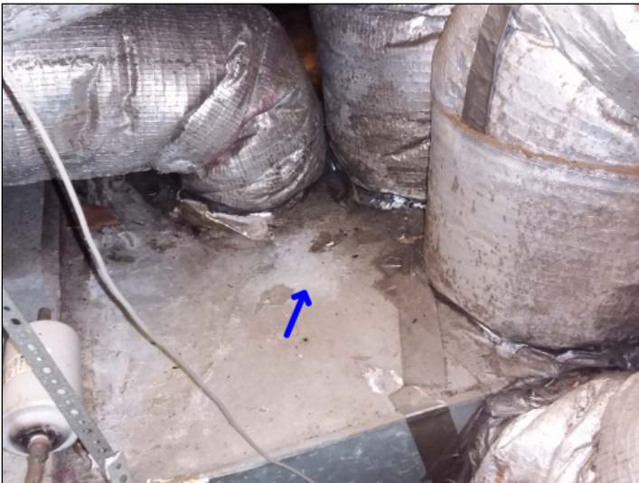
-There is a microbial growth noted at the plenum and/or evaporator. This is often caused by a conditioned air leak causing condensation and microbial growth, recommend sealing all air leaks and cleaning all surfaces.
