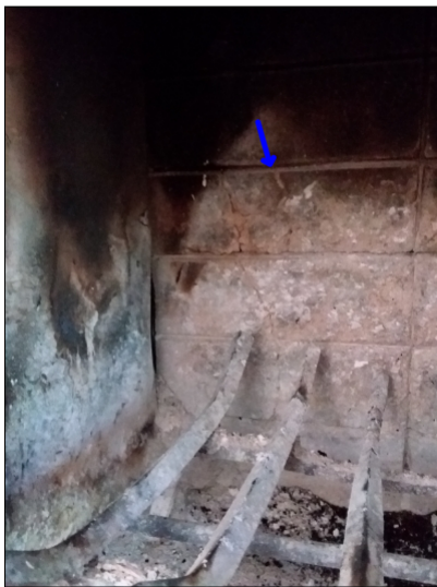
-The mortar in the fire box is deteriorating, recommend repairs.
