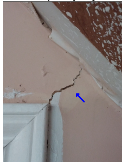
-Settlement cracks were noted in the drywall. Mainly at -garage
