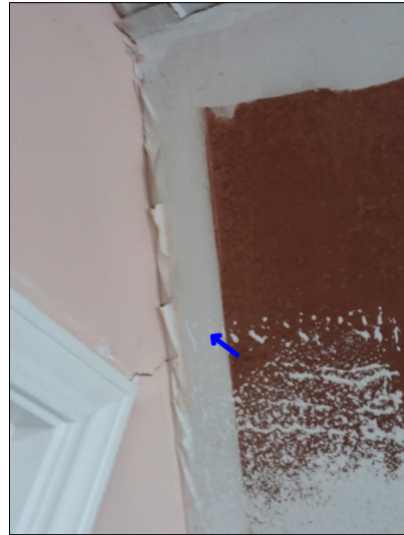
-Tape is twisting due to movement in the corners of the drywall, this is normally a sign of foundation movement or structural settlement, other movement noted may give signs of the cause. Mainly at - garage
