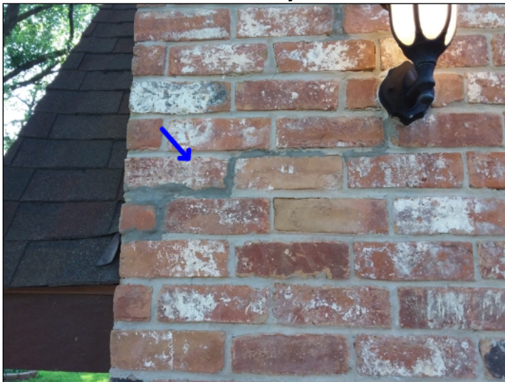
-There are signs of previous repairs in the brickwork. Mainly at -front
