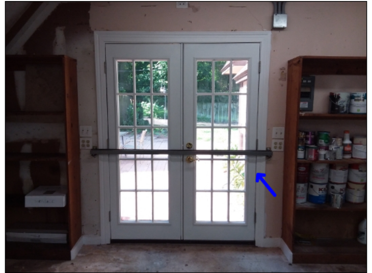
-The double doors door has been sealed off. Mainly at -garage
