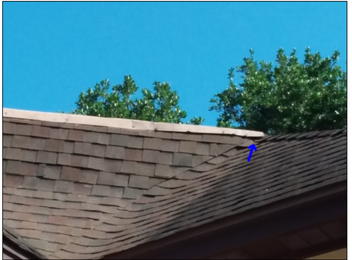
-The roof flashing is lifted. Recommend securing all loose or lifted flashings and sealing nails to help prevent water penetration. Mainly at - rear
