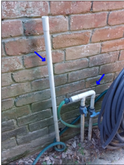
-Recommend painting all exposed plastic pipe to prevent premature deterioration from UV rays.
