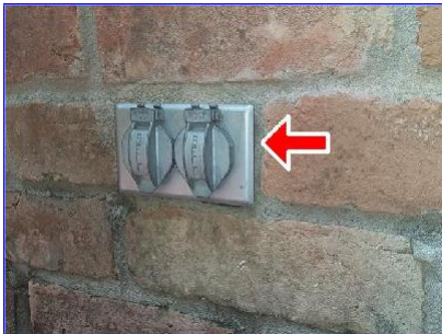
L. Item 3(Picture) multiple areas exterior outlets, lighting and service panels
