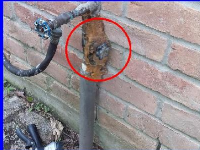
water shutoff right side of home
