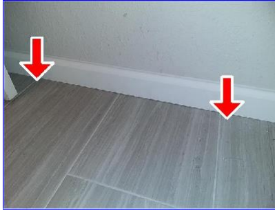
L. Item 2(Picture) multiple areas where flooring meets baseboards or door jambs
