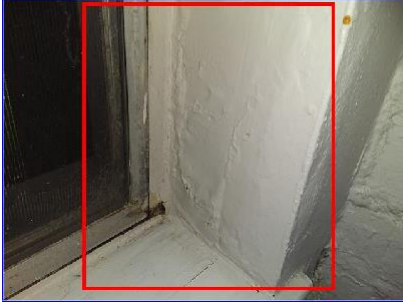
E. Item 1(Picture) living room window areas
