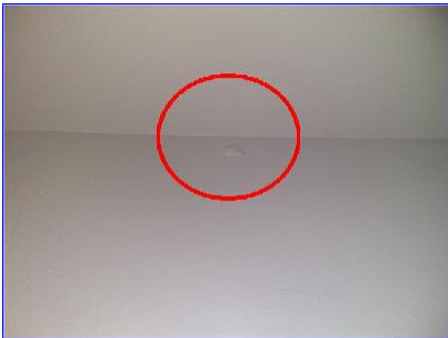
E. Item 3(Picture) multiple areas right side bedroom
