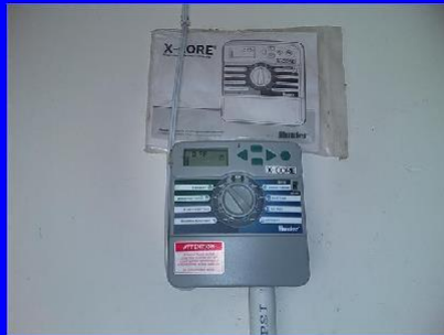
sprinkler system control panel inside garage
