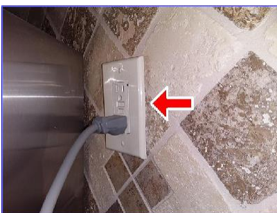
B. Item 9(Picture) most if not all rooms
