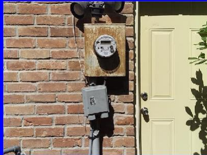
meter box left side of home underground service
