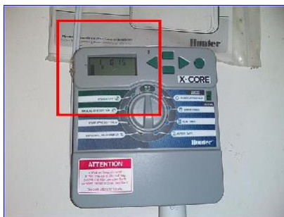
A. Item 1(Picture) zone 1 did not activate
