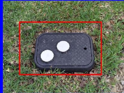
water meter front right of home
