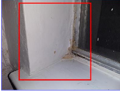
E. Item 2(Picture) living room window areas
