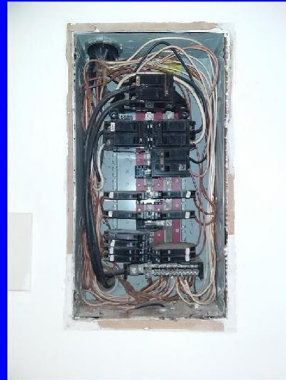
breaker box inside garage 100 amp
