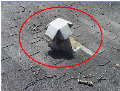
C. Item 5(Picture) furnace and water heater
