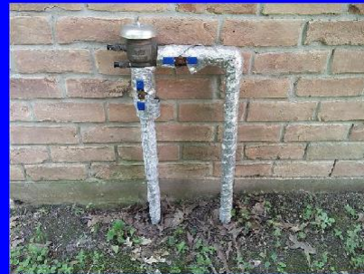
backflow preventer right side of home
