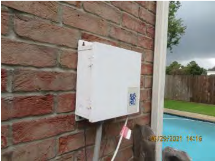
Pool control panel noted. Observational an informational purpose only.
