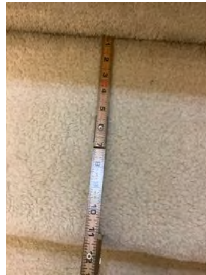
Stairs tread measurement was a normal range at time of inspection. Observational an informational purposes only
