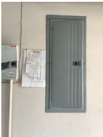
Siemens electrical panel noted in garage at time of inspection. Observational an informational purposes only
