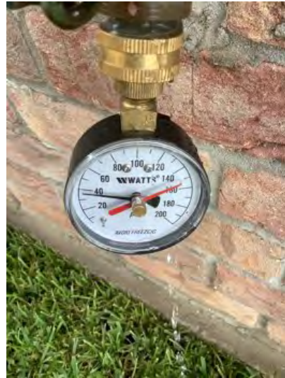
Static water pressure noted at time of inspection. Observational and informational purposes only. Was a normal range noted.
