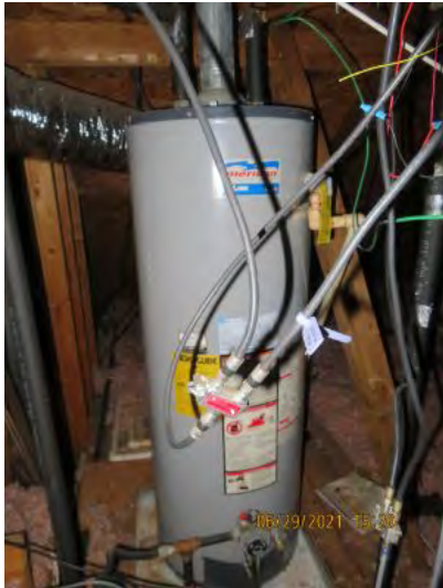
View of water heater noted. Observational an informational purpose only. 2001 Gas 50 Gallon Unit.
