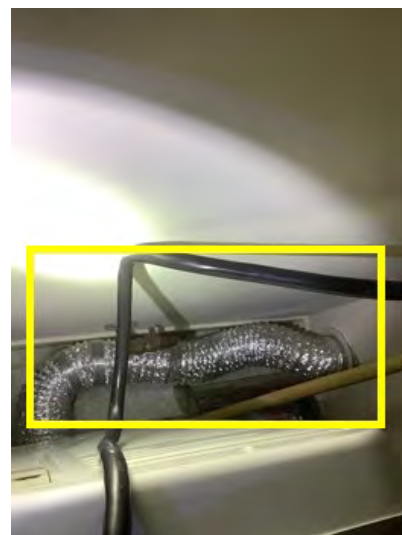
Dryer exhaust noted at time of inspection.
