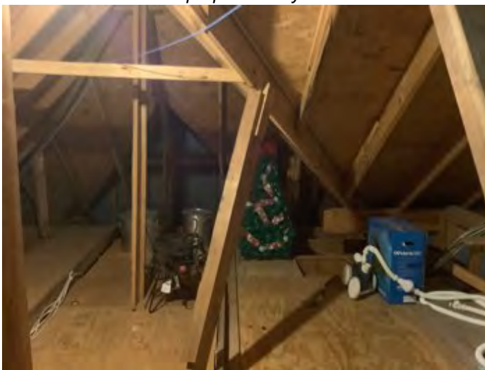
Attic storage area noted in second-floor bedroom right side door access to storage area of attic noted. Observational informational purposes only.
