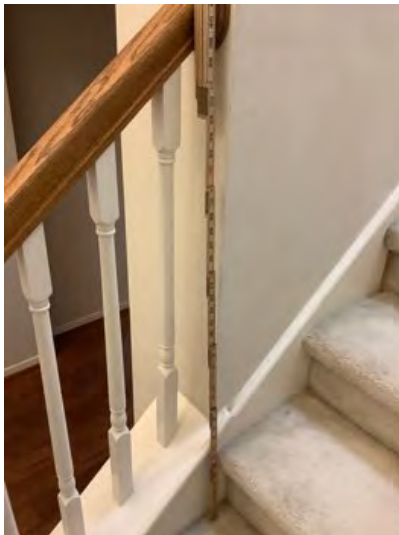
Stairs handrail height was in normal range at time of inspection. Observational and informational purposes only
