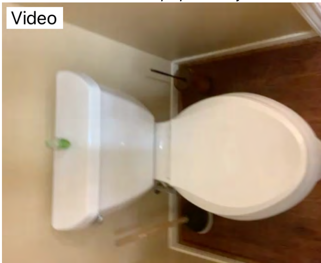
First floor Half bathroom toilet tank is slightly loose recommend taking the very least almost intrusion with damage.
