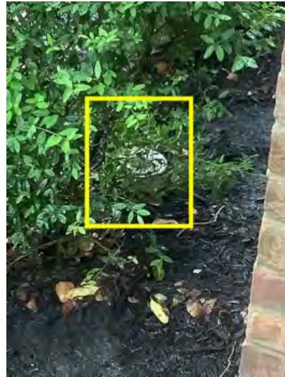
Main sewer clean out noted at time of inspection. Observational an informational purposes only.
