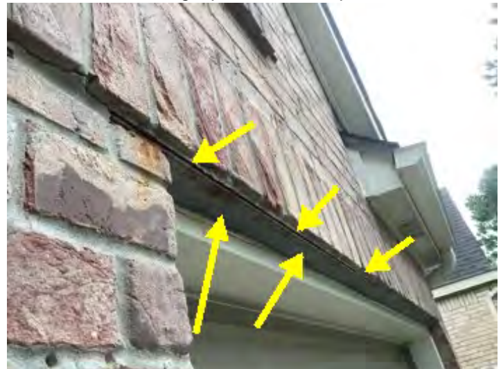
All metal lintels above garage and windows should be sanded caulked sealed and painted properly. Conducive to moisture intrusion, damage and potential WDO. Recommend having a professional inspect and correct
