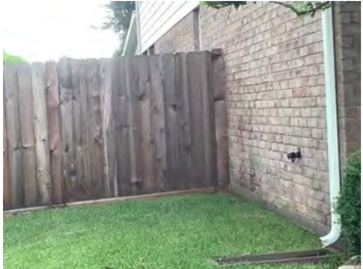
6 foot wooden fence noted at time of inspection. Observational an informational purposes only.
