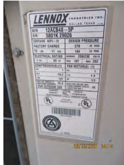
Lennox Unit # 2 HVAC exterior condenser, 4 Ton, R22 Freon, 2001 MFD, 45 AMP 12 SEER. Unit was working but appears to be at the end of its life expectancy.
