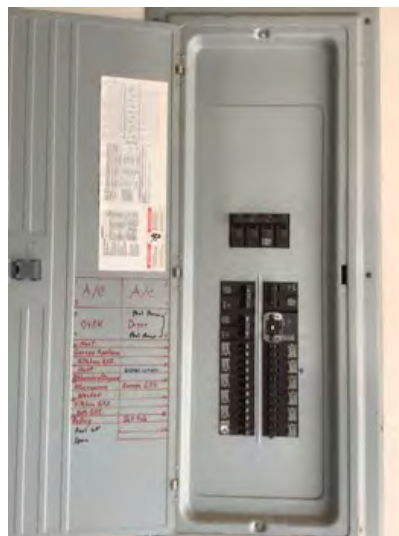
Interior view of electrical panel noted at time of inspection unit was properly labeled. Observational an informational purposes only
