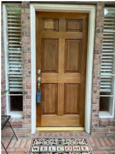
Wood fire rated front door noted at time of inspection. Observational an informational purposes only
