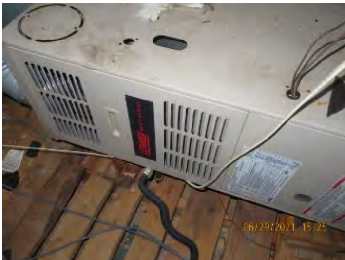
View of Gas heating (Furnace) noted. Unit not tested due to exterior temperature is above 90 degrees. Observational an informational purpose only.
