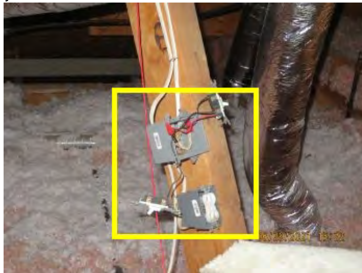
Exposed wiring in attic and outlets / receptacles missing cover plates noted. Potential hazard and recommend having a professional inspect and correct.
