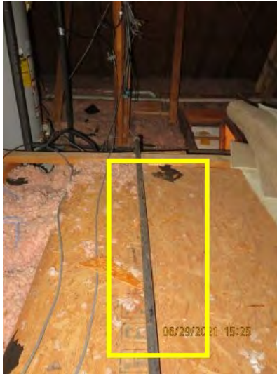
Black iron gas pipe plumbing noted. Observational an informational purpose only.
