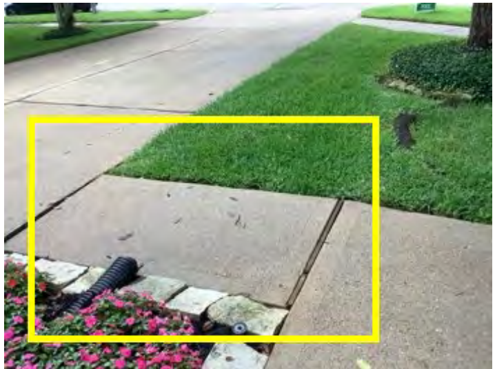
Slight bulging and heaving noted in concrete sidewalk due to expose root system from tree in front yard. Recommend having all three routes corrected by a professional.
