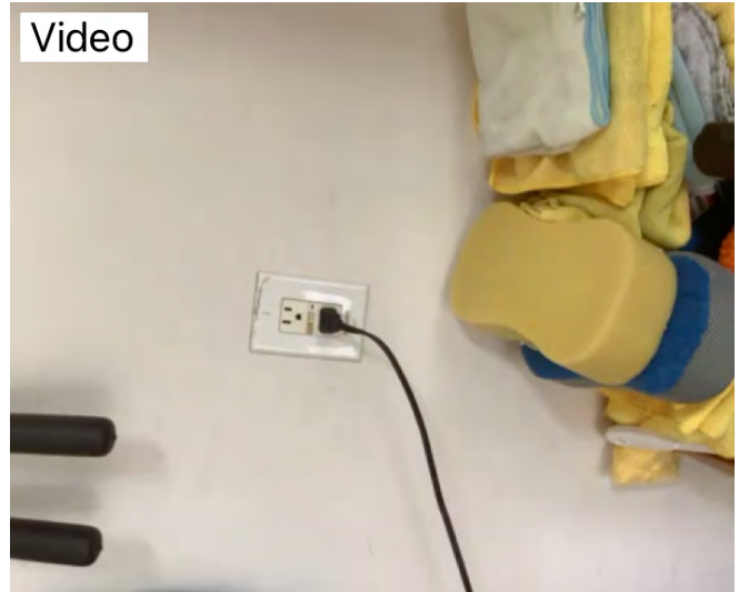
Video of GFCI in garage properly labeled and working properly at time of inspection. Observational an informational purposes only.
