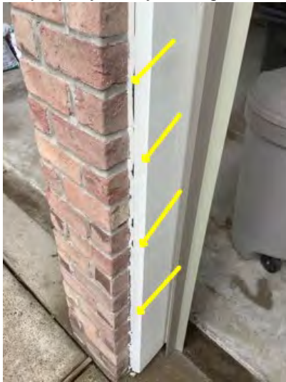
Expose penetrations on wall systems around garage should be sealed caulked and painted properly conducive to moisture intrusion, damage a potential WDO. Recommend getting a professional to expect and correct
