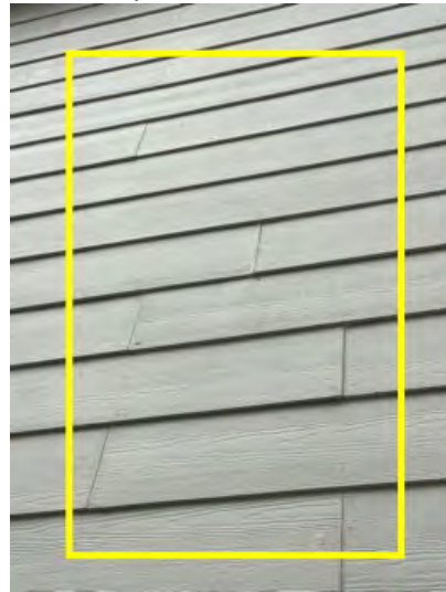
All exterior siding penetrations and seems should be sealed, caulked and painted properly. Conducive to moisture intrusion, damage and potential WDO. Recommend having a professional inspect and correct.
