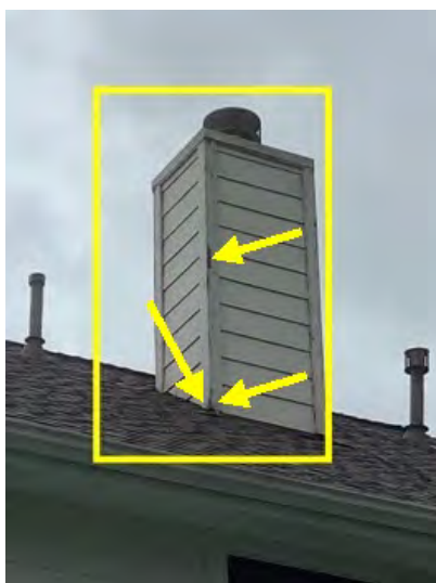
Chimney noted at time of inspection. Recommend all trim boards and siding be sealed caulked and painted properly some trim boards may need to be replaced.
