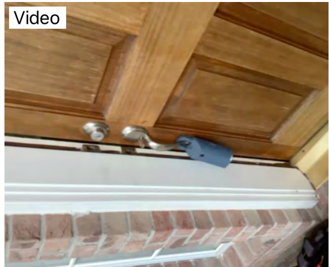
Front door not closing properly at time of inspection noted. Observational an informational purpose only.
