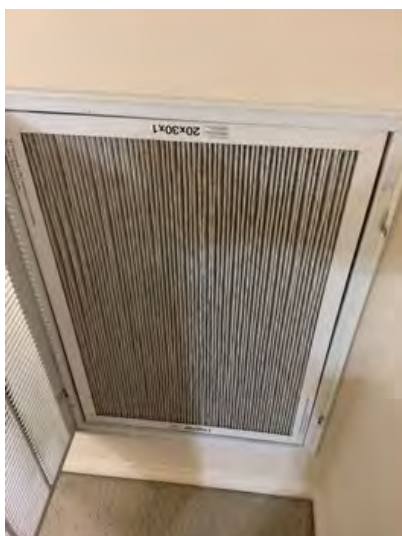
20x30x1 filter size noted. Observational an informational purpose only.
