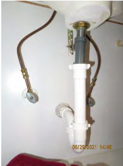
Cooper plumbing supply and PVC drains under sink noted. Observational an informational purpose only.
