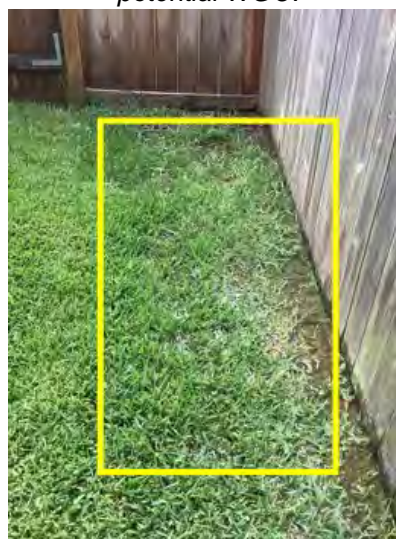
Ponding water noted on the left side of structure by fence at time of inspection. No gutters noted on that side of house. Recommend replacing or adding gutters to assist and proper drainage efficiency.
