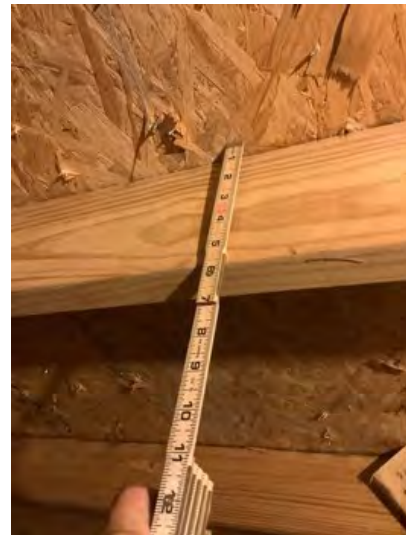
2 x 6 rafters noted at time of inspection. Observational an informational purposes only.
