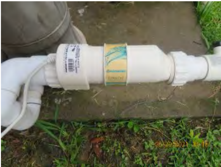
Pool components noted. Observational an informational purpose only.
