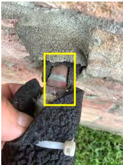
Copper plumbing supply noted at time of inspection. Observational an informational purposes only.
