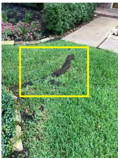
Tree roots are noted in front yard potential trip hazard recommend having a professional remove all routes that are exposed
