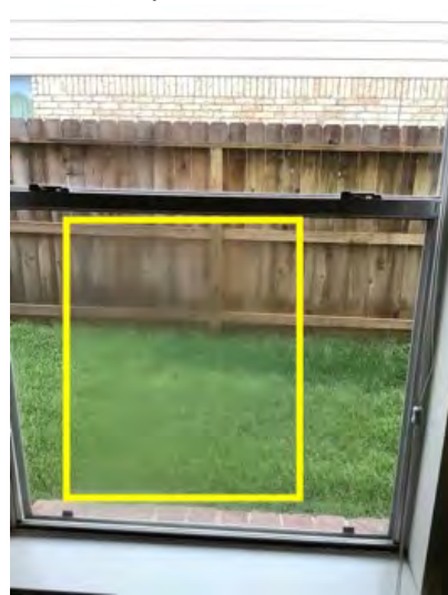
View of Haze / condensation between windows noted at time of inspection these are original as built aluminum windows noted.
