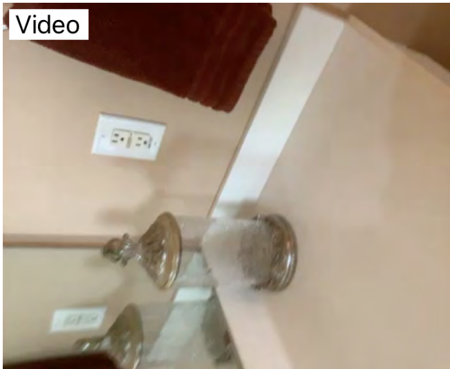
GFCI in master bathroom by the toilet is working properly at time of inspection. Observational informational purposes only.
