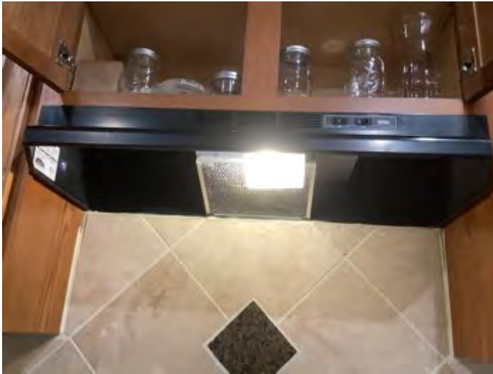
Broan brand Range hood noted at time of inspection was working properly. Observational an informational purposes only.
