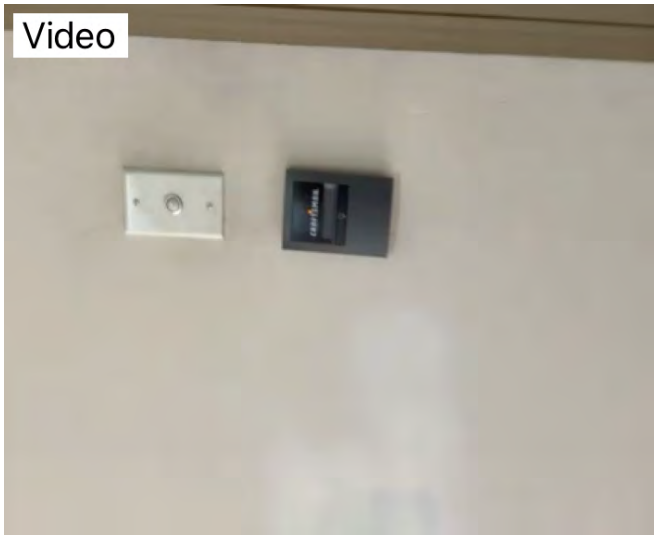
Video garage doors working properly an automatic back up sensors were working. Observational purposes only
