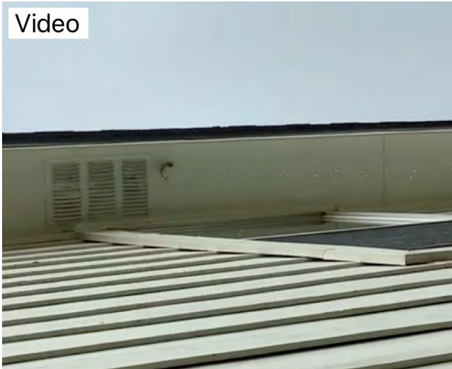
Secondary drain noted on right side of house underneath soffit he's draining at time of inspection. Conducive to main drain needing to be cleaned out. Recommend having a professional inspect incorrect problem
