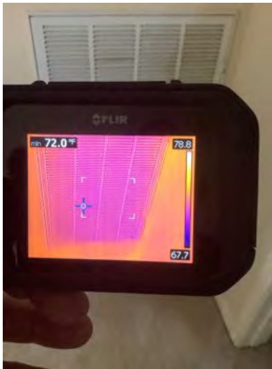
72° temperature reading on second floor return vent in wall located at top of stairs noted. Observational an informational purposes only.
