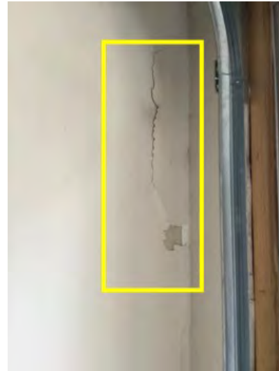
View of wall in garage by the door with paint peeling off noted. Recommend having a professional inspected
