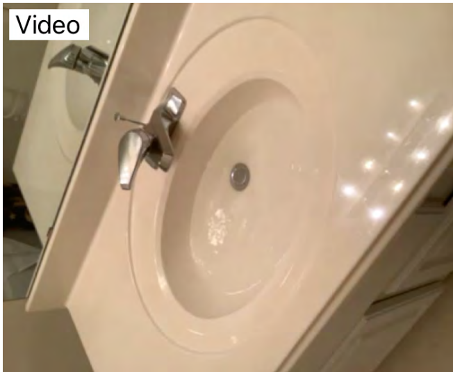
Second-floor guest bathroom right side Drain test on sink and tub or working properly. Observational an informational purposes only.
