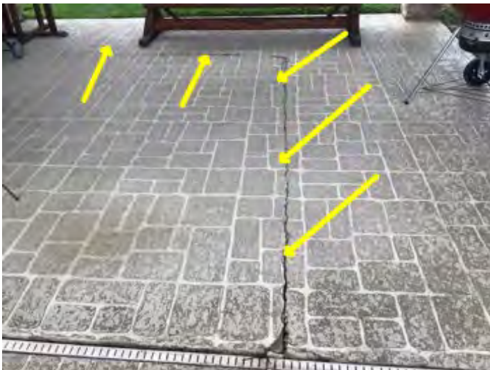
Cracking noted on back patio at time of inspection. Recommend having a professional inspected correct potential trip hazard conducive a moisture intrusion, shifting expansion and contraction potential.
