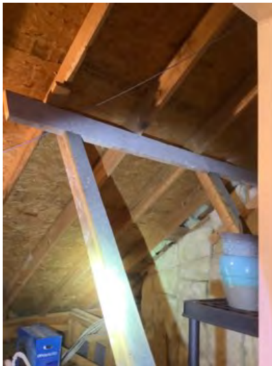
Attic structure consist of rafters, purlins and kicker support noted at time of inspection. Observational an informational purposes only.
