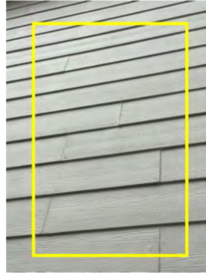
All exterior siding penetrations and seems should be sealed, caulked and painted properly. Conducive to moisture intrusion, damage and potential WDO. Recommend having a professional inspect and correct.
