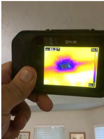
Second floor living room 61.2 slightly higher than normal temperature reading.
