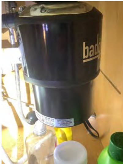
Badger food disposal noted at time of inspection. Observational an informational purposes only
