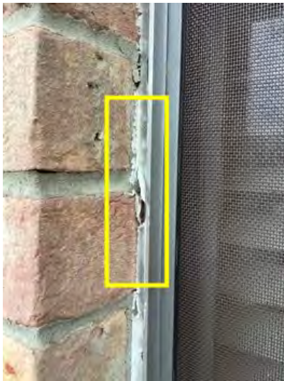
All expose window penetrations should be sealed caulked properly conducive to moisture intrusion damage of potential WDO.
