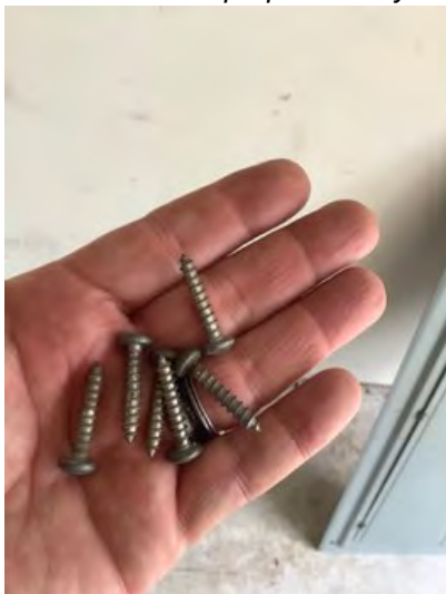
Metal screws utilized instead of proper electrical screws. Conducive to electrical hazards and issues. Recommend replacing with proper screws.
