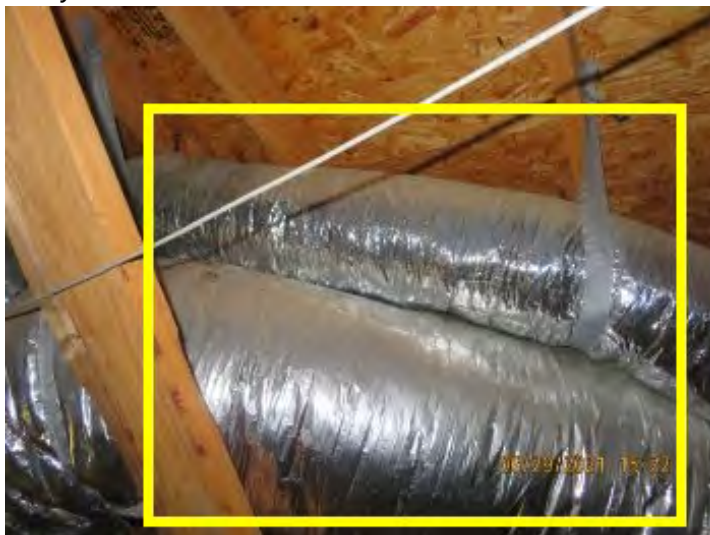
All HVAC ducts should not touch one another and be properly hung. Conducive to moisture intrusion, damage and potential WDO
