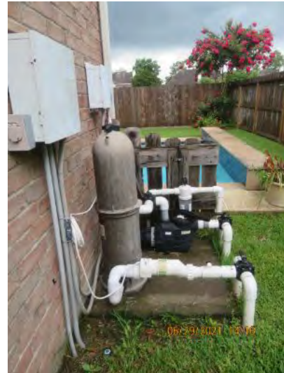
Pool equipment was working properly at time of inspection. Observational an informational purpose only.
