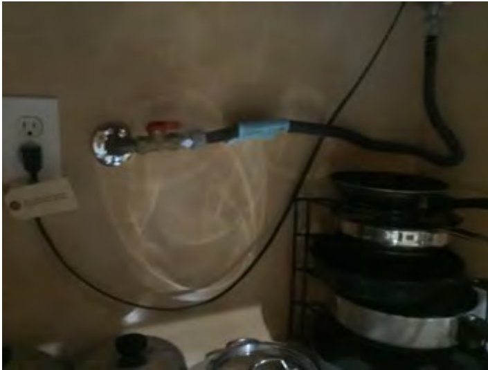
Gas cooktop flex line gas valve noted underneath unit in cabinetry. Observational an informational purposes only.
