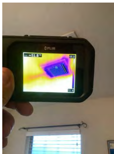
51.8° temperature reading on supply vent and second floor left bedroom noted in normal range. Observational an informational purposes only.
