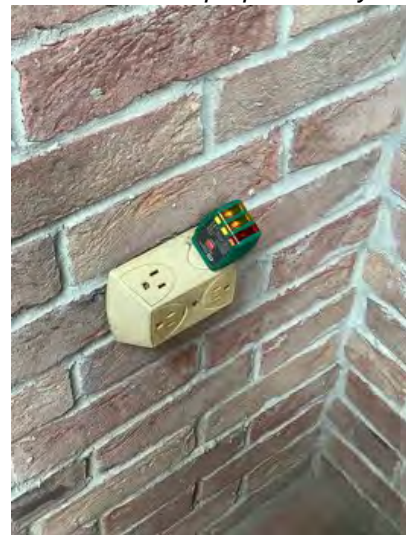
Electrical outlet by front door was working properly at time of inspection. Observational an informational purposes only.
