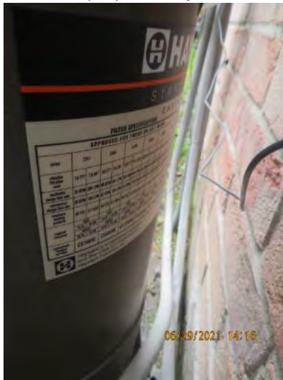
Filter manufacture label noted with limited access at time of inspection. Observational an informational purpose only.
