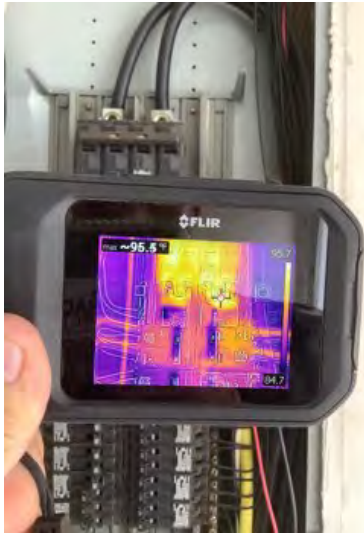
Thermal imaging temperature reading on upper area of panel noted at time of inspection. Observational an informational purposes only
