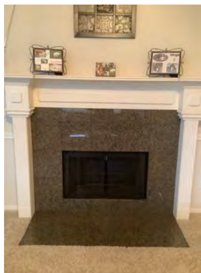
Gas fireplace noted at time of inspection. Observational an informational purposes only.
