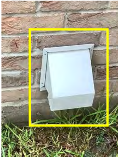
Dryer vent noted on exterior at time of inspection. Observational and informational purposes only.
