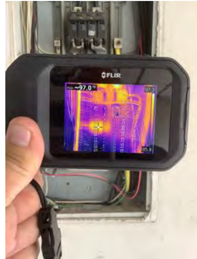
Thermal imaging temperature reading on lower area of electrical panel noted. Observational an informational purposes
