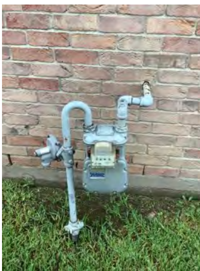
Main gas meter located on the right side of the property at time of inspection. Observational information purposes
