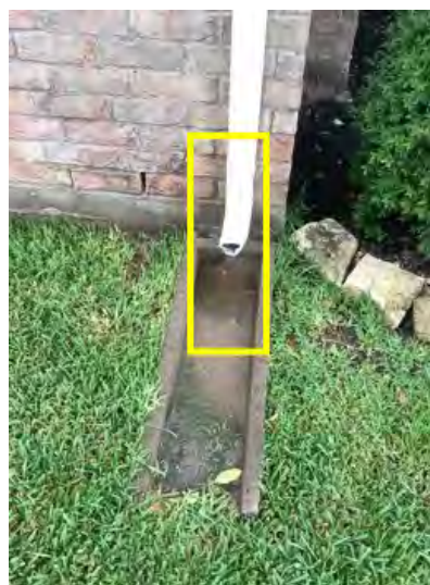
All gutters to disperse water 5 to 6 feet away from foundation. Conducive to moisture intrusion, damage and potential WGO.
