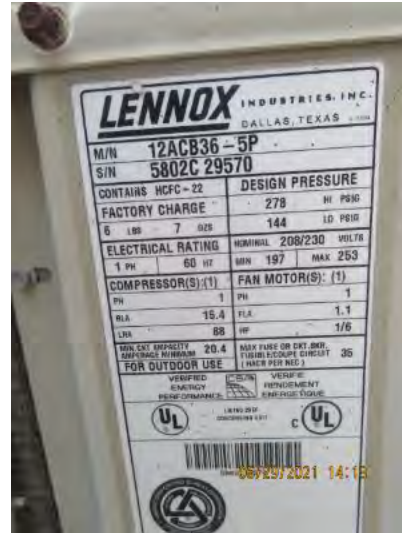
Lennox HVAC unit Manufacture label noted at time of inspection. Observational an informational purpose only.
