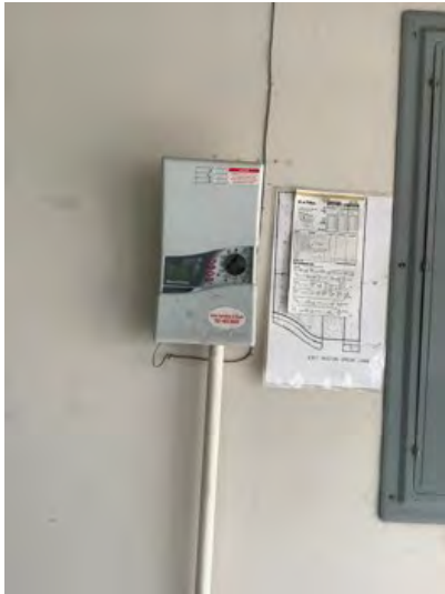
Rainbird control panel for automatic sprinkler system noted at time of inspection. Unit was not working properly.
