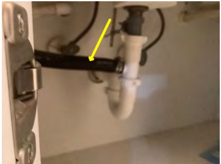
Main condensation drain noted under sink and guest bathroom at time of inspection. Observational an informational
