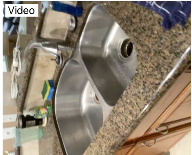
GFCI outlet located by kitchen sink while working properly recommend labeling has recommended
