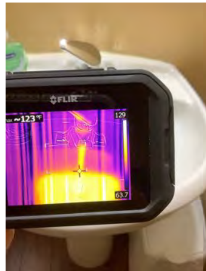
Hot water temperature reading on first floor half bathroom was in normal range. Observational an informational purposes only.
