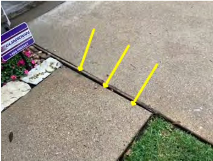
Slight deflection noted by sidewalk into front door at time of inspection. Inspectors opinion is exposed route from tree is shifting the concrete sidewalk in this area noted.
