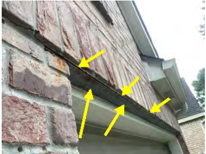
All metal lintils above garage and windows should be sanded caulked sealed and painted properly. Conducive to moisture intrusion, damage and potential WDO. Recommend having a professional inspect and correct
