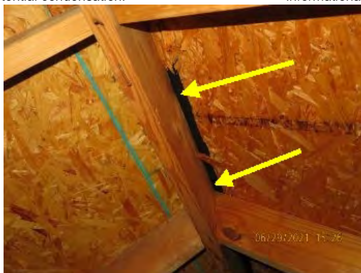
Small ridge vent noted at time of inspection. Observational an informational purpose only.
