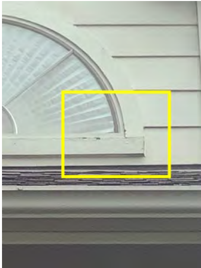
Wall systems trim and siding noted by dormer window front of house that showed signs of moisture intrusion and damage would recommend having all areas sealed caulked and painted properly in any damage wood replaced.
