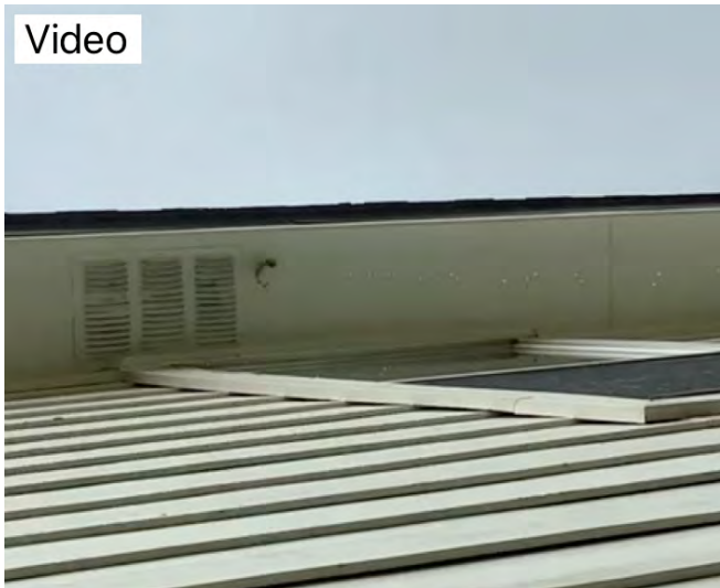
Secondary drain noted on right side of house underneath soffit he's draining at time of inspection. Conducive to main drain needing to be cleaned out. Recommend having a professional inspect incorrect problem
