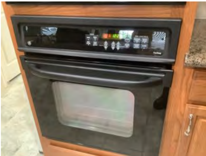
Electric GE oven noted at time of inspection. Observational an informational purposes
