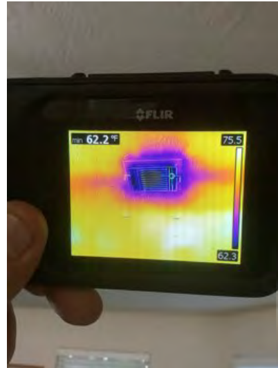
62.2° second floor living room supply vent noted at time of inspection. Observational an informational purposes
