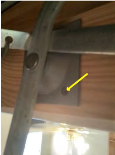
Attic ladder was missing hardware in fasteners to secure to framing recommend having a professional inspection correct potential fall hazard or damage
