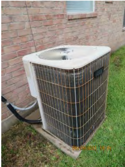
Lennox unit appears to be at end of its life expectancy noted. 3 Ton, R22 Freon, 35 Amp Max, 12 SEER, 2002 MFD. Recommend having unit inspected by a professional for over all life expectancy. Unit was operating at time of inspection but is an 18 year old unit.
