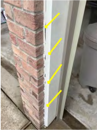
Expose penetrations on wall systems around garage should be sealed caulked and painted properly conducive to moisture intrusion, damage a potential WDO. Recommend getting a professional to expect and correc
