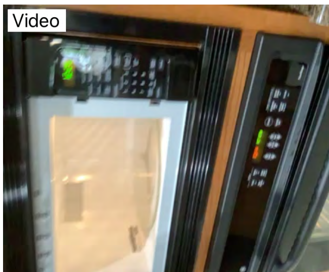
Video of microwave working properly at time of inspection. Observational an informational purposes only.
