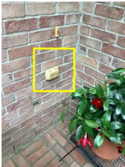
Electrical outlet by front door needs to have bubble cover to protect. Recommend have a professional inspect and install.
