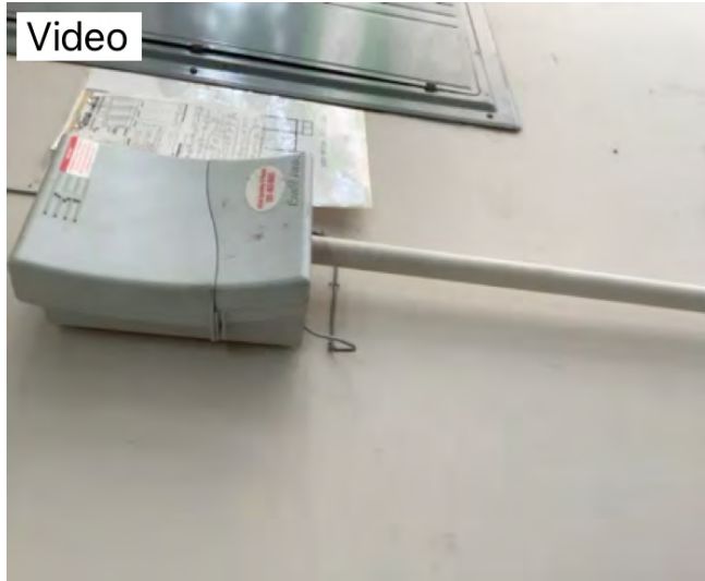
Panel for sprinkler should be secured properly at time of inspection. Observational an informational purposes only.
