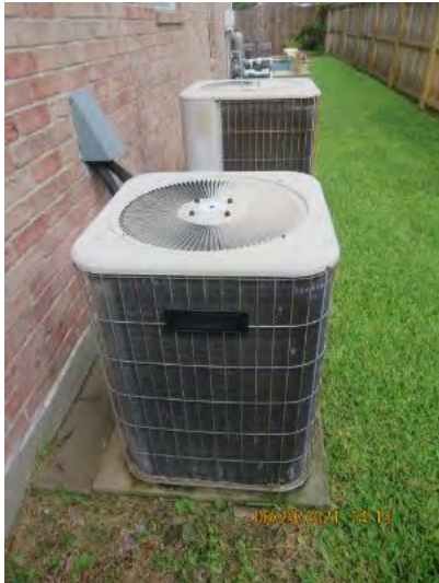
Two (2) HVAC exterior condensing units noted at time of inspection. Observational an informational purpose only.
