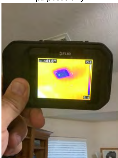
61° temperature reading second floor living room noted at time of inspection. Observational an informational purposes only
