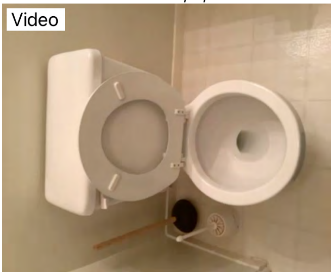
Second-floor guest bathroom right side toilet was flushing properly. Observational an informational purposes only
