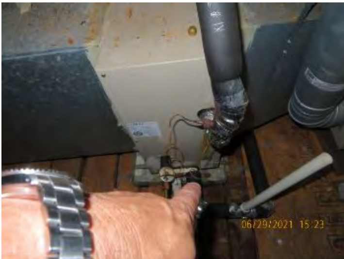
Missing float switch noted. Recommend having one added for proactive protection in case drain pan gets full of water "Float Switch" Will shut off system for protection from moisture damage and intrusion from drain pan potentially overflowing.
