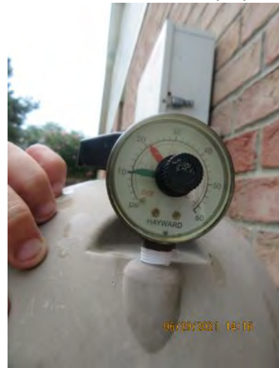
Pool filter reading noted. Observational an informational purpose only.
