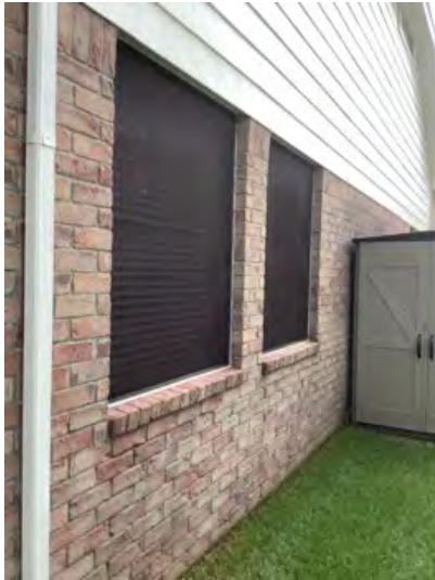
Limited inspection on exterior windows do the solar screens noted at time of inspection. Observational an informational purposes only.
