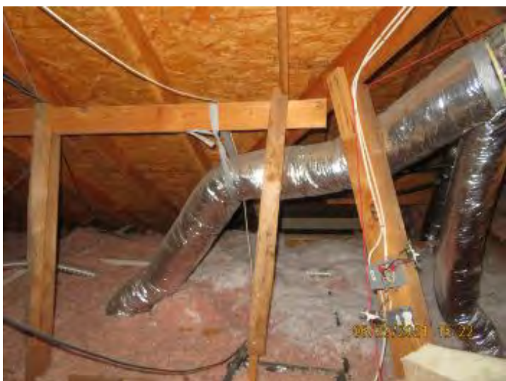
View of attic structure construction methods noted with Rafters, Purlin and Kicker support. Observational an informational purpose only.
