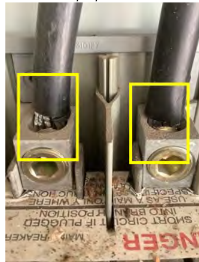
All aluminum main connector should have antioxidant jell for protective purposes. Recommend having a professional inspect and add.
