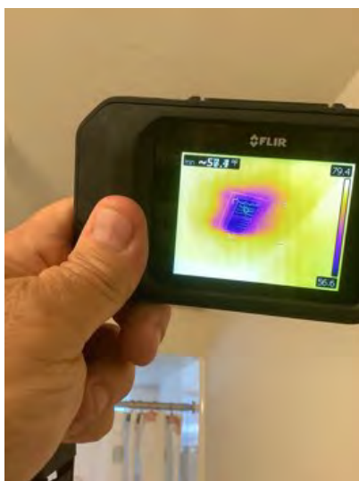
57° second-floor guest bathroom supplied meant noted at time of inspection. Observational and informational purposes only
