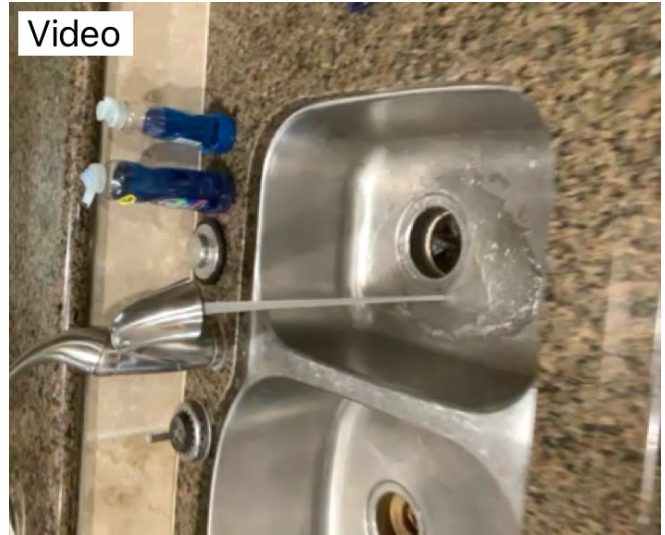
Kitchen faucet sprayer was working properly at time of inspection. Observational an informational purposes only.
