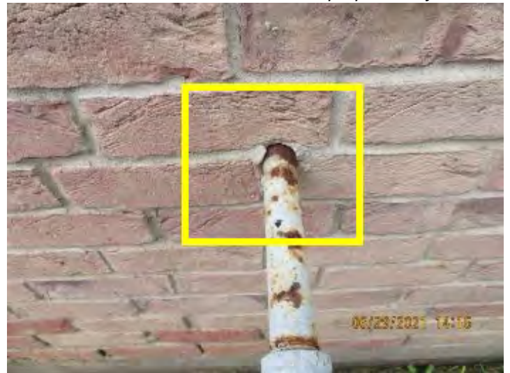
Galvanized plumbing at gas meter penetration into wall systems should be sealed properly. Conductive to moisture intrusion, damage and potential WDO.
