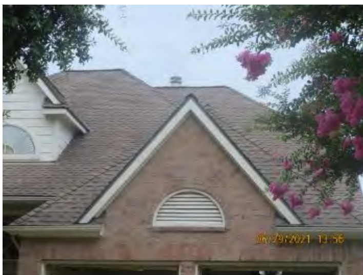
Front of roof noted. Observational an informational purpose only.
