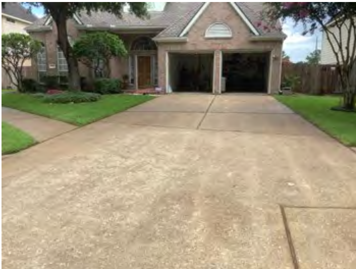
Concrete driveways and sidewalks noted at time of inspection. Observational an informational purposes only.
