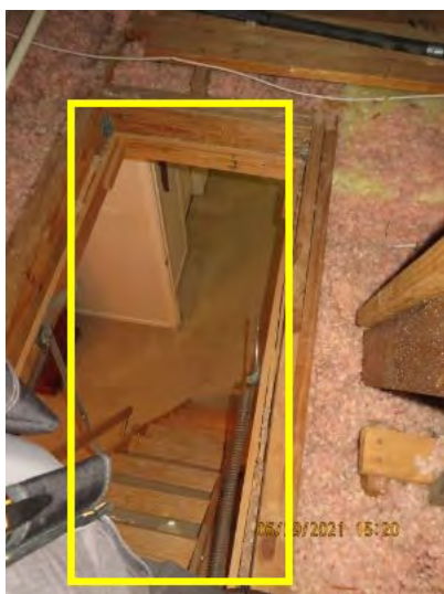
Attic ladder scuttle hole is recommended to be sealed and caulked properly. Conducive to air leaks from attic into livable space and potential condensation.
