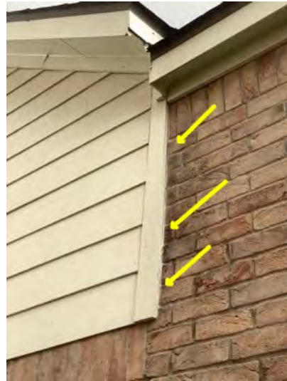
All exterior siding transition seems between brick and hardy plank siding seems need to be caulked sealed and painted properly conducive to moisture intrusion, damage and potential WDO
