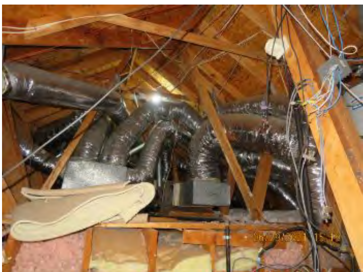
View of HVAC ducts noted in attic area at time of inspection noted. Observational an informational purpose only.
