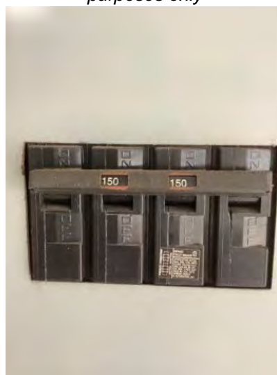
150 amp main breaker noted at time of inspection. Observational an informational purposes only
