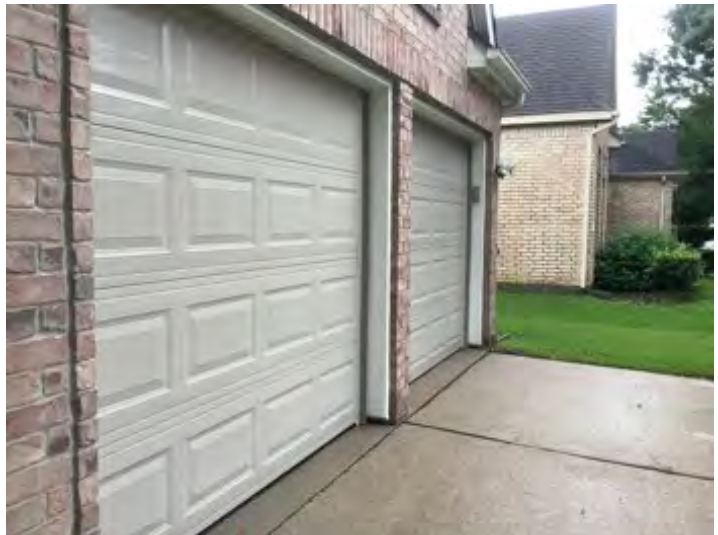
Two aluminum metal garage doors noted at time of inspection. Observational an informational purposes only
