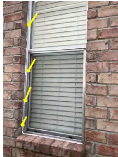
Aluminum original as built windows noted at time of inspection. Recommend ceiling all penetrations with proper caulking. Conducive to moisture intrusion, damage and potential WDO. Recommend having a professional inspected correct.
