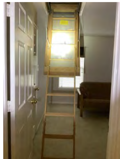
Attic ladder noted on second floor 250 pounds max rating cover was insulated. Observational an informational purposes only. 2001 manufacture date noted.
