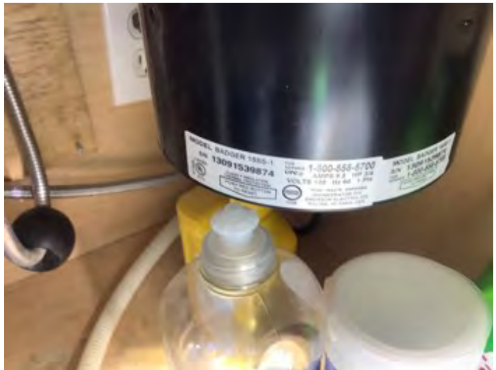
Badger food disposal manufacturers label noted at time of inspection. Observational an informational purposes only
