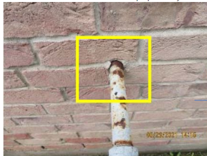
Galvanized plumbing at gas meter penetration into wall systems should be sealed properly. Conducive to moisture intrusion, damage and potential WDO.
