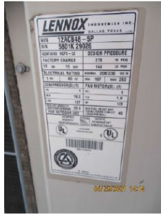
Lennox Unit # 2 HVAC exterior condensor, 4 Ton, R22 Freon, 2001 MFD, 45 AMP 12 SEER. Unit was working but appears to be at the end of its life expectancy.
