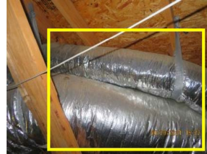
All HVAC ducts should not touch one another and be properly hung. Conducive to moisture intrusion, damage and potential WDO
