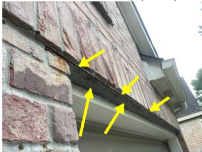
All metal lintels above garage and windows should be sanded caulked sealed and painted properly. Conducive to moisture intrusion, damage and potential WDO. Recommend having a professional inspect and correct
