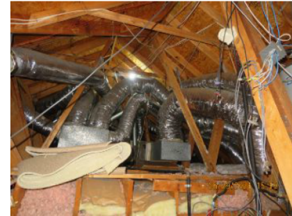
View of HVAC ducts noted in attic area at time of inspection noted. Observational an informational purpose only.
