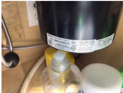
Badger food disposal manufacturers label noted at time of inspection. Observational an informational purposes only
