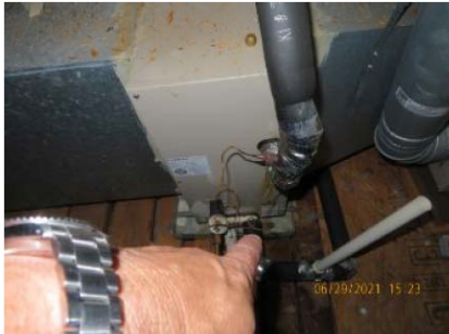
Missing float switch noted. Recommend having one added for proactive protection in case drain pan gets full of water "Float Switch" Will shut off system for protection from moisture damage and intrusion from drain pan potentially overflowing.
