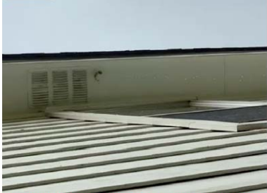
Secondary drain noted on right side of house underneath soffit he's draining at time of inspection. Conducive to main drain needing to be cleaned out. Recommend having a professional inspect incorrect problem
