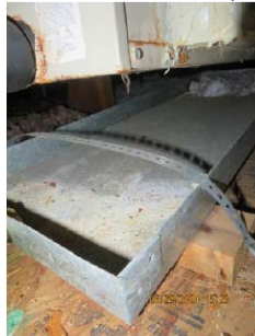
Interior view of drain pan noted. Observational an informational purpose only.
