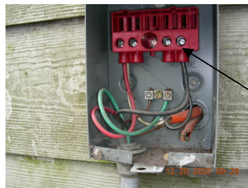
Unit A air conditioner circuit does not have a disconnect pullout
