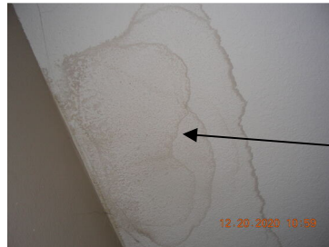
Water stained ceiling in Unit B
