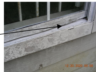
Exterior damage on rear window on unit B
