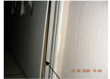
Damaged door skin on hallway door in unit B
