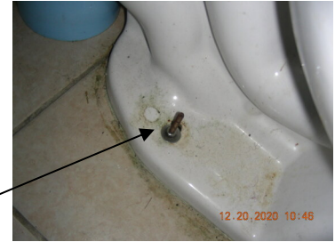
Missing toilet bolt caps on Unit B guest bath toilet
