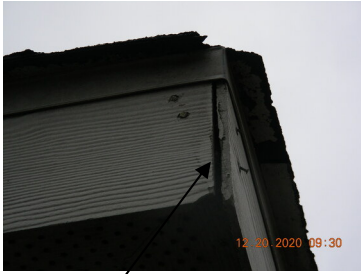
Example of damaged fascia board
