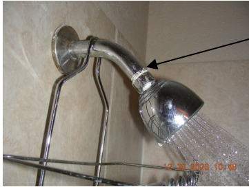
Water leak on Unit B guest bath showerhead
