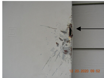
Damaged latch on unit B main electric panel
