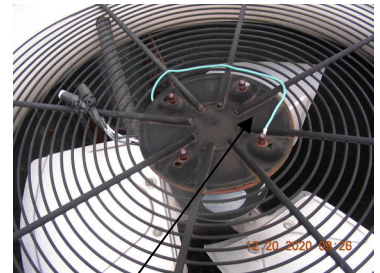
Exposed wire on Unit A condenser unit
