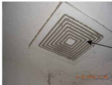
Unit A primary bath exhaust fan grill is filled with debris
