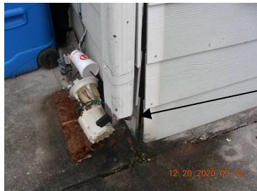
Examples of gutter downspouts that terminate too close to the wall and foundation
