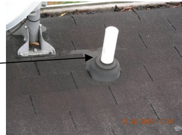
Example of PVC pipe in need of paint
