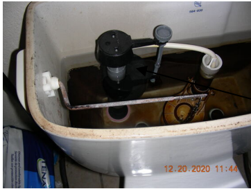
Unit A toilet fill valves are in need of replacement
