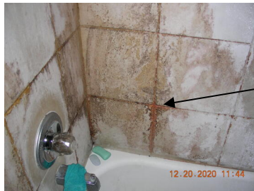
Damaged tile and mildew growth on shower wall in unit A's primary bath
