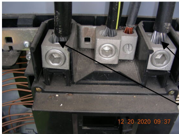
Main aluminum power lines need antioxidant coating
