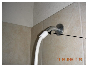
Water leak on Unit A guest bath showerhead
