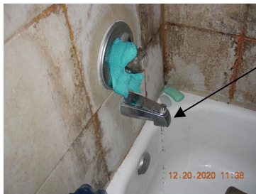
Unit B primary bathtub faucet leaks when the handle is turned to the off position
