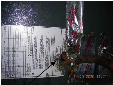
Refrigerant line is not sealed against evaporator box in unit A
