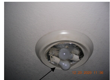
Missing globe on light fixture in unit A
