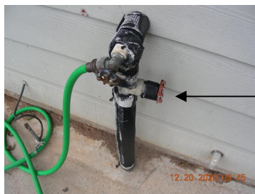
Main water shutoff valve for Unit B
