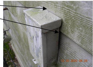
Sealant needed on top and sides of electric panels
